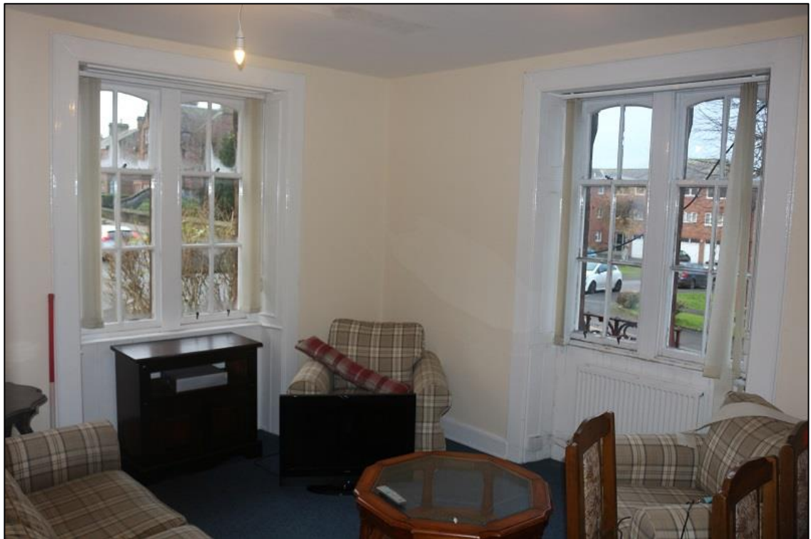
Figure 7b: Room NL3, Showing Absence of Cornice
