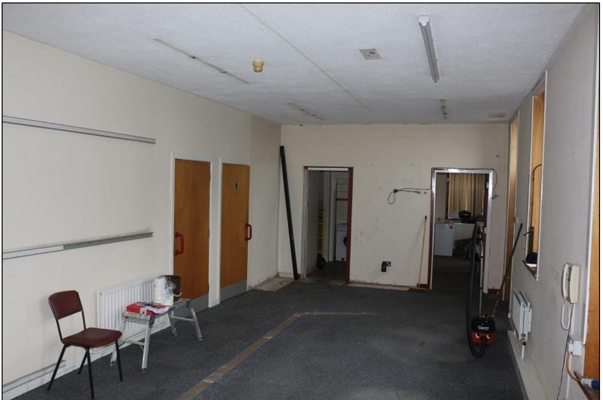
Figure 14b: Occupational Health Building – Interior of Room OH5, showing Original Internal S Wall
