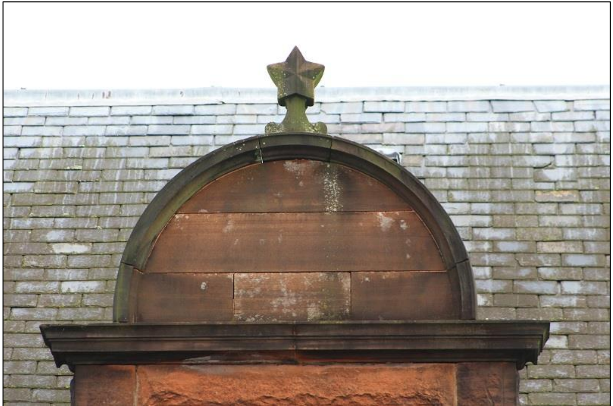
Figure 11b: Occupational Health building – W Elevation, Detail of Segmented Pedimented Gablet with Star Finial
