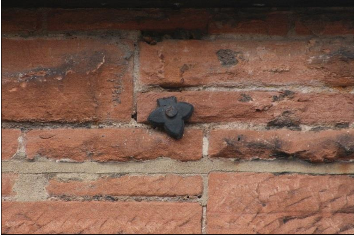
Figure 14a: Occupational Health Building – Cast Cross-Tie set at High Level, S End E Elevation
