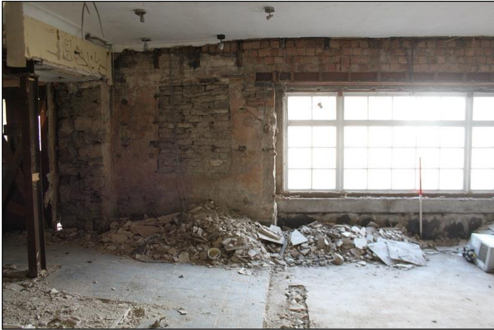
Figure 10a: Room q, Wider View, With Wall Return to LHS of Blocked Window
