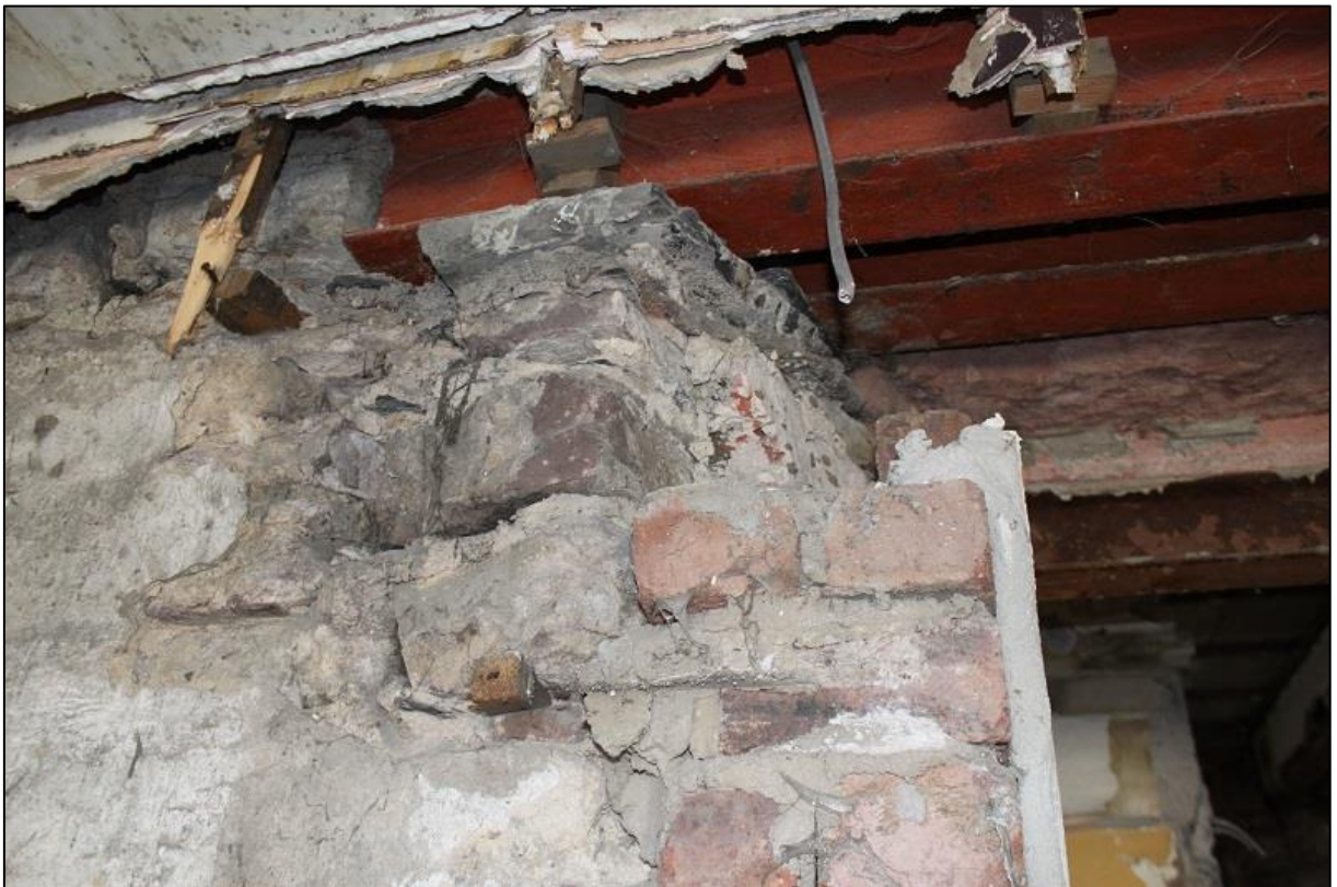
Figure 7b: Room j, Splayed Embrasure and Sandstone Lintel Over Opening in SW Wall
