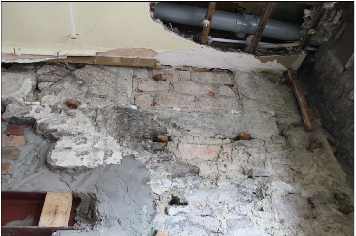
Figure 5b: Room g, NW Wall, Blocked Window at Original 1 st Floor Level
