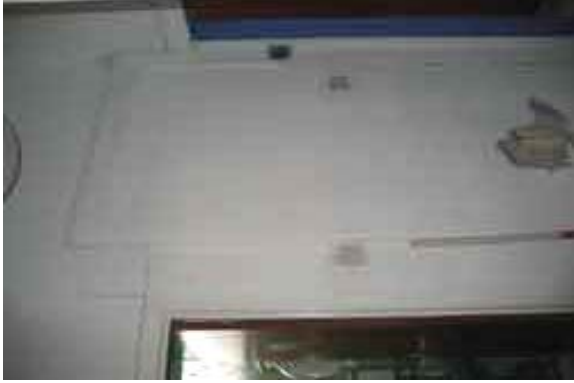
Figure 5a: Blocked Entrance, Flat 5 (1st Floor)
