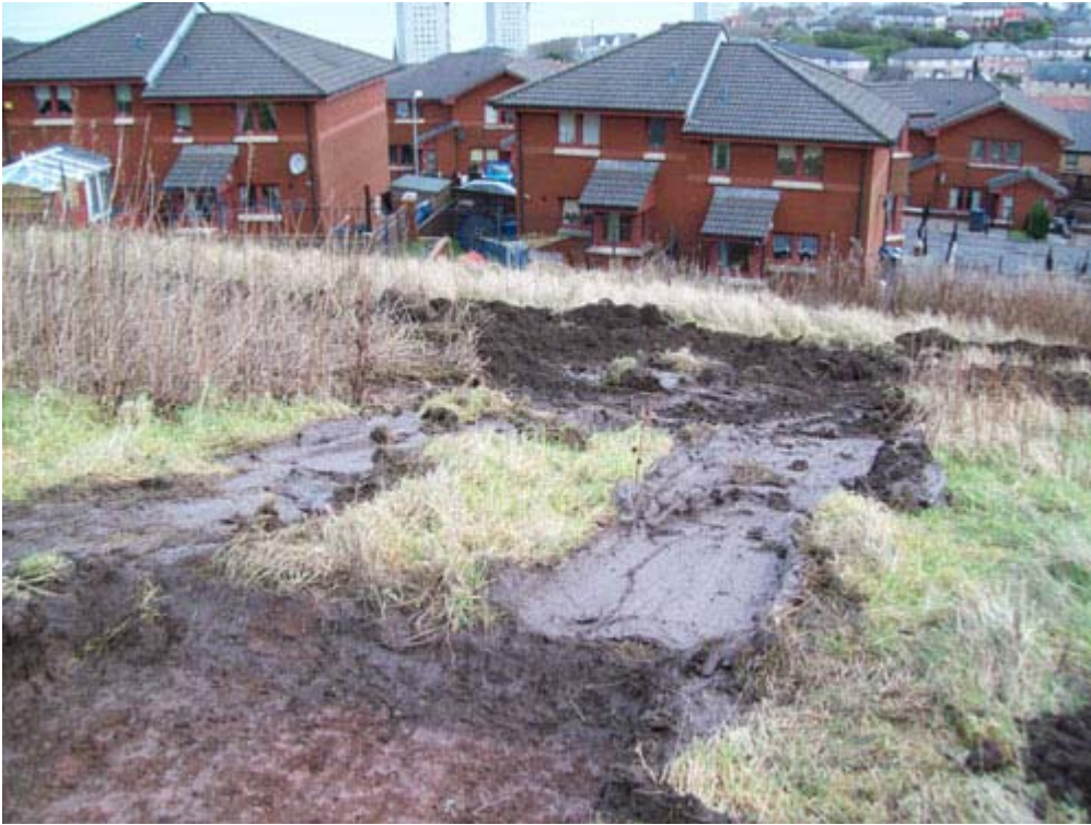
Figure 1: Digger slide due to saturated topsoil
