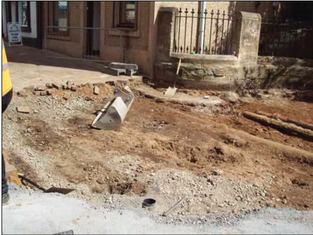
Figure 6a: Area 3: Disturbance caused by 19 th & 20 th Century Service Pipes
