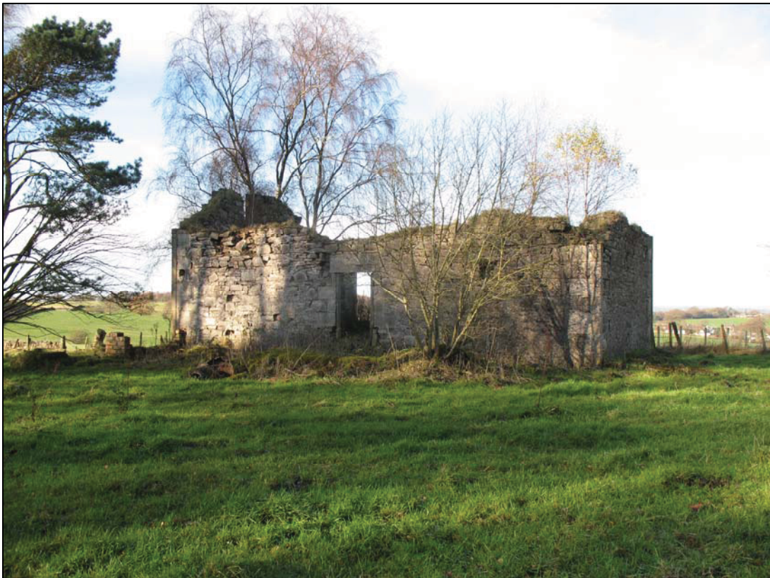
Figure 5b: Ruined Dwelling S1 , rear elevation from southeast
