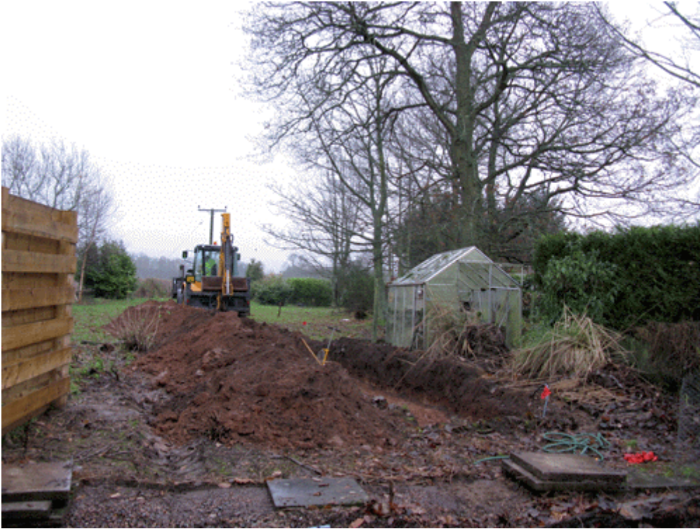
Figure 3a: General shot of site from the north with trench 2 in the foreground
