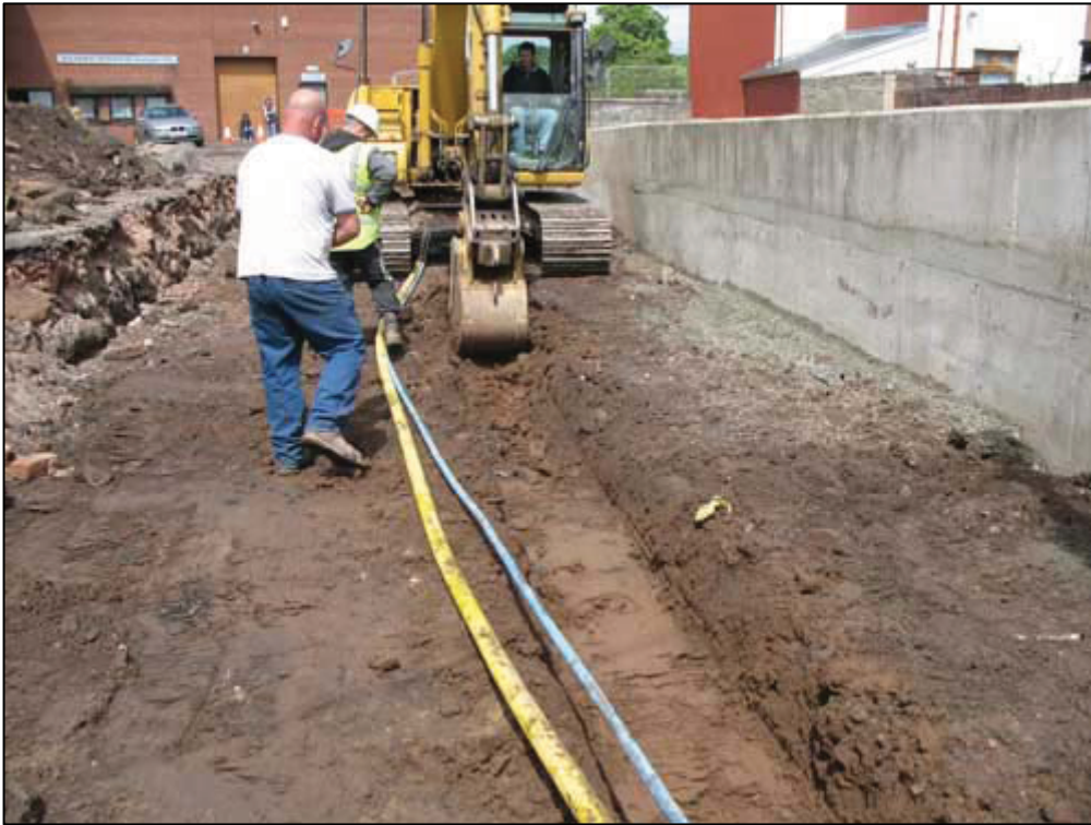
Figure 6a: Ground Reduction complete, Area A, With the digging of Drainage Trench i in progress
