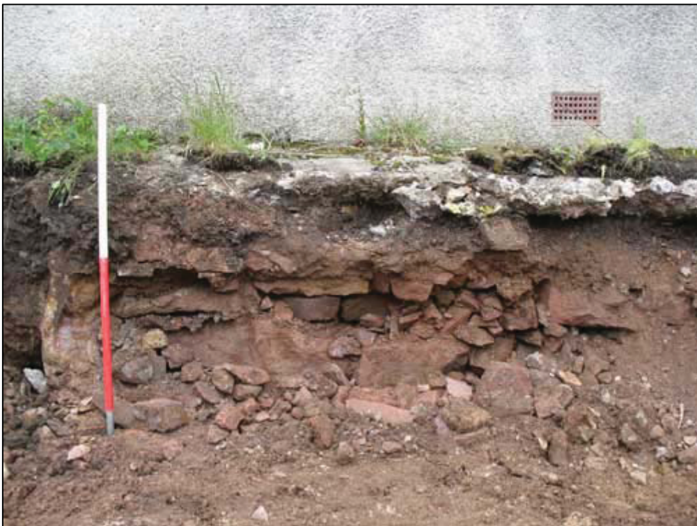
Figure 4b: Sandstone foundation revealed at W edge of Area C (NW Parking Bay)
