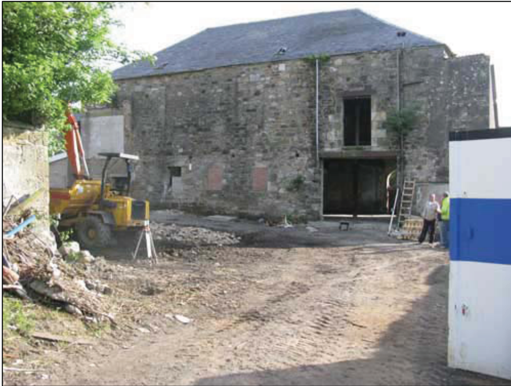
Fig. 3a: View Showing Rear of Late 19 th Century Granary Prior to Ground Reduction
