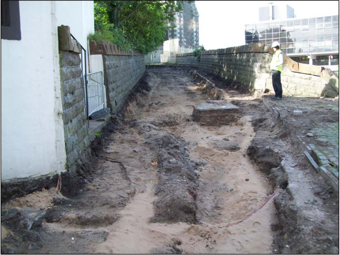
Figure 4a: The access lane to Trinity Church demonstrating the natural (004) and heavy truncation by services
