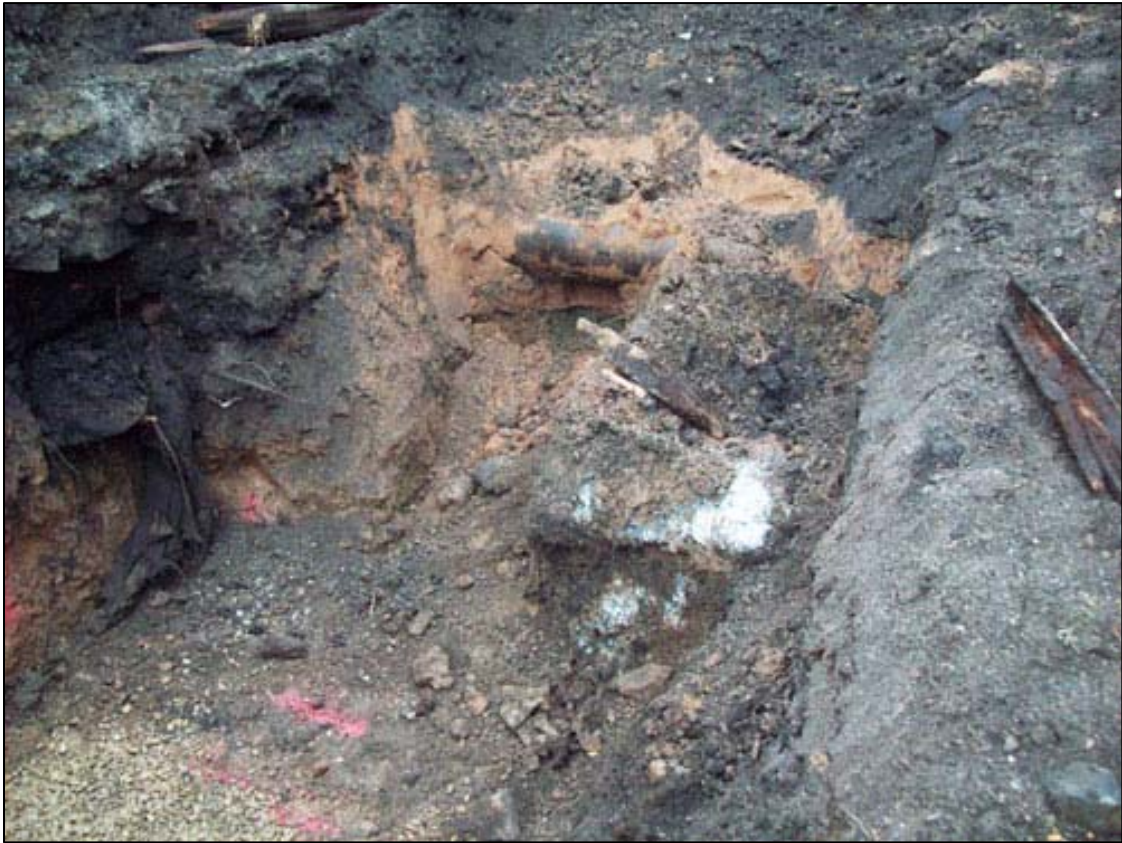
Figure 4a: Concrete anchor and large gas pipe
