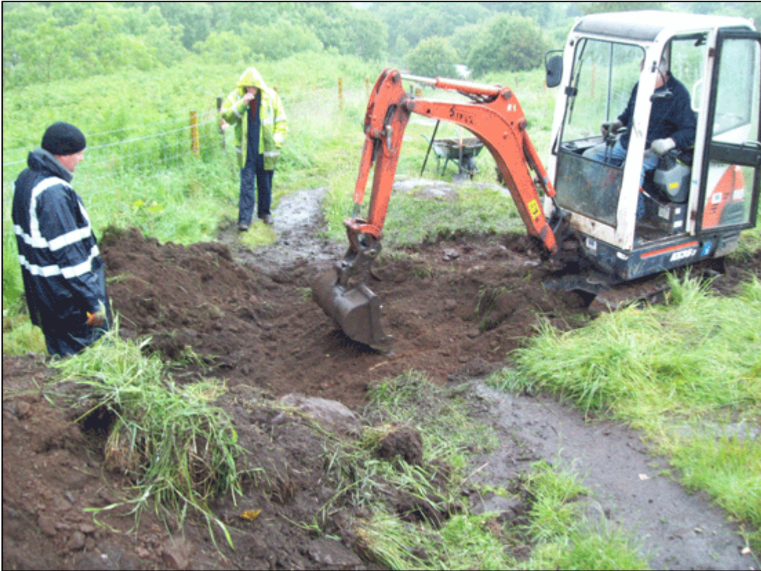
Figure 8a: Stripping the area for new entrance gate at the location of ENT 1
