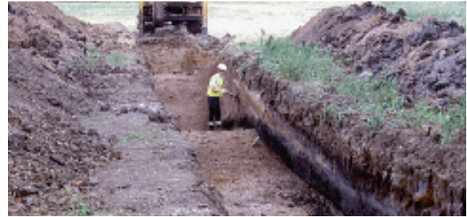
Late prehistoric palaeochannel at Hicken's Bridge, Aston-upon-Trent, Derbyshire; deposits of peat show as a dark wedge in the side of the excavation (photograph: A.J. Howard)
