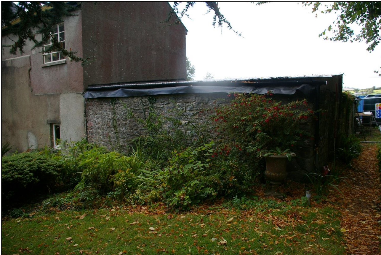
16. THE EAST AND NORTH WALLS OF B3, WITH 2M SCALE; FROM THE NORTH-EAST.
