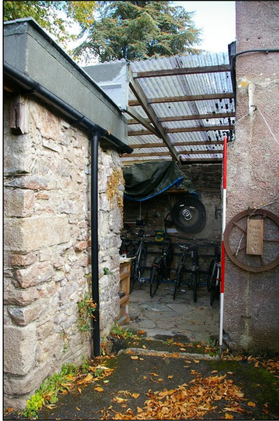
3. THE FORCED HOLE IN THE WALL OF THE 'GARDEN WING' WHICH LEADS INTO B3C AND RUINED CONTINUING WALL; FROM THE WEST-SOUTH-WEST (2M SCALE).
