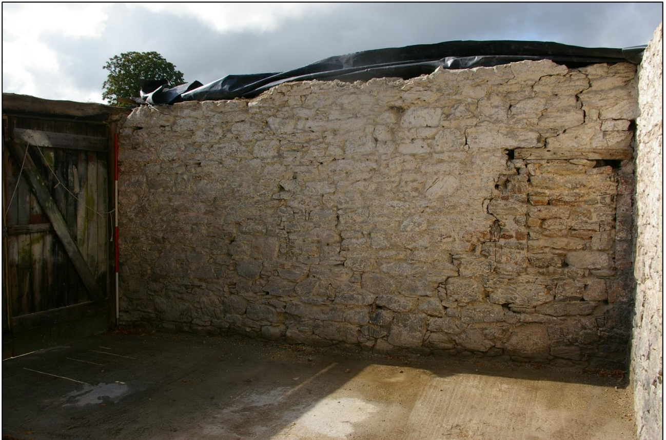
40. THE WEST WALL OF B2, WITH 2M SCALE, FROM WITHIN B2A; FROM THE NORTH-EAST (2M SCALE).
