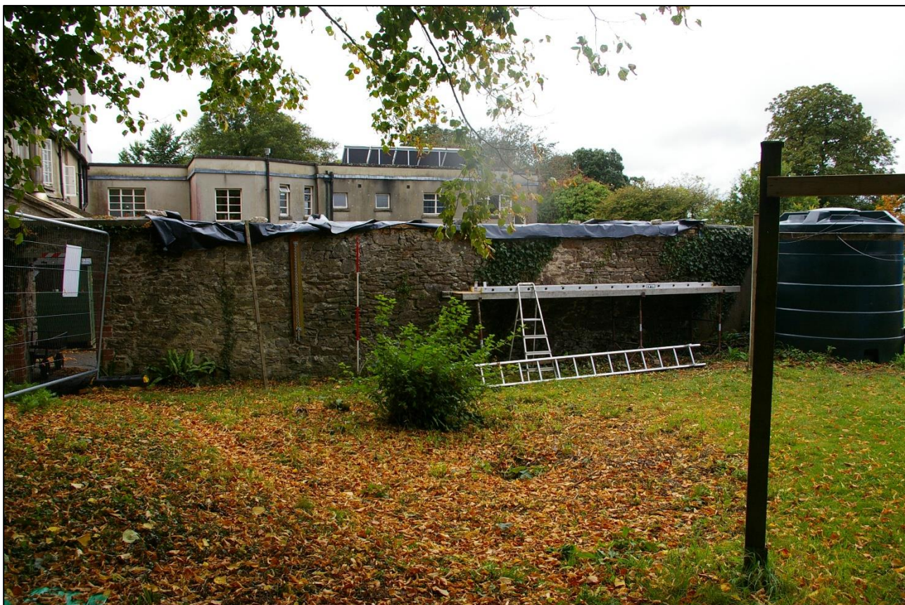
17. THE NORTH WALL OF B2 AND TO THE EAST END, JUST BEFORE THE FORCED ARCHWAY THE CHANGE OF BUILD AND CLEAR LINKING REPAIR SECTION OF WALLING; FROM THE NORTH-NORTH-EAST (2M SCALE).
