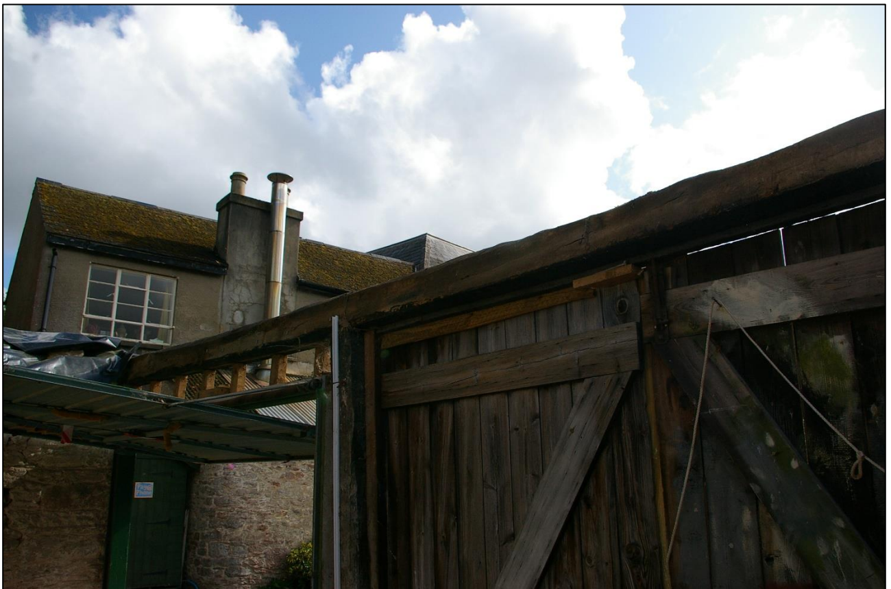
29. THE HEAVY POST AND BEAM WHICH BRACE THE SOUTH WALL OF B2; FROM THE WEST-NORTH-WEST.
