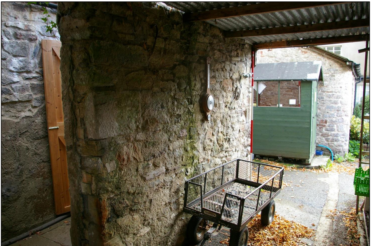
12. THE WEST WALL OF B3B, A DIFFERENT FORM OF BUILD, MUCH LOOSER WITH DRESSED STONES TO CORNERS; (2M SCALE).
