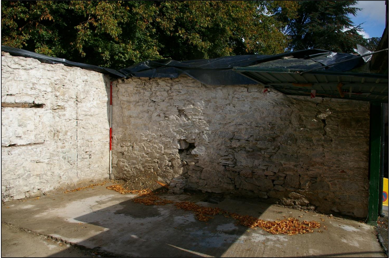
32. THE PARTITION WALL AND NORTH WALL, IN B2A; FROM THE SOUTH-WEST (2M SCALE).
