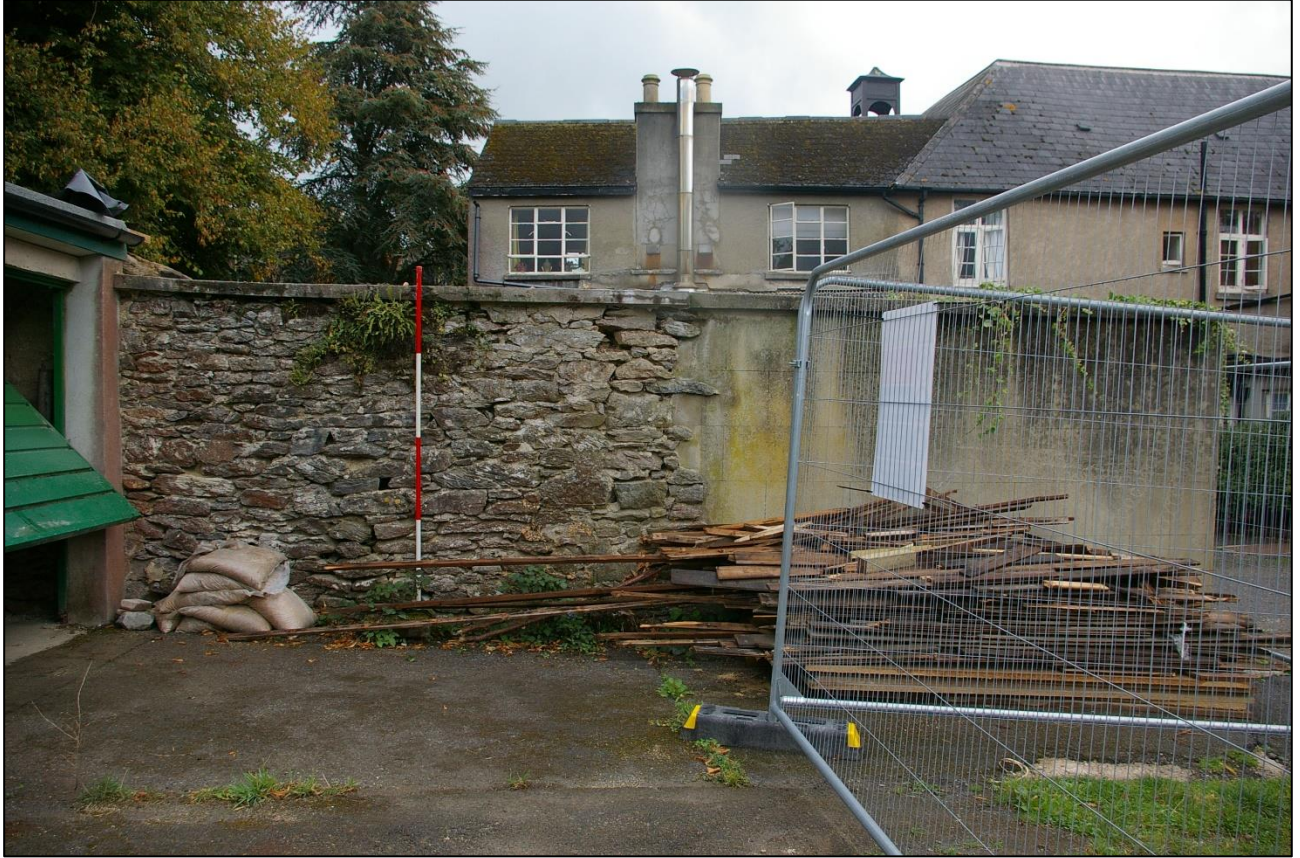
22. THE WEST WALL OF B2, SHOWING TRUNCATION AND POOR REPAIR AND RENDERED (BLOCK) END; FROM THE WEST (2M SCALE).
