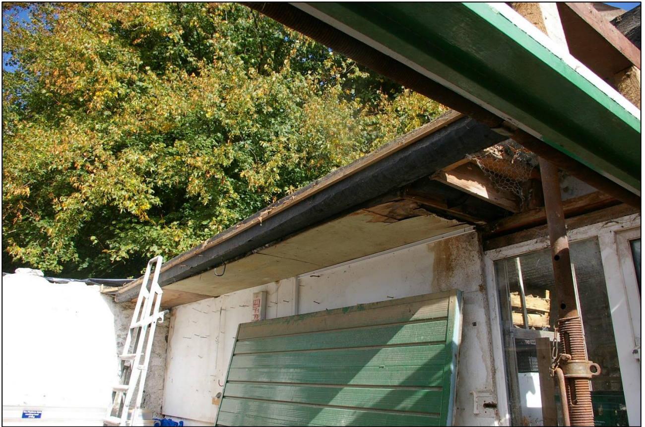
42. THE HEAVY BEAM WHICH CARRIED THE END OF THE SLATE ROOF OVER B2, AS THE EAST WALL, NOW CONCRETE BLOCK HAD BEEN BUILT OUT OF LINE FROM THE ORIGINAL BUILDING; FROM THE SOUTH-WEST.
