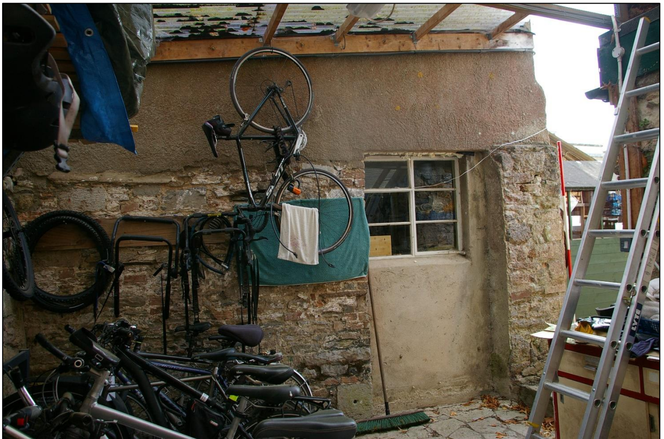
6. THE NORTH WALL OF THE 'GARDEN WING', FROM INSIDE B3C; FROM THE NORTH-NORTH-EAST (WITH 2M SCALE).
