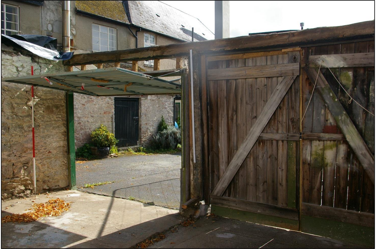
30. THE SOUTH WALL OF B2, SHOWING THE DIFFERENT TYPES OF DOORS; FROM THE NORTH-WEST (2M SCALE).
