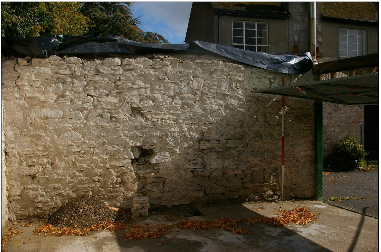
31. THE PARTITION WALL BETWEEN B2A AND B2B, OF LOOSER MORE IRREGULAR RUBBLE STONE; FROM THE NORTH-WEST (2M SCALE).
