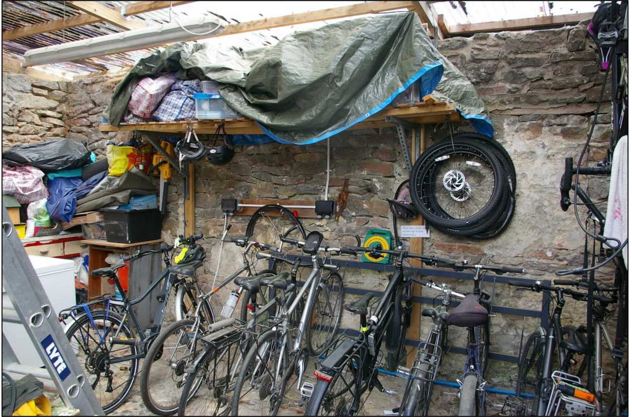
7. THE EAST WALL OF B3, FROM WITHIN B3C, SHOWING BLOCKED WINDOW BW5, TO THE SOUTH END; FROM THE SOUTH-WEST.
