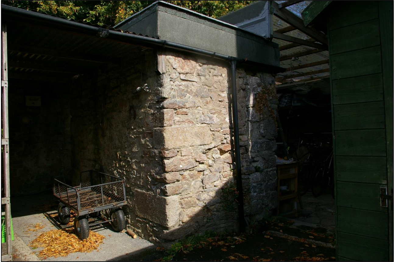
11. THE L-SHAPED SECTION OF NEWER WALLING WHICH ENCLOSES AND FORMS B3B WITHIN THIS INFILL AND REMODELLED STRUCTURE; FROM THE SOUTH-WEST.
