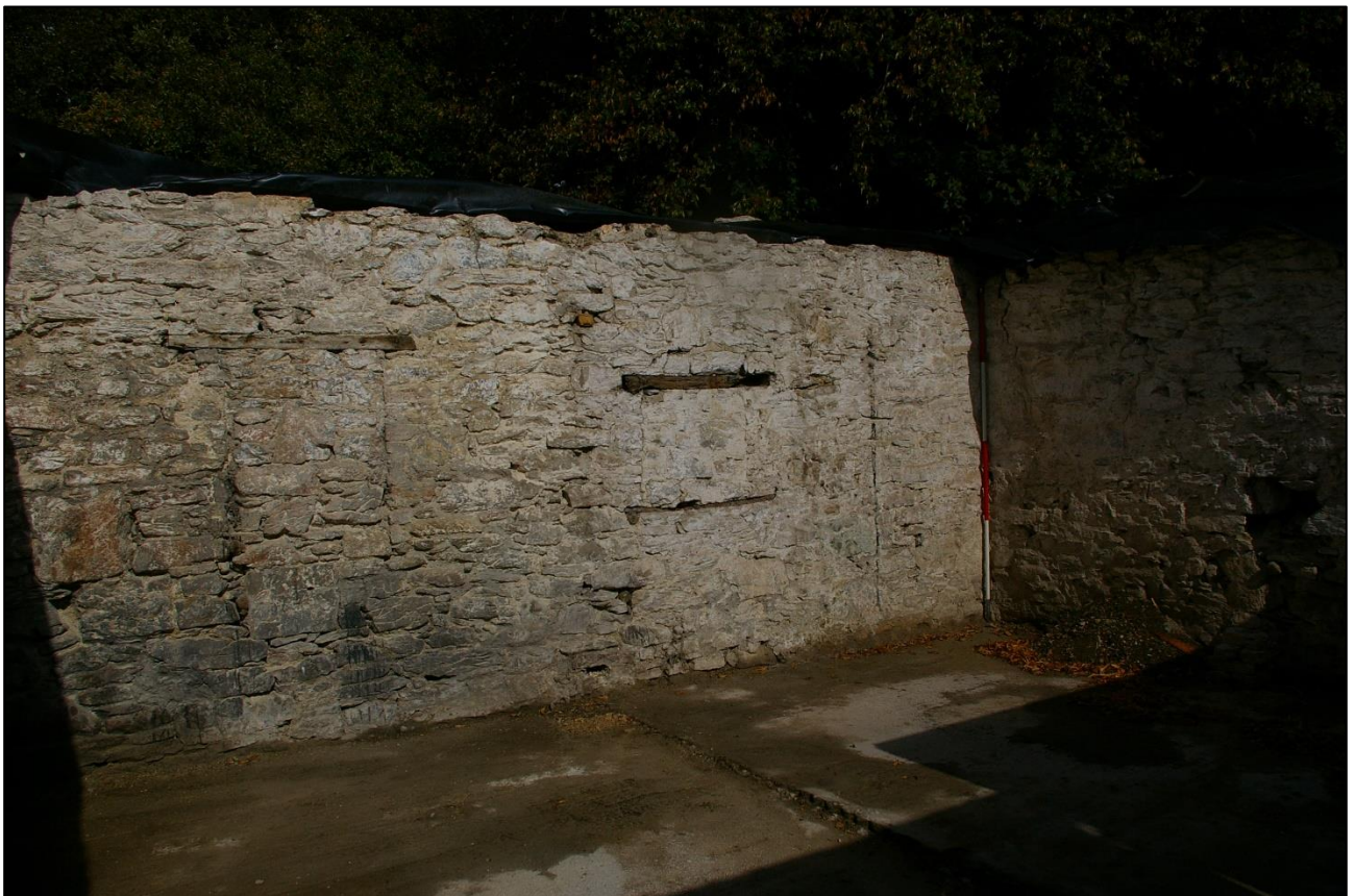
33. THE NORTH WALL WITH THE TWO VERY DIFFERENT BLOCKED OPENINGS BW1 AND BW2; FROM THE SOUTH-WEST (2M SCALE).
