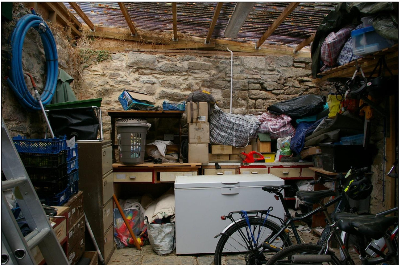
8. THE NORTH WALL OF B3, FROM WITHIN B3C, SHOWING LOTS OF REPOINTING AND REPAIR; FROM THE SOUTH.
