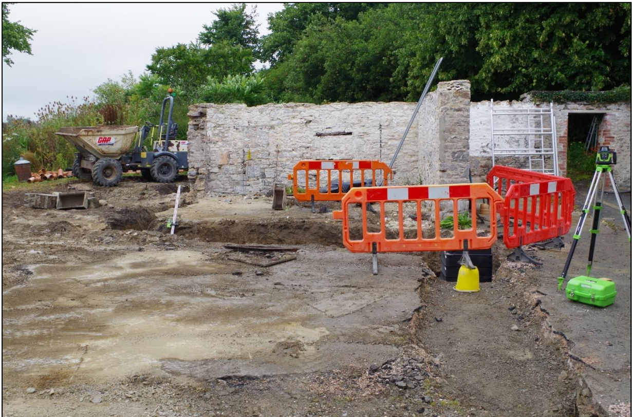
FIGURE 5: WORKS IN PROGRESS, FOLLOWING DEMOLITION OF WALL {110} AND EXCAVATIONS OF WALL FOOTINGS. FROM THE SOUTH.
