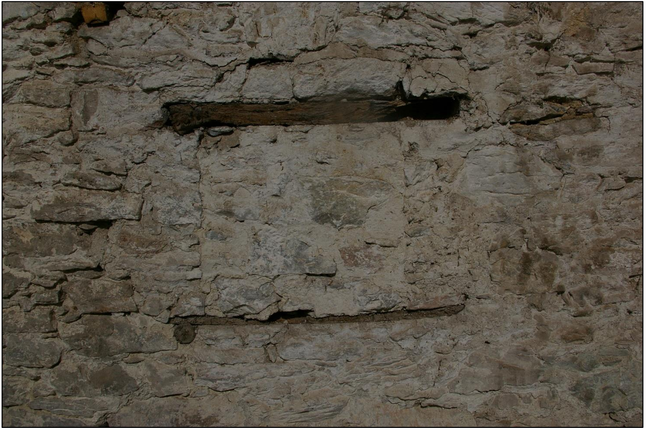
34. BW1, THE SMALLER SQUARER WINDOW, SET LOWER IN THE WALL; FROM THE SOUTH.
