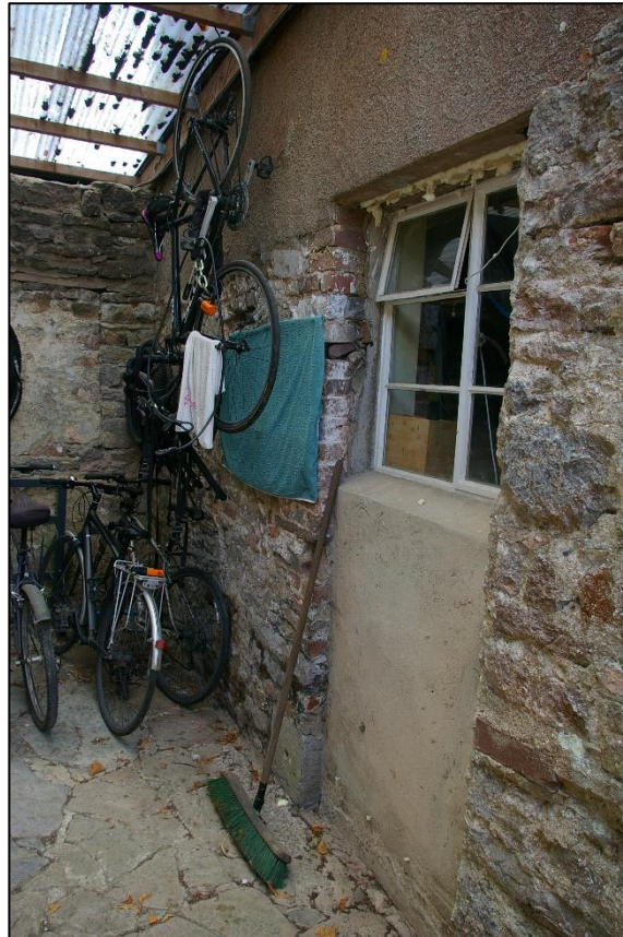
5. THE BLOCKED DOORWAY IN THE NORTH WALL OF THE CURRENT 'GARDEN WING'; FROM THE WEST-NORTH-WEST.
