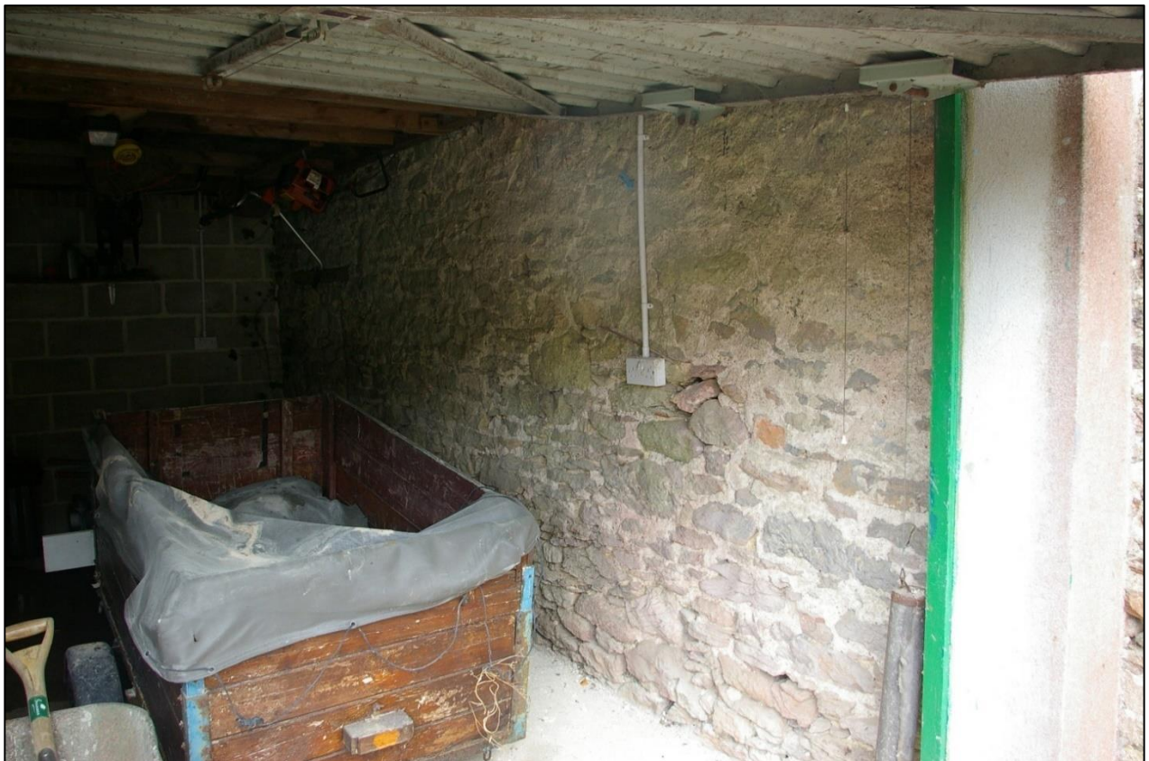
23. THE OUTER FACE OF THE WEST WALL OF B2, FROM WITHIN B1, SHOWING THE BLOCKED OPENINGS; FROM THE SOUTH-WEST.
