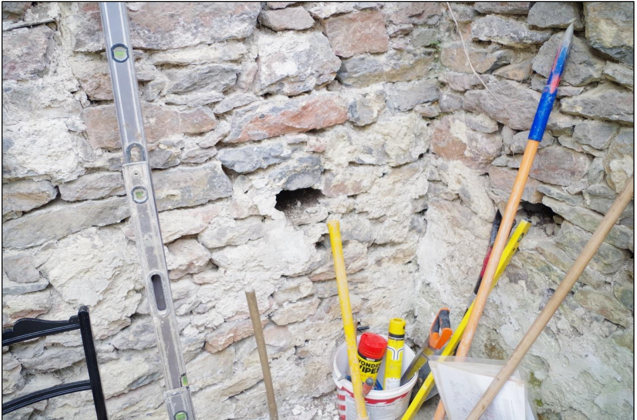
43. HIDDEN STASH HOLE IN ROOM AT END OF GARDEN WING, VIEWED FROM THE SOUTH.
