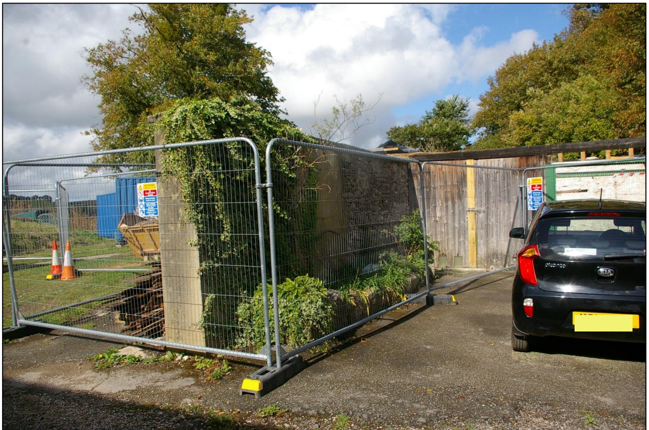
25. THE LONG PROJECTING SECTION OF WALL TO THE WEST OF B2; FROM THE SOUTH-SOUTH-EAST.
