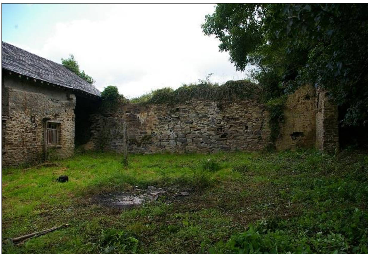
FIGURE 7: THE RUINED WALLS WHICH FRAME THE STANDING BARN ON THE SITE; FROM THE WEST.
