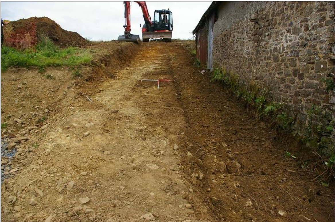
14. LOWERING THE LEVELS BEHIND THE BARN, SHOWING A CURVED CUT BEHIND THE BUILDINGS, SET INTO THE NATURAL SLOPE OF THE GROUND (2 x 1M SCALE); FROM THE WEST.
