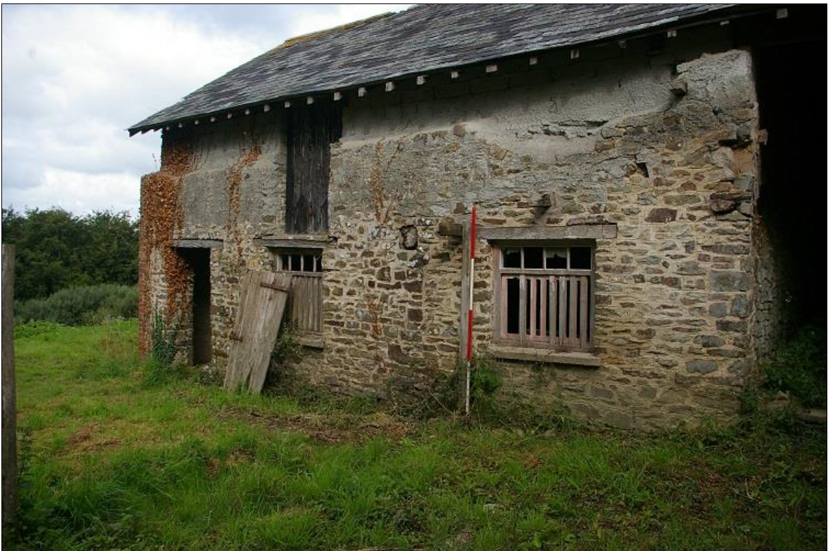
6. THE STANDING BARN (2M SCALE), SHOWING BUILD LINE TO THE CENTRE OF THE ELEVATION, FROM THE SOUTH-EAST.
