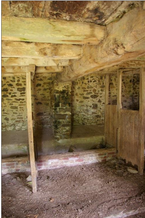
21. EXAMPLE OF ONE OF THE PIERS HOLDING UP THE SHORTER BEAMS AND BRACING THE LOFT FLOOR, AS WELL AS THE TROUGHS AND CONCRETE BRACING; FROM THE SOUTH-WEST.
