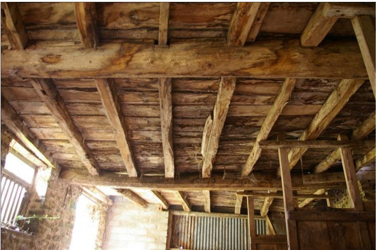
20. THE TIMBER LOFT, REUSING SOME EARLIER MATERIAL, CRANKED TO THE WEST END WHERE THE WALL HAS BEEN TRUNCATED; FROM THE EAST.
