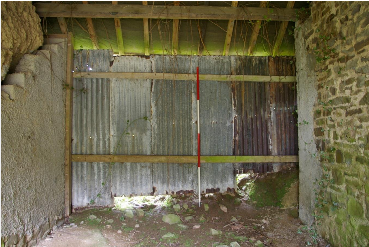
8. THE TIMBER AND CORRUGATED FRAMING AT THE EASTERN END OF THE STANDING RANGE (2M SCALE); FROM THE SOUTH.
