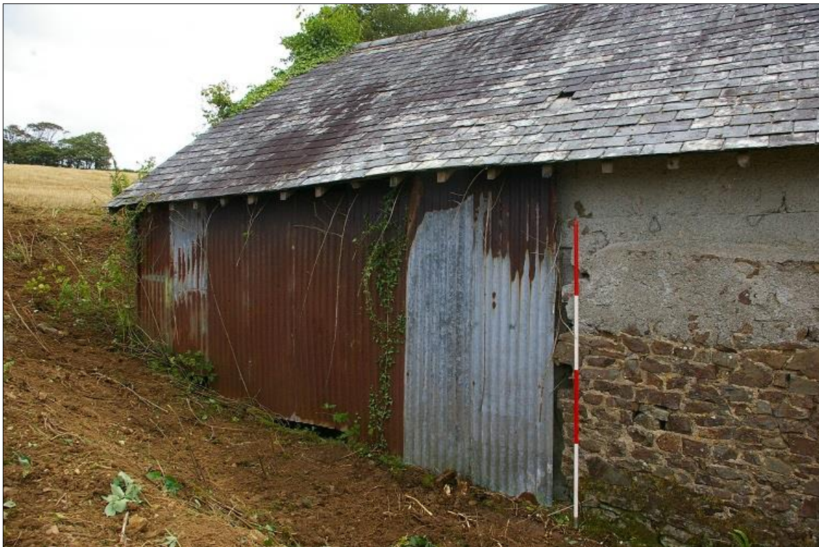
4. THE EAST END OF THE NORTH WALL (2M SCALE); FROM THE NORTH-NORTH-WEST.
