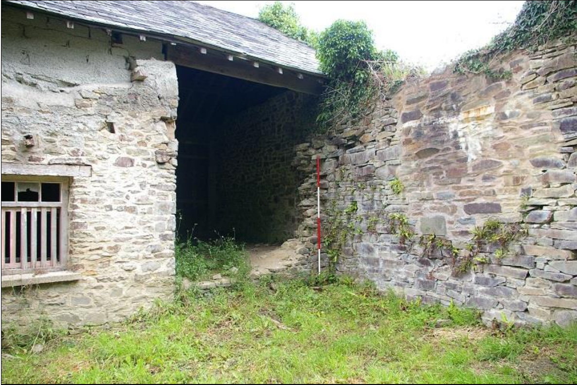
7. THE EAST WALL OF THE COMPLEX, WITH MULTIPLE PHASES OF REBUILT WITHIN THE STONE (2M SCALE) AND TRUNCATED EAST END OF THE STANDING RANGE; FROM THE SOUTH-WEST.
