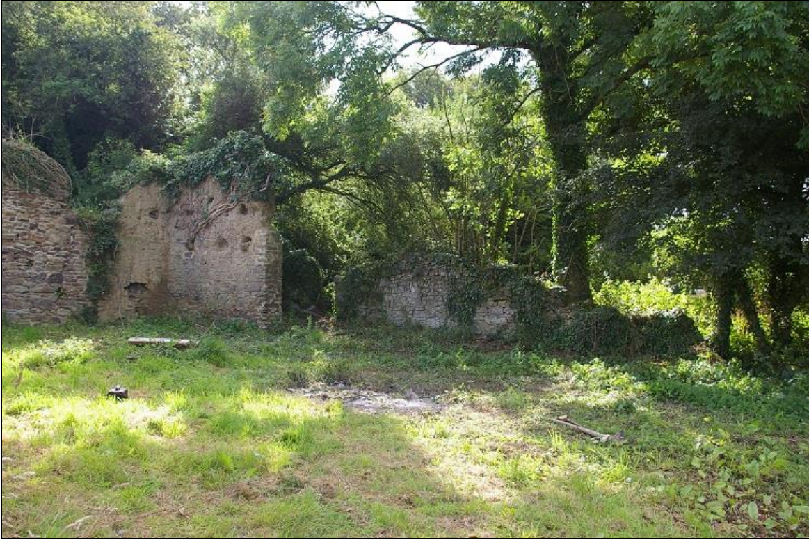
11. THE COB RUINED RANGE, PARALLEL TO THE STANDING RANGE; FROM THE WEST-NORTH-WEST.
