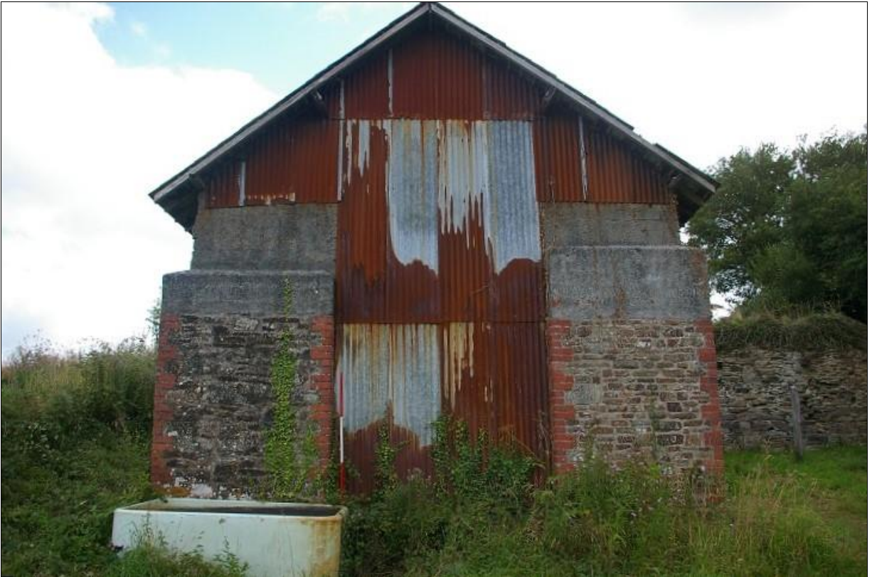
2. THE WESTERN, TRUNCATED ELEVATION OF THE BARN (2M SCALE), REBUILT IN THE 20 TH CENTURY; FROM THE WEST.
