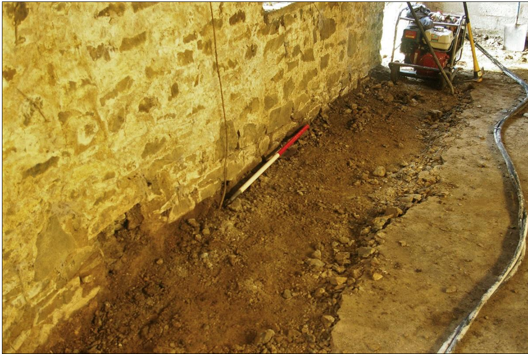
38. VIEW OF REMOVAL OF CONCRETE FLOOR IN BARN, SHOWING LOOSE DAMAGED FORMER COBBLED FLOOR BENEATH (1M SCALE); FROM THE EAST-NORTH-EAST.
