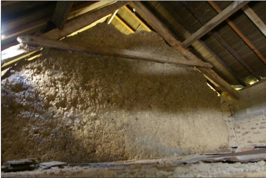
24. THE COB WALL IN THE STANDING BARN, WITH A-FRAME; FROM THE WEST-NORTH-WEST.
