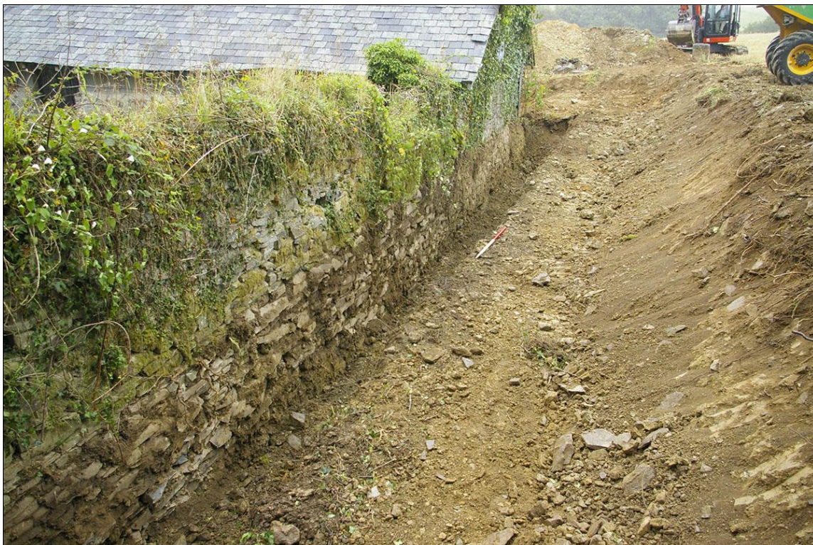
25. VIEW OF THE DRAINAGE TRENCH BEING EXCAVATED BEHIND THE EAST WALL, EXPOSED THE TRADITIONAL BUILD, WITHOUT A 'FACE', AS IT HAS BEEN BUILT INTO THE BANK, WITH 1M SCALE; FROM THE SOUTH-EAST.
