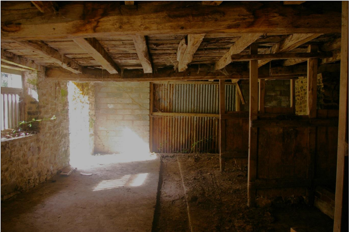
19. THE INTERIOR GROUND FLOOR OF THE BARN, SHOWING REBUILT WEST WALL WHERE THE RANGE HAS BEEN TRUNCATED; FROM THE EAST.
