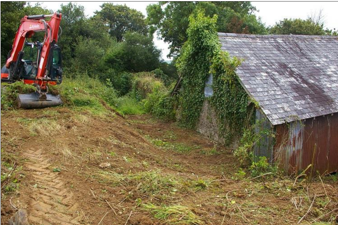
16. THE RUINED EAST WALL OF THE COMPLEX, BEING CLEARED OF VEGETATION; FROM THE NORTH-EAST.
