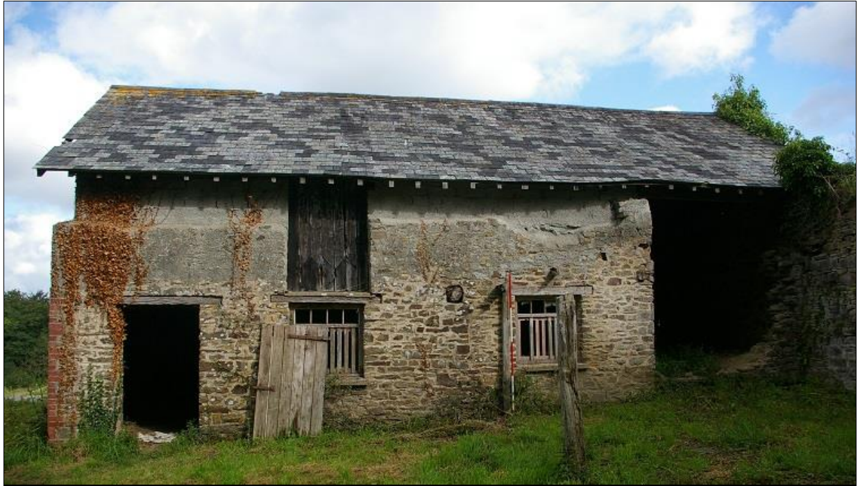
FIGURE 8: THE SOUTHERN ELEVATION OF THE STANDING BARN; FROM THE SOUTH-SOUTH-EAST (2M SCALE).
