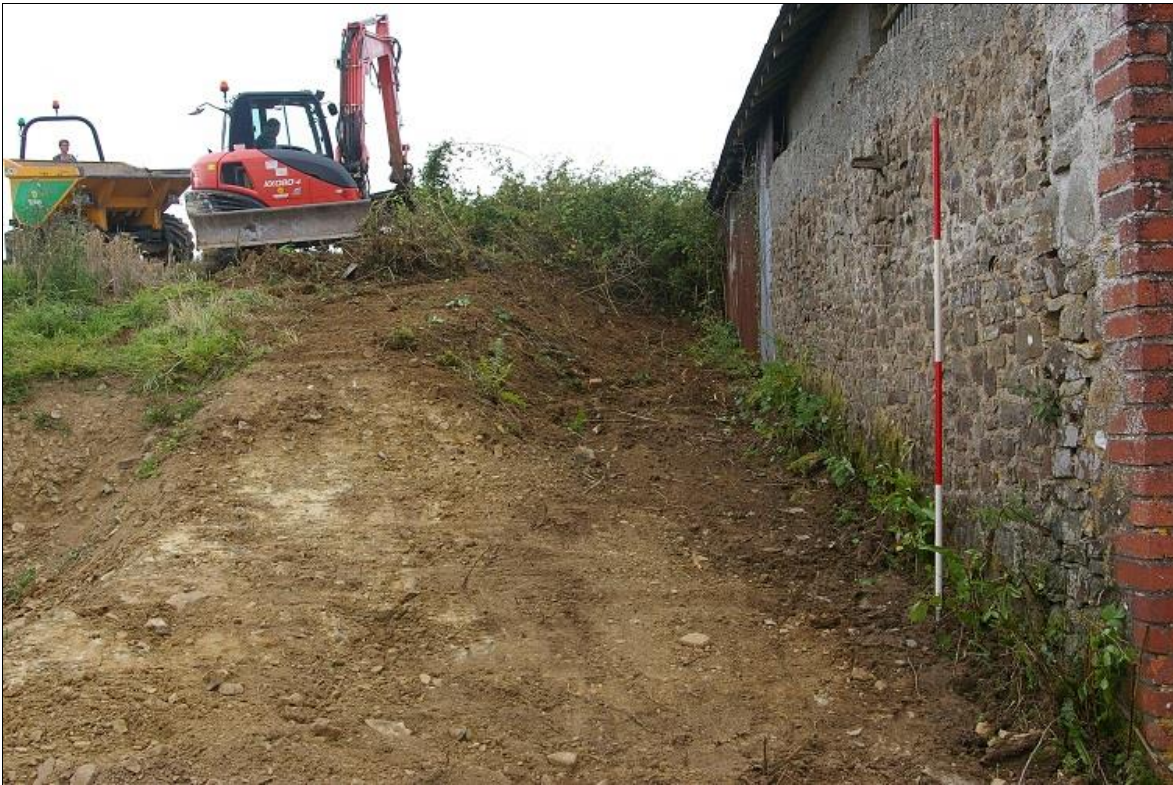
12. VIEW ALONG THE NORTH ELEVATION OF THE STANDING BARN, WITH FOLIAGE REMOVED, SHOWING BANK AND HISTORIC CUT/TERRACE FOR THE BUILDING, FILLED WITH DARKER, LOOSE SOIL (2M SCALE TO SIDE); FROM THE WEST.
