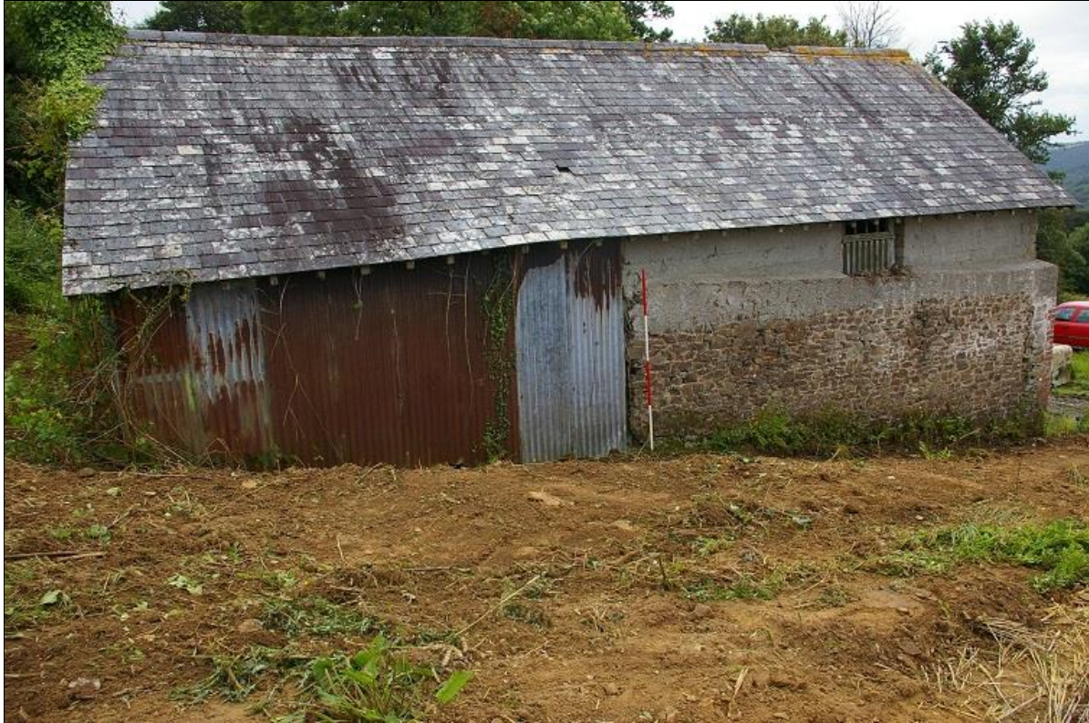
3. THE NORTH WALL OF THE BARN (2M SCALE), WITH CLEARED VEGETATION; FROM THE NORTH-NORTH-EAST.
