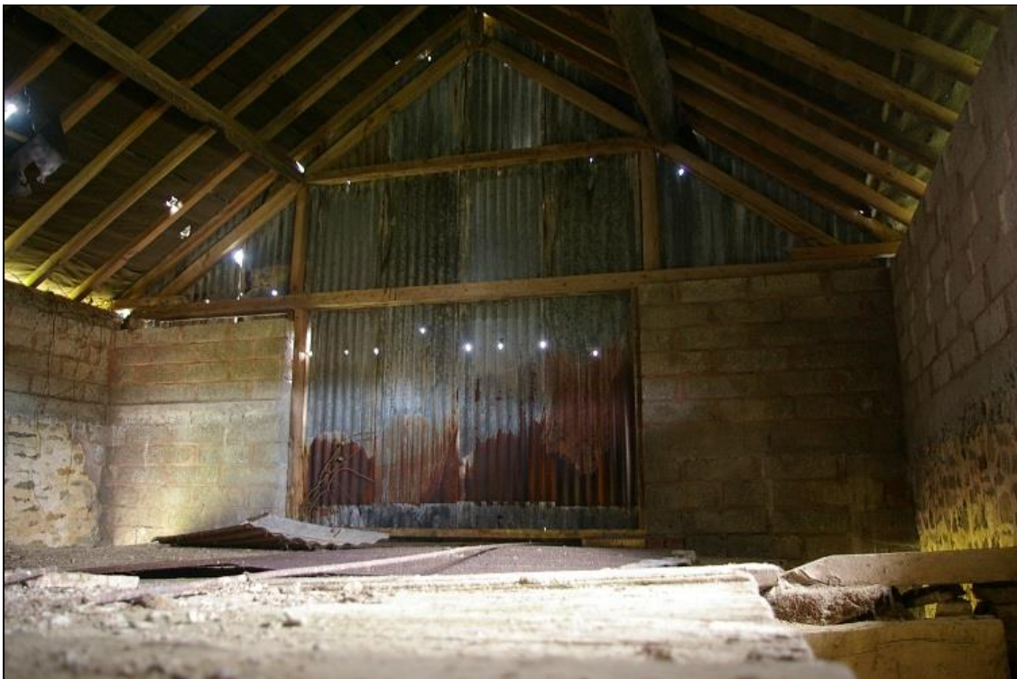
22. THE WEST WALL OF THE BARN, WITHIN THE LOFT; FROM THE EAST-NORTH-EAST.
