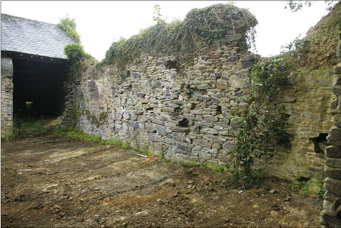
28. STRIPPED AREA WITHIN EASTERN DEMOLISHED BARN RANGE; FROM THE WEST (1M SCALE).
