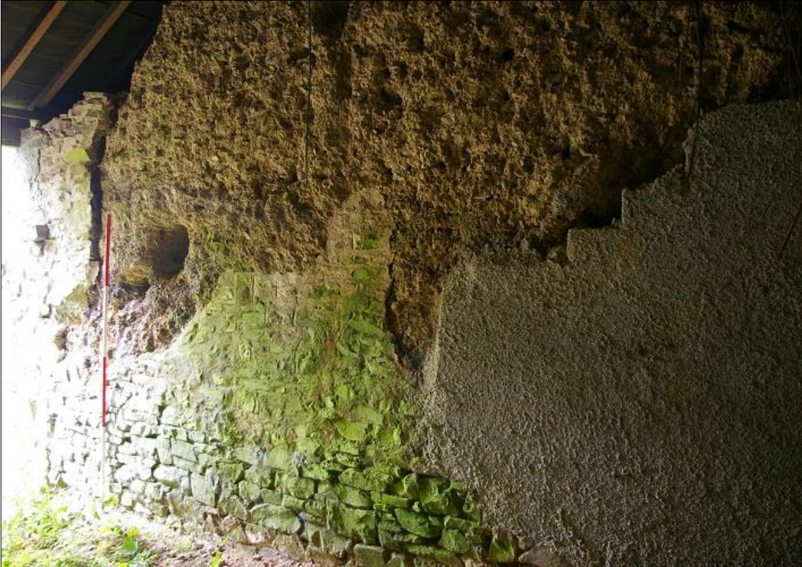
9. THE THICK COB WALL TO THE EAST END OF THE STANDING RANGE, A FRAGMENT OF AN EARLIER COMPLEX (2M SCALE); FROM THE NORTH-EAST.
