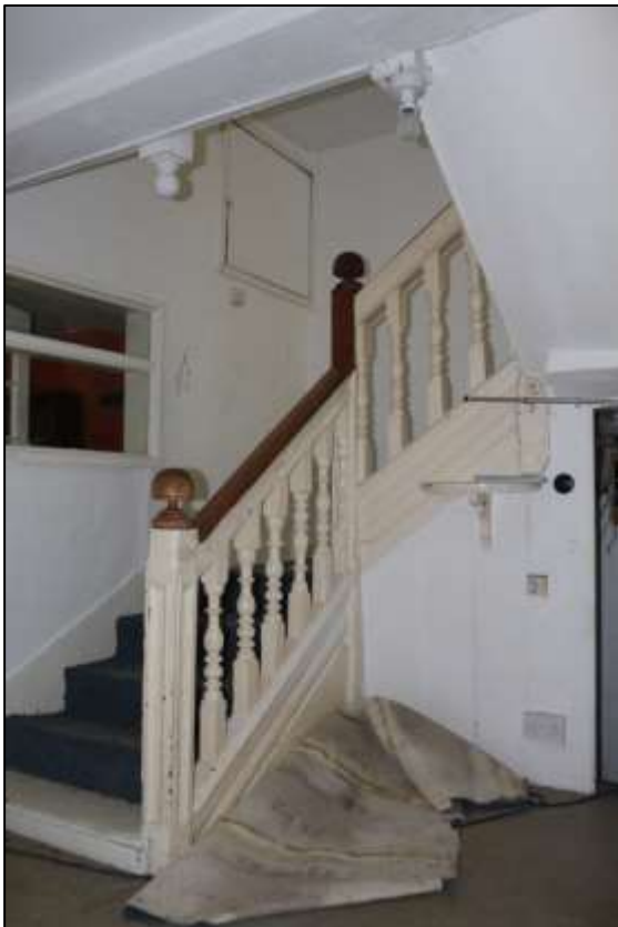
LEFT FIGURE 27: R2, THE BASE OF THE STAIRWELL; VIEWED FROM THE SOUTH.
