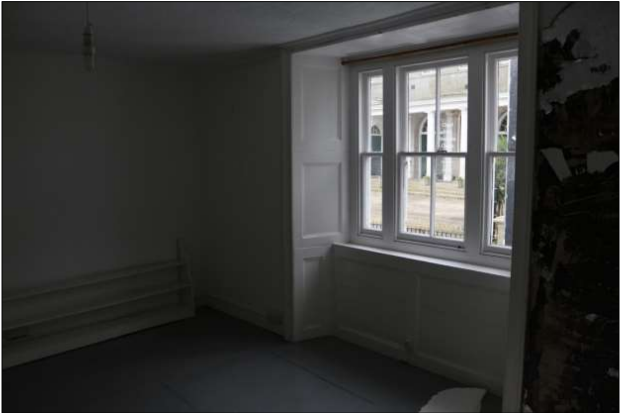
FIGURE 15: R7, THE EARLY C19 PANELLED SURROUND TO THE LATER C19 TRIPARTITE SASH; VIEWED FROM THE NORTH-WEST.
