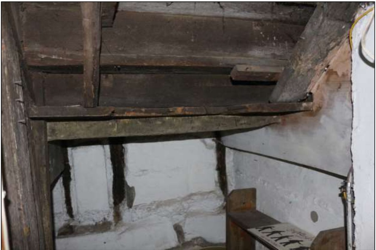
FIGURE 30: R2, BENEATH THE SECOND FLIGHT OF STEPS, SHOWING THEM BRACED AGAINST THE FLOORBOARDS OF THE FIRST HALF-LANDING; VIEWED FROM THE WEST.
