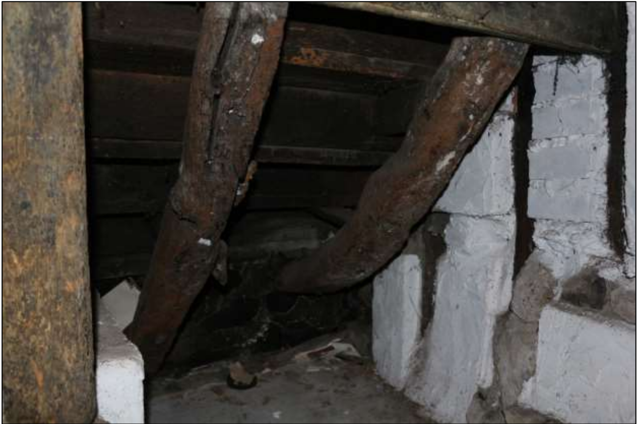
FIGURE 29: R2, BENEATH THE FIRST FLIGHT OF STEPS, SHOWING THE ?INSERTED CARRIAGE BRACES; VIEWED FROM THE NORTH.
