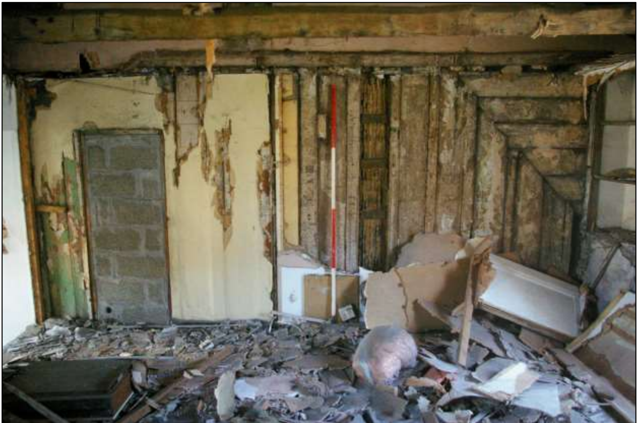
FIGURE 23: R8/R10, THE EAST PARTY WALL SHOWING THE VERTICAL PLANK BOARDING AND EVIDENT OF THE RAISE (LEFT); VIEWED FROM THE WEST.
