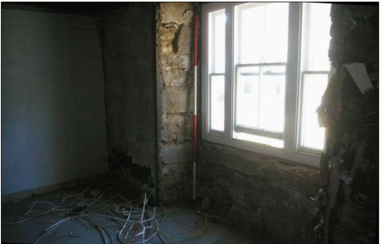
FIGURE 18: R7, THE WINDOW FOLLOWING THE REMOVAL OF THE PANELS; VIEWED FROM THE NORTH-WEST (SCALE 2M).
