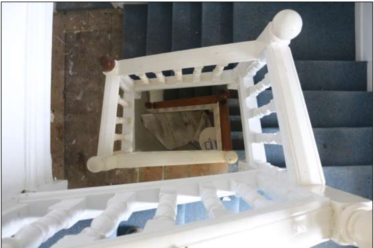
FIGURE 39: THE VIEW DOWN THE STAIRWELL FROM THE TOP; VIEWED FROM THE EAST.
