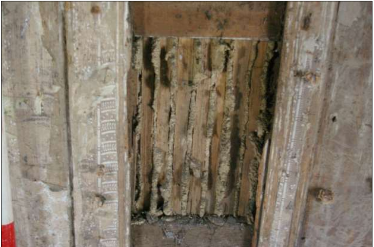
FIGURE 25: R10, DETAIL OF THE REGENCY WALLPAPER ADHERING TO THE PLANKS, AND THE VERTICAL LATH AND PLASTER ON THE REVERSE OF THE WALL; VIEWED FROM THE WEST.
