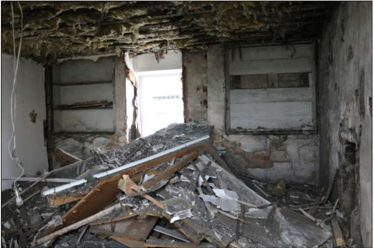
FIGURE 19: R9/R10 DURING THE STRIP, SHOWING THE RAISE TO THE SOUTH WALL AND THE INSERTED SHELVES; VIEWED FROM THE NORTH.
