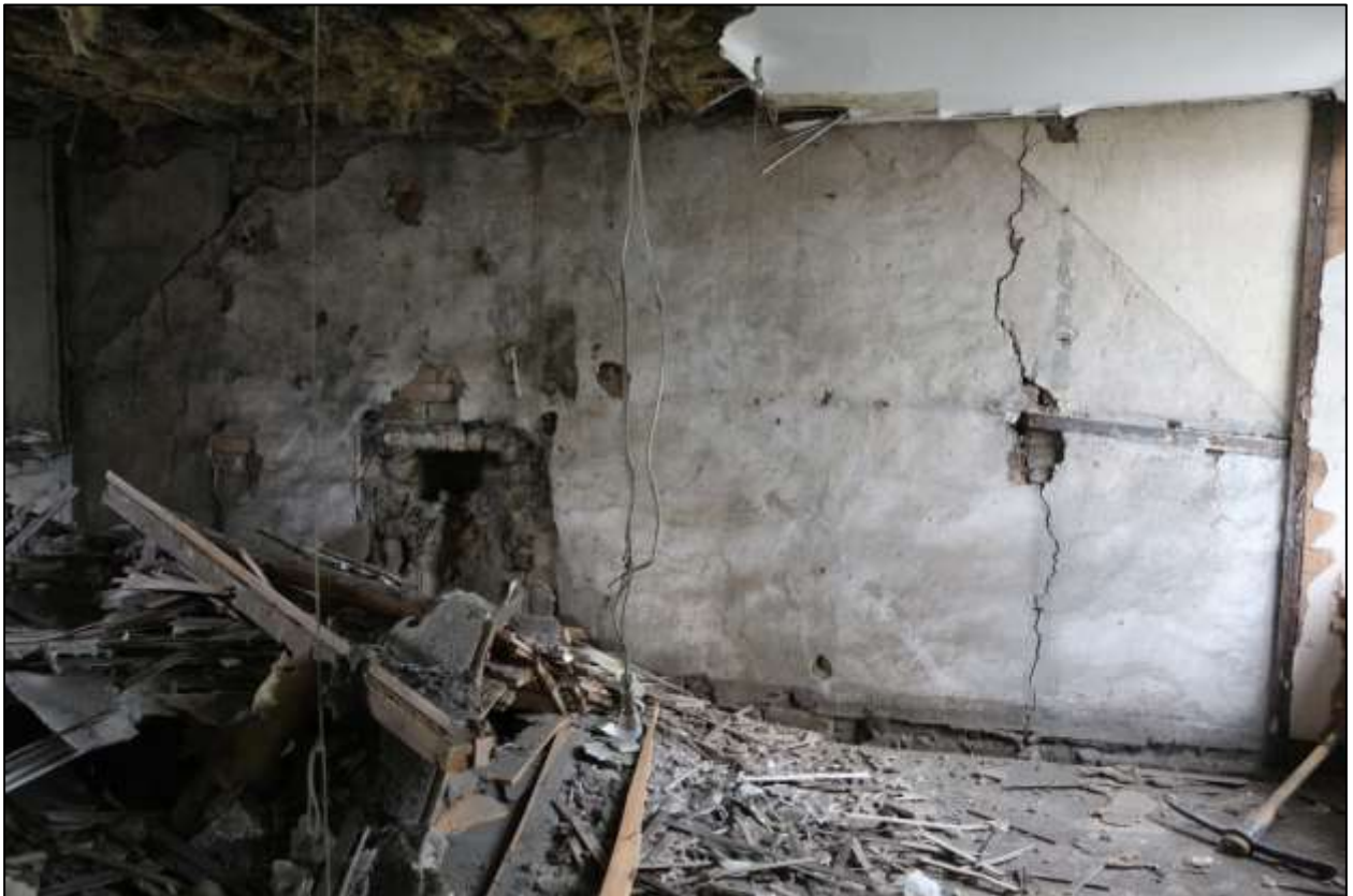
FIGURE 20: R9/R10, THE WEST GABLE WALL SHOWING THE FORCED FIREPLACE AND THE LINE OF THE ORIGINAL ROOF; VIEWED FROM THE EAST.
