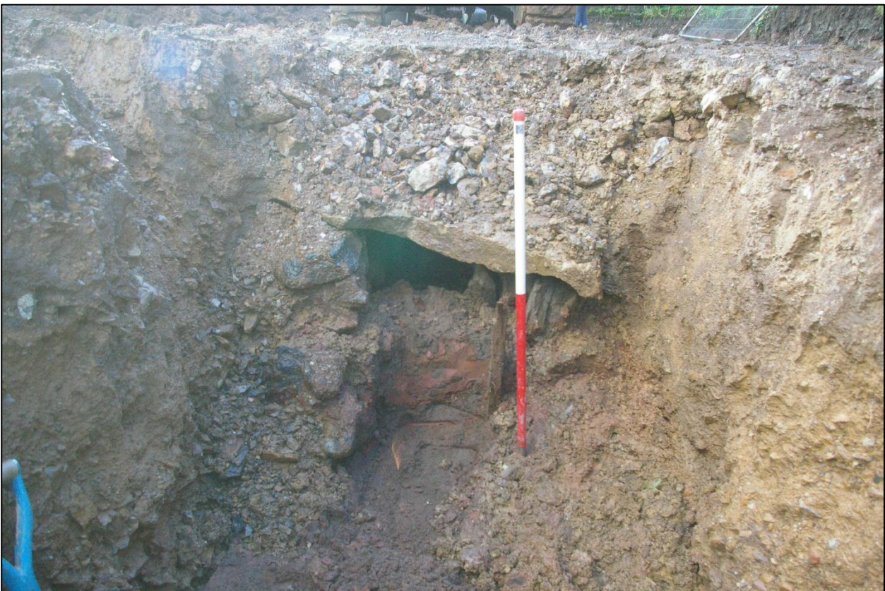
6. COLLAPSED NORTH FACING SECTION THROUGH CULVERTS IN CUT [1002], VIEWED FROM THE NORTH (1M SCALE).
