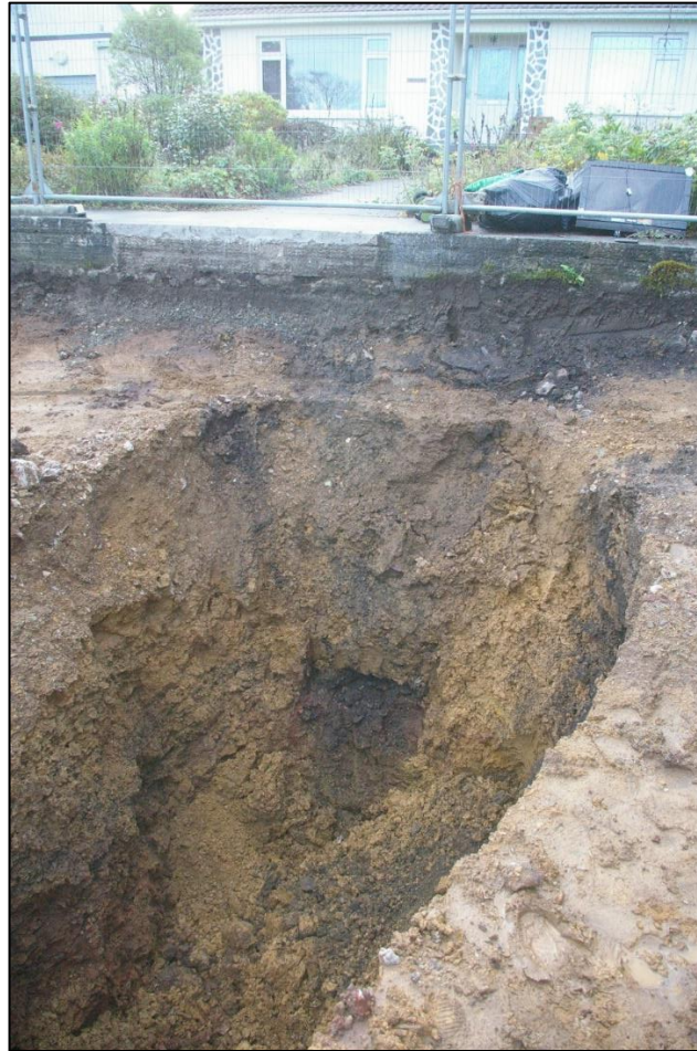
3. DRAIN [1002] IN SECTION AT THE SOUTHERN LIMIT OF THE SITE; VIEWED FROM THE NORTH-WEST (NO SCALE).
