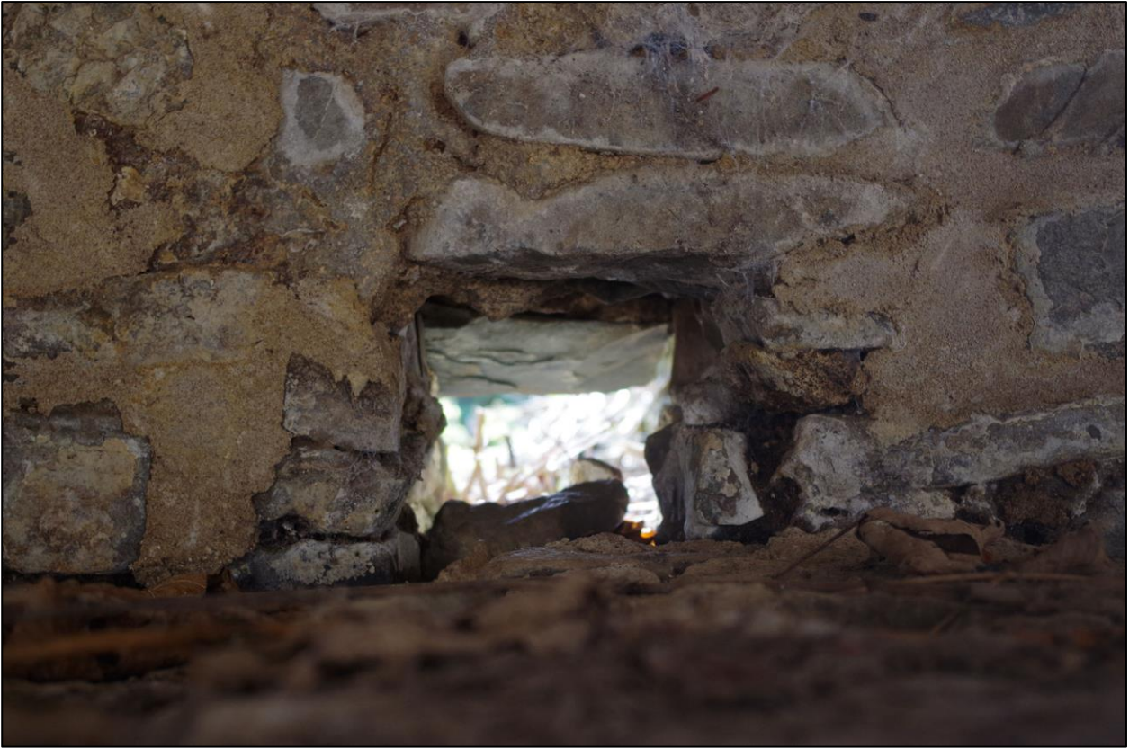
13. INTERNAL GUTTER-HOLE. TAKEN FROM THE NORTH.
