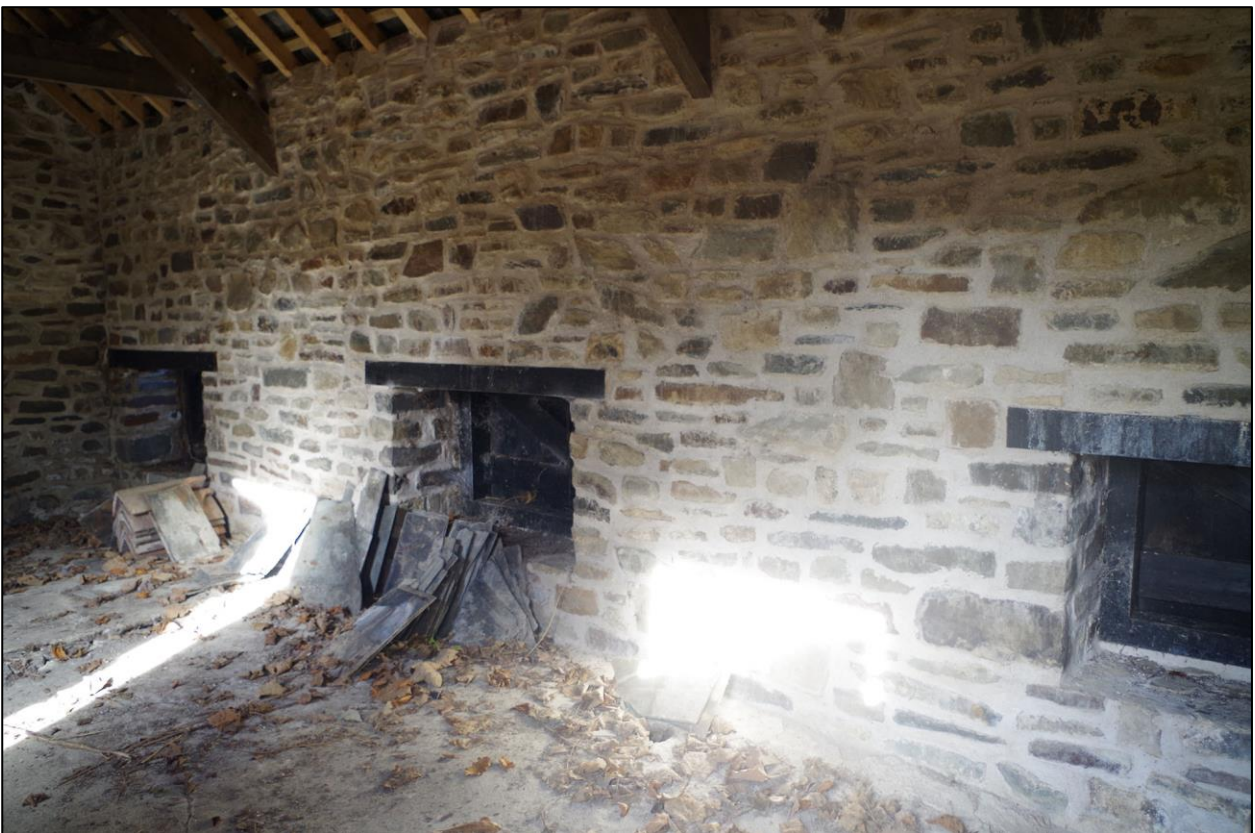
8. THE INTERNAL WINDOW OPENINGS WITH LEDGED AND BRACED WINDOWS. TAKEN FROM THE SOUTH-EAST.
