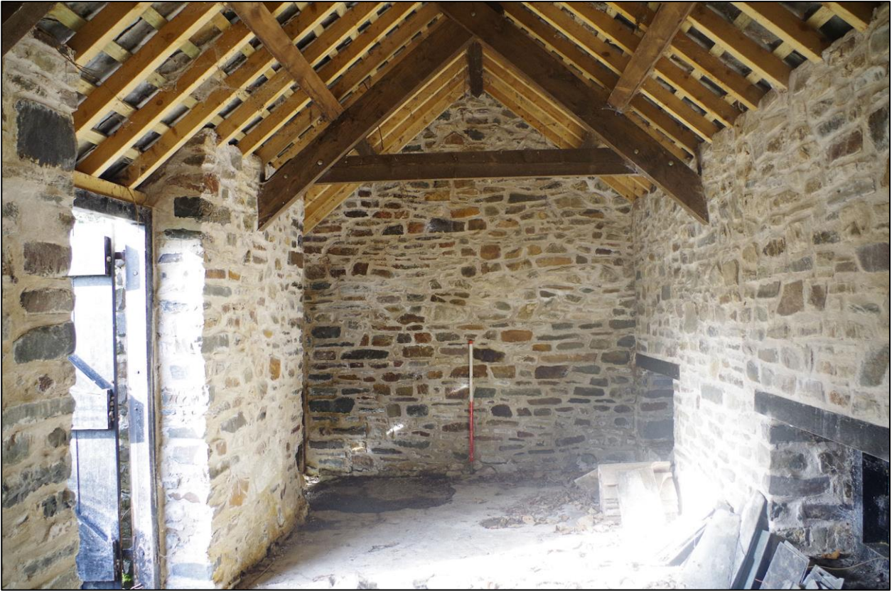
7. THE INTERIOR SPACE OF THE PIGGERY LOOKING TO THE WEST ELEVATION, DOORS MIRROR WINDOWS. TAKEN FROM THE EAST.
