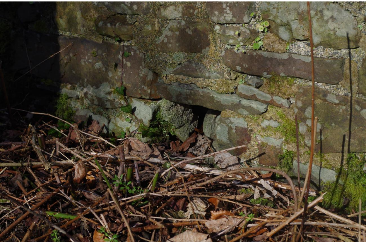
10. THE GUTTER HOLE TO THE EXTERNAL SOUTH ELEVATION ON THE EAST SIDE. TAKEN FROM THE SOUTH-EAST.
