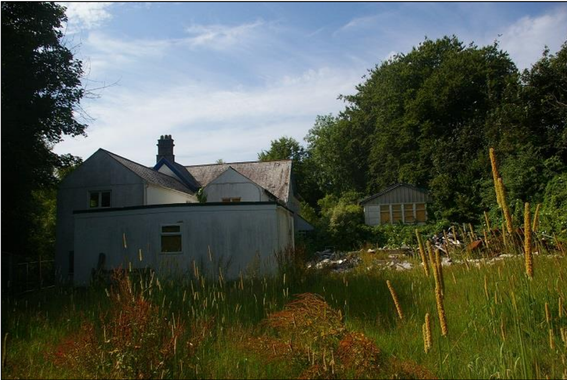
13. THE SETTING OF THE HOUSE TO THE REAR, WITH ONE OF THE OTHER TEMPORARY CLASSROOM BLOCKS AND BURNT FORMER GYMNASIUM; FROM THE NORTH.
