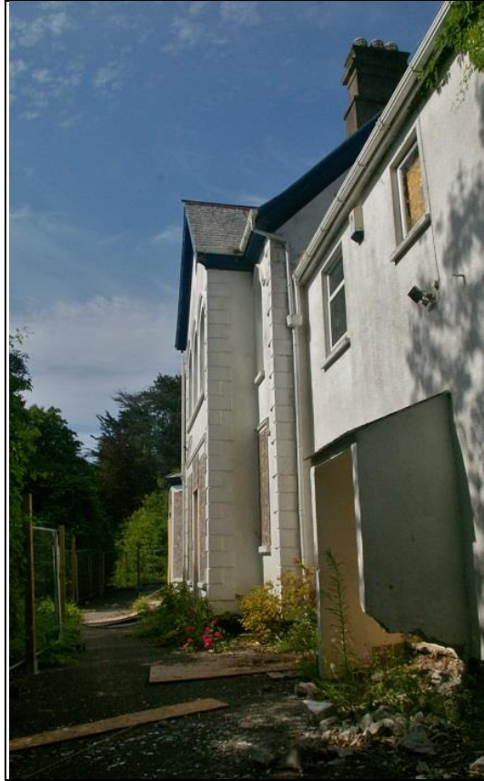
17. THE EAST ELEVATION OF THE HOUSE, SHOWING THE PROJECTING BAY SERVING THE FORMAL ENTERTAINING ROOM AND TERRACE AREA; FROM THE NORTH.
