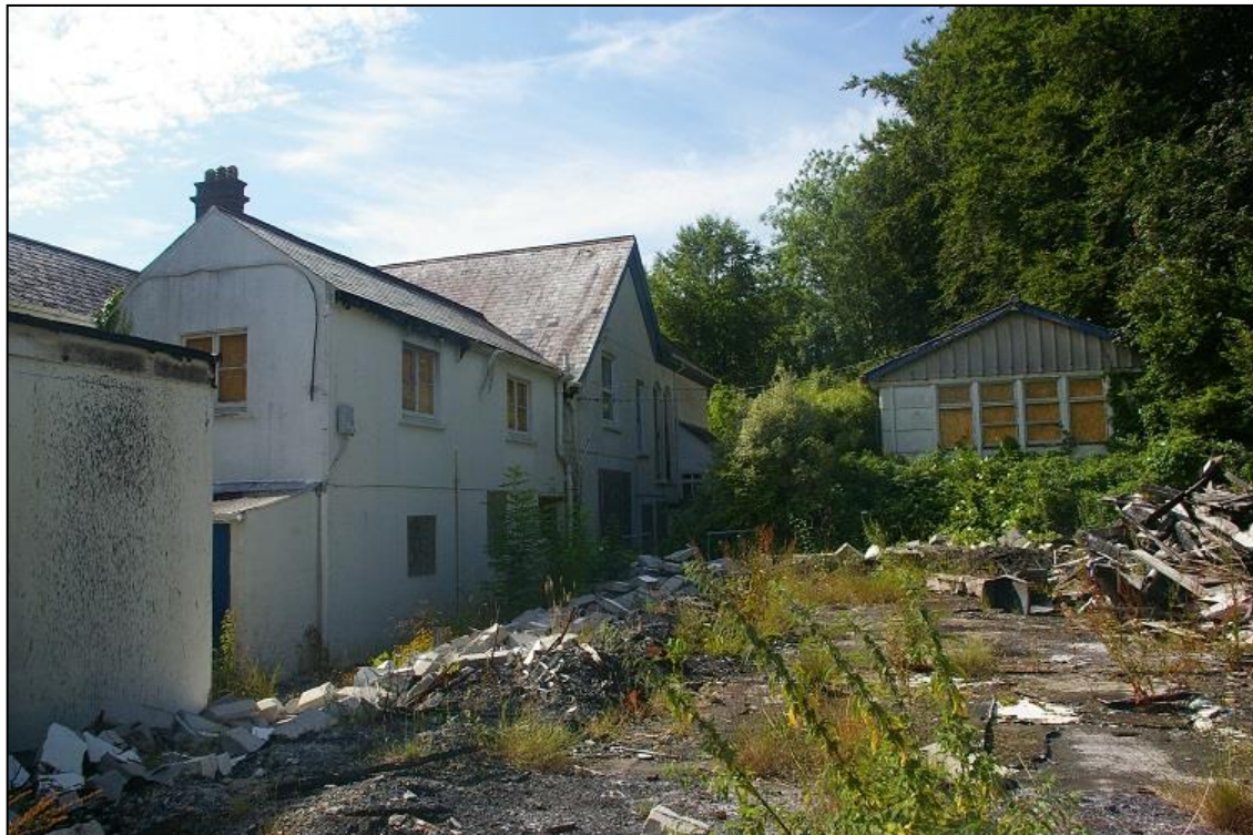
14. THE WEST ELEVATION OF THE HOUSE AND REAR SERVICE WING; FROM THE NORTH-NORTH-WEST.
