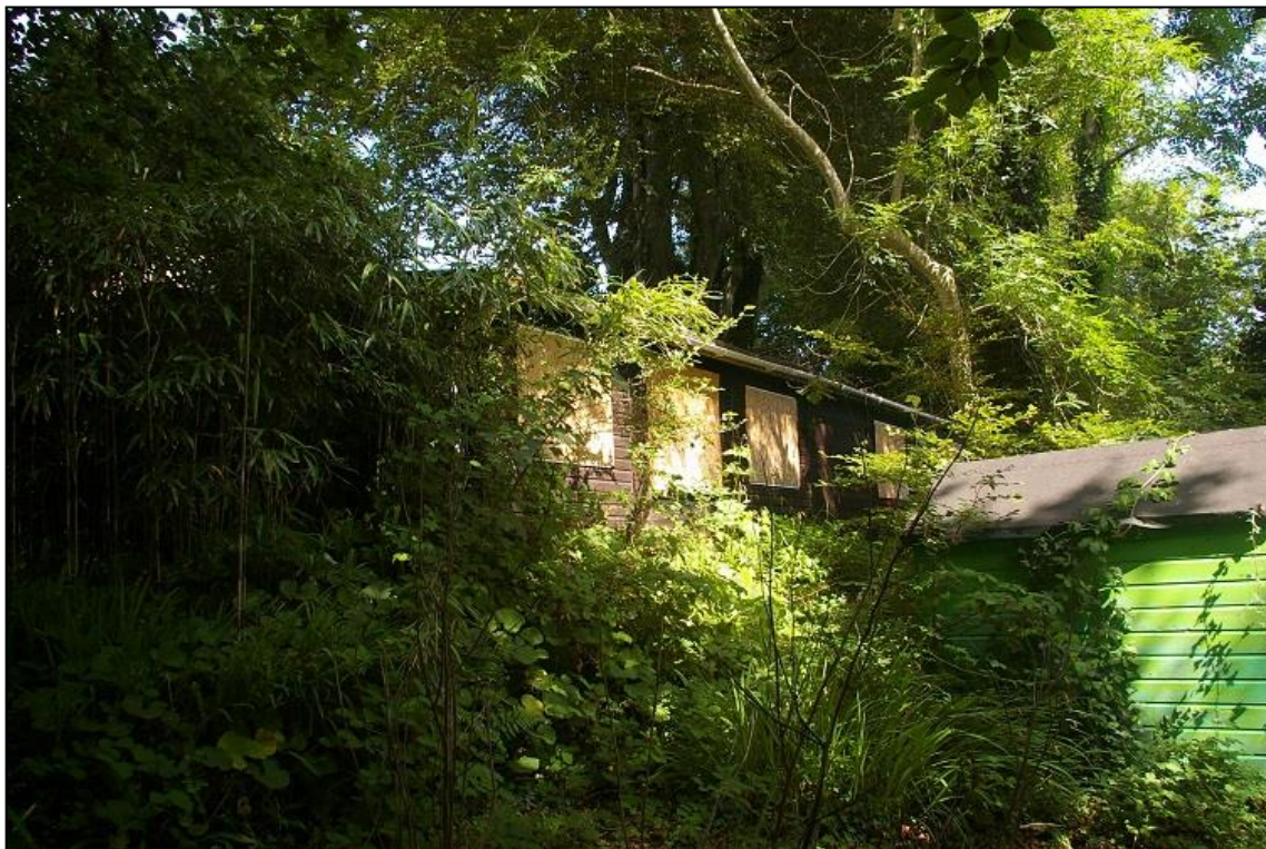
12. THE WOODEN TEMPORARY CLASSROOM TO THE WEST OF THE HOUSE; FROM THE SOUTH-EAST.
