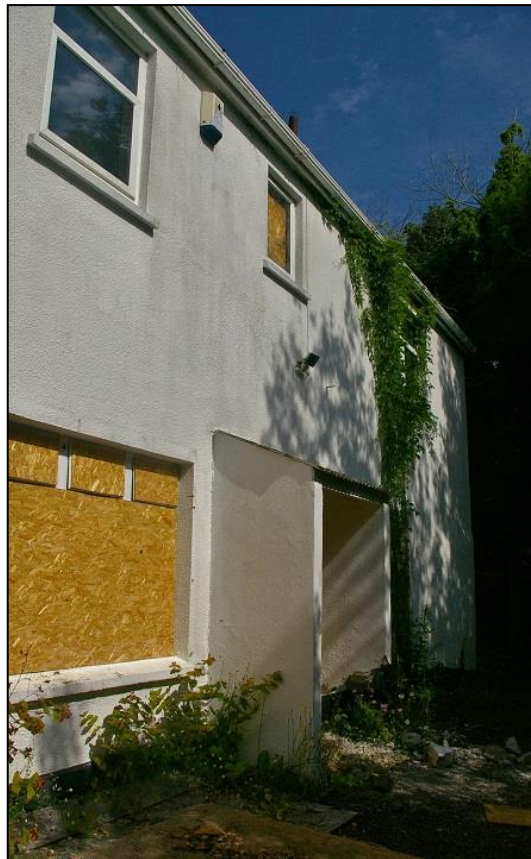
16. THE NORTH-EAST WING, WHICH HAS BEEN THOROUGHLY MODERNISED, THE EAST ELEVATION; FROM THE SOUTH-EAST.
