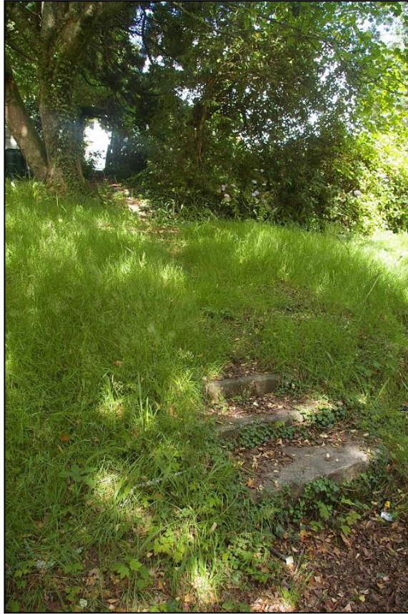
FIGURE 26: OVERGROWN STEPS BETWEEN THE HOUSE AND PARTERRE; FROM THE SOUTH-EAST.
