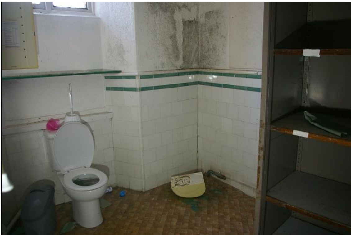
26. THE REAR ROOM OFF THE LANDING, WITH GOOD EARLY CERAMIC TILE SCHEME, POTENTIALLY AN EDWARDIAN BATHROOM; FROM THE SOUTH-WEST.
