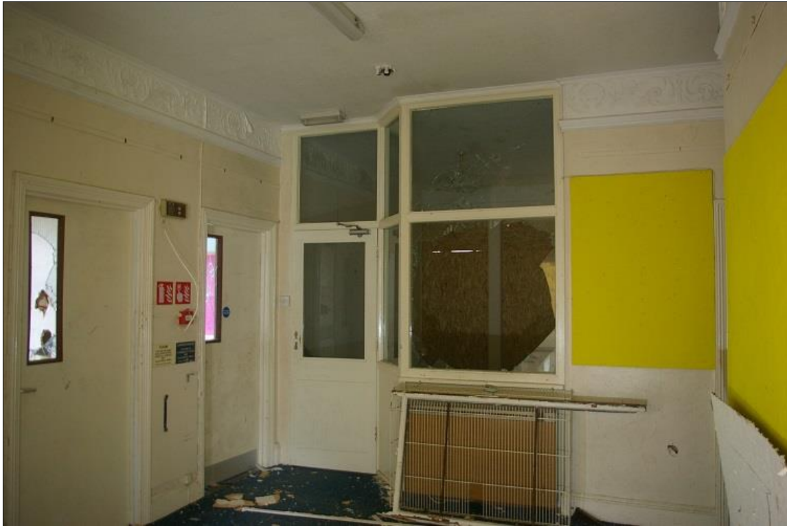
25. THE FIRST FLOOR LANDING WITH FIRE ESCAPE LOBBY BUILT ACROSS THE STAIRS; FROM THE EAST-NORTH-EAST.
