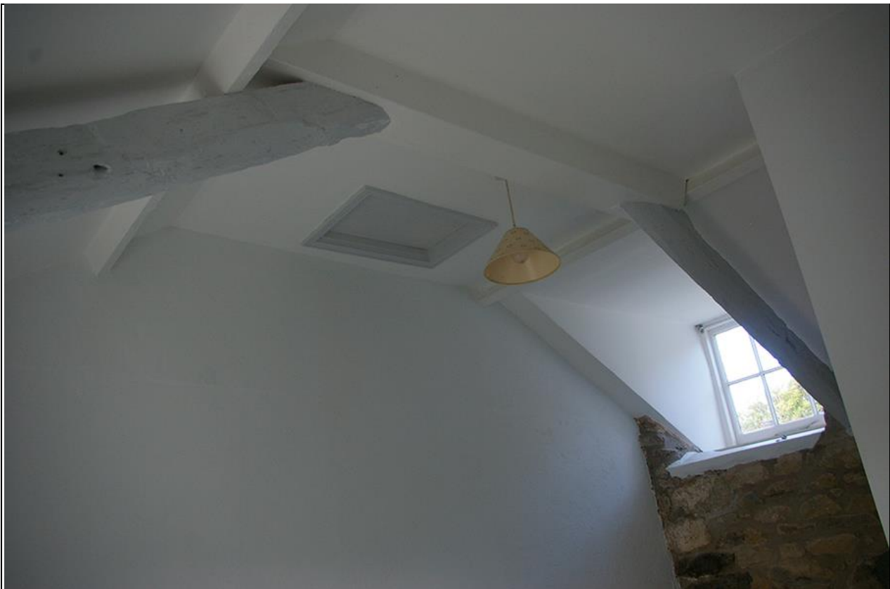
38. VIEW OF THE CEILINGS ON THE FIRST FLOOR – RAISED OVER THE RUSTIC TRUSSES ON A NEW ROOF STRUCTURE.
