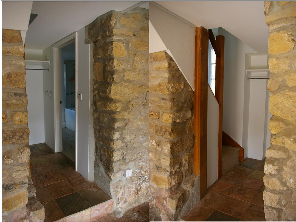
28. LEFT: VIEW INTO THE STAIR HALL, SHOWING THE FORCED OR ENLARGED OPENING IN THE BACK WALL; FROM THE SOUTH-WEST.
