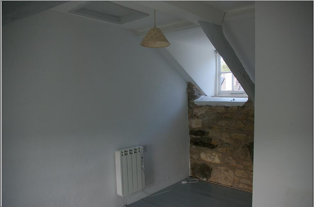
37. THE PLASTERED, RENOVATED END GABLE WALL – PROBABLY CONTAINING A BLOCKED FIREPLACE; FROM THE SOUTH-EAST.
