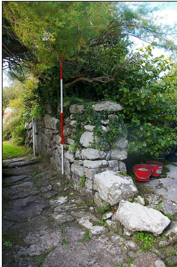
2. THE FRONT WALL OF THE RUINED SECTION OF BUILDING WEST OF THE COTTAGE, WITH 2M SCALE; FROM THE SOUTH-EAST.
