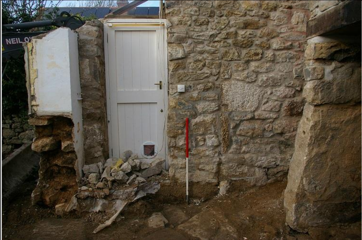
24. THE NORTH WALL OF R2 {067}, SHOWING THE STONE FLOOR ABUTTING THE NORTH WALL, WITH THE BLOCKED AND RE-CUT DOORWAY (1M SCALE); FROM THE SOUTH.
