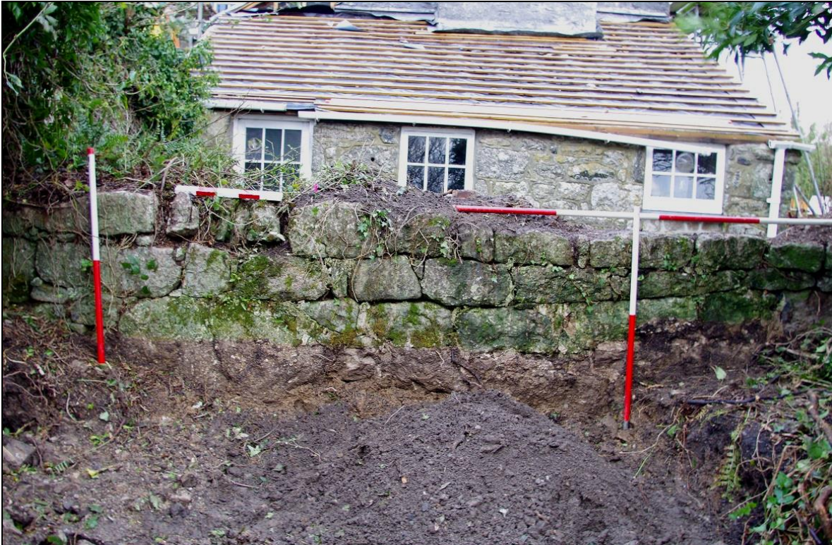
1. THE WEST WALL {041} OF THE RUIN, SHOWING THE WINDOW AND BLOCKED DOORWAY; FROM THE WEST (1M AND 2M SCALES).
