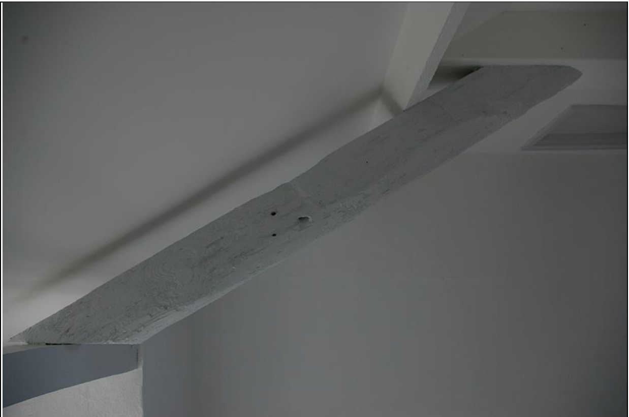
36. DETAIL OF THE RUSTIC A-FRAME OF THE ROOF, WITH HOLES WHERE COLLAR HAS BEEN REMOVED, WITH SPIKE HOLES AND A PEG HOLE; FROM THE EAST.
