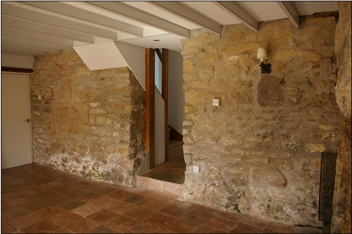
FIGURE 16: THE REAR WALL OF BUILDING 1, THE 18 TH CENTURY COTTAGE, SHOWING BLOCKED OPENINGS AND STRUCTURAL PHASING; THE EVIDENTIAL VALUE OF THE BUILDING BEING HIGH. PHOTOGRAPH TAKEN FROM THE EAST-NORTH-EAST.
