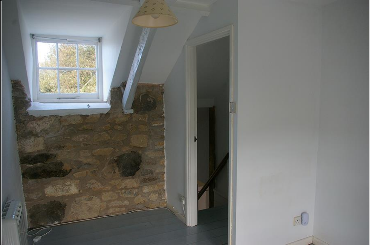
35. ROOM 8, WITH STONE WALL EXPOSED TO REAR, WITH RUSTIC A-FRAME TRUSS — MODERN PARTITIONS FORM R7, THE LANDING; FROM THE SOUTH-WEST.
