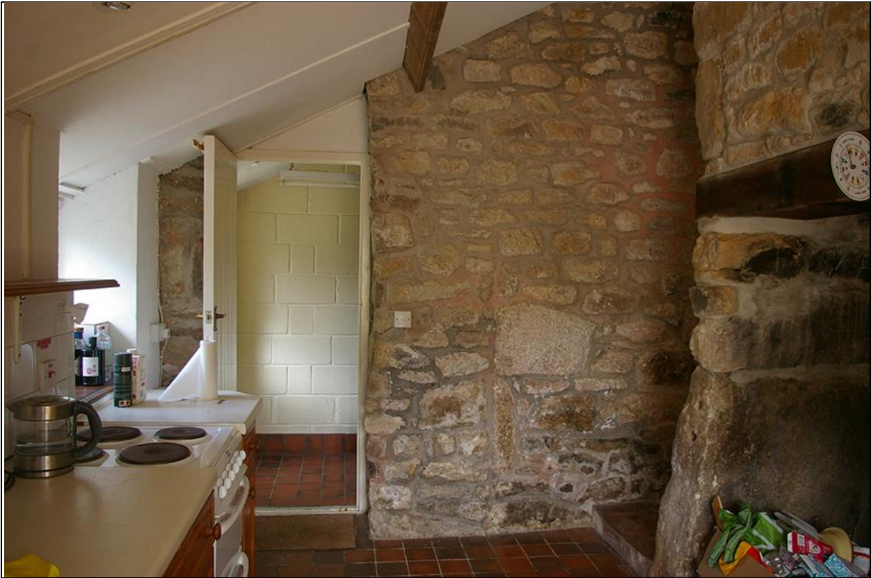
25. ROOM 2 , THE KITCHEN, SHOWING THE REAR WALL, WITH BLOCKED AND RE-CUT DOORWAY; FROM THE SOUTH-WEST.
