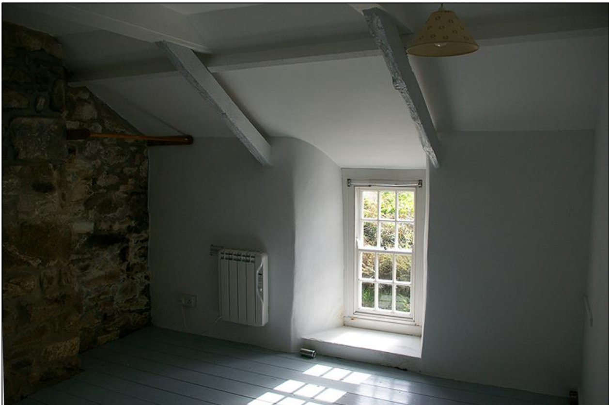
42. THE FRONT SOUTH WALL OF R9, AGAIN SHOWING ENLARGED WINDOW OPENING, CUT UP AT THE EAVES AND RUSTIC TRUSSES; FROM THE NORTH-WEST.
