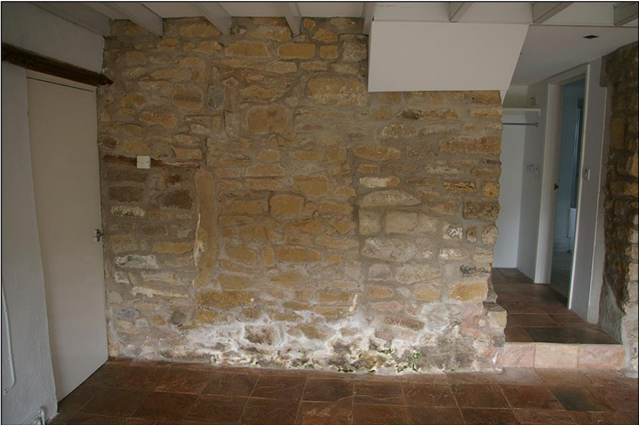
18. ROOM 1, THE BLOCKED OPENING AND BUILD LINES IN THE REAR WALL OF THE COTTAGE; FROM THE SOUTH.
