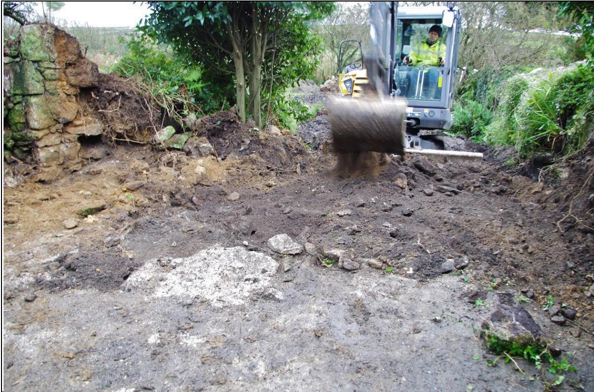
THE WEST WALL {041} OF THE RUIN BEING DEMOLISHED, WORKING SHOT; FROM THE EAST-NORTH-EAST.
