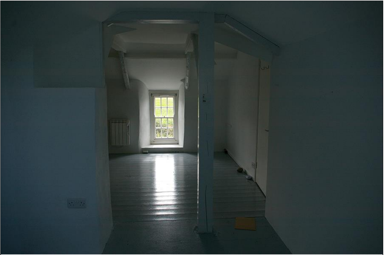
45. LOOKING THROUGH THE LARGE OPENING FORCED IN THE REAR WALL, FROM R10 TO R9; FROM THE NORTH.
