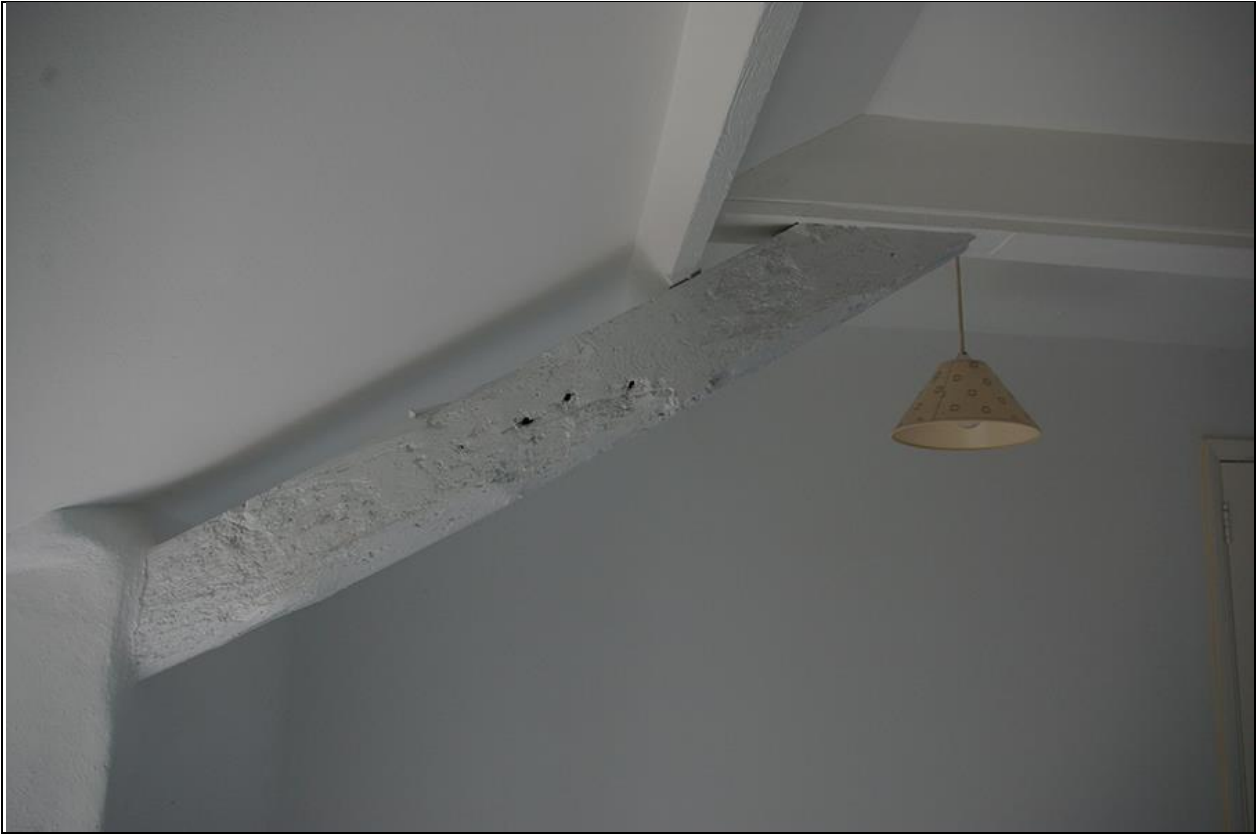
41. DETAIL OF THE TRUSS IN R9, AGAIN SHOWING HOLES FROM TURNED OVER SPIKES, FROM THE REMOVED COLLAR; FROM THE SOUTH-EAST.
