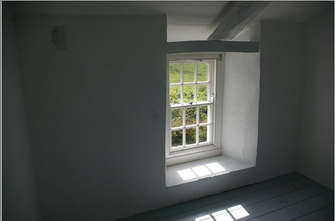
39. THE WINDOW OPENING IN R8, SHOWING DISTURBED REVEALS, SUGGESTIVE OF SLIGHT WIDENING WITHIN THE ROOM AND DEFINITE RAISING/REMOVAL OF THE EAVES, HENCE THE AWKWARD RELATIONSHIP WITH THE ORIGINAL ROOF TRUSS; FROM THE NORTH-NORTH-EAST.
