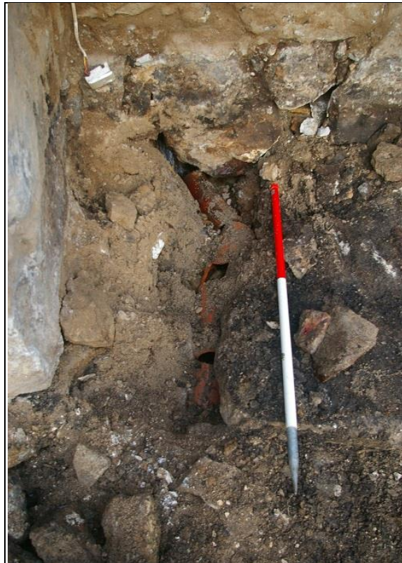
29. THE DRAIN WITH TERRACOTTA 19 TH CENTURY PIPES INSERTED, WHICH HAS COLLAPSED DURING CLEARANCE; FROM THE WEST (1M SCALE).
