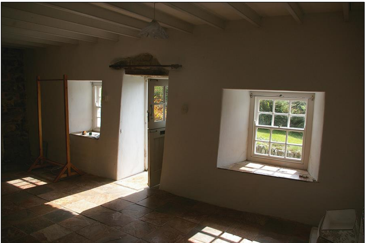
17. ROOM 1, SHOWING THE BATTERED FRONT SOUTH WALL; FROM THE NORTH-WEST.
