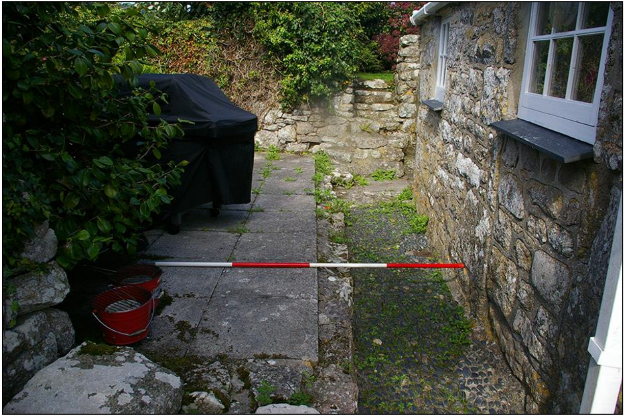
9. THE COBBLED PATH AND CONCRETE PATIO, WEST OF THE LEAN-TO; FROM THE WEST (2M SCALE).
