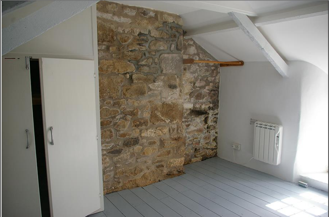
43. R9, THE LARGE HISTORIC STACK, HEAVILY RE-POINTED, THERE DOESN'T APPEAR TO BE A CLEAR BUILD LINE HERE FOR ANY BLOCKED FIREPLACE – SUGGESTING AN UNHEATED FIRST FLOOR FOR THIS SPACE; FROM THE WEST-NORTH-WEST.
