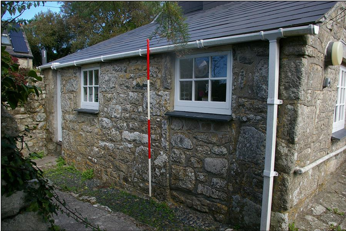
7. THE LEAN-TO, BUILDING 2, WITH 2M SCALE; FROM THE SOUTH-WEST, SHOWING BLOCKED DOORWAY.
