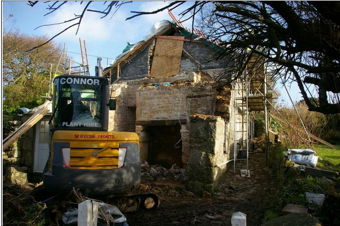
20. WORKING SHOT OF THE DEMOLITION OF B2, THE LEAN-TO; FROM THE WEST-SOUTH-WEST.
