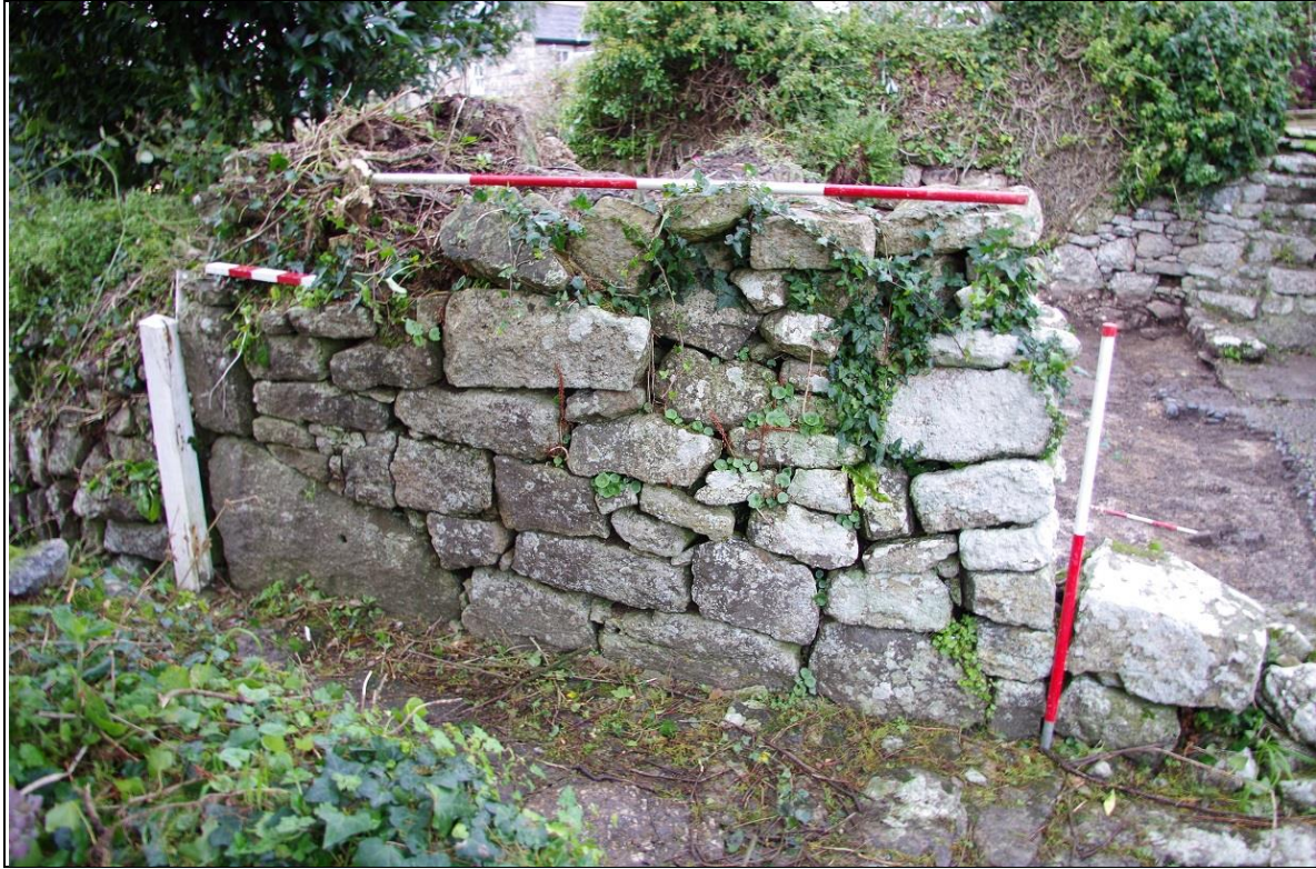
3. THE FRONT GARDEN WALL BANK {084}, DURING DEMOLITION; FROM THE SOUTH-EAST (2M, 1M AND 0.5M SCALES).
