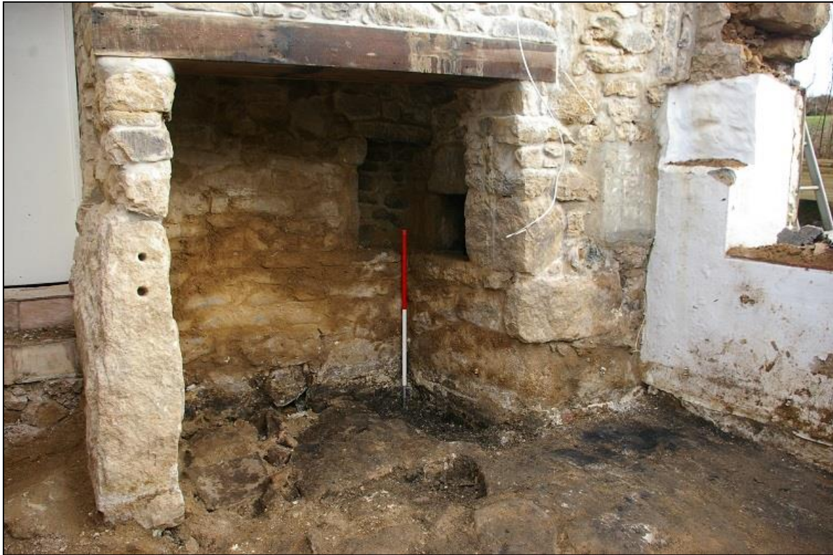
22. DETAILED VIEW OF THE FIREPLACE, WITH BREAD OVEN, BLOCKED KEEPING PLACE AND BLOCKED FIREPLACE AT FIRST FLOOR (1M SCALE); FROM THE NORTH-WEST.
