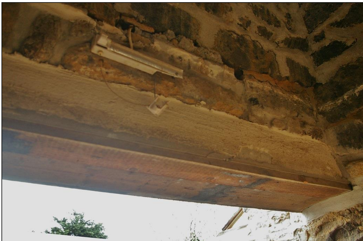
23. THE CONCRETE BEAM AND REBUILT SECTIONS OF THE STACK WHICH INDICATES A LINTEL HAS BEEN REMOVED AND A NEW LINTEL INSTALLED AT A MUCH HIGHER LEVEL; FROM THE SOUTH-EAST.
