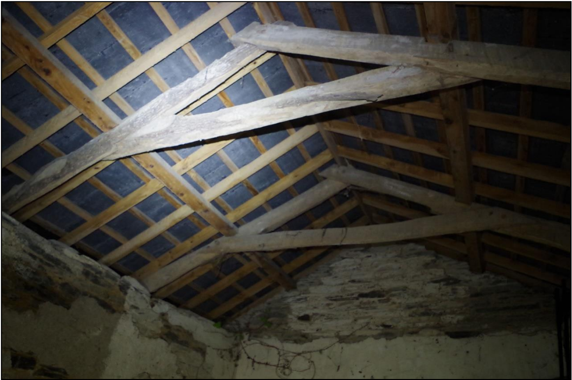
3. THE GOOD, ORIGINAL A FRAME TRUSSES TO B1C. VIEWED FROM THE WEST.
