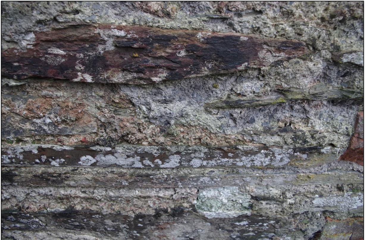
FIGURE 15: PICTURE OF THE STONEMWORK AND LIME AND SLATE REPOINTING TO THE WEST ELEVATION OF B1.
