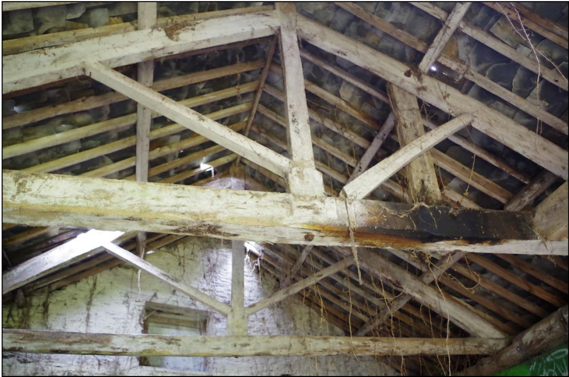
11. BOLTED KING POST TRUSSES WITH QUEEN STRUTS IN B2, MID-LATE 19 TH CENTURY.
