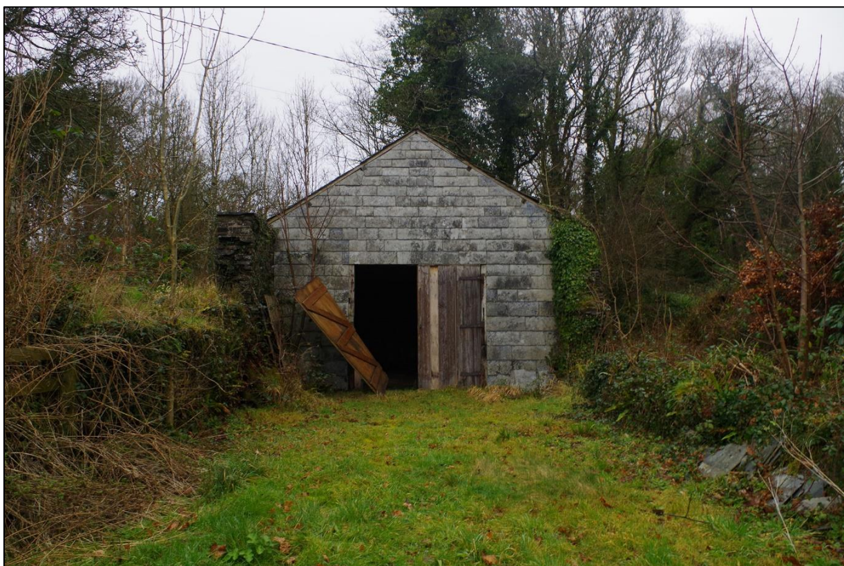
FIGURE 12: THE SOUTH ELEVATION OF B2, WITH SLATE CLADDING, OVERGROWN AND RUINOUS SURVIVING SECTIONS OF B2A RUNNING FURTHER SOUTH. TAKEN FROM THE SOUTH-WEST.
