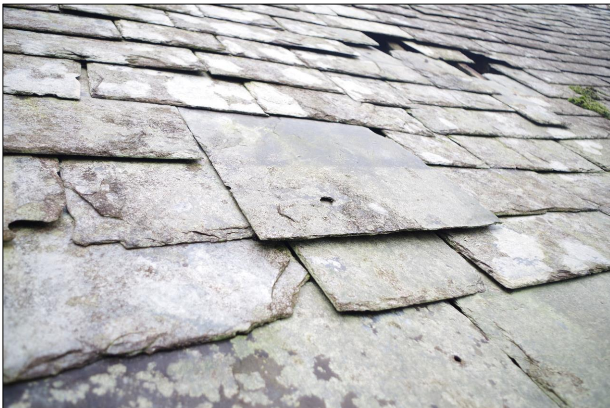
FIGURE 16: BARN 2 RETAINED AN ORIGINAL SLATE ROOF, COMPLETE WITH VERY LARGE, SQUARE SLATE TILES WITH NEATLY PUNCHED HOLES FOR TACKS. TAKEN FROM THE NORTH-WEST LOOKING AT THE WESTERN RIDGE.
