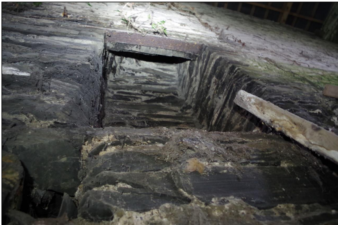
8. FIRST FLOOR CHIMNEY FLUE TO B1D, STACK WAS REMOVED WHEN ROOF WAS REPLACED.
