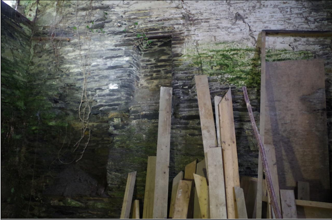
7. THE SURVIVING FLUE HOLES TO FIRST FLOOR AND GROUND FLOOR IN B1D, VIEWED FROM THE WEST.
