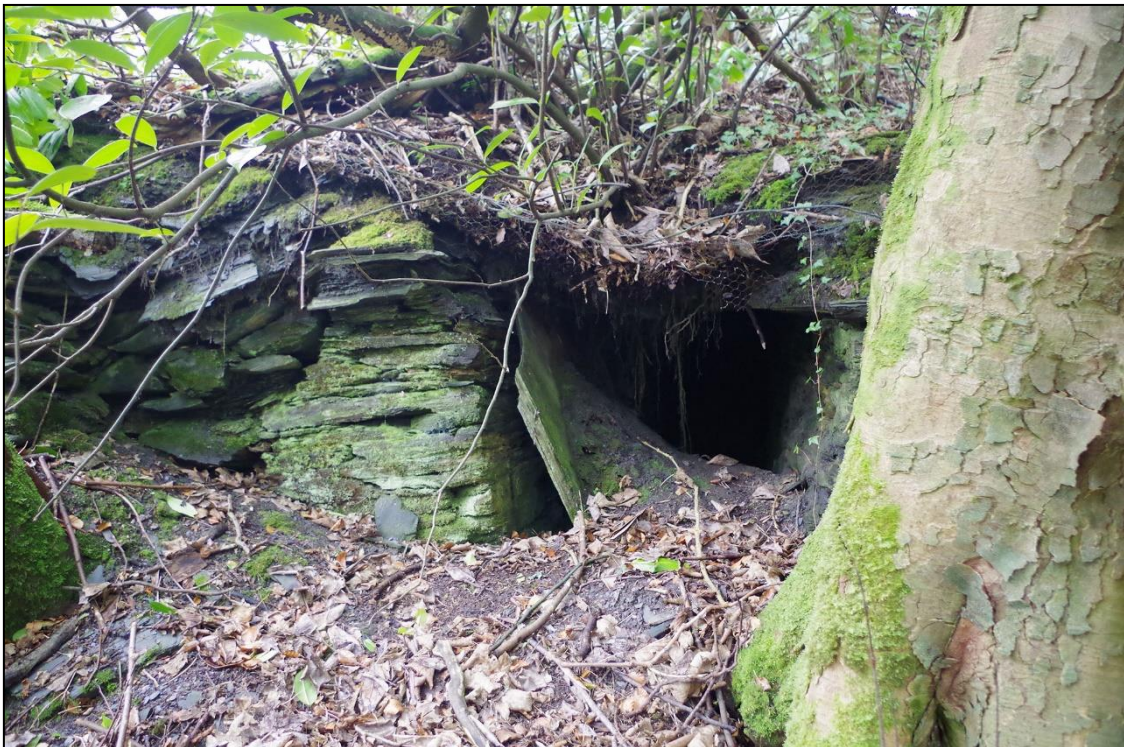
14. FORMER STRUCTURES ASSOCIATED WITH WATERWORKS SITTING BELOW POND TO THE EAST, THIS STRUCTURE APPEARS ON EARLIER MAPPING. VIEWED FROM THE SOUTH.
