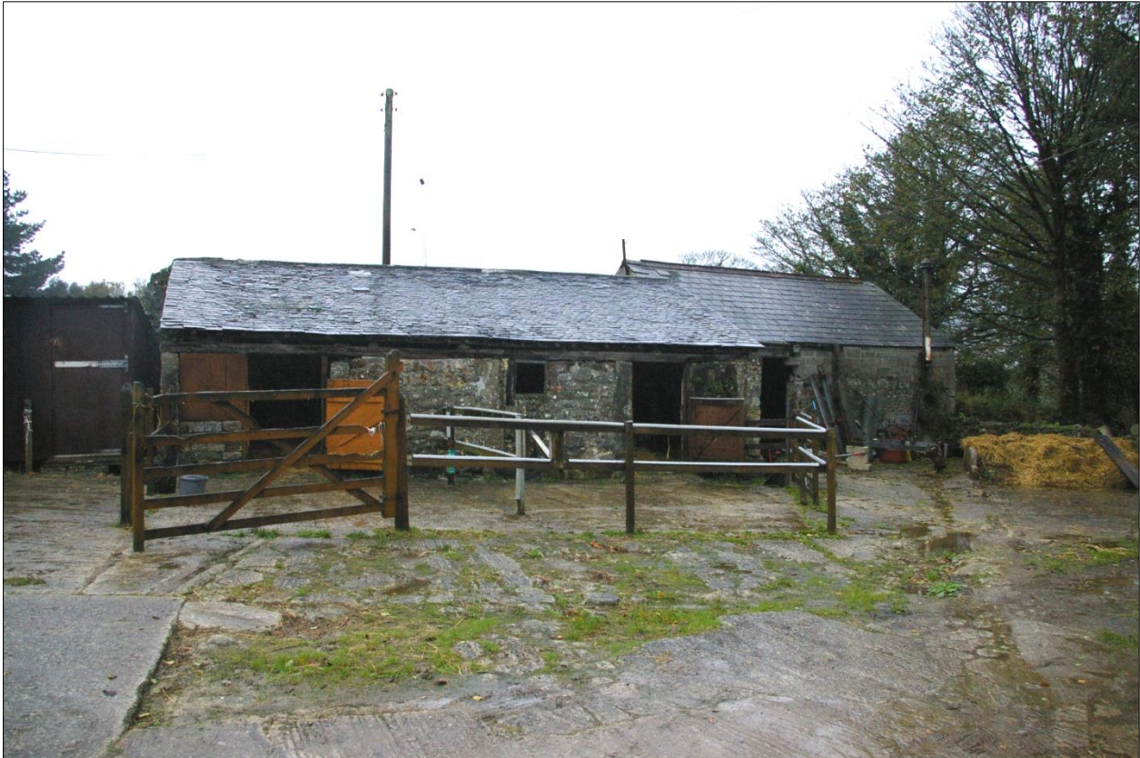
Trehiddle Farm: sheds north of the farm, including a former open-fronted shed; viewed from the south, looking north.
