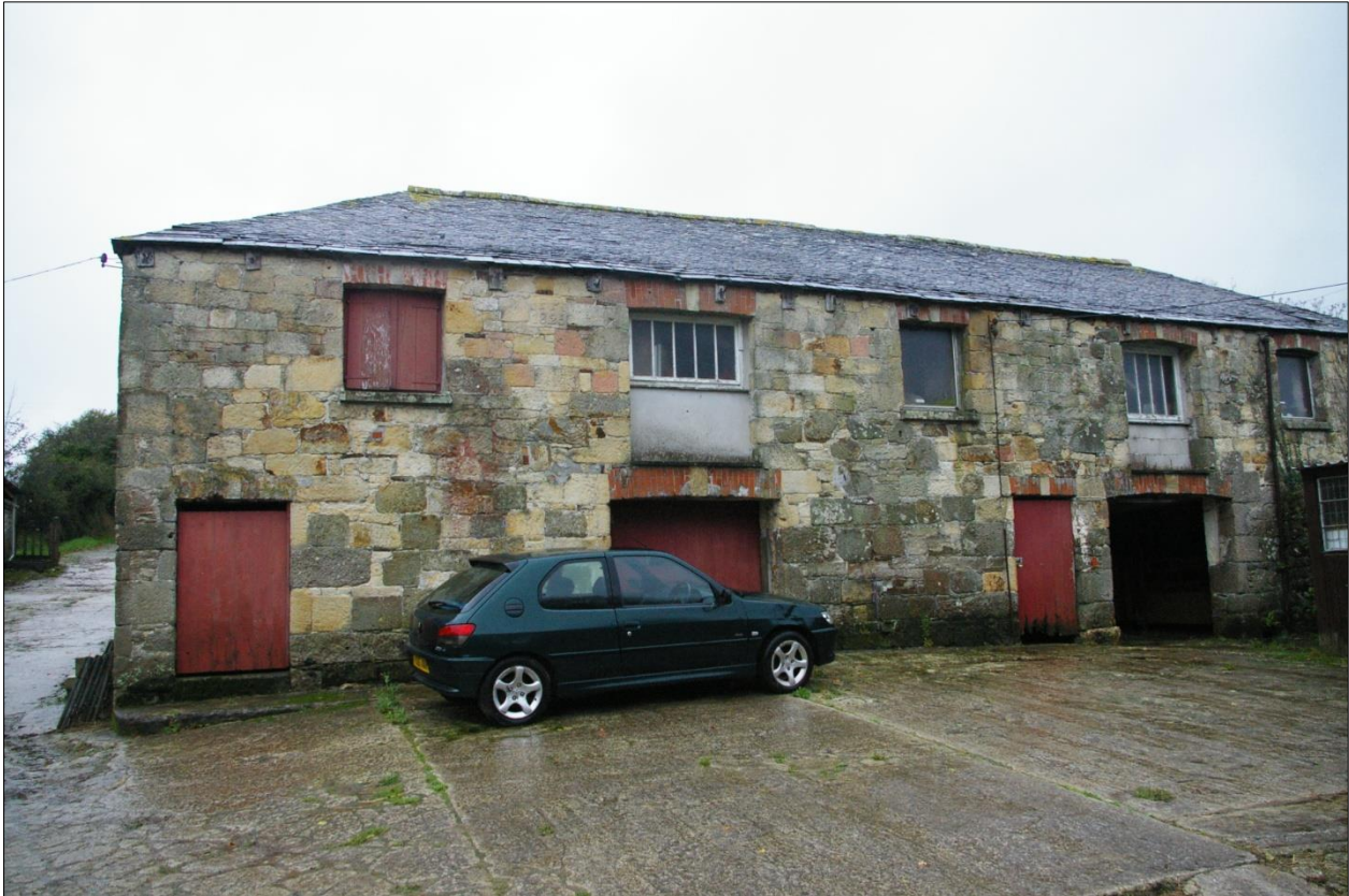
Trehiddle Farm: east elevation of the bank barn; viewed from the east.
