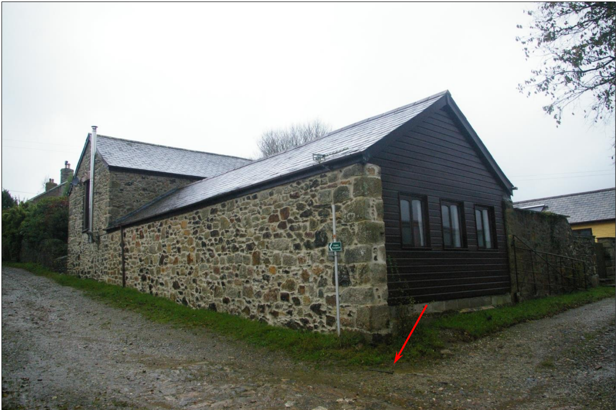
As above, viewed from the south-east, looking north-west. The iron waterpipe – probably the one identified in the geophysical survey – is indicated.
