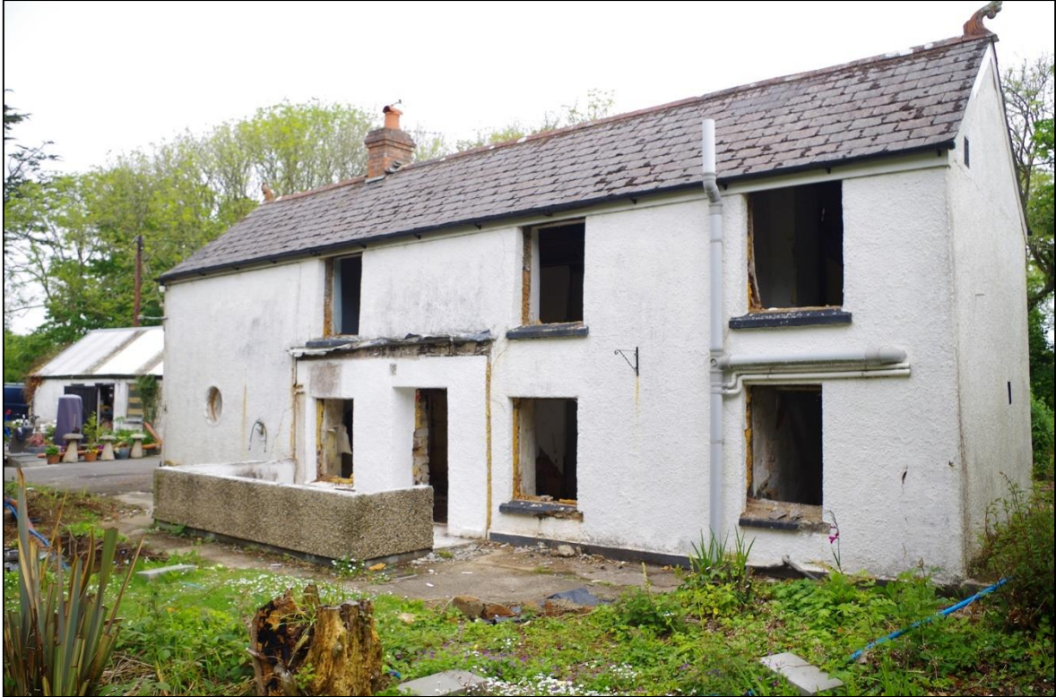
FIGURE 8: THE SOUTH ELEVATION, SHOWING MODERN EXTENSIONS, AMONGST AN EARLIER COB BUILD, THE EAST END IS BATTERED. TAKEN FROM THE SOUTH-EAST.
