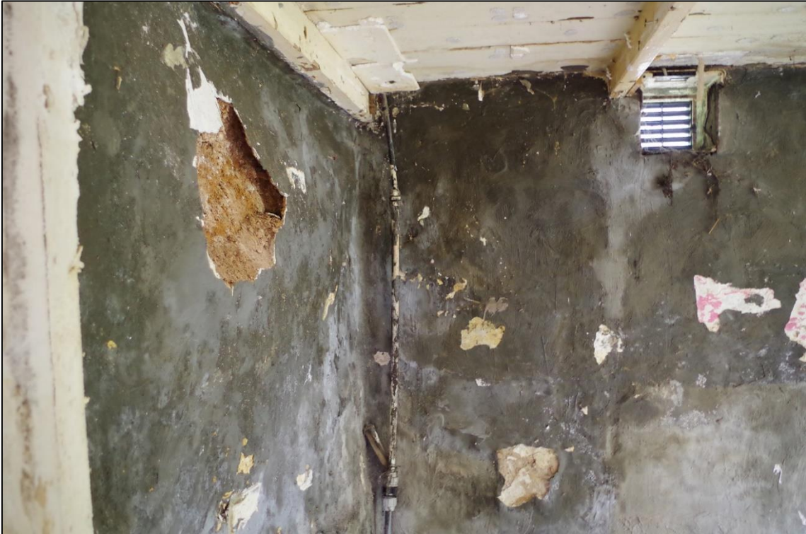
FIGURE 10: BATTERED COB WALLS WITHIN THE EAST EXTENSION, AND EVEN-WIDTH PLANKED FLOOR TO FIRST FLOOR, WITH CHAMFERED JOISTS -KEY 19TH CENTURY DETAILS. TAKEN FROM THE WEST.
