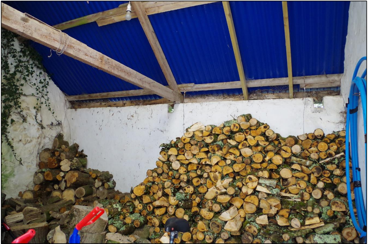
FIGURE 14: SOCKET HOLES SHOW THE OUTBUILDING HAS CHANGED USE AND DEVELOPED OVER ITS PERIOD, AND SUGGEST A CHANGE OF PITCH FOR THE BUILDING. IT IS CLEAR THE ROOF HAS BEEN REPLACED, LIKELY TWICE, EARLY-MID 20 TH HALF-LAPPED TRUSSES AND LATER EARLY 21 ST PLASTIC CORRUGATED ROOF, WITH SIMPLE PINE A-FRAMES AND RAFTERS.
