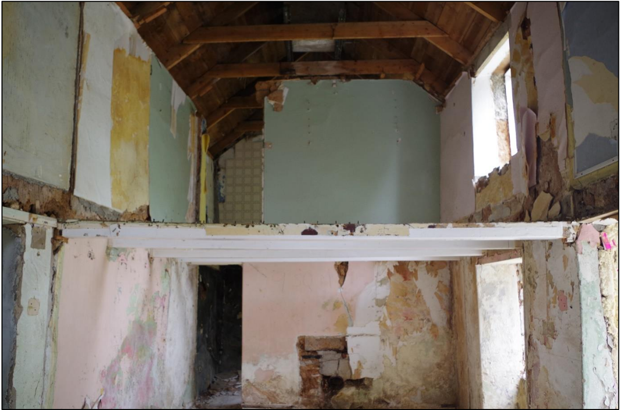
FIGURE 9: R3 INCLUDES THE MAJORITY OF COB WALLS WITHIN THE BUILD AND CUT HISTORIC STACK, AND BLOCKED FIREPLACE BELOW. TAKEN FROM THE WEST.
