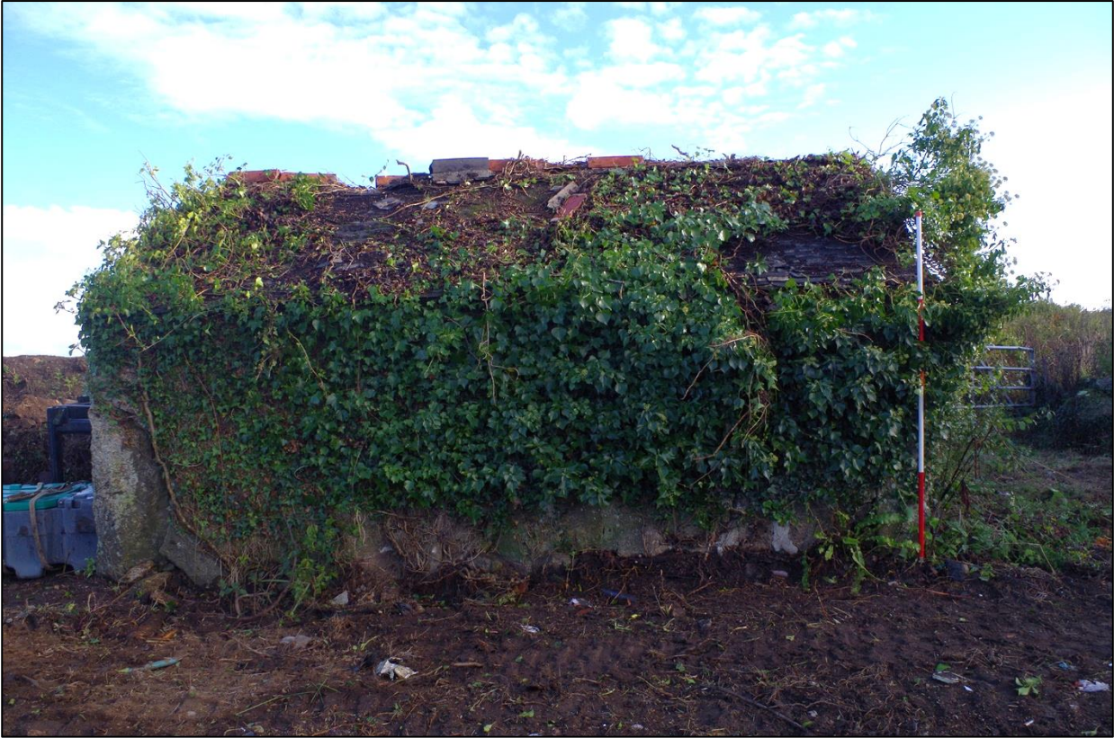
96. B3 SOUTH EXTERNAL ELEVATION, OVERGROWN SHRUBBERY HIDING STONWORK DETAILS; VIEWED FROM THE SOUTH (2M SCALES).
