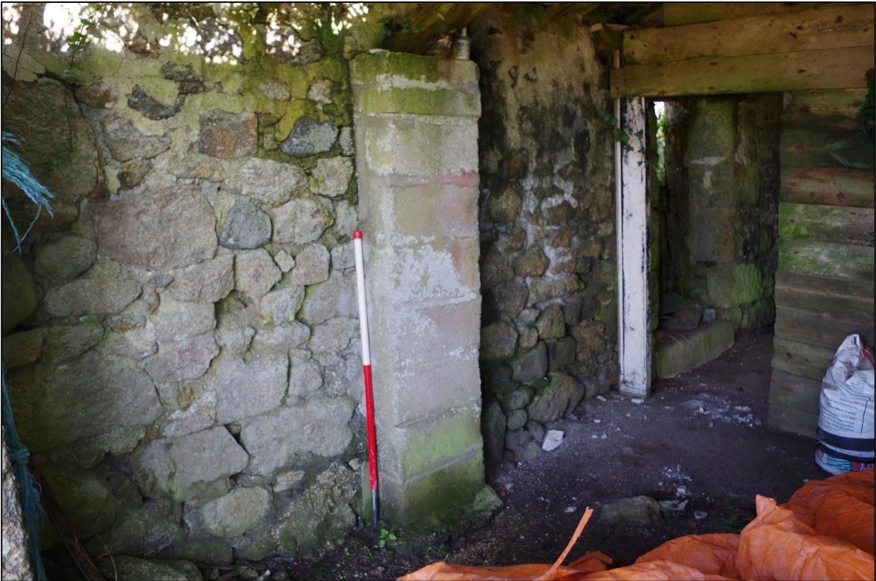
18. B1A, NORTH INTERNAL ELEVATION, SHOWING SECTION OF REBUILD AND MODERN CONCRETE BUTTRESS; VIEWED FROM THE WEST (SCALE 1M).
