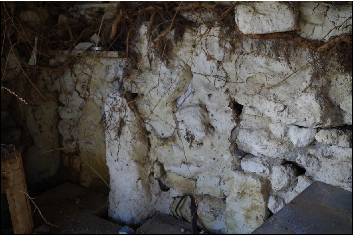
106. B3 SOUTH-EAST CORNER, SMALL GATE POSTS REUSED, POSS. BLOCKED OPENINGS; VIEWED FROM THE NNW.
