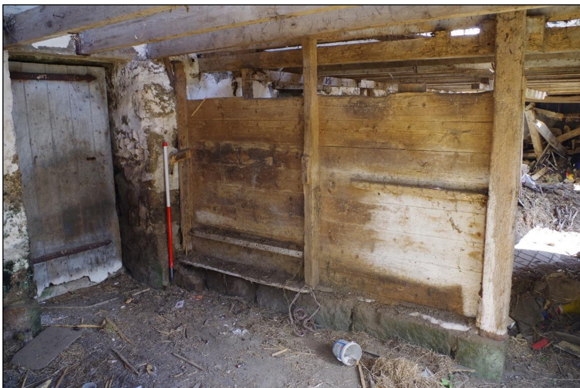
FIGURE 13: D5 LEADING FROM B1B (ONLY DOOR FITTING SURVIVING TO SITE), AND THE TIMBER PARTITION ALONG EAST ELEVATION OF B1C ON A SINGLE RUSTIC COURSE OF GRANITE BLOCK; FROM THE SOUTH-WEST (1M SCALE).
