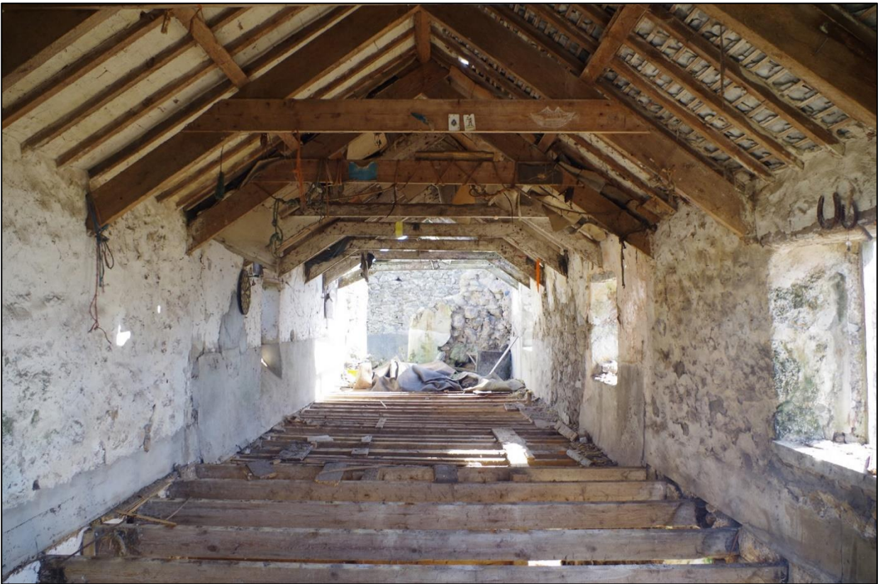
59. B1C & B1D FF LEVEL, CEILING STRIPPED AND COLLAPSE TO EAST END; VIEWED FROM D12 FROM WEST.
