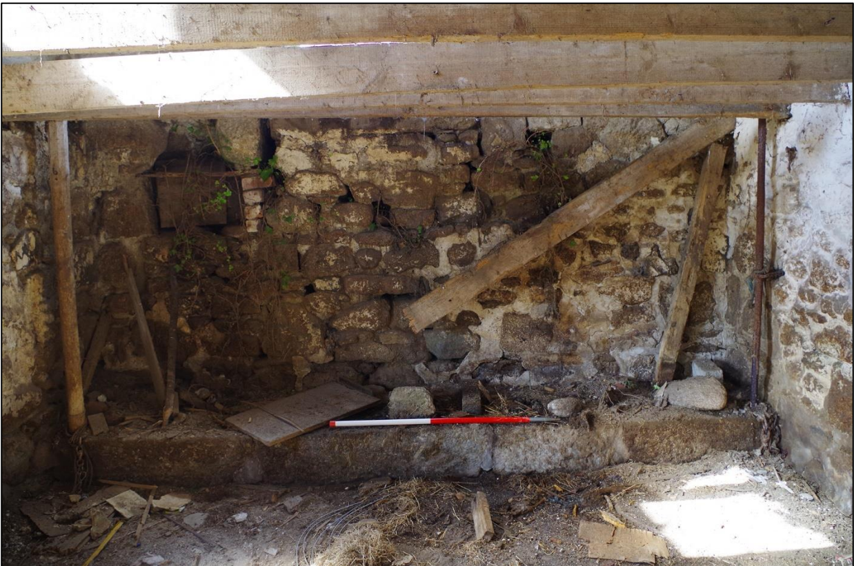
33. B1C, WEST INTERNAL ELEVATION, INCLUDING BLOCKED OPENING TO SOUTH AND POSSIBLE BLOCKED GF DOORWAY; VIEWED FROM THE EAST (SCALE 1M).
