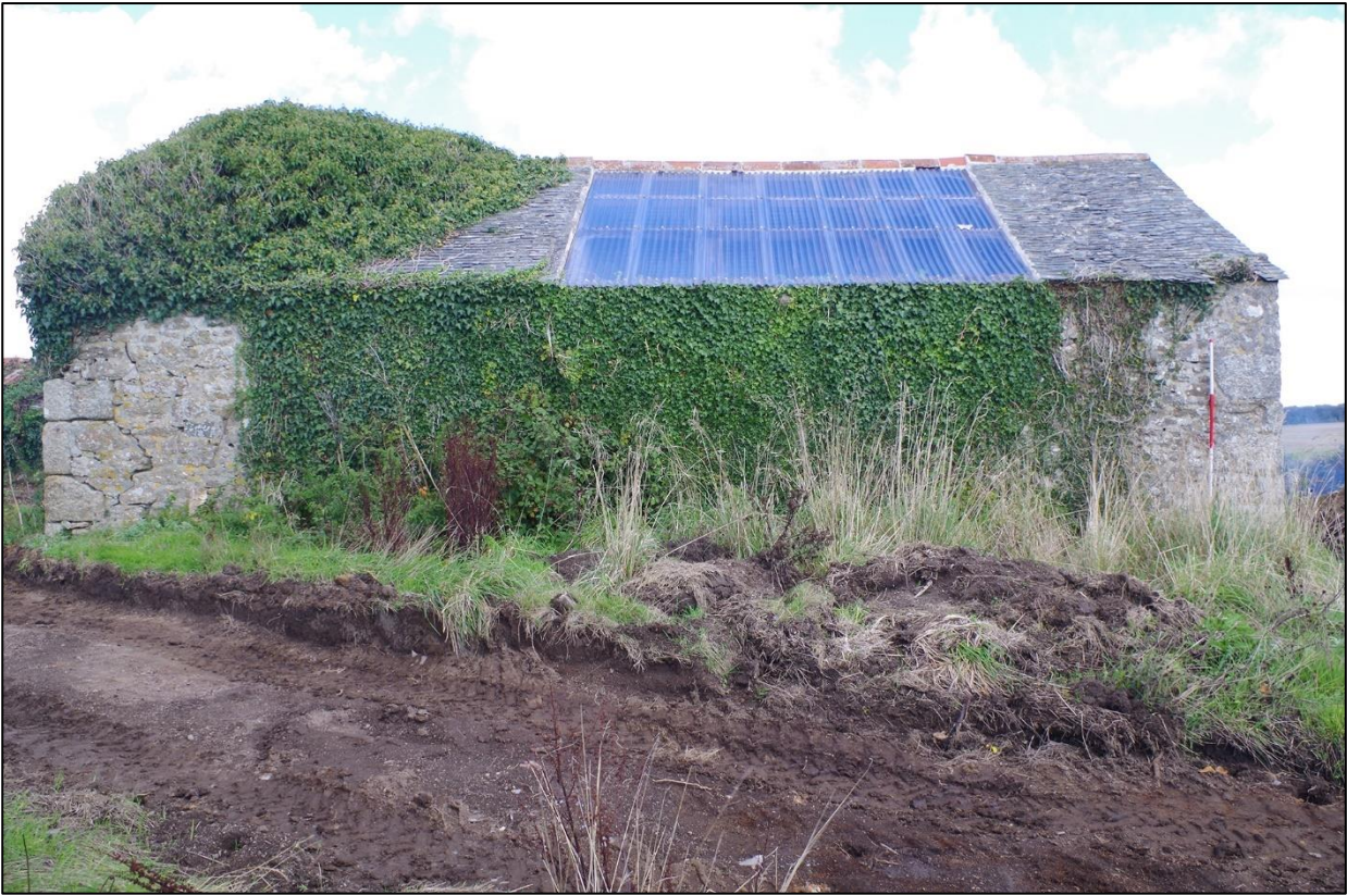
63. B2, THE SOUTH ELEVATION, SOUTH PITCH HEAVILY MODIFIED; VIEWED FROM THE SOUTH (SCALE 2M).
