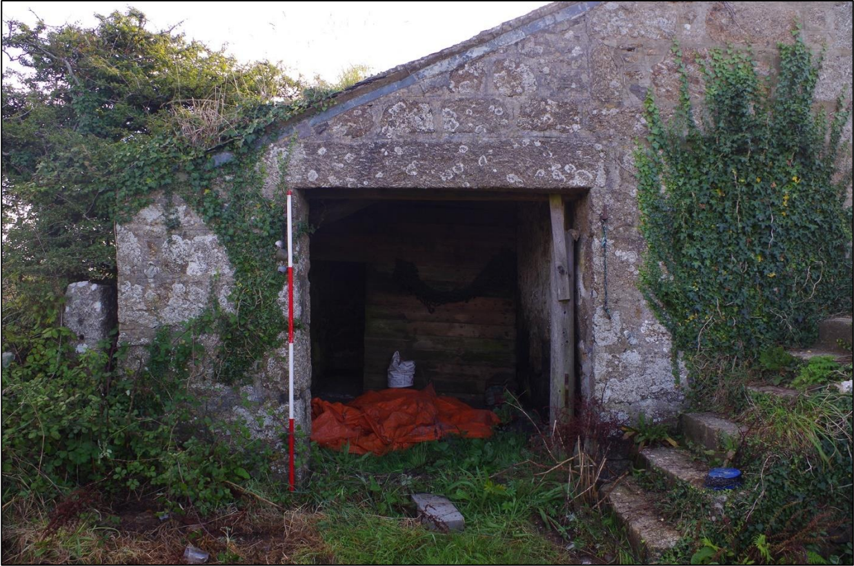
5. B1A WEST ENTRANCE WITH DOUBLE-WIDTH OPENING, INC BASE OF GRANARY STEPS; VIEWED FROM THE WEST (SCALE 2M).
