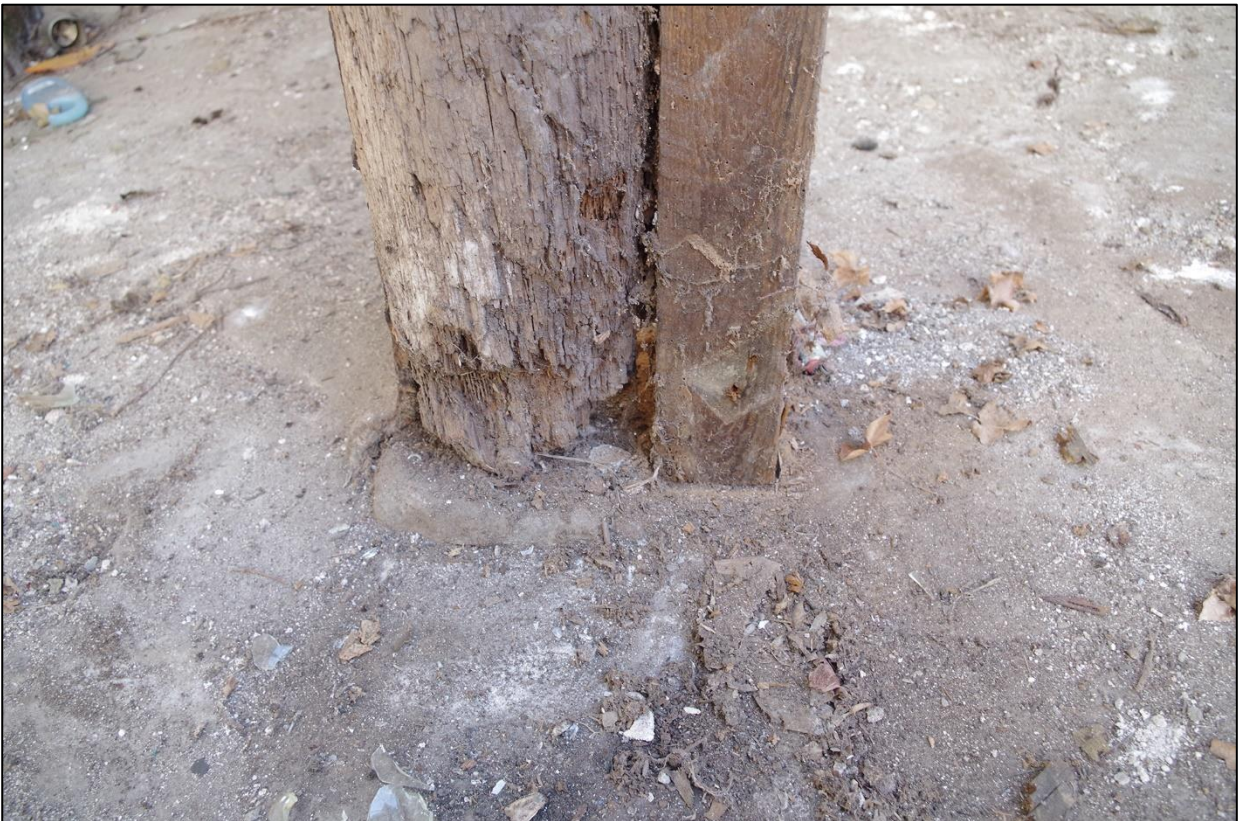
81. B2A, TIMBER POST BRACING ALTERED TRUSS SAT ON STONE PAD FOR EARLIER PARTITION; VIEWED FROM THE EAST.
