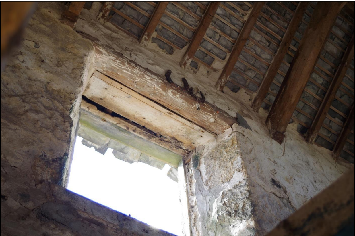
37. B1C, W10 TO FF WEST END, WITH GRANITE SPLAYED EMBRASURES AND TIMBER LINTEL; VIEWED FROM GF LEVEL.
