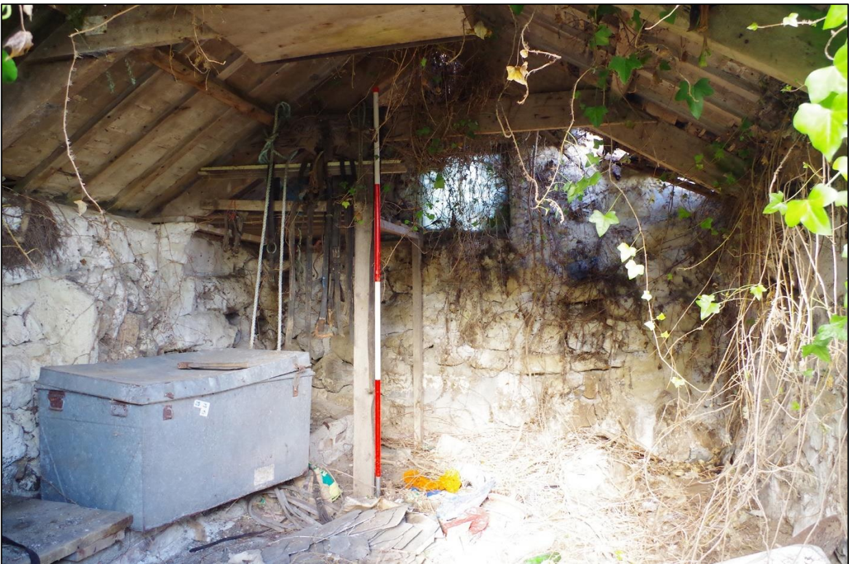
99. B3, THE WEST INTERNAL ELEVATION SHOWING ROOF STRUCTURE AND MIXED BUILD; VIEWED FROM EAST (2M SCALES).
