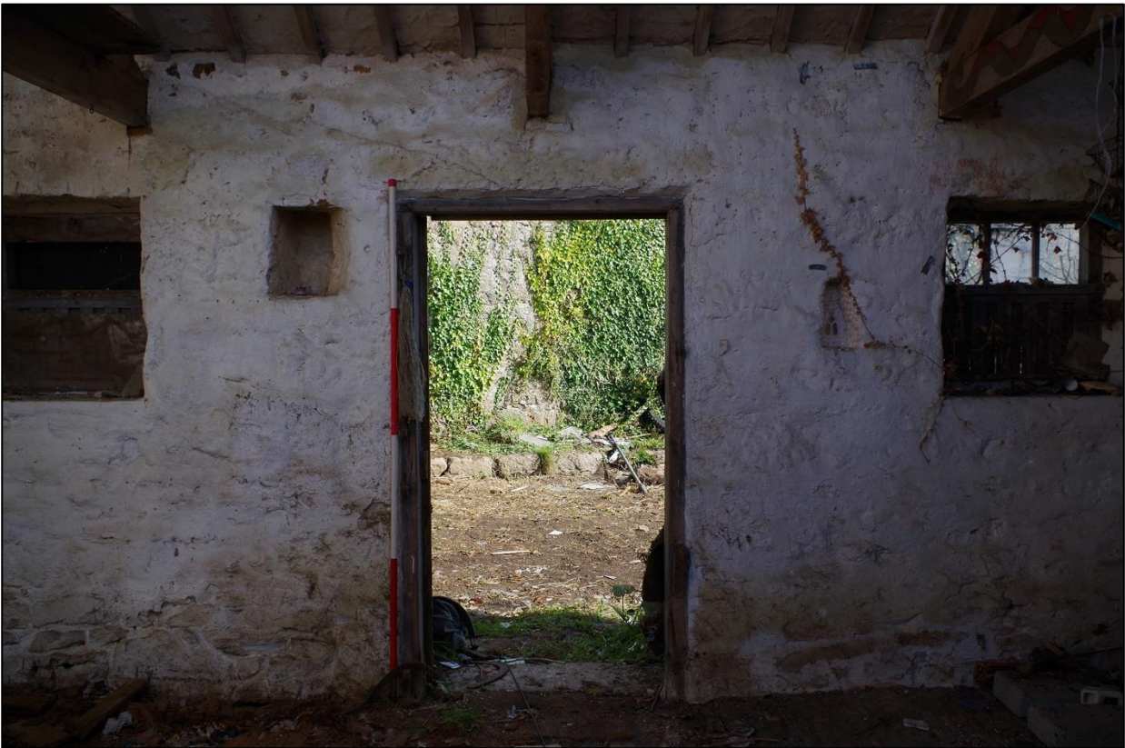
68. B2A, NORTH ELEVATION SHOWING W16, W17 & D13; VIEWED FROM THE SOUTH (SCALE 2M).
