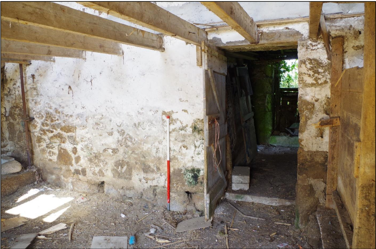
26. B1C, THE NORTH INTERNAL ELEVATION WITH D5 LOOKING THROUGH TO B1B; VIEWED FROM THE SOUTH (SCALE 1M).
