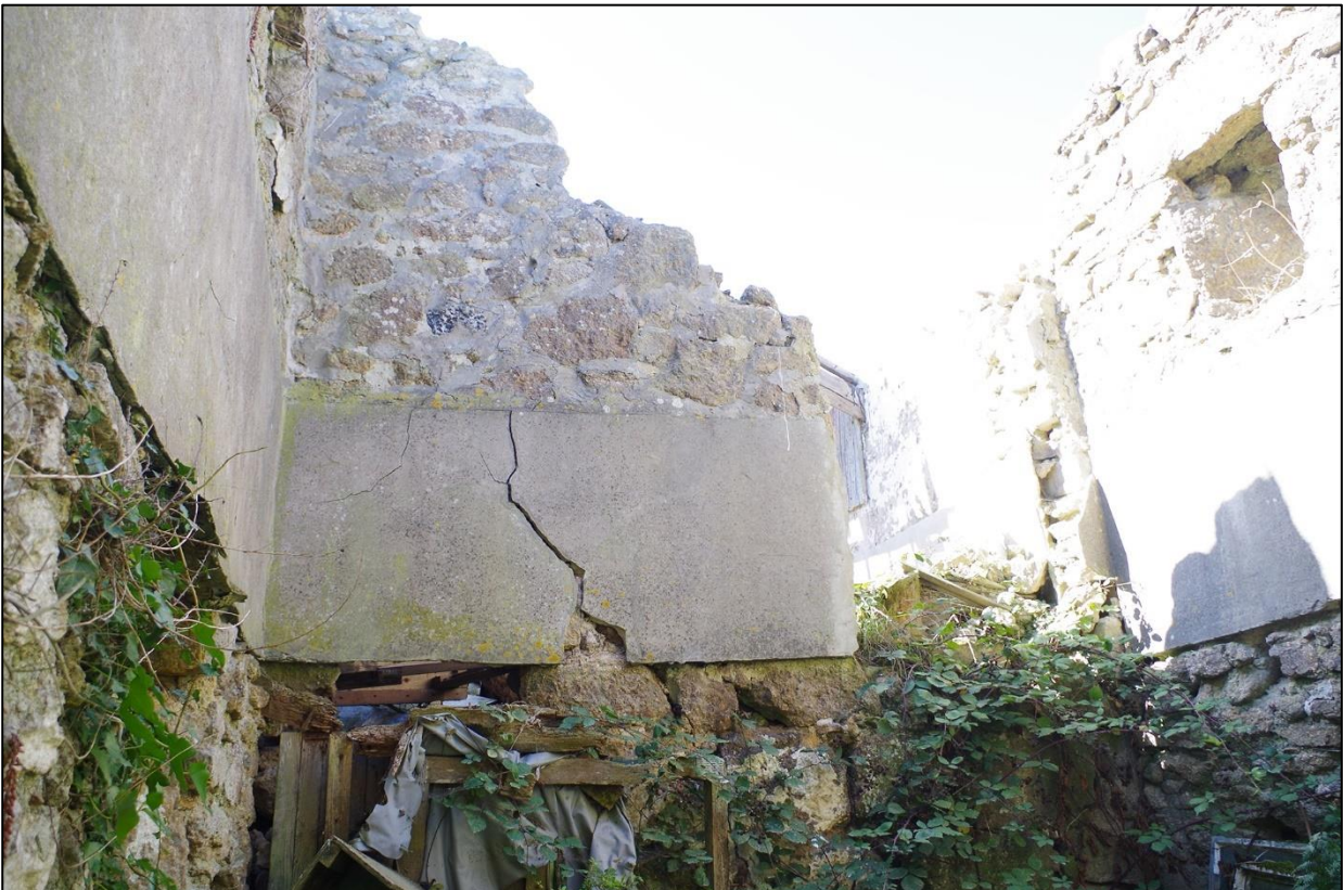
57. B1E, WEST GABLE ELEVATION, SUFFERED LARGE COLLAPSE, HARD TO DECIPHER FEATURES TO GF DUE TO UNSTABLE RUBBLE, BUT HEAVIER BUILD TO BASE IS VISIBLE.
