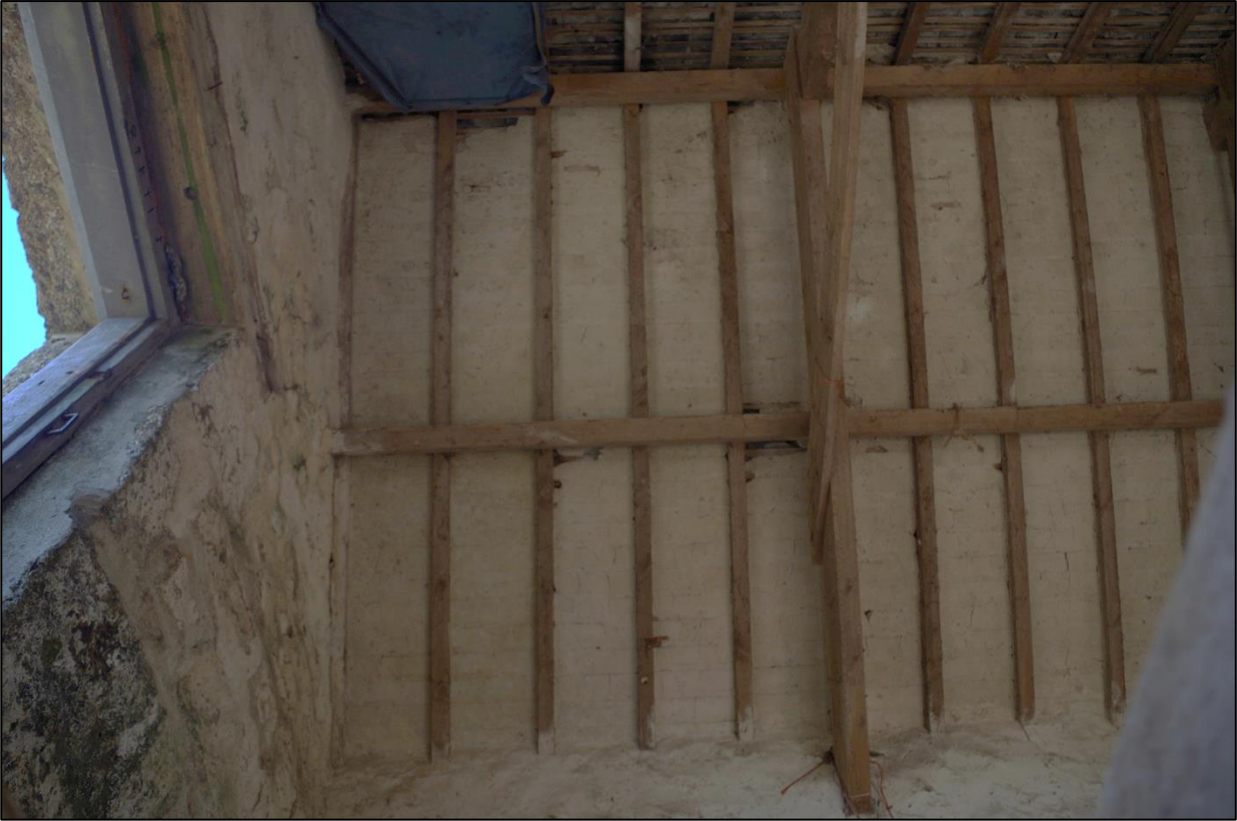
36. B1C, ROOF STRUCTURE TO THE WEST END, PLASTER REMAINING BETWEEN RAFTERS; VIEWED FROM THE GF.
