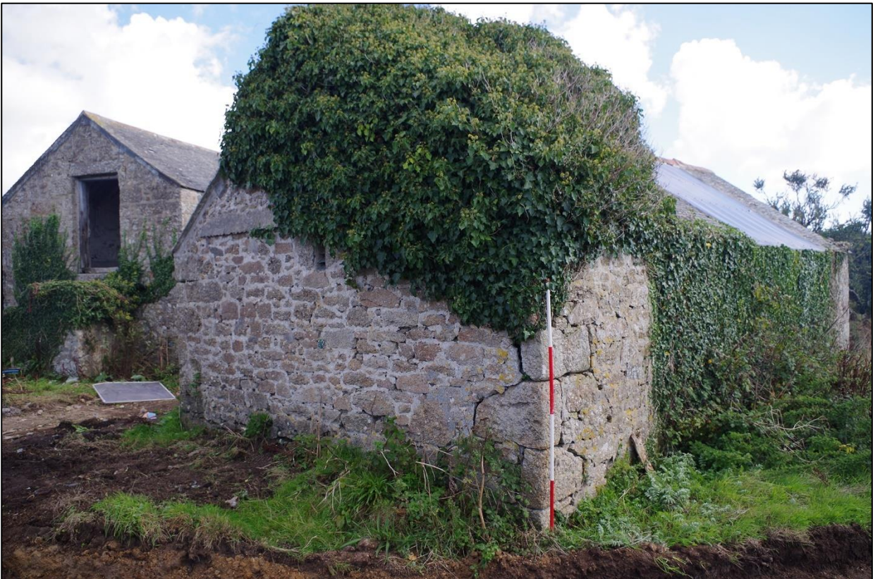
62. B2B, WEST EXTERNAL ELEVATION, SHOWING CONCRETE CORRUGATED SCARRING BELOW EAVES AND SLIT VENT; VIEWED FROM THE SOUTH-WEST (SCALE 2M).
