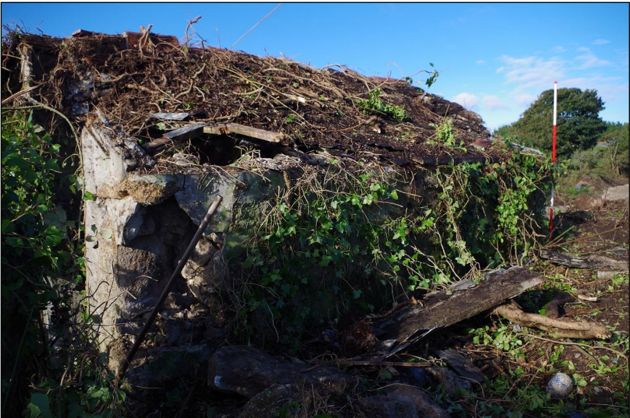
95. B3, THE NORTH ELEVATION, NORTH-EAST CORNER COLLAPSE FROM CLEARING; VIEWED FROM THE NORTH-EAST (SCALE 2M).
