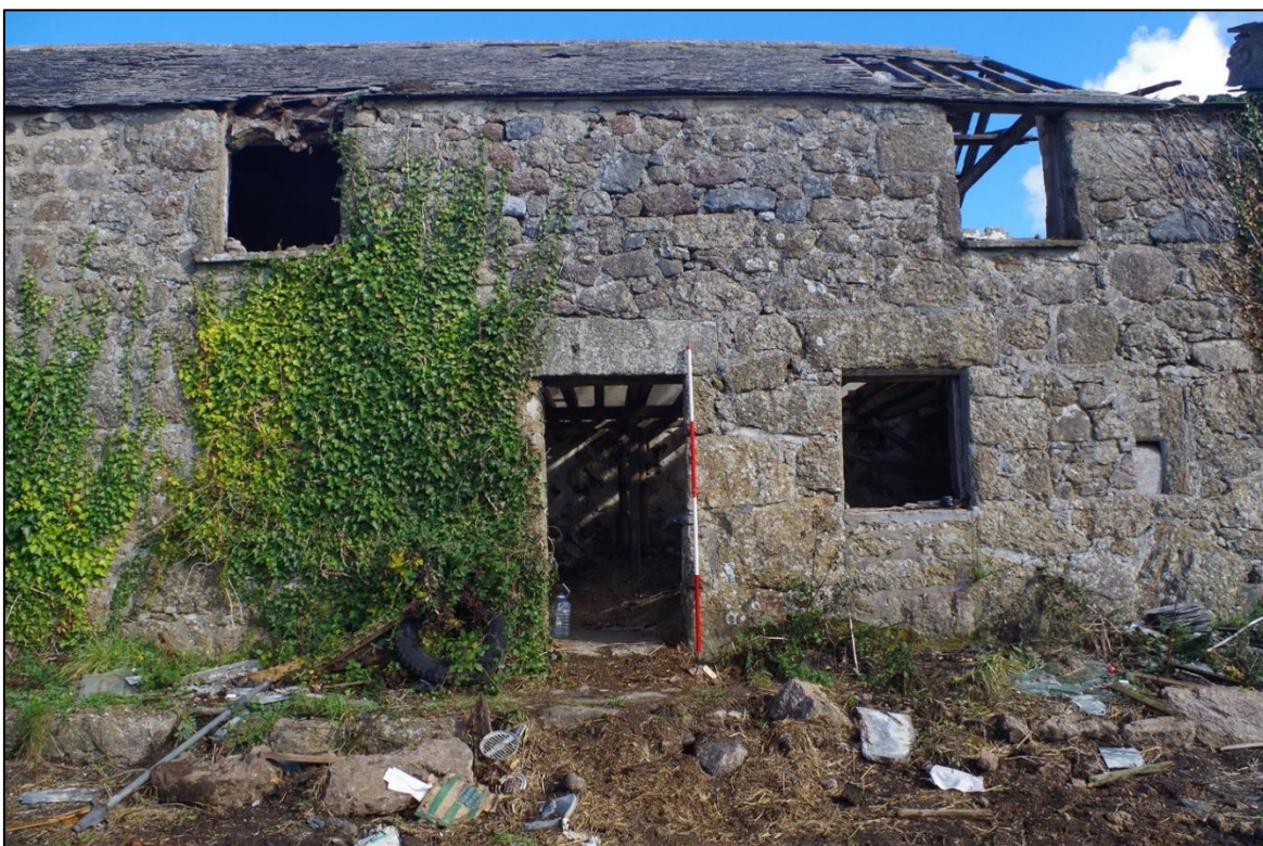
FIGURE 11: THE CENTRAL SECTION OF THE SOUTH ELEVATION. A CRUDER, HEAVIER BUILD CAN BE IDENTIFIED TO THE BASE, AND A SLIGHTLY DIFFERENT STONEWORK TO FF WITH ODD SLATESTONES, WHICH COULD REPRESENT A LATER RAISE TO THE RANGE. BLOCKED DOORWAY (W5) AND REDUCED SLIT VENT (W6) SEEN TO GF (EAST SIDE); FROM THE SOUTH (2M SCALE).
