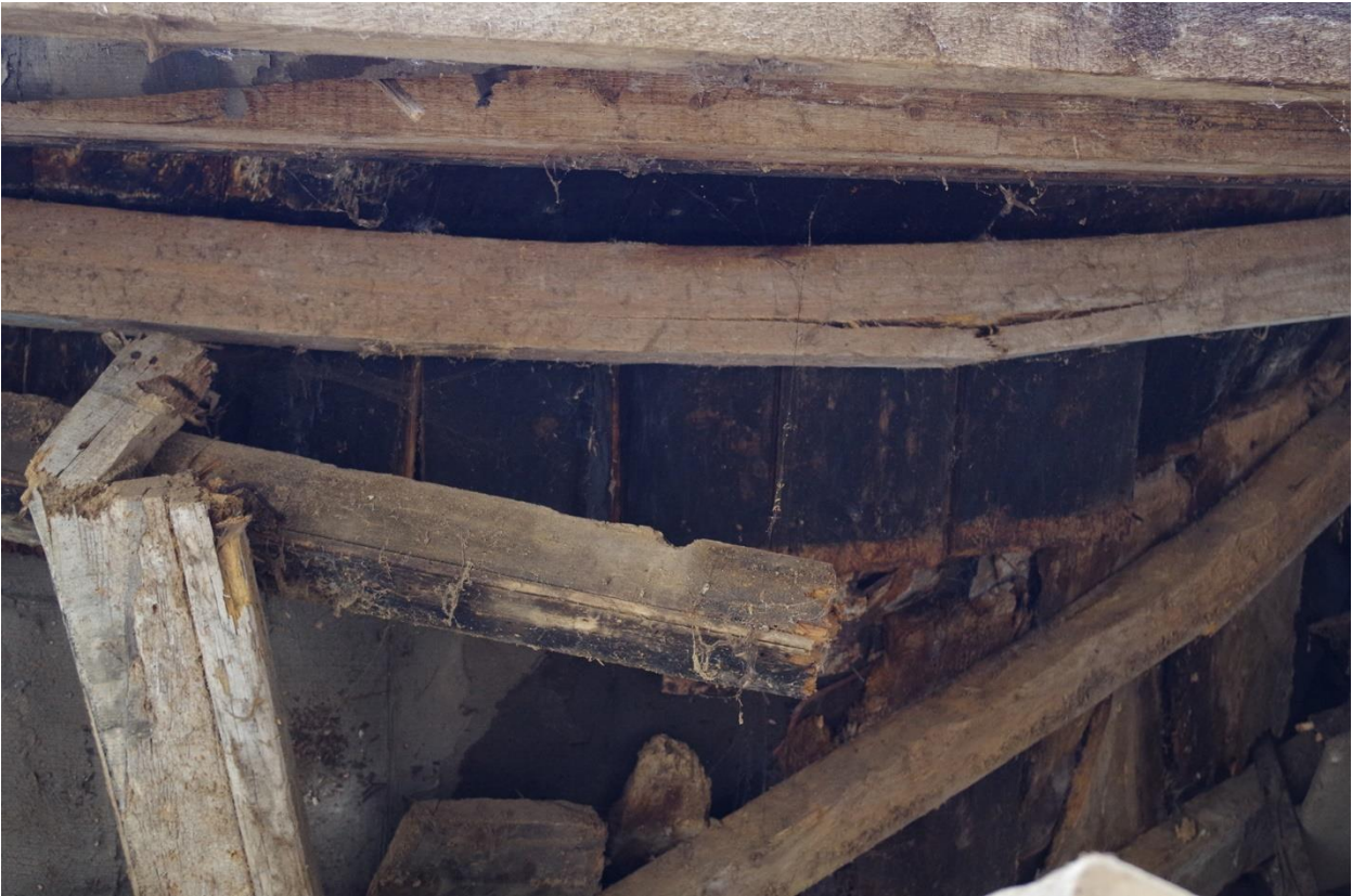
46. B1D, DETAIL OF CEILING COLLAPSE TO EAST END SHOWS FORMER FLOORBOARDS AND REUSED BEADED BRACING JOISTS; VIEWED FROM BELOW.
