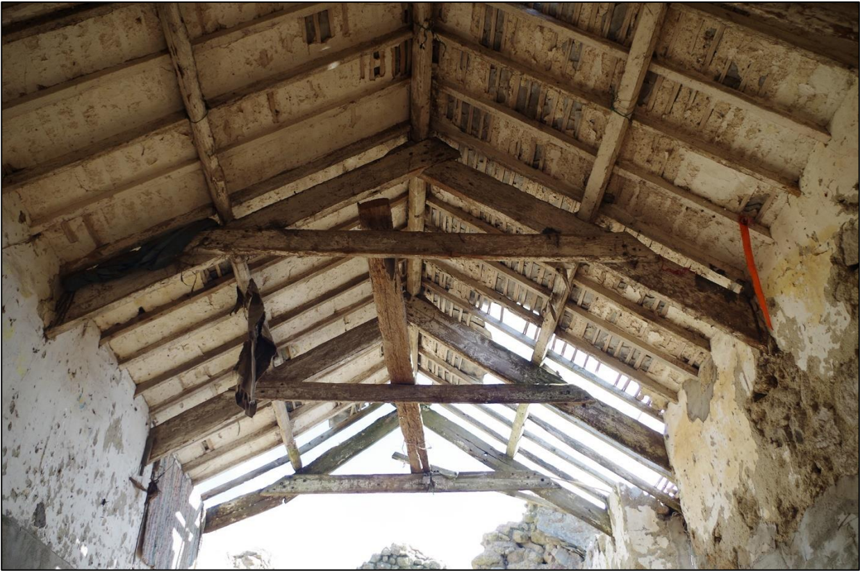
52. B1D, EAST END SUFFERED COLLAPSE, INCLUDING EAST GABLE WALL.
