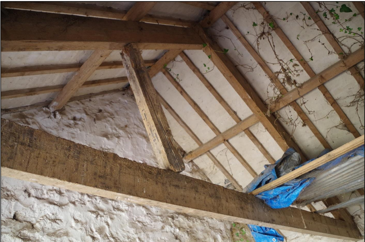
93. B2B UNALTERED ROOF STRUCTURE WITH BASIC SPIKED A-FRAMES WITH TIE BEAM, OF GOOD 19 TH CENTURY CHARACTER.
