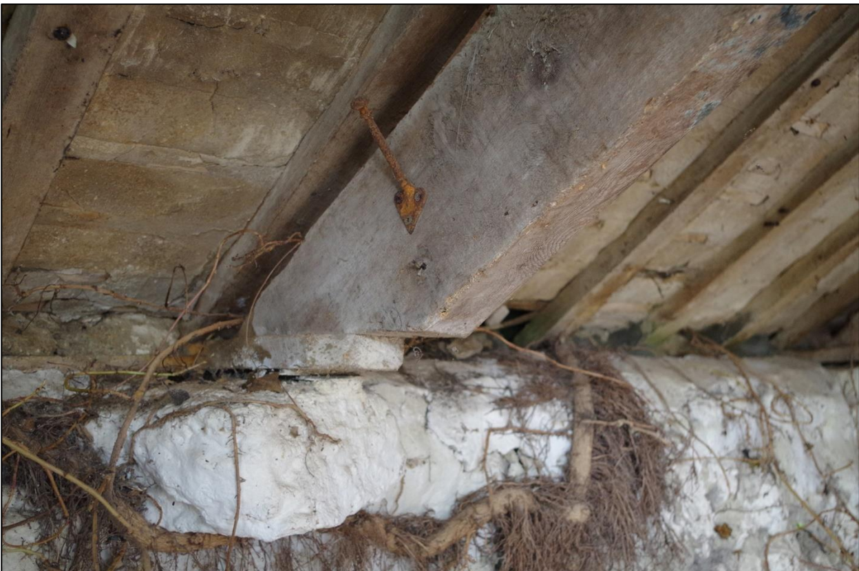
103. B3 ROOF STRUCTURE, DOES NOT FIT ADEQUATELY SUGGESTING THE TRUSSES ARE SALVAGE PIECES, THIS TRUSS SITS ON INSERTED PUTLOCK AND RAISED WITH A TIMBER PAD; VIEWED FROM THE NORTH-EAST.
