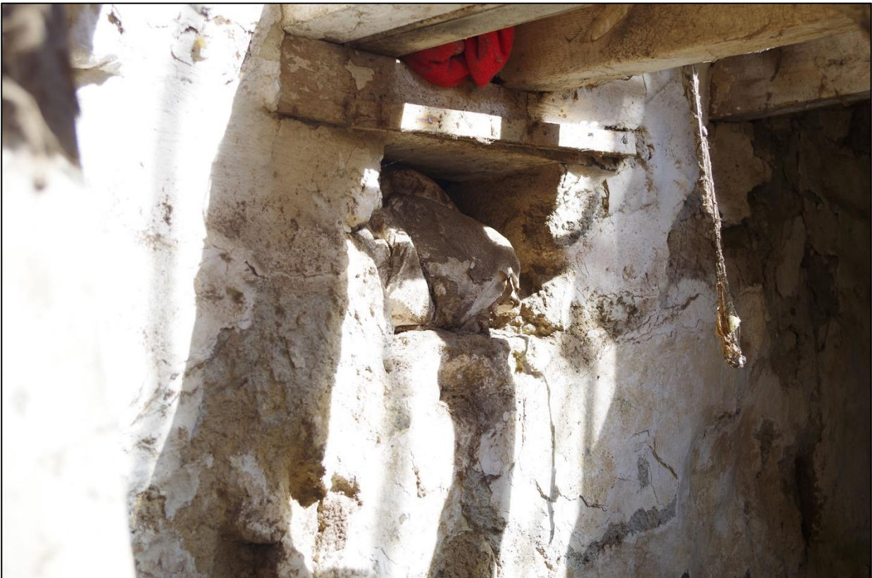
45. B1D, FORCED SECONDARY BLOCKED OPENING TO EAST END OF NORTH ELEVATION; VIEWED FROM THE SOUTH-WEST.
