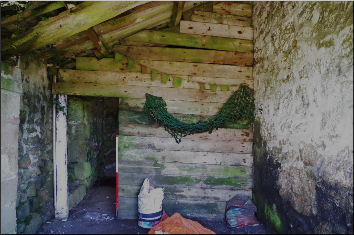
20. B1A, UNFINISHED TIMBER PARTITION, BRACED PRECARIOUSLY ON SALVAGED POSTS; VIEWED FROM THE WEST (SCALE 1M).
