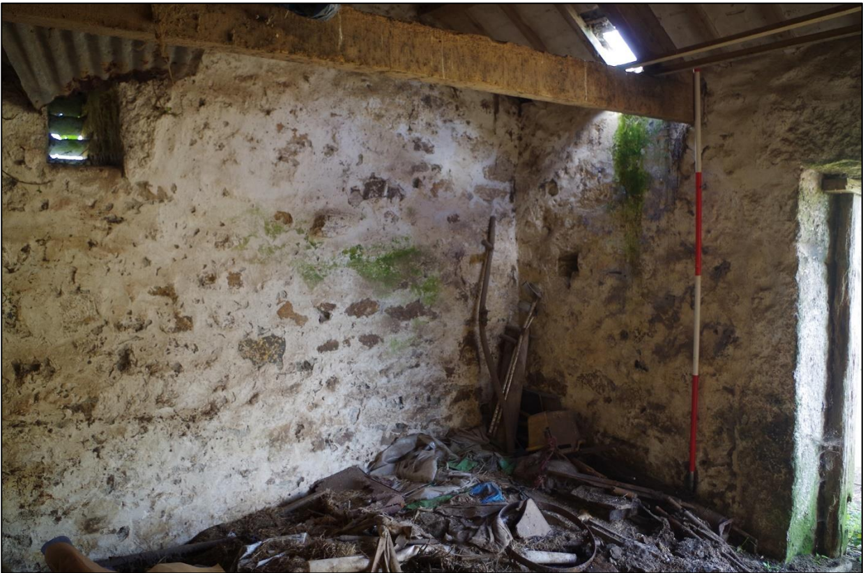
89. B2B, WEST INTERNAL ELEVATION, WITH SLIT VENT; VIEWED FROM THE EAST (2M SCALES).
