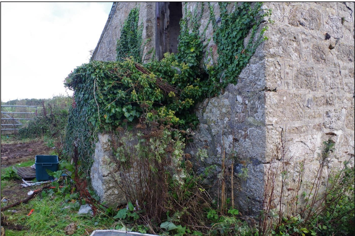
17. SOUTH ELEVATION OF GRANARY STEPS NOT TIED TO WEST WALL OF B1; VIEWED FROM THE SOUTH.
