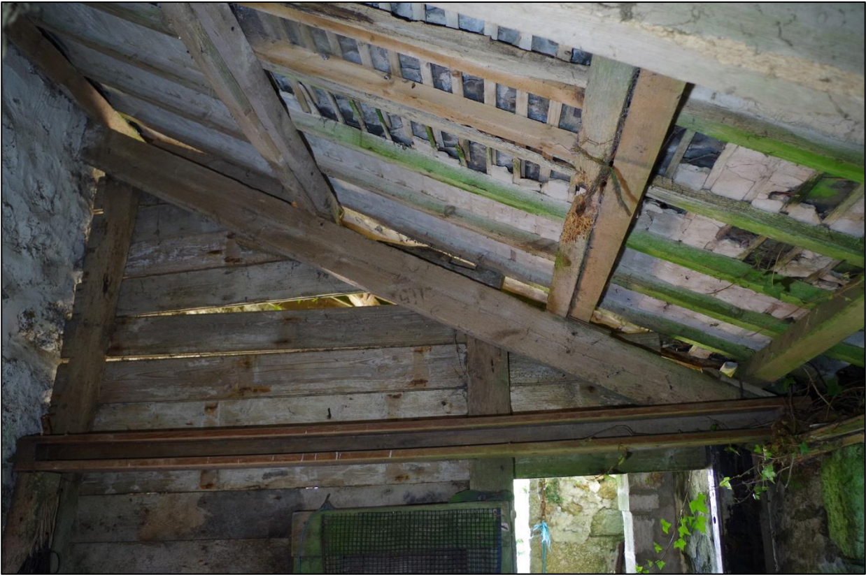
22. B1B, THE EAST SIDE OF TIMBER PARTITION AND RUSTIC ROOF WITH PLASTER SURVIVING BETWEEN RAFTERS; VIEWED FROM BELOW.
