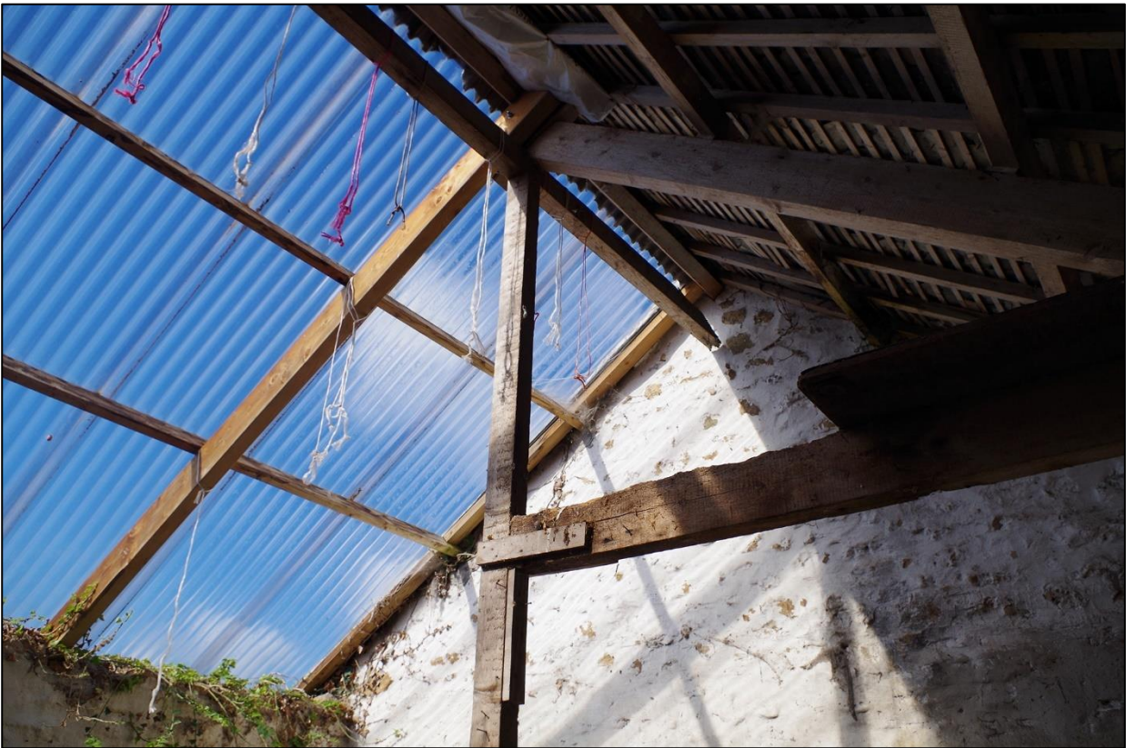
85. B2A, TRUSSES HEAVILY ALTERED TO ACCOMMODATE MODERN PLASTIC SKYLIGHT; VIEWED FROM THE NORTH-EAST.
