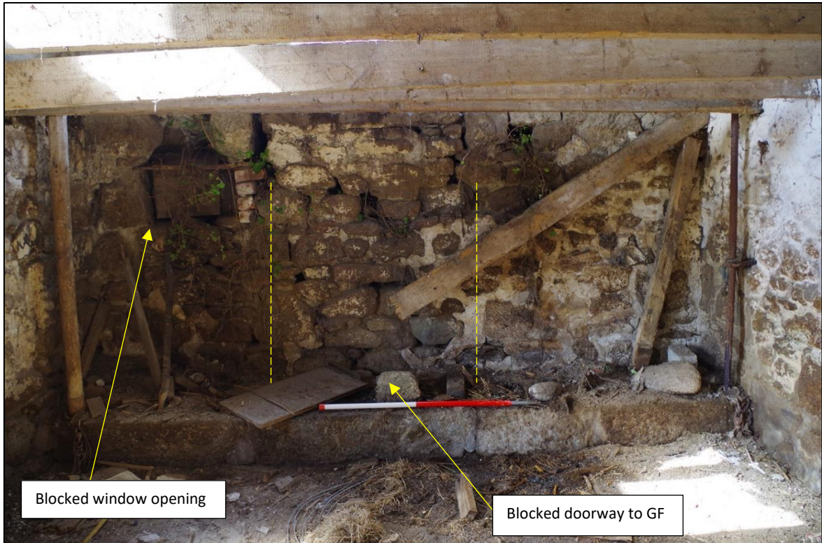
FIGURE 14: WEST ELEVATION OF B1C, POSSIBLE BLOCKED DOORWAY TO GF BELOW D12 AND BLOCKED WINDOW OPENING TO SOUTH SIDE LABELLED; FROM THE EAST (1M SCALE).
