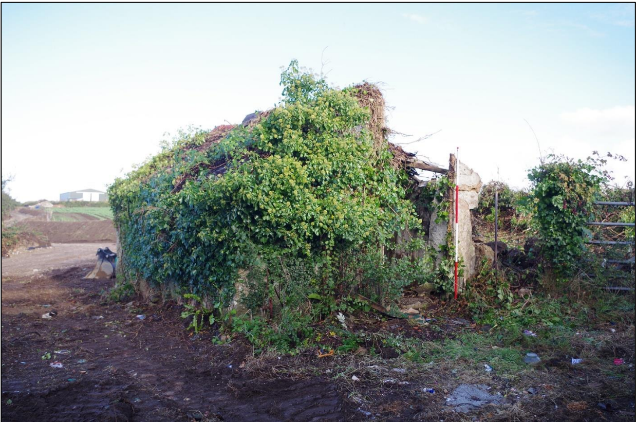
97. B3 EAST ELEVATION, NORTH-EAST CORNER SUFFERED FROM COLLAPSE; VIEWED FROM THE SOUTH-EAST (2M SCALES).
