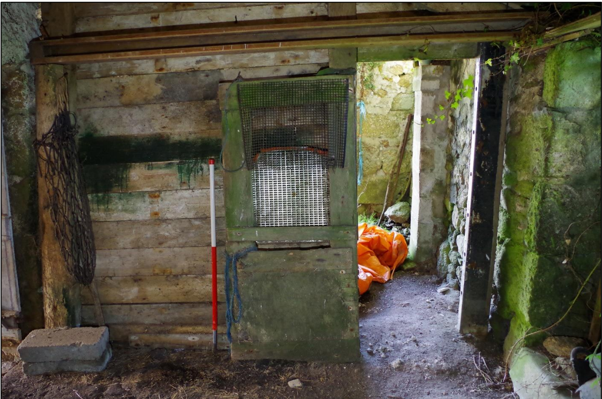
21. THE REAR SIDE OF TIMBER PARTITION IN B1B COMPLETE WITH MAKE-SHIFT PEN DOOR; VIEWED FROM THE EAST (SCALE 1M).
