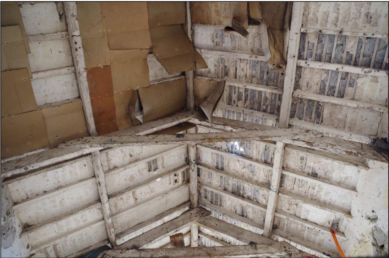
51. B1D, ROOF STRUCTURE WITH SURVIVING PLASTER BETWEEN RAFTERS, WITH SPIKED TIMBER A-FRAMES.
