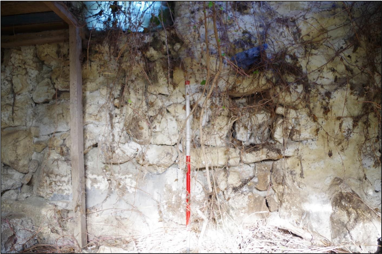
102. B3 WEST INTERNAL ELEVATION, MIXED RUBBLE BUILD, WITH HEAVY UNSHAPED BOULDERS TO BASE AND POSS. BLOCKED OPENING; VIEWED FROM THE EAST (1M SCALES).
