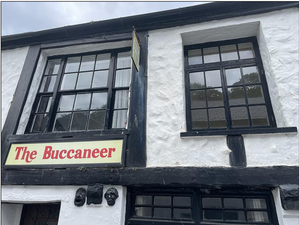
FIGURE 7: THE FF WINDOWS PROPOSED FOR CHANGE ON THE NORTH-WEST ELEVATION, INCLUDING TRI-PARTITE LARGE SASH WINDOW FRAMED BY MOCK-TUDOR TIMBER DÉCOR, VIEWED FROM THE STREET.
