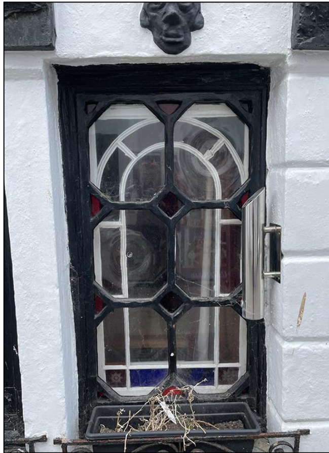
FIGURE 10: DELICATE INTERNAL ROUND-HEADED 19TH CENTURY STAINED GLASS WINDOW - A GOOD SURVIVING FEATURE OF THE PROPERTY WHEN SO MUCH ALREADY TO HAVE BEEN LOST. TAKEN FROM THE STREET.
