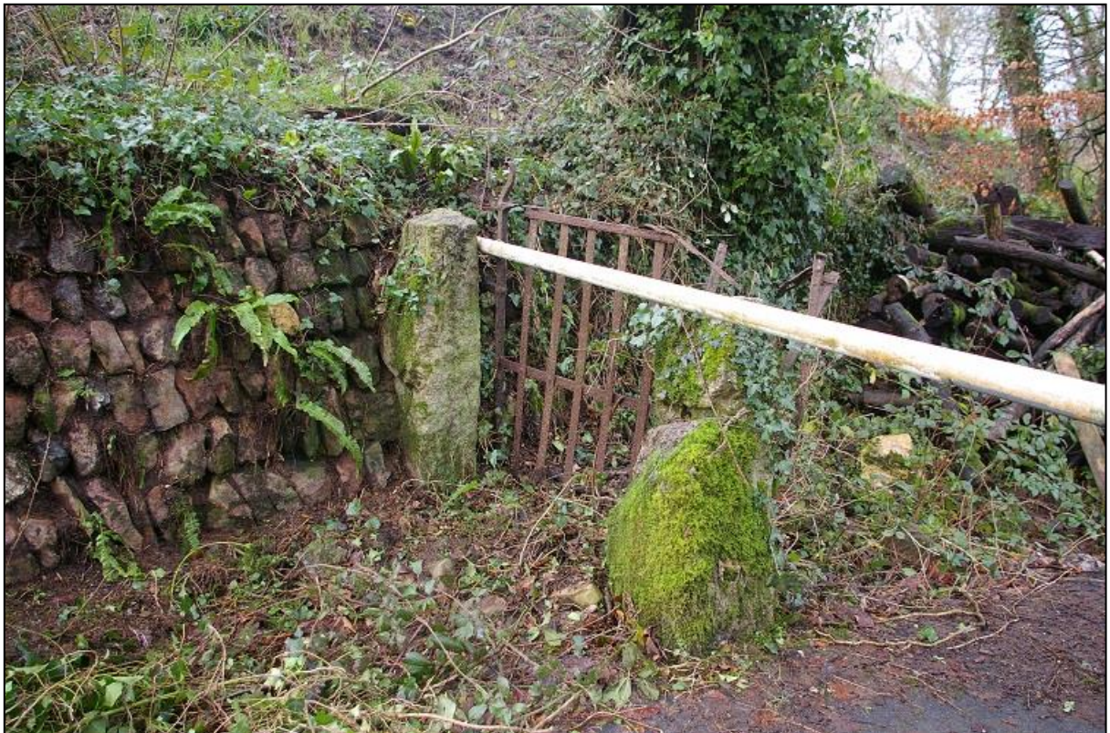
10. DETAIL OF THE GRANITE GATE POSTS AND DAMAGED PEDESTRIAN GATE TO A FORMER CART ENTRANCE BETWEEN THE HOUSE AND ITS GROUNDS AND THE TRACK TO THE MILL BUILDING; FROM THE SOUTH-EAST.
