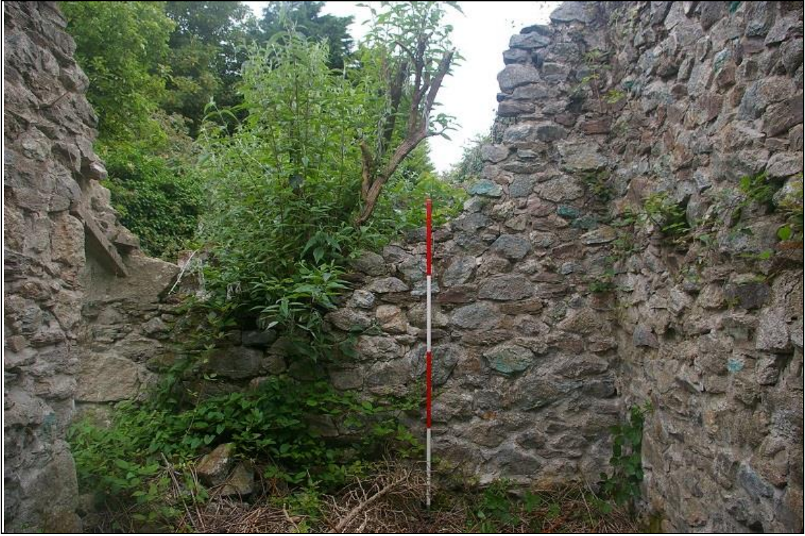
11. THE PARTITION WALL BETWEEN THE ANIMAL HOUSE AND TRAP HOUSE IN BUILDING 2; WITH 2M SCALE, FROM THE SOUTH.
