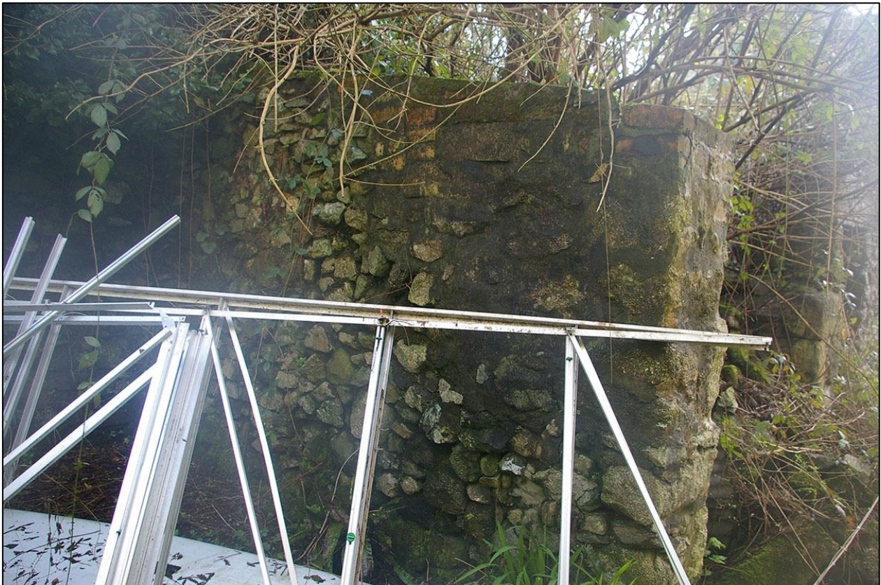
28. THE NORTH WALL OF SECTION C, BUILDING 2, SHOWING REBUILDING IN PART IN CEMENT MORTARS.
