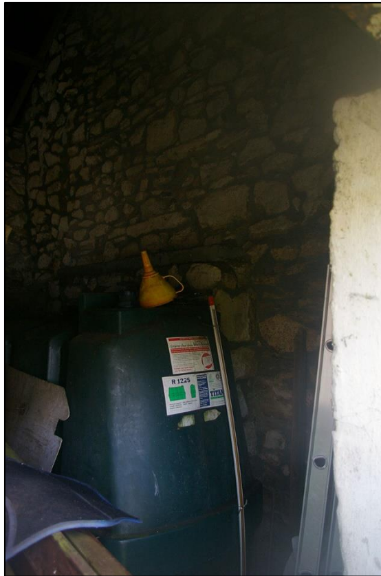
14. THE PROJECTING LOWER PART OF THE FIREPLACE, THE REST OF THE STACK SEEMINGLY TRUNCATED AS IT IS CAPPED WITH CONCRETE BLOCKS AND OBSCURED BY THE OIL TANK.
