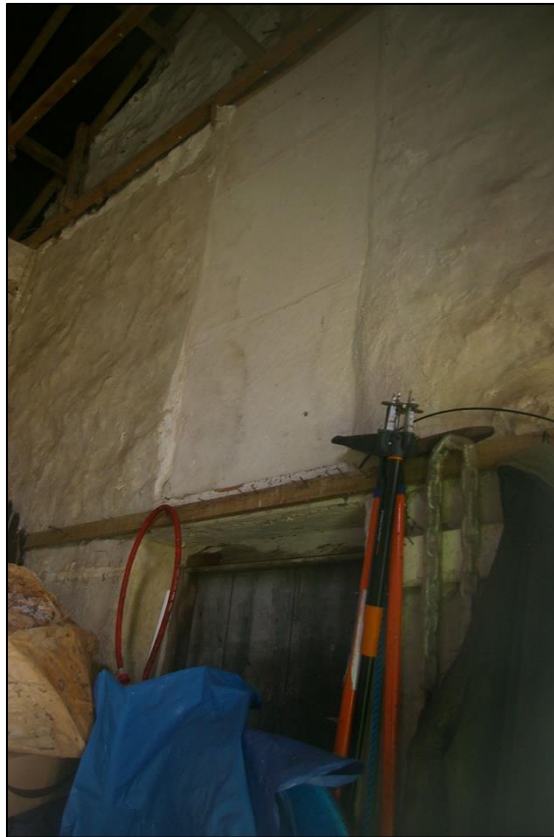
20. VIEW OF THE PLASTERED OVER LOADING DOOR LINKING TO SECTION A, FROM SECTION B, BUILDING 1.
