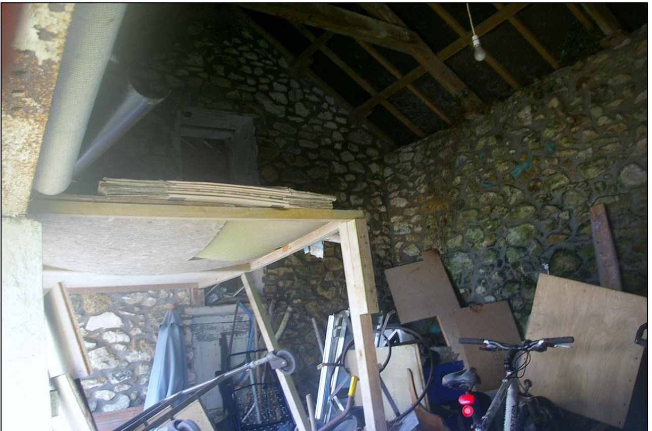
17. VIEW OF THE RAISED STORAGE AREA AND NORTH PARTITION WALL WITH LOADING DOOR AND GROUND FLOOR DOOR TO SECTION B, BUILDING 1.
