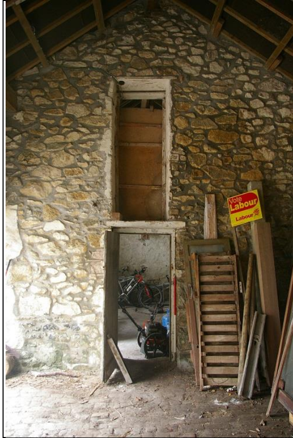
1. INTERIOR PARTITION WALL BETWEEN SECTION A & B, IN BUILDING 1; FROM THE SOUTH.
