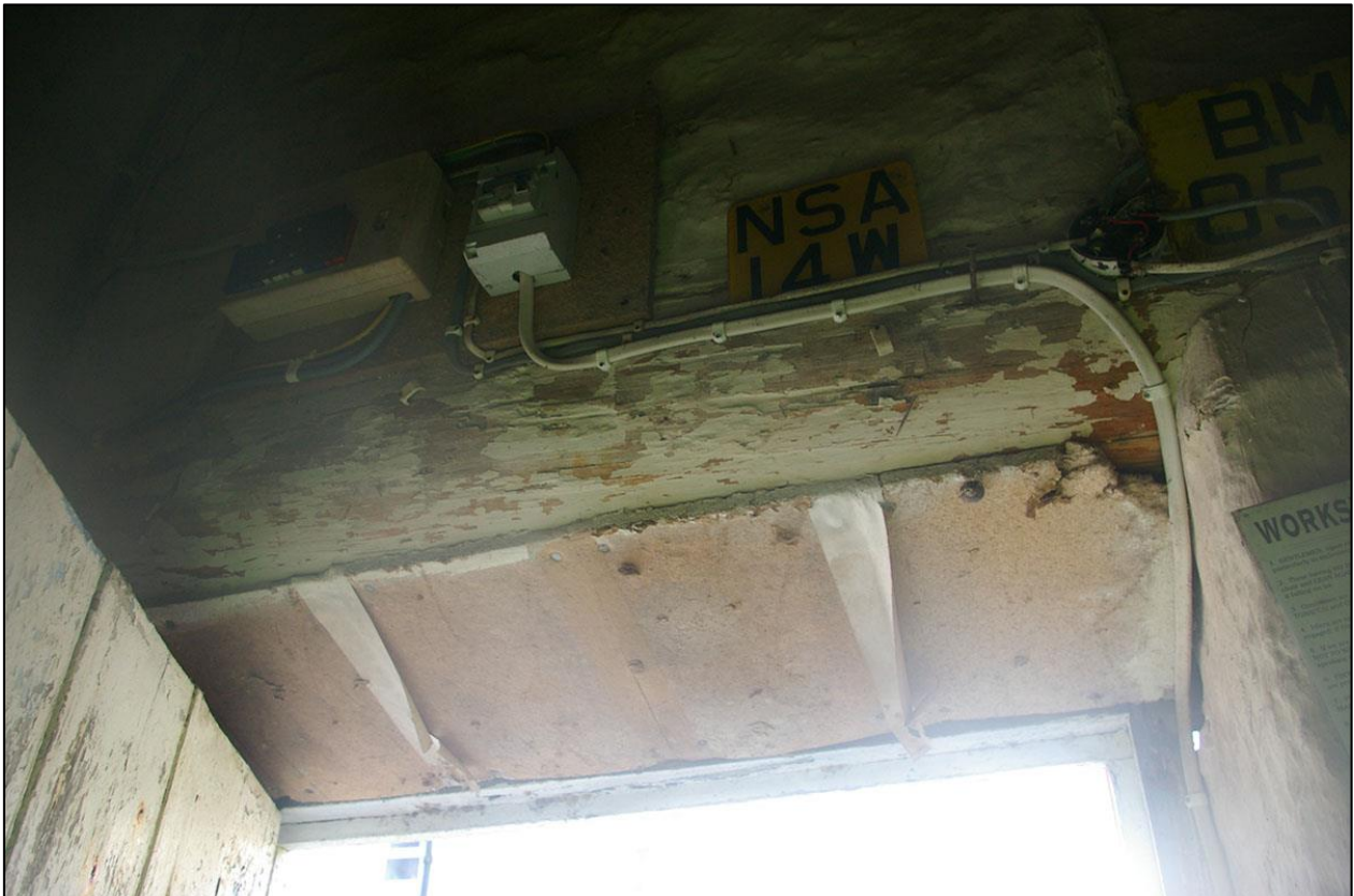
19. ROUND PROFILE TAPERING TIMBER OVER D1 ON THE INTERNAL FACE OF THE WALL, POSSIBLY A SHIPS MAST DUE TO ITS UNUSUAL PROFILE AND DENSE GRAIN AND POLISHED SURFACE?
