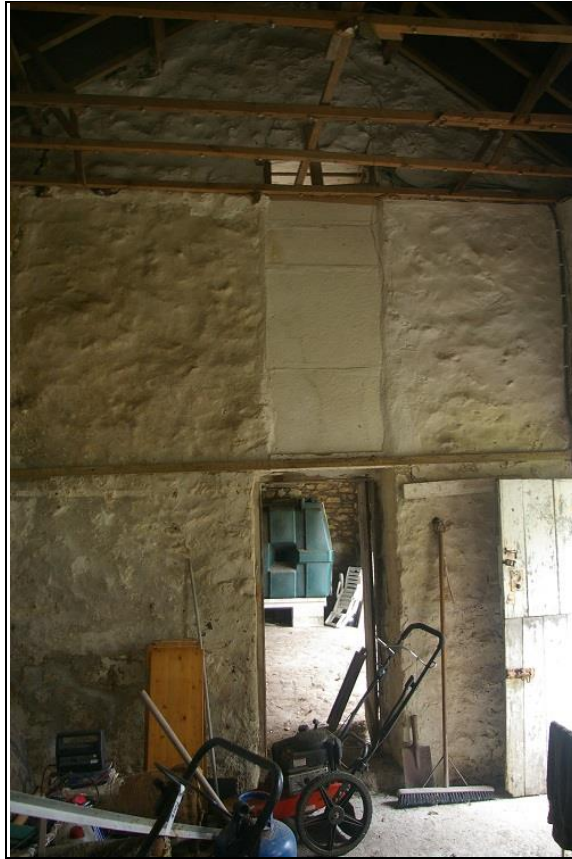
7. THE PARTITION WALL BETWEEN SECTIONS A& B, IN BUILDING 1; FROM THE NORTH.
