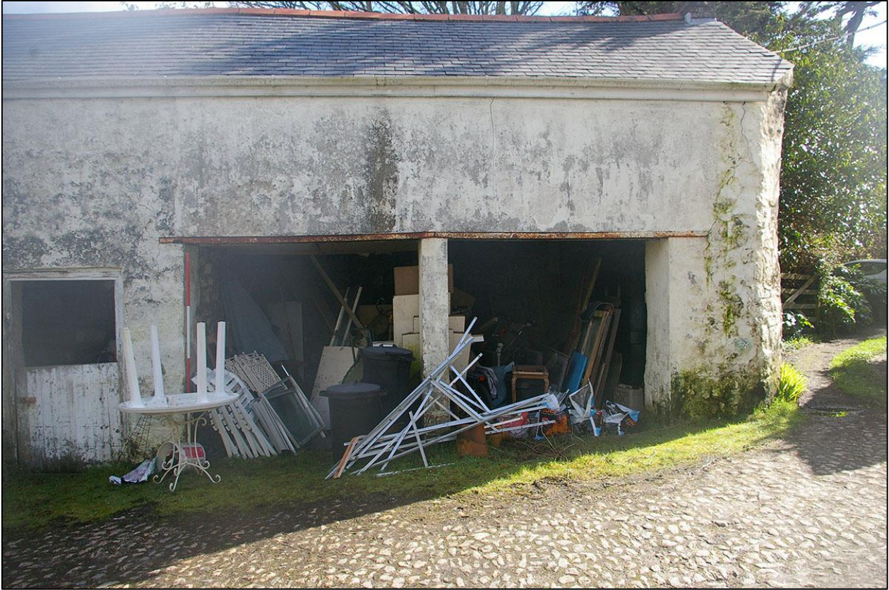
10. SECTION A, BUILDING 1 THE WEST ELEVATION WITH FORCED OPENINGS, 2M SCALE.
