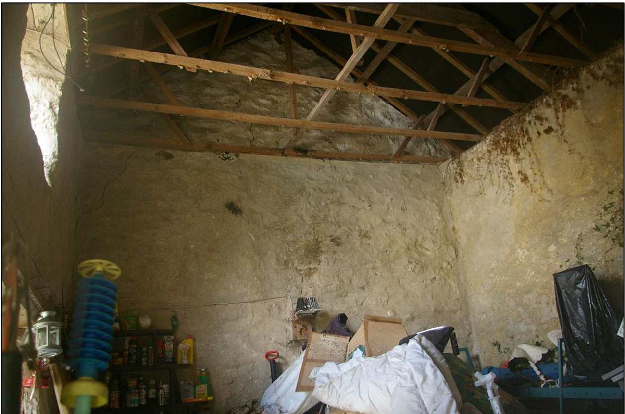
21. GENERAL VIEW OF SECTION B, BUILDING 1, WHITWASHED WALLS AND USED AS A STORE, WITH ITS CONTENTS OBSCURING FURTHER DETAILS.
