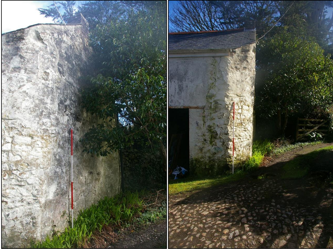
7. LEFT: THE SOUTH GABLE OF BUILDING 1, WITH 2M SCALE. 8. RIGHT: THE TRUNCATED SOUTH-WEST CORNER, WITH 2M SCALE.
