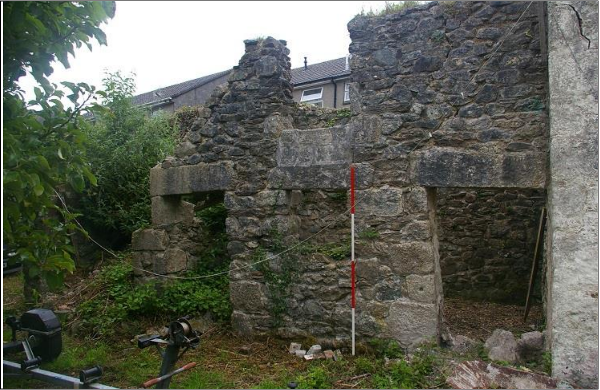
FIGURE 7: RUINED, ROOFLESS BUILDING 2, WITH 2M SCALE; FROM THE WEST-SOUTH-WEST.
