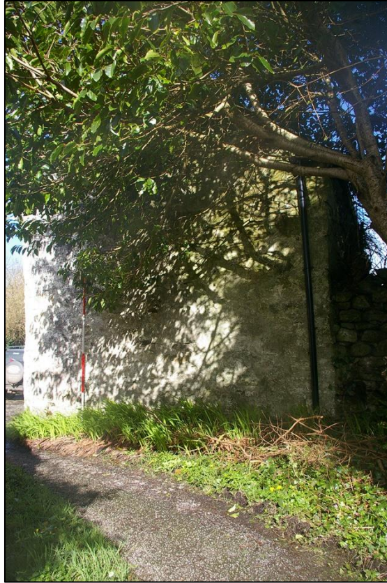
5. VIEW FROM THE SERVICE DRIVE TO THE SOUTH GABLE OF THE OUTBUILDING.
