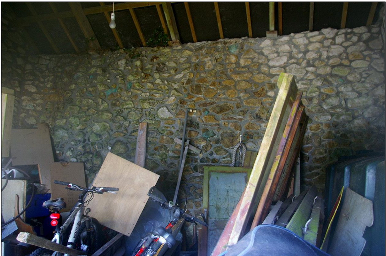
15. THE REAR EAST WALL OF SECTION A, BUILDING 1, SHOWING RE-POINTING IN CEMENT MORTAR.
