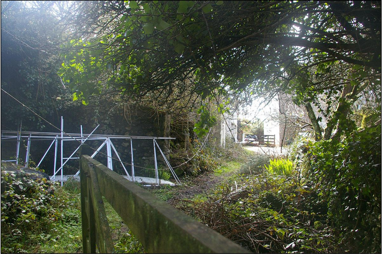
29. THE OVERGROWN RUINED SECTION D OF BUILDING 2, WITH TALL REAR WALL AND CONCRETE PLINTH FLOOR.
