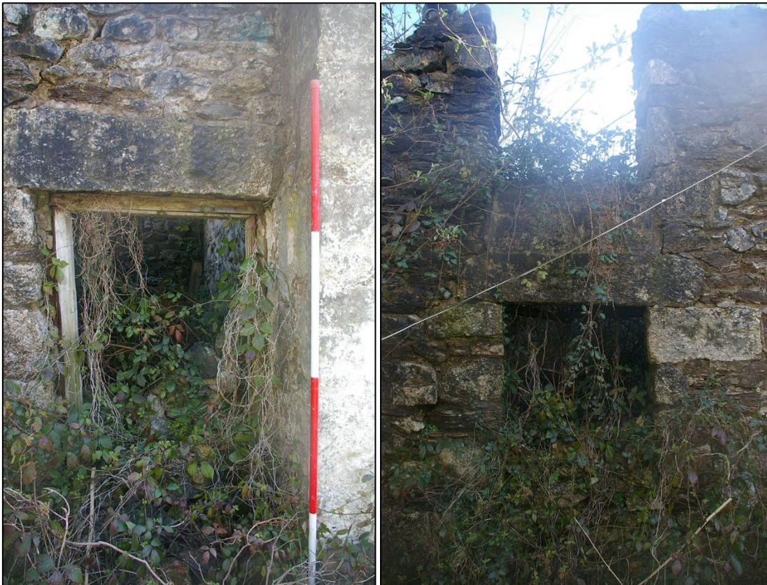
25. LEFT: VIEW OF THE SOUTHERN DOORWAY IN THE WEST WALL OF BUILDING 2, WITH INSET BEADED DOORFRAME, WITH 2M SCALE. 26. RIGHT: THE WINDOW AND LOADING DOOR ABOVE ON THE WEST ELEVATION OF BUILDING 2, THE WINDOW IS A BLOCKED DOORWAY AND EVEN THE LOADING DOOR HAS BEEN PARTIALLY BLOCKED ABOVE.
