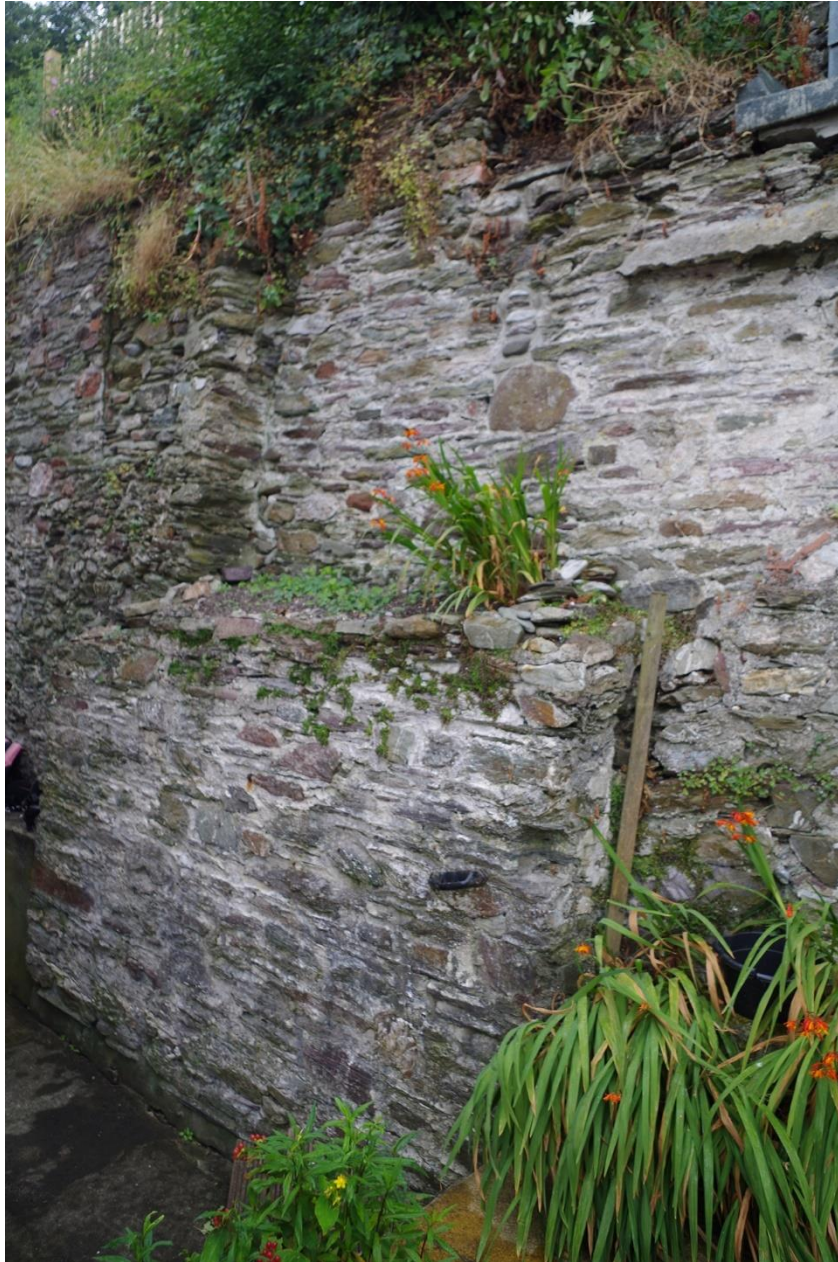
10. THE SCARRING FROM FORMER OUTBUILDINGS ON WEST BOUNDARY WALL. TAKEN FROM THE NORTH-EAST.
