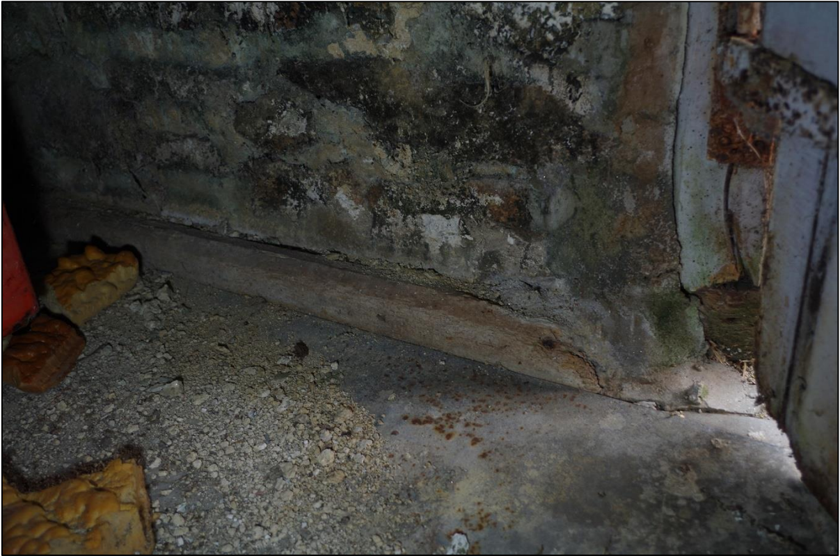
FIGURE 11: BLOCKED CHUTE TO SOUTH SIDE AMONGST LIGHTLY CHAMFERED JOIST TO GF B2, SUGGESTIVE OF GRANARY ASSOCIATION.
