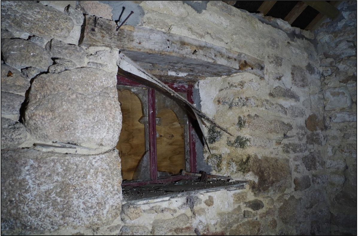
31. W4 TO SOUTH END OF EAST ELEVATION WITH REUSED PEGGED TIMBER WINDOWS OF DOMESTIC CHARACTER; FROM THE NORTH-WEST.
