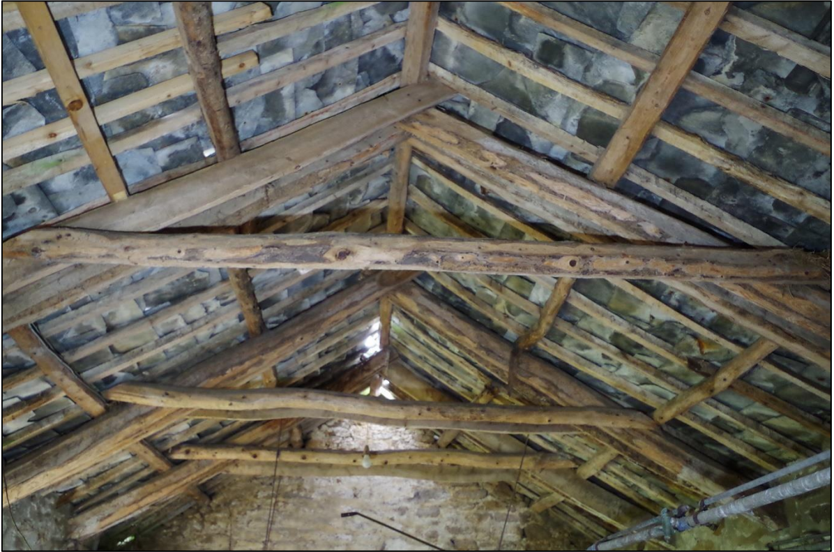
57. THE ROOF SCAPE OF B4 USING COMPOSITE PAIRED TRUSSES FROM YOUNG PINE TREES LIKELY SOURCED LOCALLY FROM EARLY PINE PLANTATIONS.
