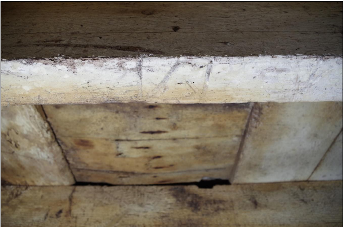
40. GOOD JOINERS MARKS TO THE CEILING JOIST IN GF B2, WITH TWO OF TWO BLOCKED CHUTES (SOUTH).
