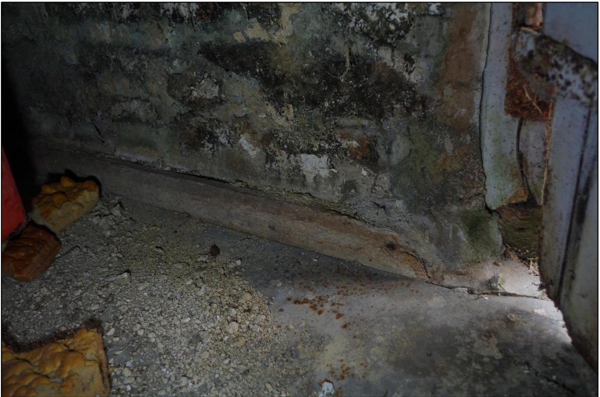
32. SECTION OF CHAMFERED TIMBER PLINTH SURVIVING TO THE BASE OF THE EAST INTERNAL ELEVATION B2 FF.
