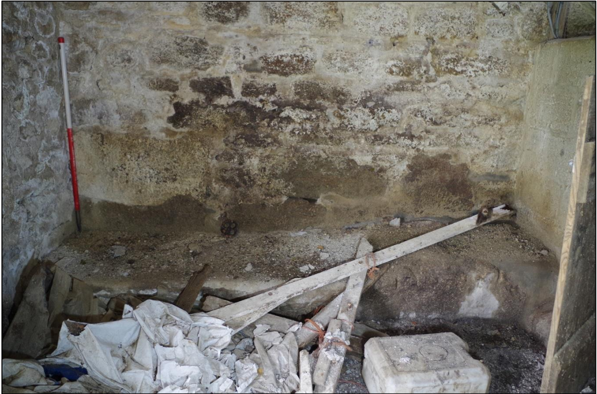
FIGURE 14: RAISED GRANITE PLATFORM TO THE NORTH ELEVATION AGAINST SOUTH ELEVATION OF B2 GABLE END; FROM THE SOUTH (1M SCALE).
