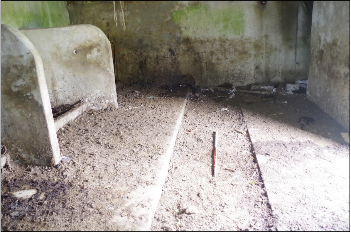
55. THE FLOOR OF B4B WITH CONCRETE PARTITIONS ALONG NORTH WALL; FROM WEST (1M SCALE).
