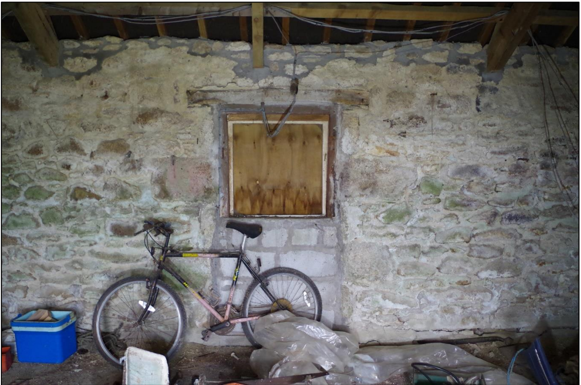
28. WEST INTERNAL ELEVATION OF B2 FF ROOM, SHOWING SECTION OF MORTAR SEAL TO BASE AND CEMENT PATCHING TO EAVES, AND THE OPPOSING WINNOWING DOOR (D5); FROM THE WEST.
