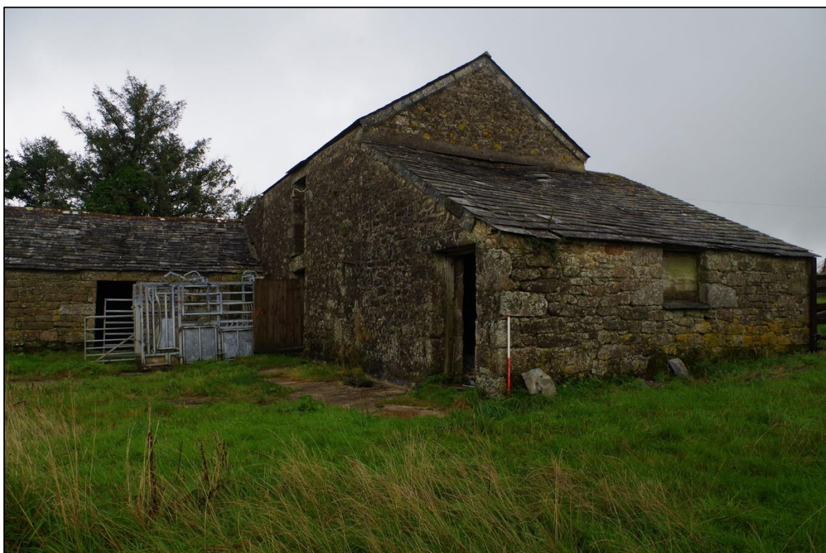
FIGURE 13: B3 LEAN-TO WRAPPING SOUTH END OF B2. THE SOUTH ELEVATION HAS LARGER BLOCKS TO THE BUILD AND GRANITE DRESSINGS, THE WEST ELEVATION HAS BEEN OBTAINED BY MODERN RIBBON-BAND REPOINTING. B3 ADDRESSES CENTRAL FARMYARD. TAKEN FROM THE SOUTH-WEST (1M SCALE).
