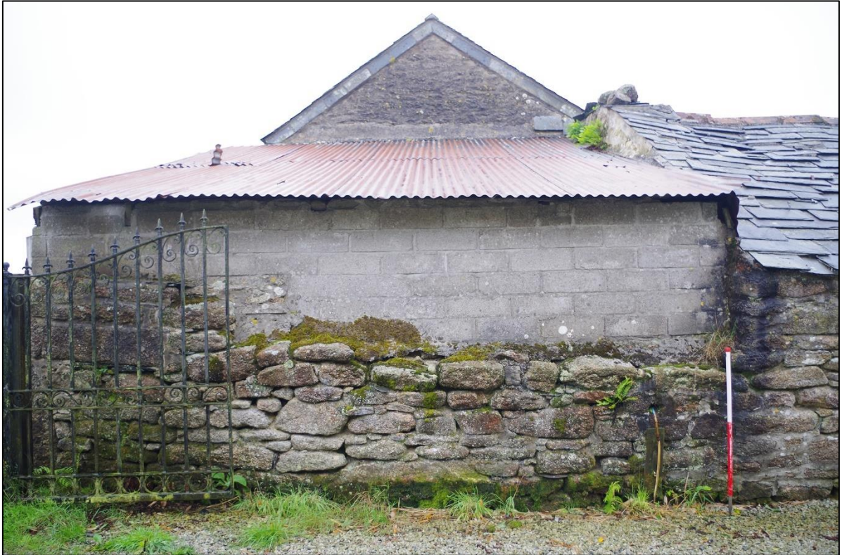
7. NORTH ELEVATION OF BUILDING 1, WITH CONCRETE RAISING EARLIER RUINOUS BUILDING; FROM THE NORTH (1M SCALE).
