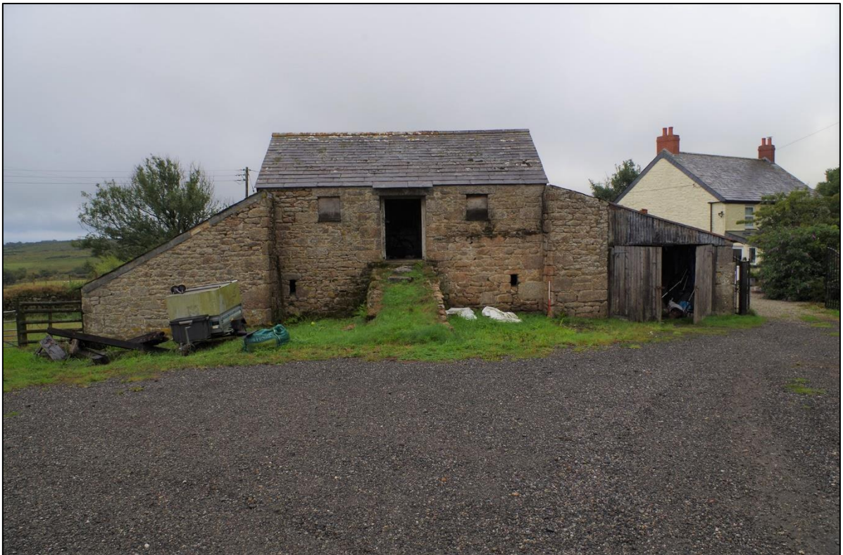
4. THE ENTRANCE YARD AND EAST ELEVATIONS OF B1, B2 & B3, 19 TH CENTURY FARMHOUSE TO THE NORTH-WEST. TAKEN FROM THE EAST (1M SCALE).
