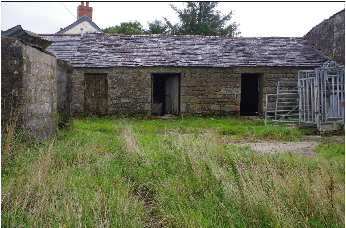
23. SOUTH ELEVATION OF B4 WITH OVERGROWN CENTRAL YARD AND LATER LIMECRETE FLOORING; FROM THE SOUTH (1M SCALE).
