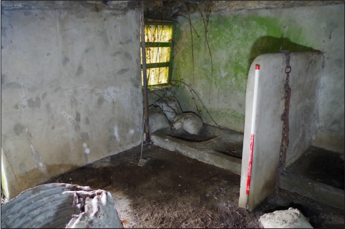
51. THE SOUTH-WEST CORNER OF B4A AND 20 TH C PARTITIONS WITH COW CHAINS; FROM THE NORTH-EAST (1M SCALE).
