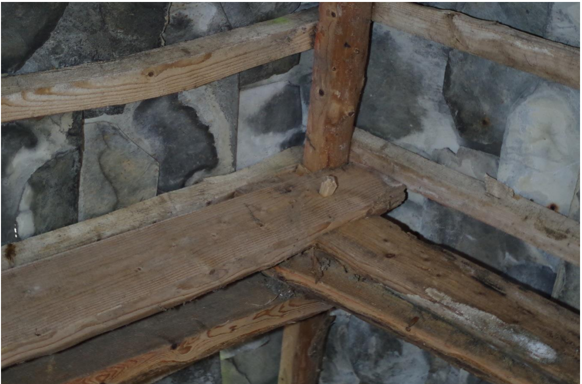
56. PEGGED COMPOSITE TRUSSES TO THE RIDGE, HOLDING RAG-SLATE ROOF AND REUSED SLATE TILES – OF GOOD 19 TH C FORM.
