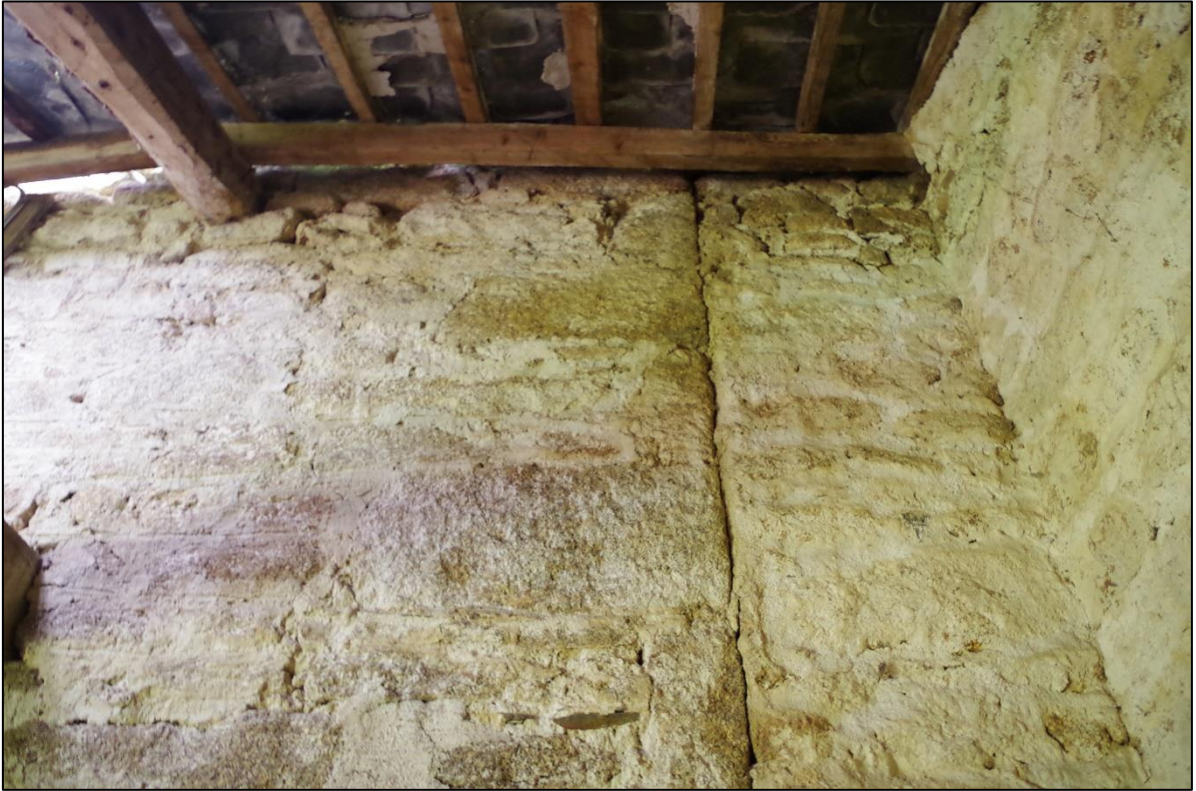
49. BUILD LINE SHOWING B3 BUILT AGAINST SOUTH-EAST CORNER OF B2, QUINS EVIDENT TO B2.
