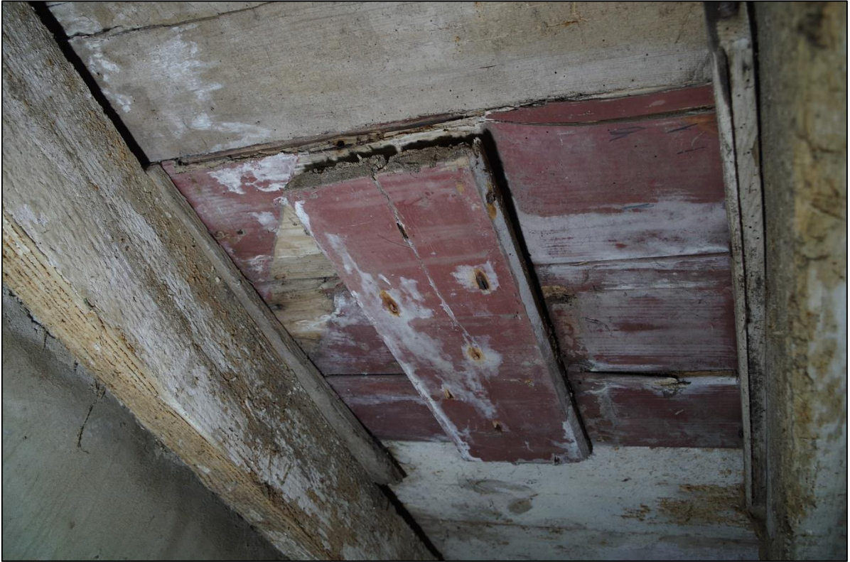
39. ONE OF TWO BLOCKED CHUTES TO THE GF SPACE OF B2 (NORTH) — A SURVIVING FEATURE FROM EARLIER GRAIN PROCESSING.
