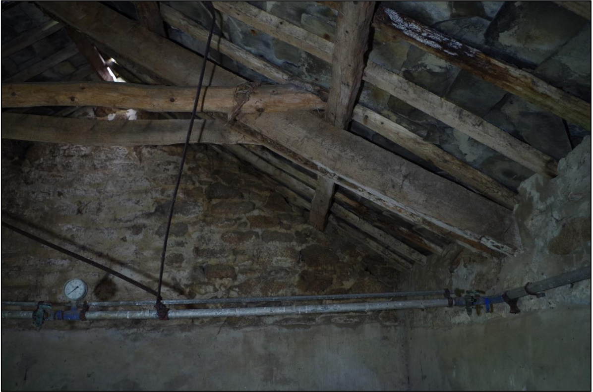
53. WEST ELEVATION OF B4A SHOWING COMPOSITE TRUSSES PEGGED RIDGE AND SPIKED AT COLLAR; FROM THE EAST.
