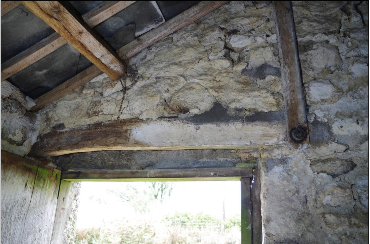
45. RUSTIC TIMBER LINTEL ABOVE B3 ENTRANCE WITH 20 TH CENTURY ELECTRIC FITTINGS SURVIVING.
