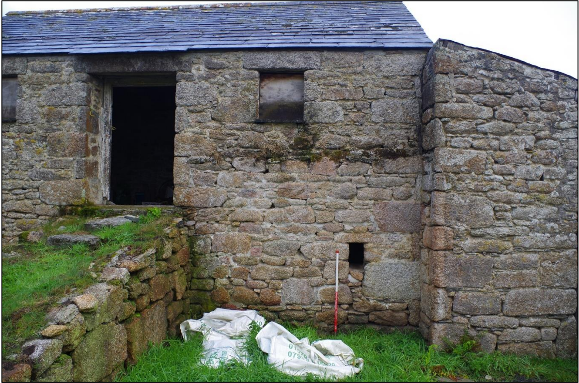
11. EAST ELEVATION OF BUILDING 1 NORTH-END WITH GF SLIT VENT W1 & W3 ABOVE; FROM THE EAST (1M SCALE).
