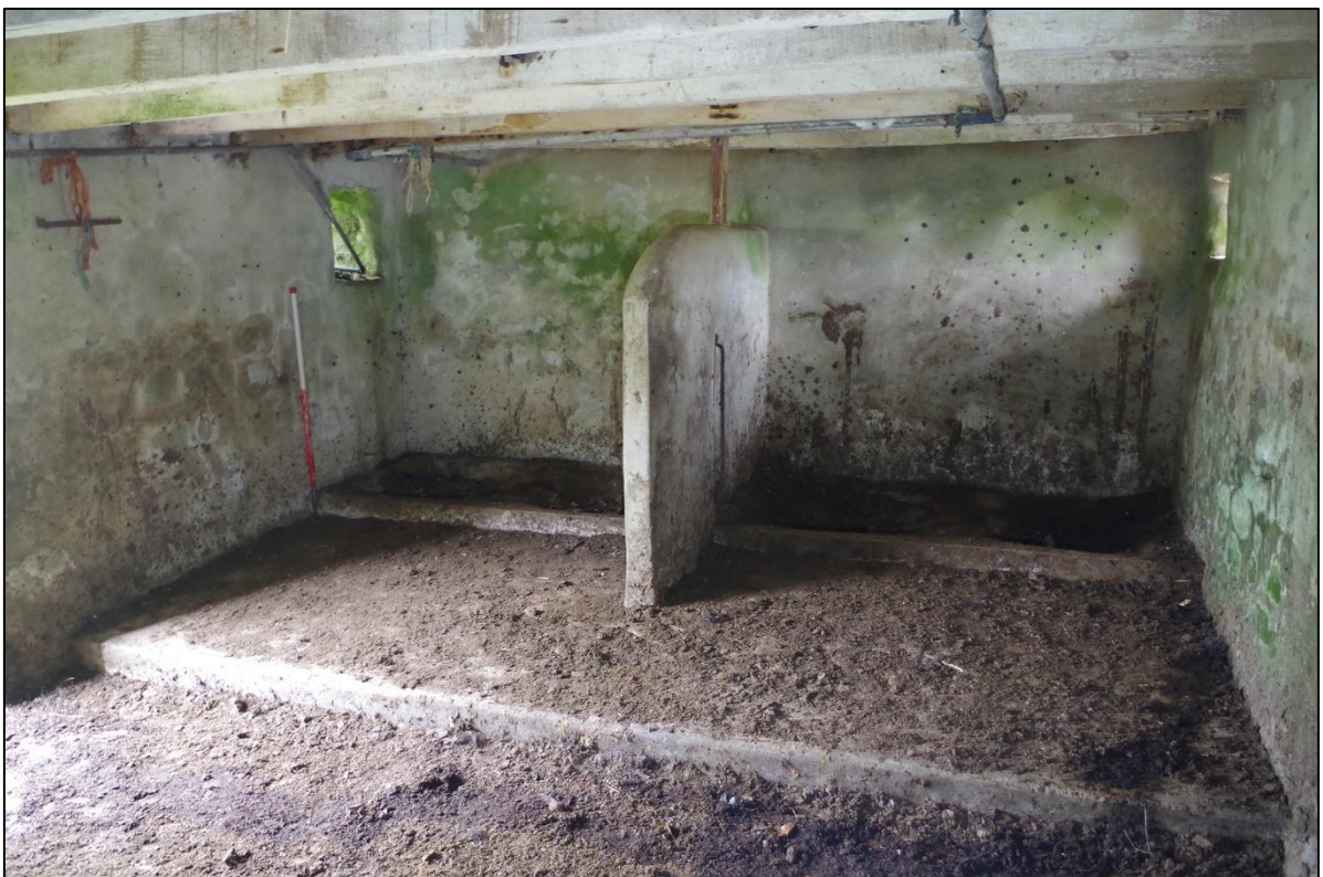
34. 20 TH CENTURY PARTITIONS AGAINST THE NORTH WALL OF B2; TAKEN FROM THE SOUTH-EAST (1M SCALE).
