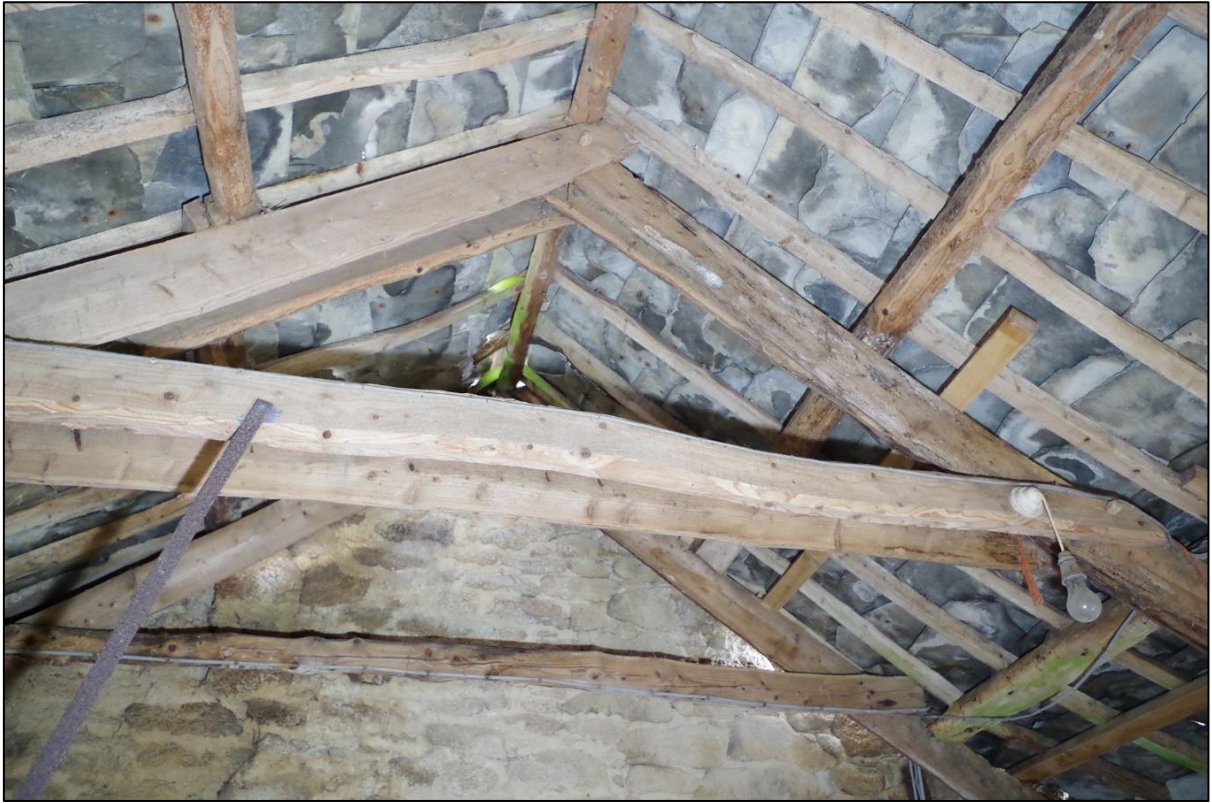
FIGURE 16: THE PAIRED COMPOSITE TRUSSES TO B4 USING YOUNG PINE TREES IS HOLDING UP A HEAVY RAG-SLATE ROOF THAT REUSES SLATE TILES.
