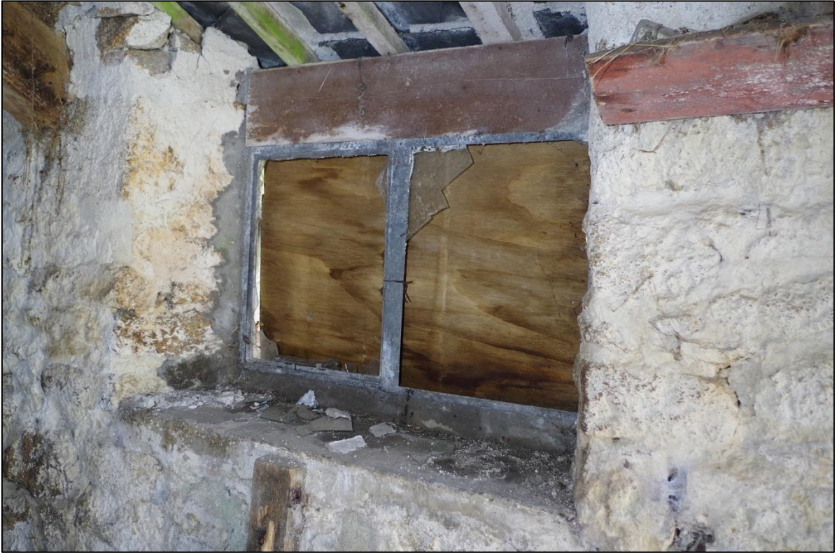
47. W5 IN SOUTH ELEVATION OF B3 WITH CRITTLE WINDOW REPLACEMENT AND SLATE SILL; FROM THE NORTH-WEST.
