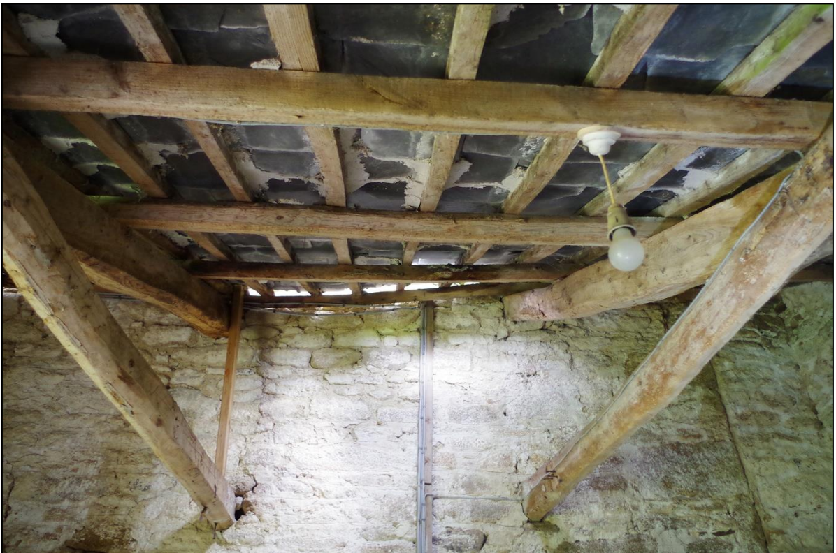
48. ROOF STRUCTURE OF B3, ORIGINAL TO ITS BUILD, INCLUDES RUSTIC TRUSSES AND TIE BEAMS FORCED INTO SOUTH GABLE END OF B2.
