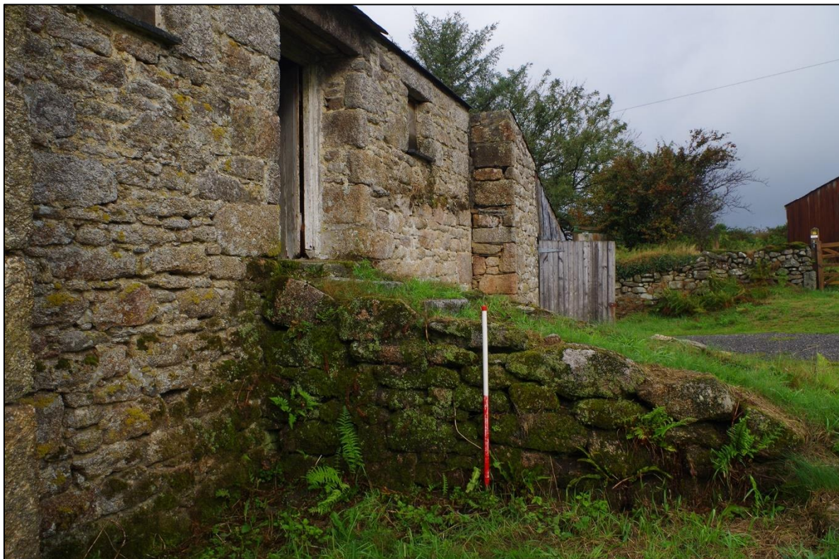
13. SOUTH ELEVATION OF GRANARY STEPS SHOWING BUILT USING GRANITE RUBBLE; TAKEN FROM THE SOUTH (1M SCALE).
