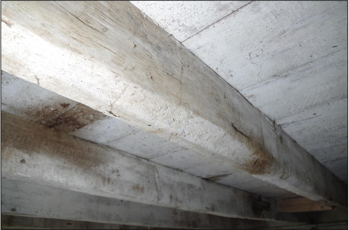
37. EXAMPLES OF CHAMFERED JOISTS SURVIVED TO B2 CEILING – GOOD 18 TH -19 TH CENTURY FEATURE.
