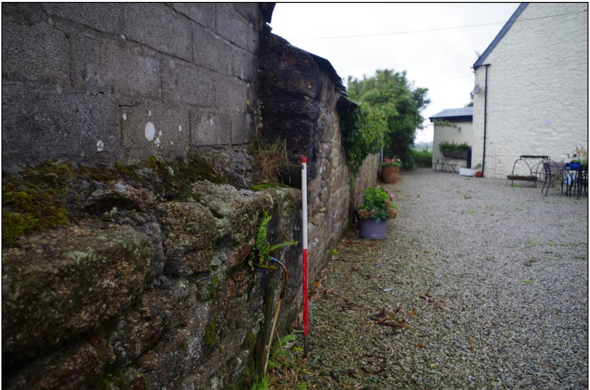
8. NORTH ELEVATION OF B1 SHOWING COMPROMISED INTEGRITY BEING PUSHED OUT BY MODERN ROOF; FROM THE EAST (1M SCALE).
