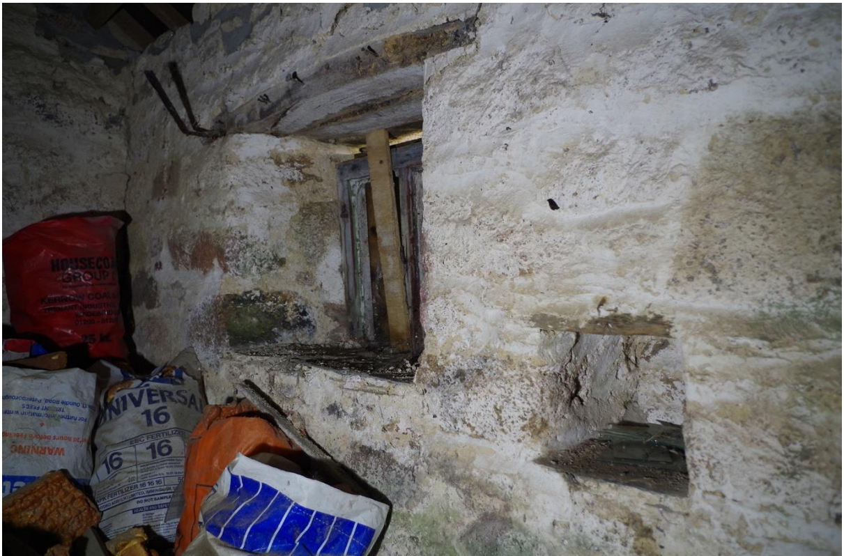
FIGURE 12: W3 TO THE NORTH END OF EAST INTERNAL ELEVATION, WITH GOOD PEGGED TIMBER WINDOWS WITH PINTLES FOR LOST SHUTTERS, A RUSTIC TIMBER LINTEL AND SLATE SILL; SUGGESTS A POSSIBLE DOMESTIC FUNCTION FOR THIS SPACE, HOWEVER THE WINDOW FRAMES COULD BE SALVAGED PIECES. KEEPING PLACE TO THE SOUTH SIDE OF W3; FROM SOUTH-WEST.
