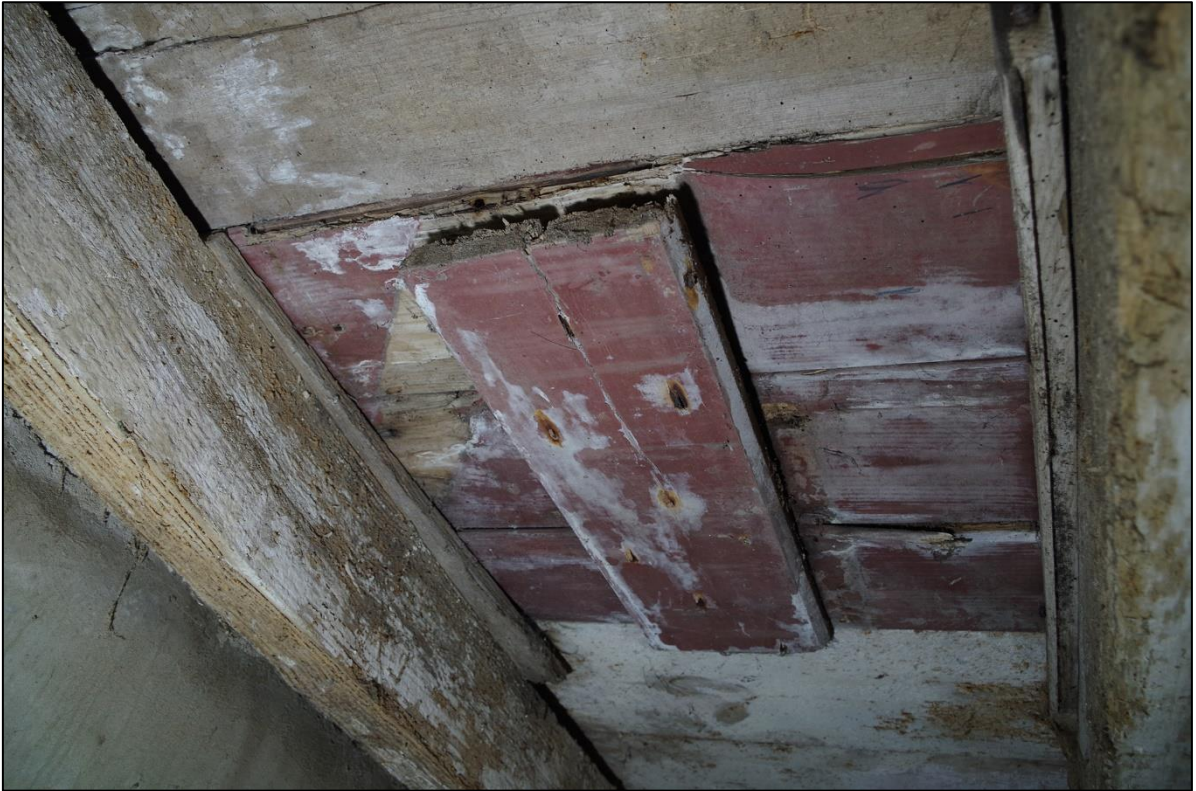
FIGURE 10: BLOCKED CHUTE TO SOUTH SIDE AMONGST LIGHTLY CHAMFERED JOIST TO GF B2, SUGGESTIVE OF GRANARY ASSOCIATION.
