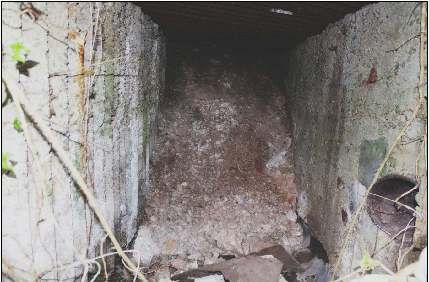
Figure 4: The interior of the covered leat, with walls of shuttered concrete and corrugated iron sheet roof, and partly infilled following the construction of the late 20 th century phase of the Cowlins Mill building. Viewed from the north-east (no scale).
