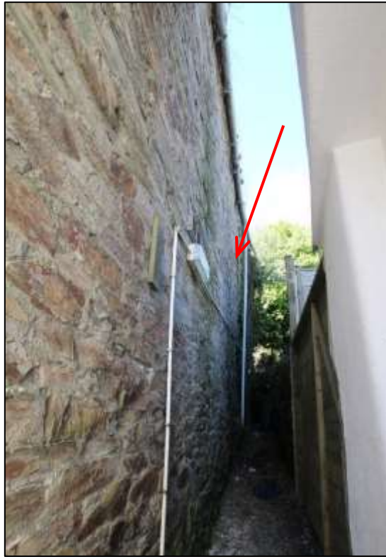
FIGURE 14: THE NORTH ELEVATION SHOWING THE BUILD LINE AND MARKED CHANGE OF ALIGNMENT ALONG THE LONG RECTANGULAR RANGE (INDICATED); VIEWED FROM THE EAST.
