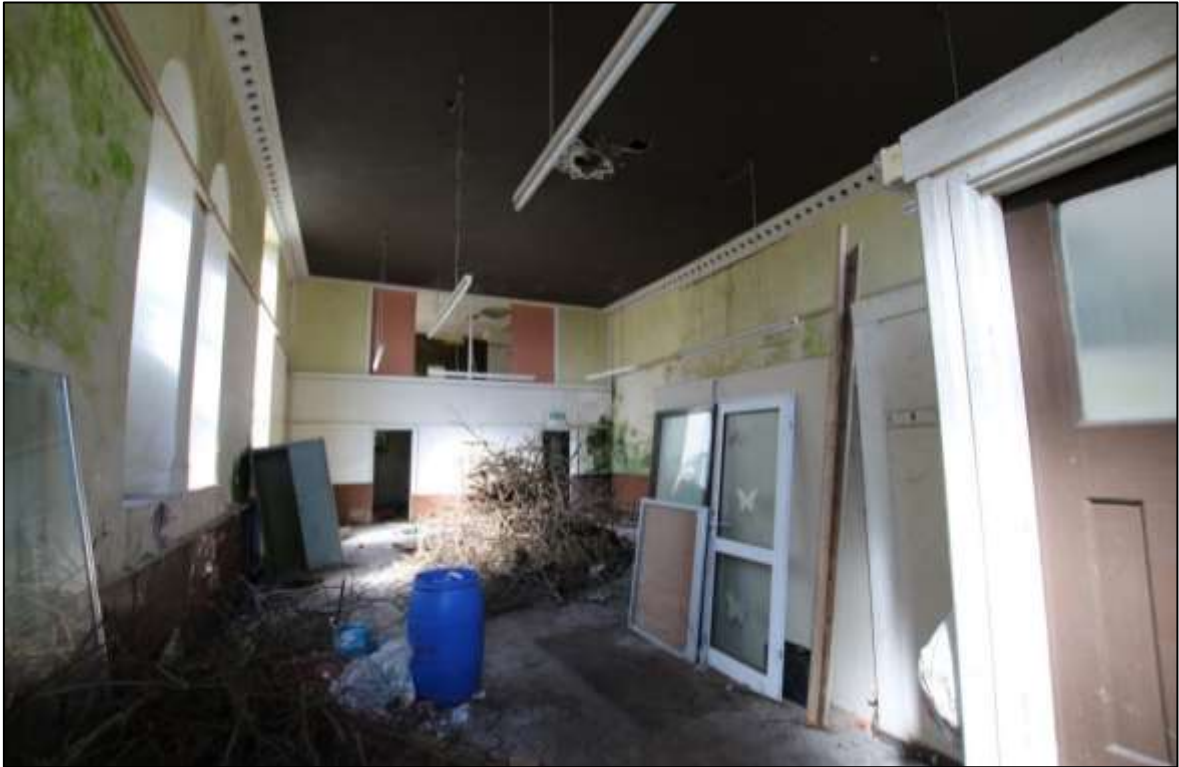
FIGURE 15: THE MAIN SPACE IN THE CHAPEL, WITH INSERTED PARISH ROOMS AND ORGAN LOFT TO THE WEST END; VIEWED FROM THE ESE.
