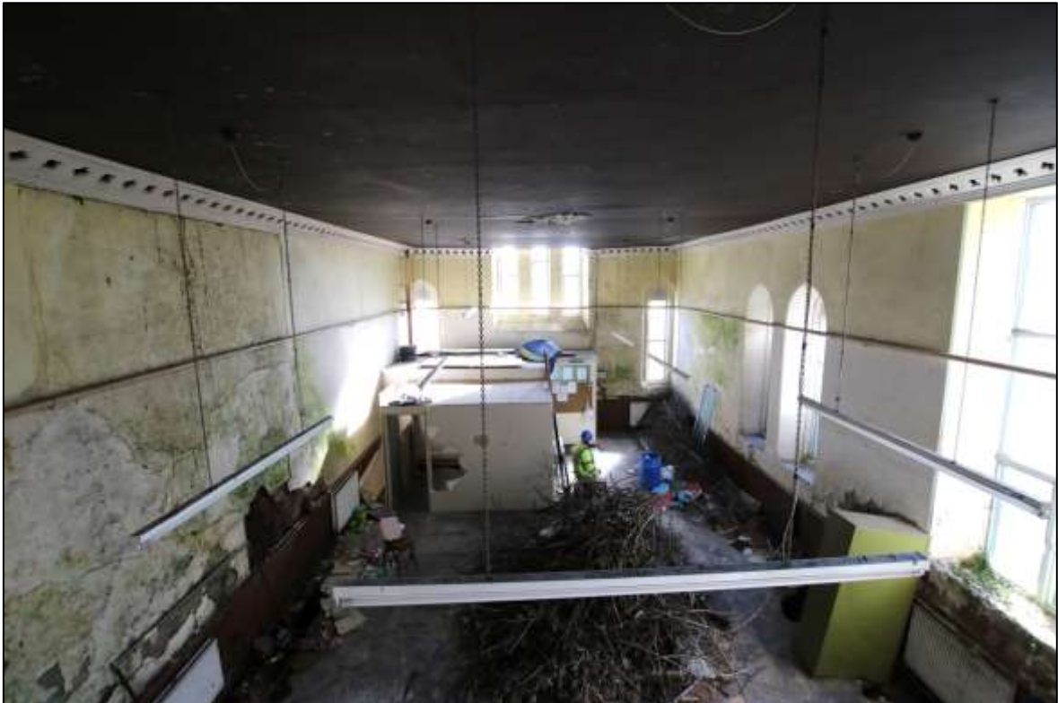
FIGURE 21: THE INTERIOR OF THE CHAPEL, WITH INSERTED CEILING WHICH CUTS THE VARIOUS WINDOWS, AS WELL AS THE CLEAR PHASING VISIBLE IN THE WALLS; VIEWED FROM THE WEST.
