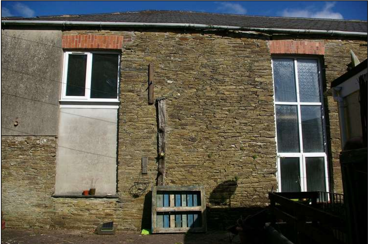
FIGURE 13: THE SOUTH WALL OF THE CHAPEL SHOWING THE OLDER BUILD, WITH BRICK DETAILING TO FULL HEIGHT CHAPEL WINDOWS IN THE GENERIC NEO-CLASSICAL CORNISH STYLE, RESTRAINED AND SIMPLE BUT WITH SYMMETRY, USING LOCAL VERNACULAR MATERIALS; VIEWED FROM THE SOUTH.
