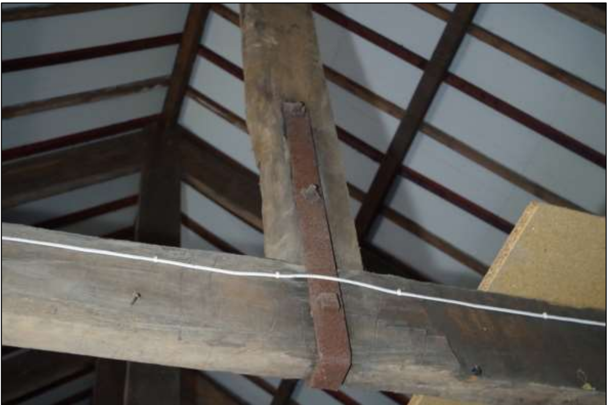
FIGURE 18: THE LARGE, HEAVY IRON STRAPS BRACING KING POST AND TIE BEAM REPRESENTING GOOD INDUSTRIAL FORM, WITH JOINERS MARKS. TAKEN IN BELOW TO THE SOUTH END OF R3.
