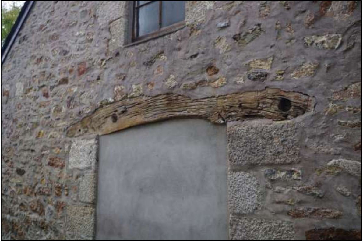
FIGURE 11: TIMBER LINTEL SURVIVING TO BLOCKED DOOR IN SOUTH ELEVATION. INCLUDES PEGS HOLES, BLOCKED SOCKET HOLES AND MAY HAVE FORMED PART OF AN EARLIER ROOF STRUCTURE OR WAS AN ELEMENT OF OLDER MACHINERY.
