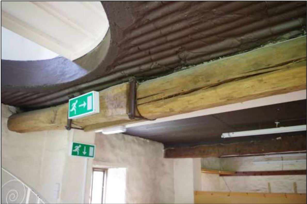
FIGURE 12: BEAM TO NORTH END OF R1, WITH DEEPLY CHAMFERED EDGES AND BRACED WITH HEAVY IRON STRAPS.
