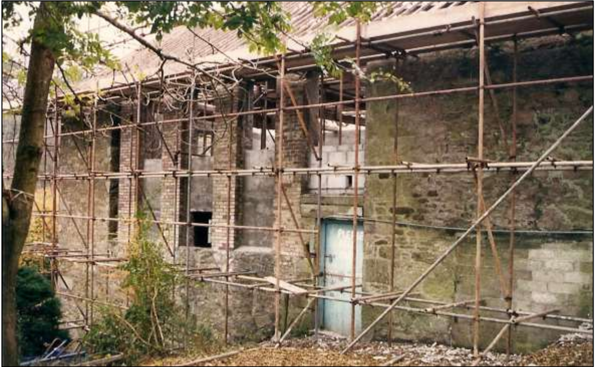
FIGURE 8: THE WEST ELEVATION, THE WALL ABOVE THE FORMER WHEEL PIT HAD BEEN REBUILT DURING THE EARLY-MID 20 TH CENTURY; FROM THE SOUTH-WEST. PHOTOGRAPH COURTESY OF THE CLIENT.
