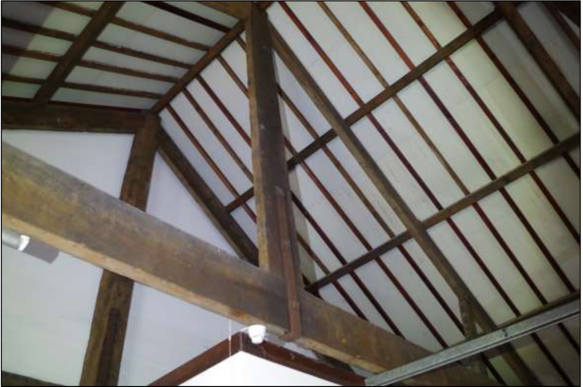
FIGURE 17: A-FRAMES TO THE SOUTH SIDE OF THE BUILDING EXUDE POST-MEDIEVAL, INDUSTRIAL FORM – WITH CENTRAL KING POST STRAPPED WITH HEAVY IRON BRACES TO THE TIE BEAM. TAKEN FROM BELOW TO THE SOUTH END OF R3.
