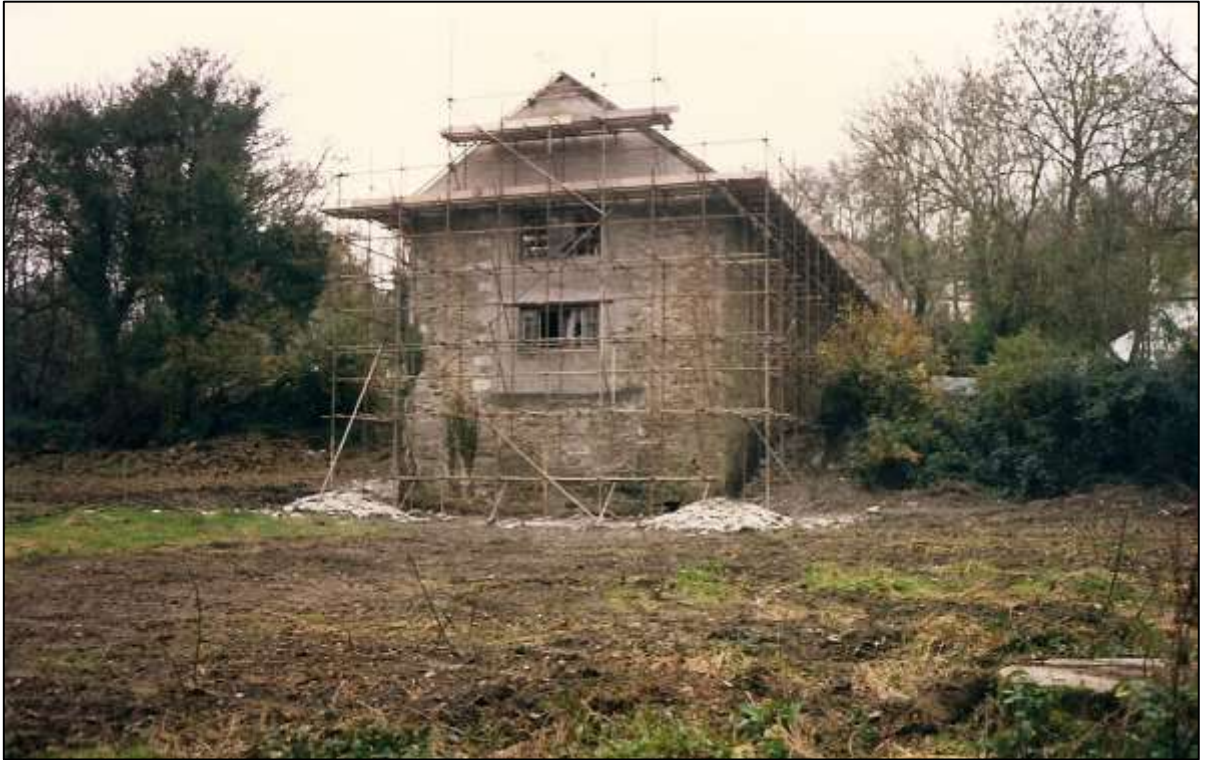
FIGURE 6: THE REBUILDING OF THE NORTH ELEVATION, NOW NEATLY COVERED WITH SLATE-HANGING; FROM THE NORTH-WEST. PHOTOGRAPH COURTESY OF THE CLIENT.
