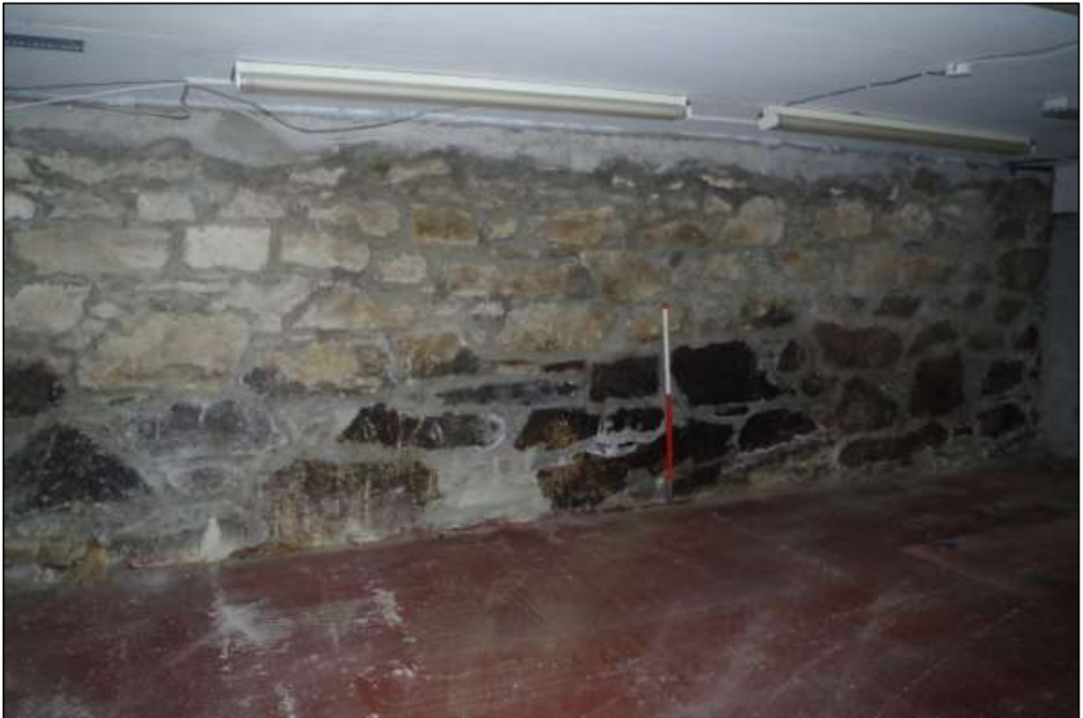
FIGURE 13: THIS IS THE HEAVIEST SECTION OF STONEWORK SEEN THROUGHOUT THE BUILD (ALONG GF SOUTH END), AND INCLUDES LARGE BLOCKS OF GRANITE INDICATIVE OF AN EARLIER BUILD FORM. TAKEN IN R2B FROM NORTH-NORTH-EAST, WITH 1M SCALES.
