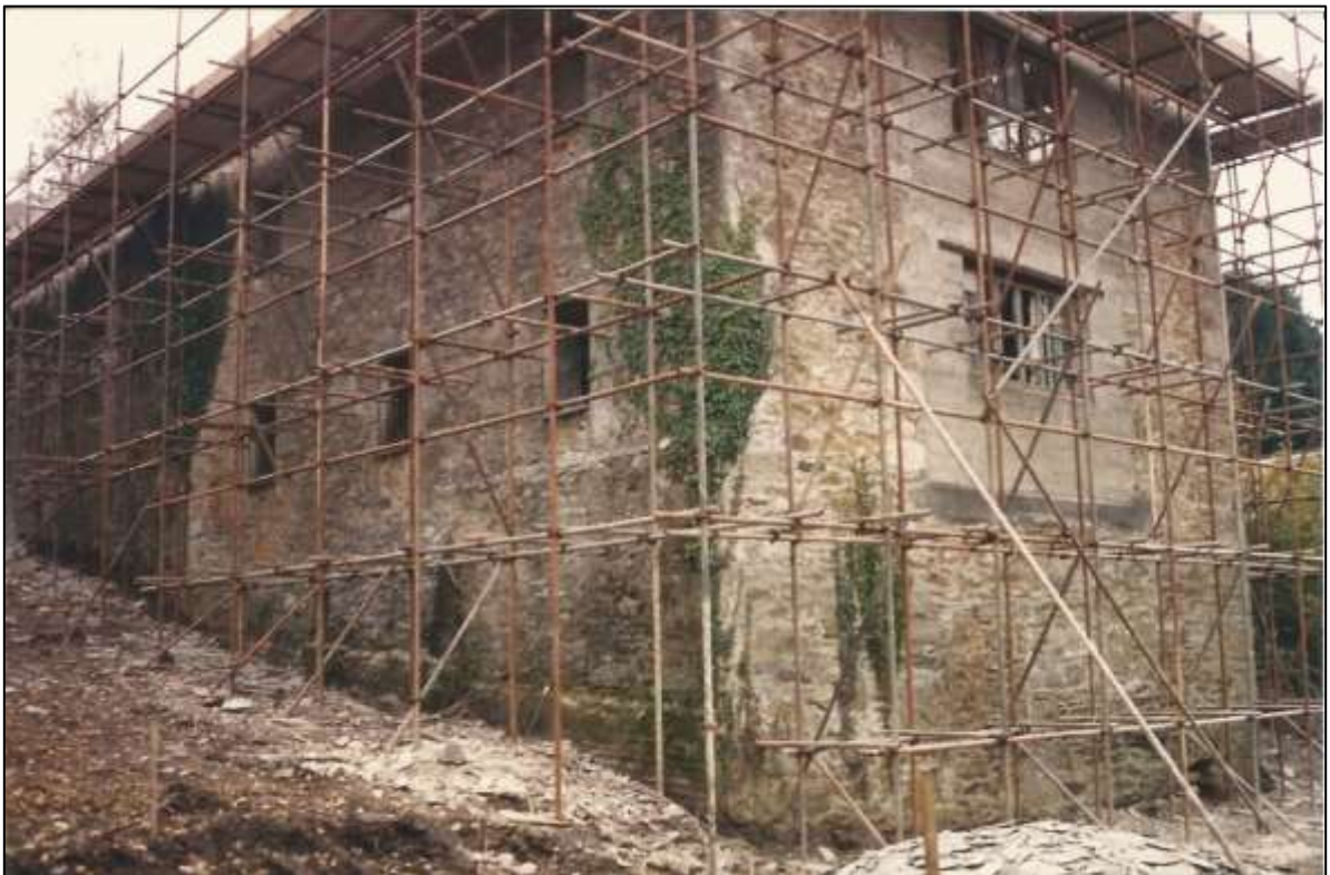
FIGURE 7: THE EAST ELEVATION SHOWING THE OPENINGS HAD BEEN REDUCED BEFORE THIS DATE. NORTH ELEVATION SHOWING POSSIBLY TWO FORMER BLOCKED WINDOW OPENINGS, ONE OF WHICH NOW EXISTS AS A FIRE DOOR AND SLATE RUBBLE FROM FORMER ROOF; FROM THE NORTH-EAST. PHOTOGRAPH COURTESY OF THE CLIENT.
