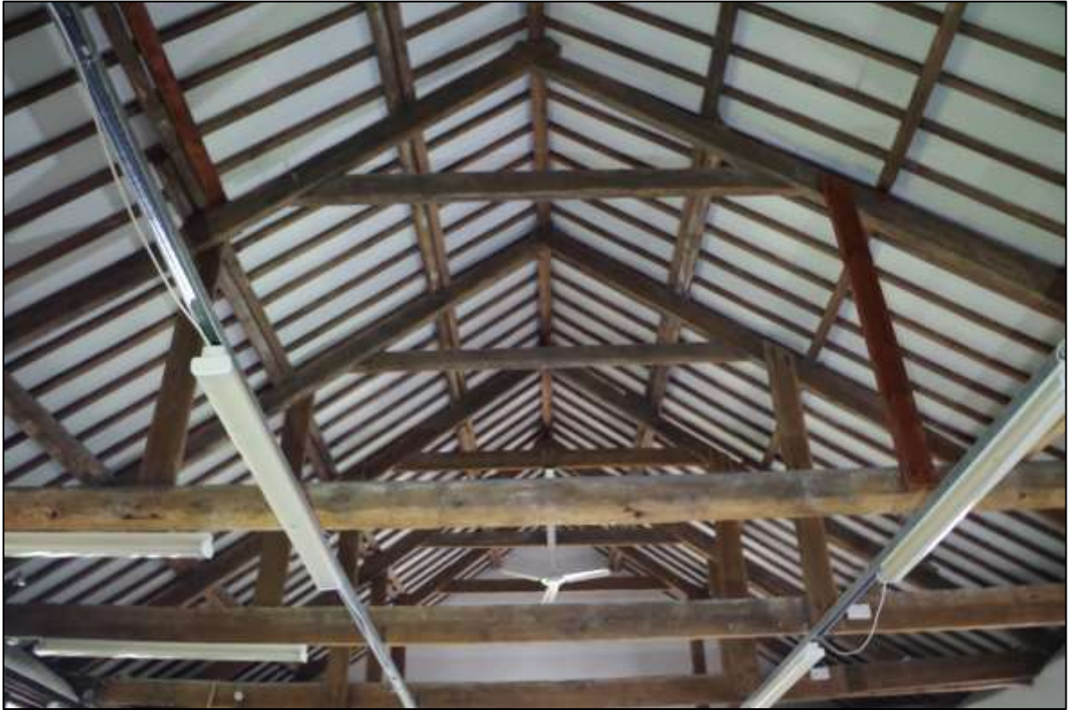
FIGURE 15: THE A-FRAMES TO THE NORTH OF R3 WERE DIFFERENT IN STYLE, PEGGED AT THE RIDGE WITH HALF-LAPPED COLLARS AND RUSTIC TIE-BEAM. TAKEN IN FROM BELOW IN NORTH END OF R3.
