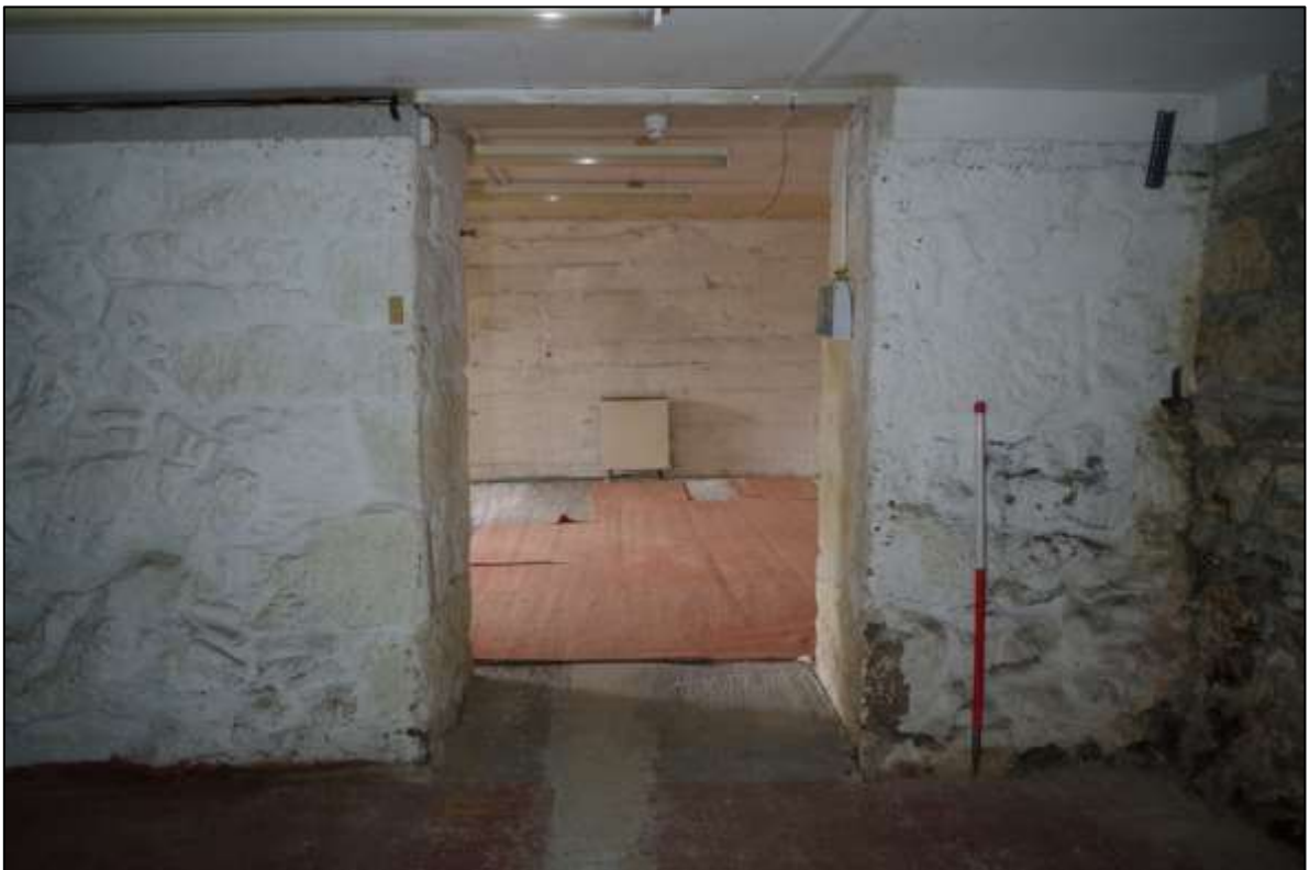
FIGURE 14: THICK STONE WALLS LINING SOUTH ELEVATION OF R2A, LEADING INTO R2B. WALLS HERE ARE PARTICULARLY DEEP, APPROX. 1M, WITH BATTERED WALLS AND VERY GOOD, LARGE QUOIN DETAILING TO THE OPENING (FORMER EXTERIOR WALL SOUTH ELEVATION OF R2A?), ALTHOUGH HAS BEEN REBUILT IN CONCRETE TO TOP. TAKEN FROM THE SOUTH FROM R2B WITH 1M SCALE.
