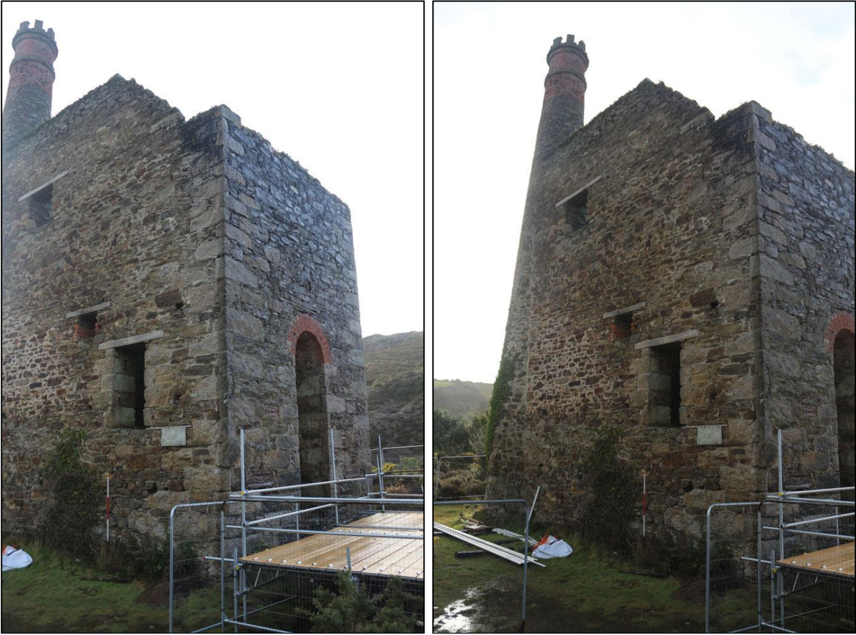
LEFT: THE NORTH-EAST AND NORTH-WEST ELEVATION; VIEWED FROM THE NORTH (2M SCALE). RIGHT: THE NORTH-EAST ELEVATION; VIEWED FROM THE NORTH (2M SCALE).
