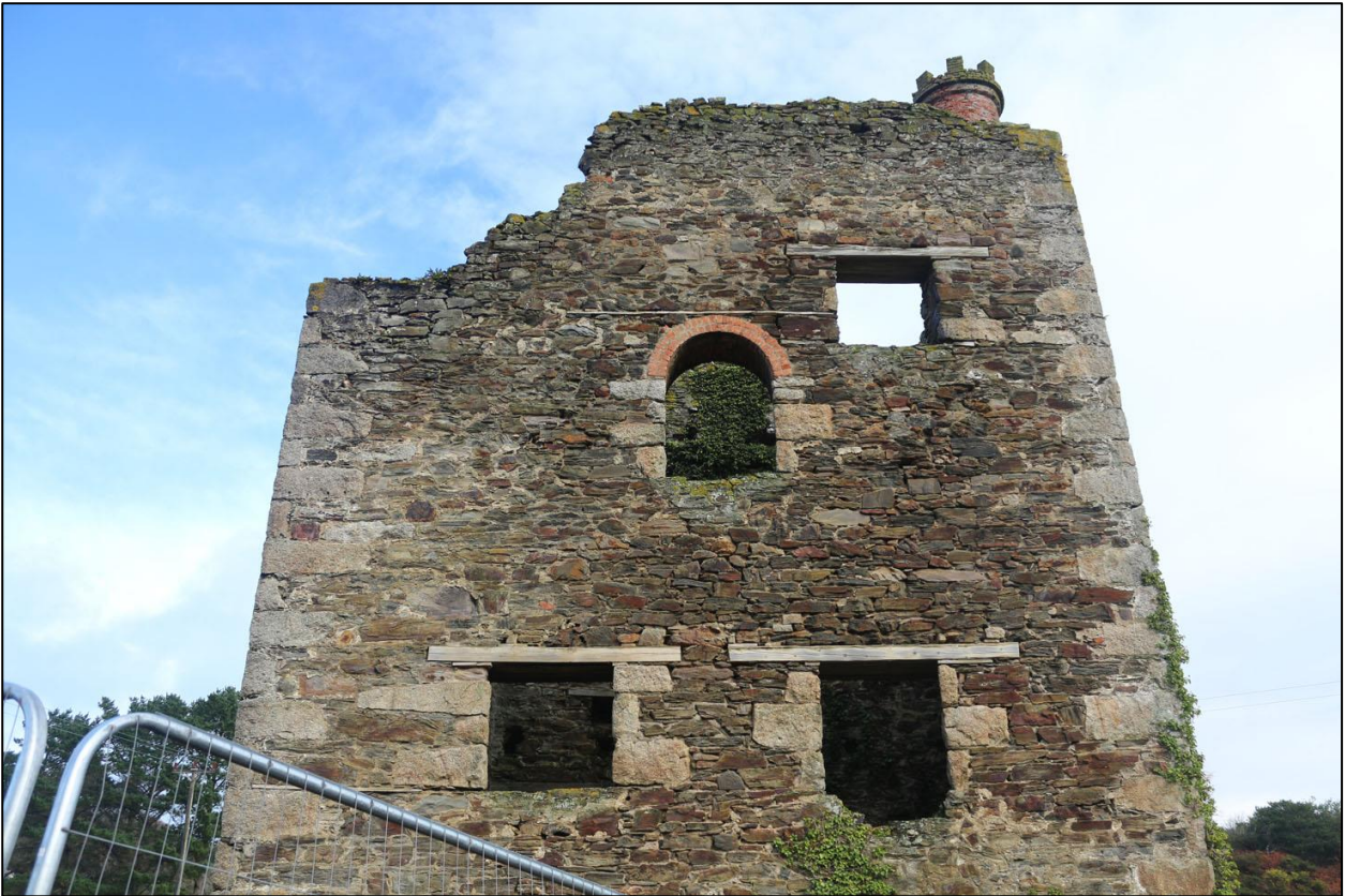
THE UPPER PART OF THE SOUTH-WEST ELEVATION; VIEWED FROM THE SOUTH-WEST (NO SCALE).
