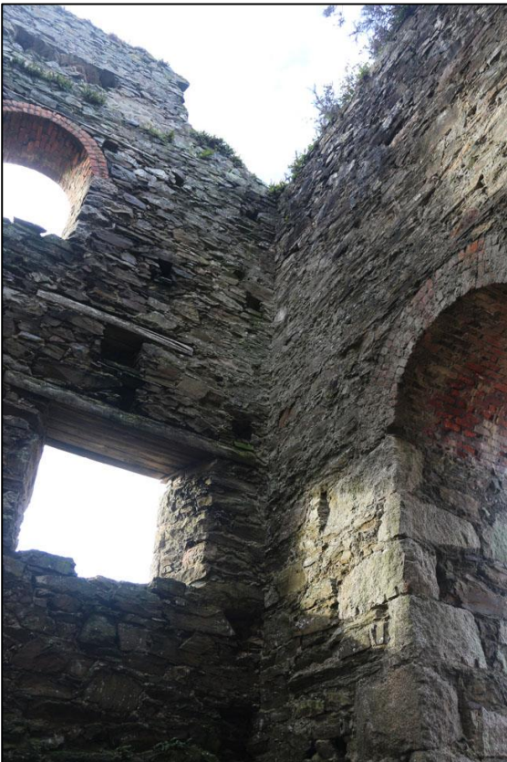
THE WEST CORNER OF THE ENGINE HOUSE AND PLUG DOOR; VIEWED FROM THE EAST (NO SCALE).
