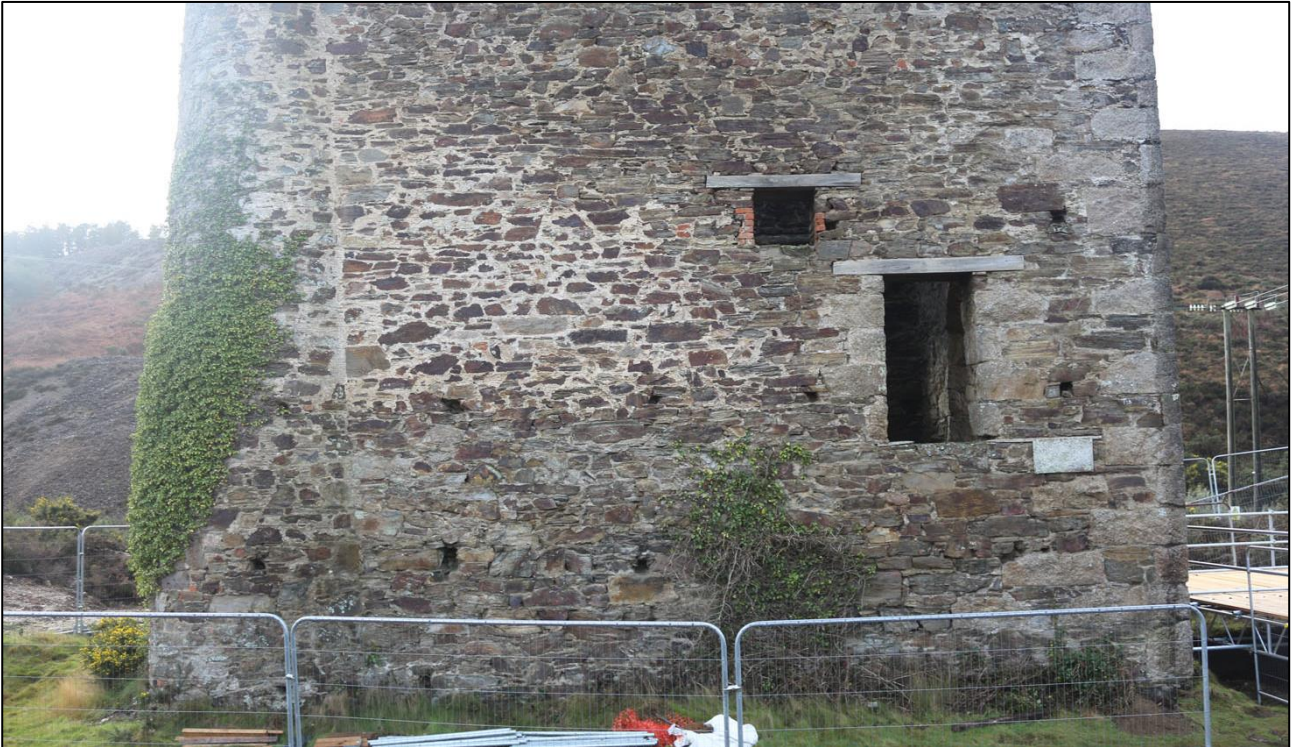
THE LOWER PART OF THE NORTH-EAST ELEVATION; VIEWED FROM THE NORTH-EAST (NO SCALE). NOTE THE PUTLOG HOLES.
