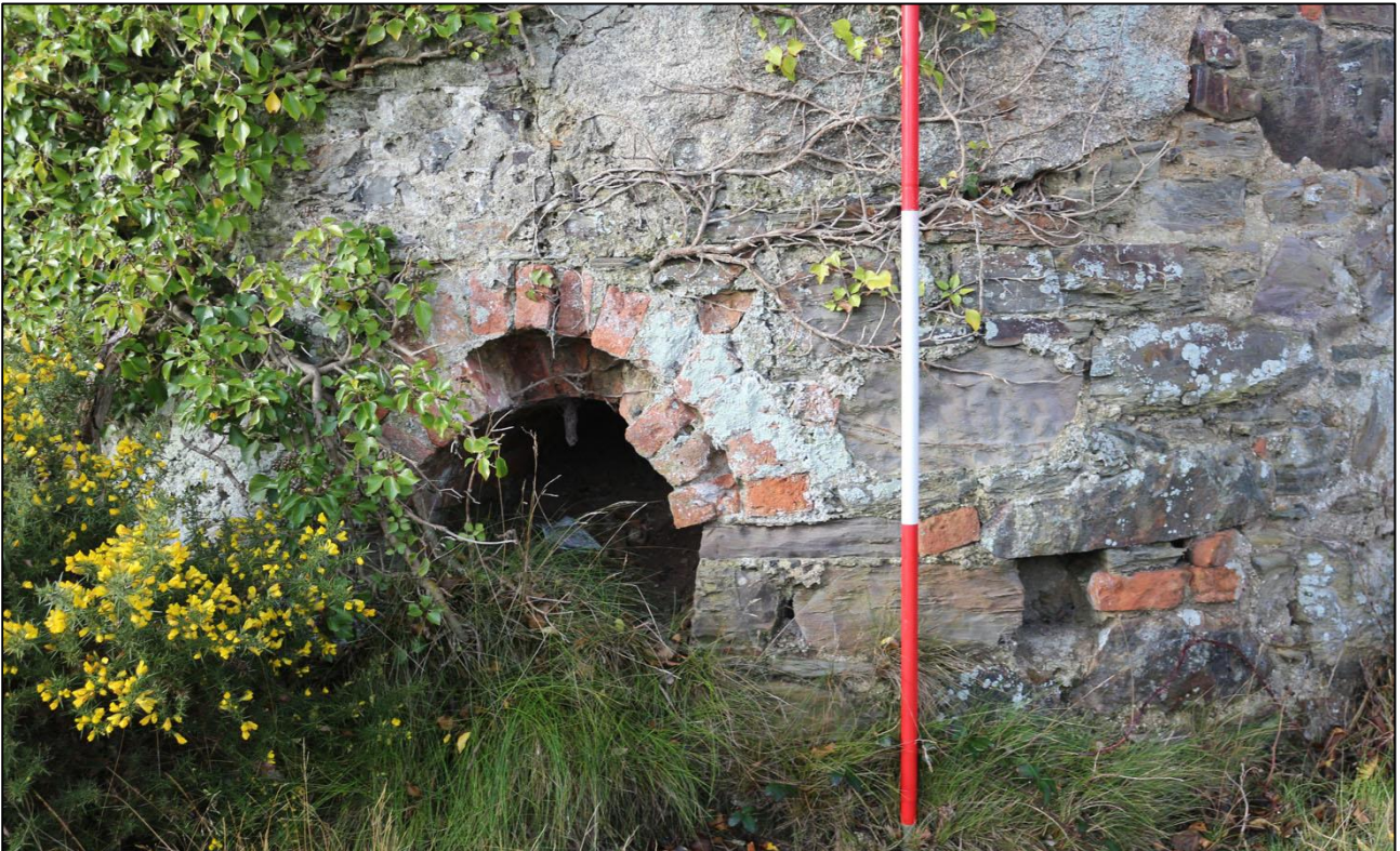
THE BASE OF THE CHIMNEY SHOWING THE STOKE HOLE; VIEWED FROM THE SOUTH-EAST (2M SCALE).
