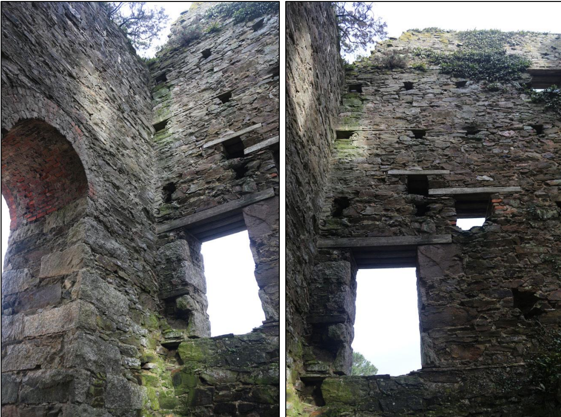
LEFT: THE NORTH CORNER OF THE ENGINE HOUSE AND BOILER HOUSE DOOR; VIEWED FROM THE SOUTH (NO SCALE).
