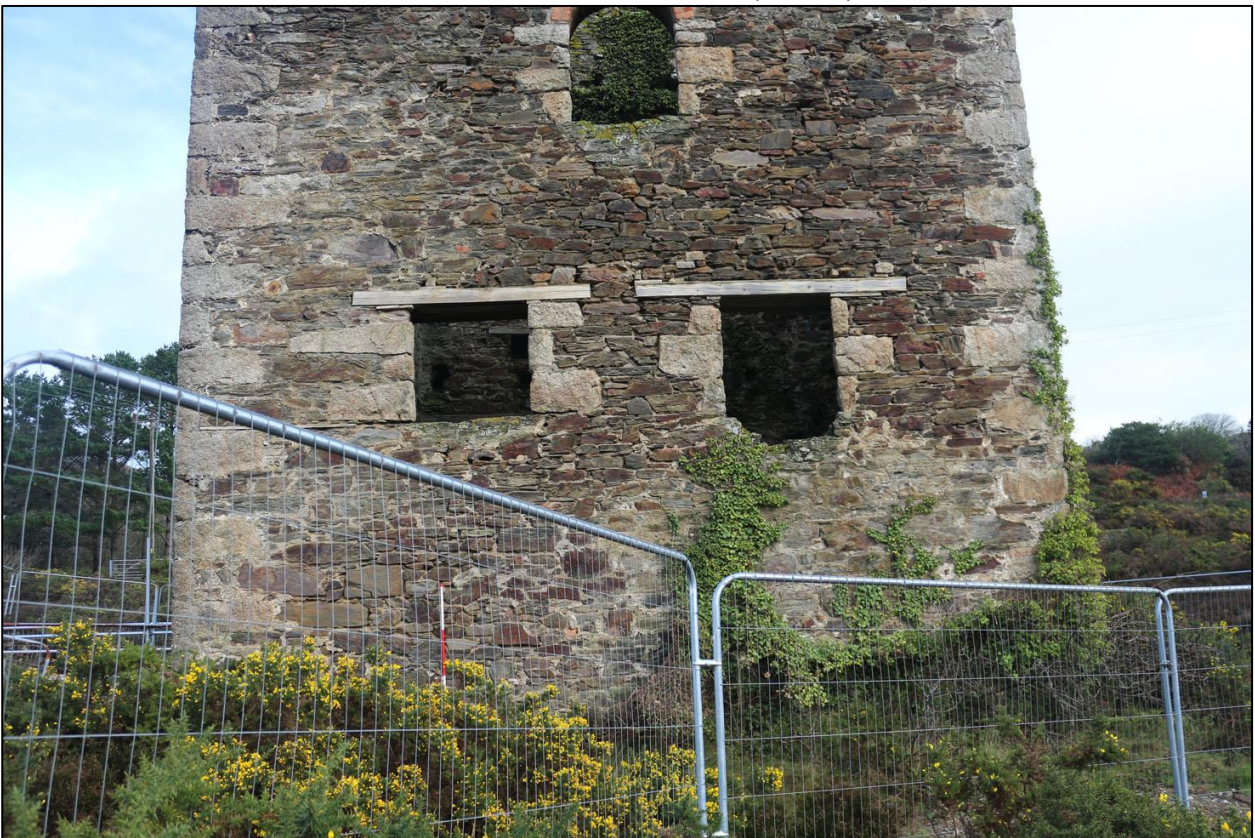
THE LOWER PART OF THE SOUTH-WEST ELEVATION; VIEWED FROM THE SOUTH-WEST (2M SCALE).
