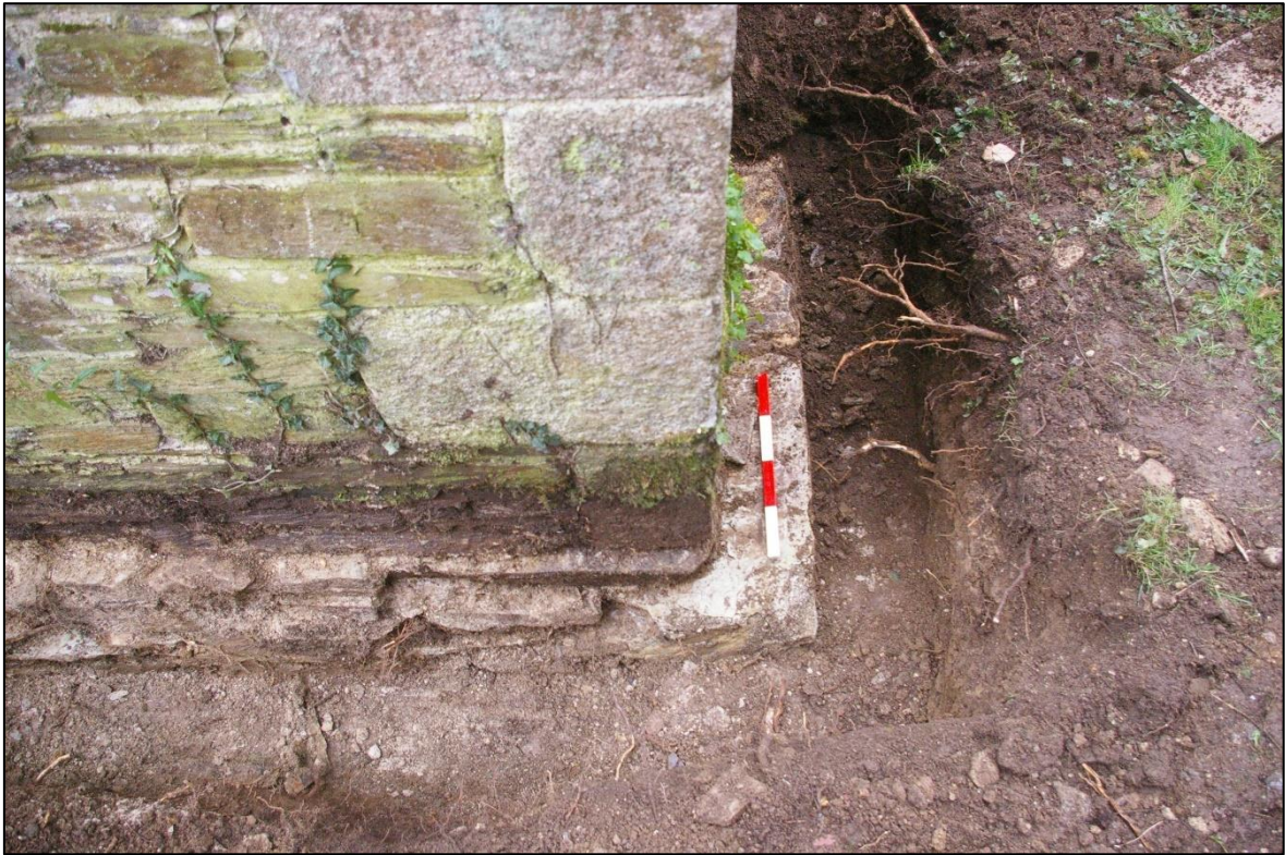
FIGURE 4: THE FOOTING AT THE WESTERN END OF NORTH TRANSEPT; VIEWED FROM THE NORTH (0.4M SCALE).
