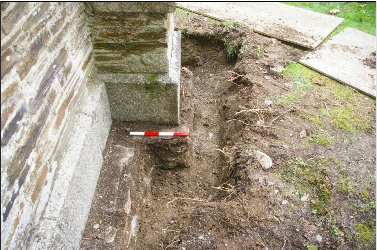
2. THE FOOTINGS OF THE WEST WALL OF THE PORCH AND BUTTRESS; VIEWED FROM THE SOUTH (0.4M SCALE).
