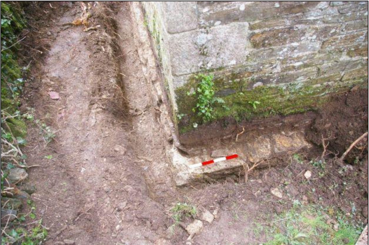
13. THE FOOTINGS OF THE WEST WALL OF THE NORTH TRANSEPT; VIEWED FROM THE EAST (0.4M SCALE).
