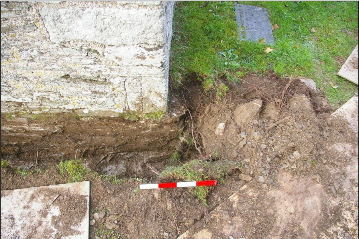
6. THE FOOTINGS OF THE EAST END OF THE SOUTH WALL OF THE SOUTH TRANSEPT; VIEWED FROM THE SOUTH (0.4M SCALE).
