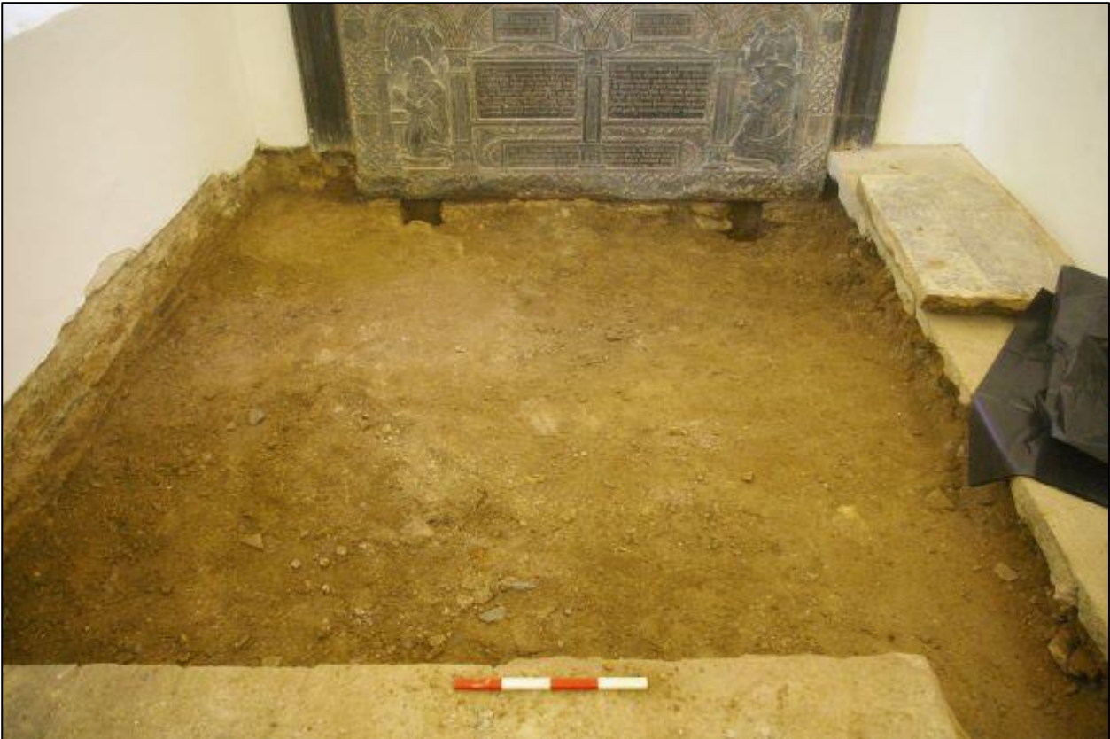
23. THE SOUTH TRANSEPT FOLLOWING THE WORK; VIEWED FROM THE NORTH (0.4M SCALE).
