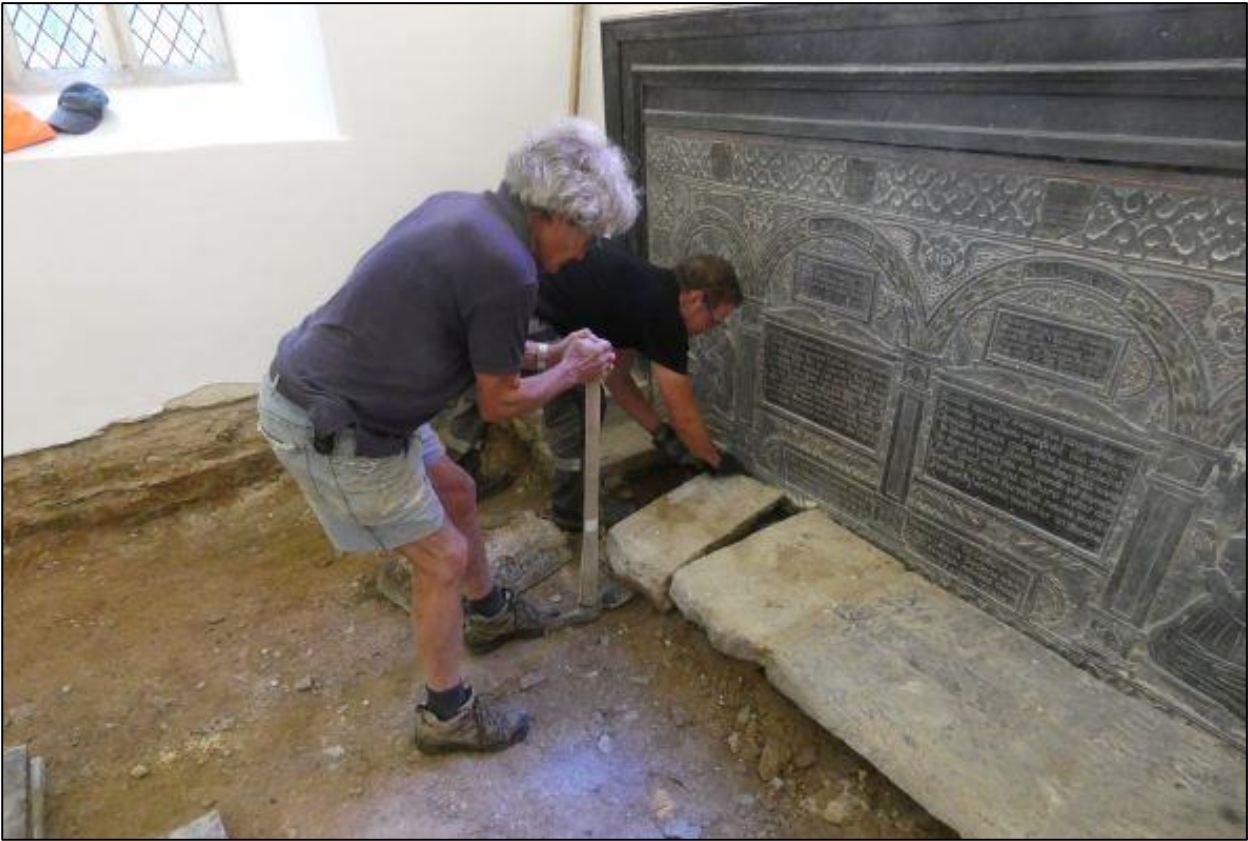
15. WORKS IN PROGRESS LIFTING SLABS IN FRONT OF VERMAN MEMORIAL; VIEWED FROM THE NORTH-WEST (PHOTO BY A. LANGDON).
