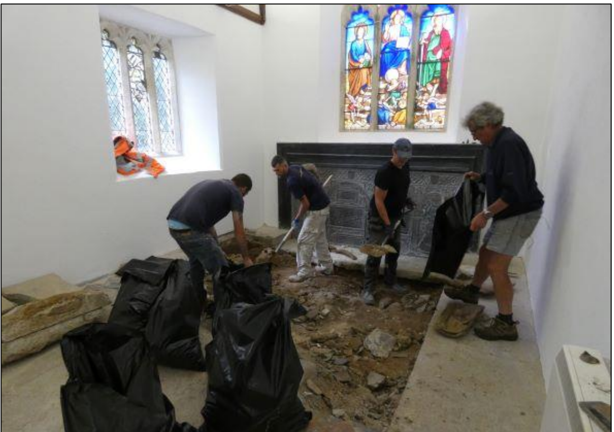
14. WORKS IN PROGRESS REDUCING THE FLOORS IN THE SOUTH CHANCEL; VIEWED FROM THE NNW (PHOTO BY A. LANGDON).
