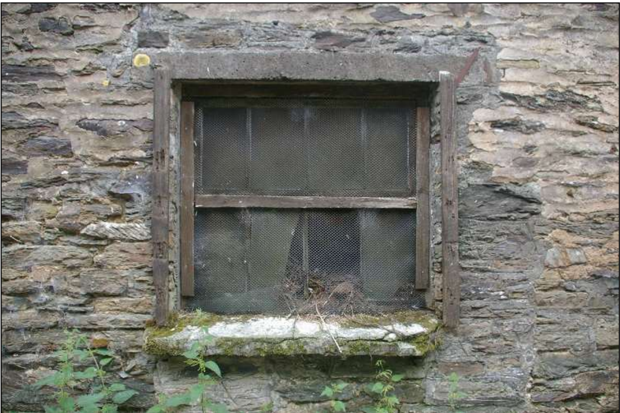
2. ONE OF THE GROUND-FLOOR WINDOWS FORCED INTO THE EAST WALL OF THE GREAT BARN AT CORNHAM; VIEWED FROM THE EAST.
