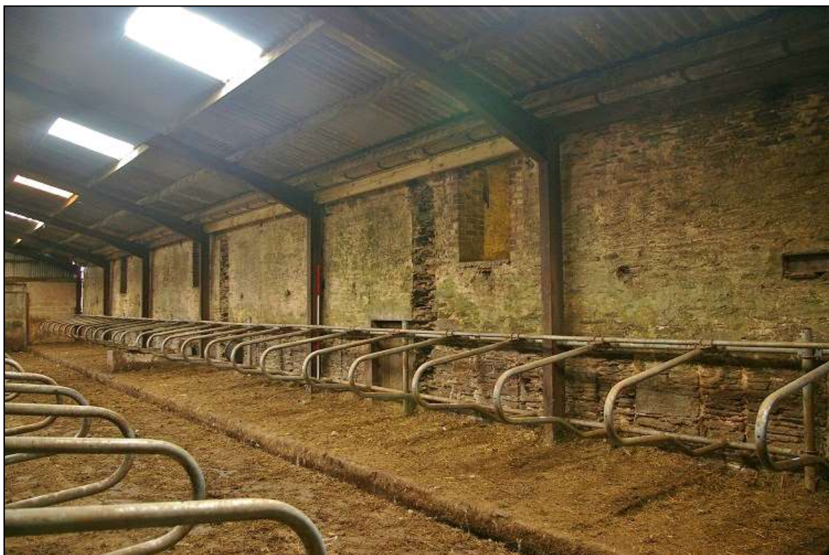
FIGURE 6: THE WEST ELEVATION OF CORNHAM GREAT BARN, ENCLOSED WITHIN A MODERN COWSHED (2M SCALE); VIEWED FROM THE SOUTH-WEST.
