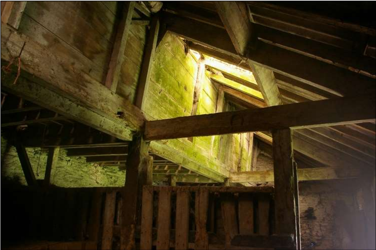
22. THE JETTIED LOFT, AS SEEN IN ROOM B, NOW A STABLES; VIEWED FROM THE SOUTH-EAST.
