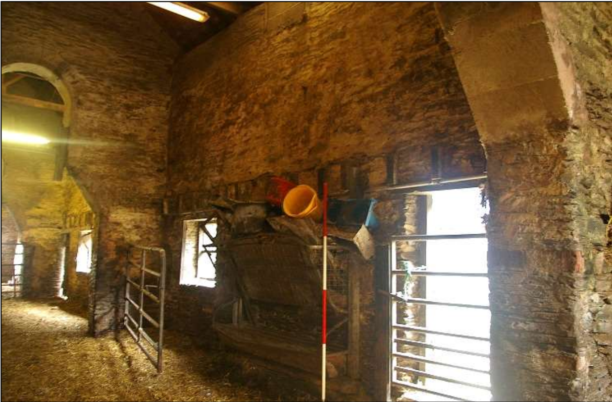
10. THE EAST WALL OF CORNHAM GREAT BARN, SHOWING THE HEAVY SAWN LOFT JOISTS (2M SCALE); VIEWED FROM THE SOUTH-WEST.
