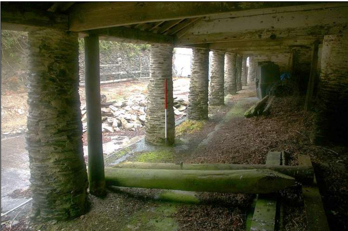
31. THE EAST END OF THE NORTH AISLE (2M SCALE); VIEWED FROM THE WEST.
