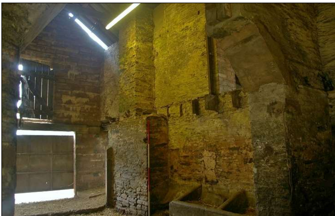
FIGURE 8: THE FIREPLACE INSERTED INTO THE SOUTHERN BAY (ROOM D) (2M SCALE); VIEWED FROM THE NORTH-EAST.
