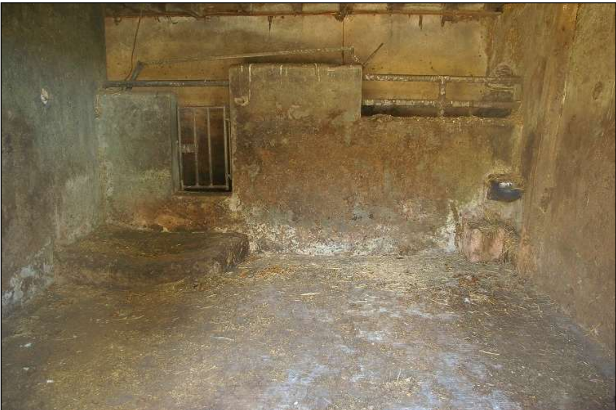
23. ONE OF THE MODERNISED RENDERED PENS TO THE WEST SIDE OF THE BUILDING; VIEWED FROM THE WEST.
