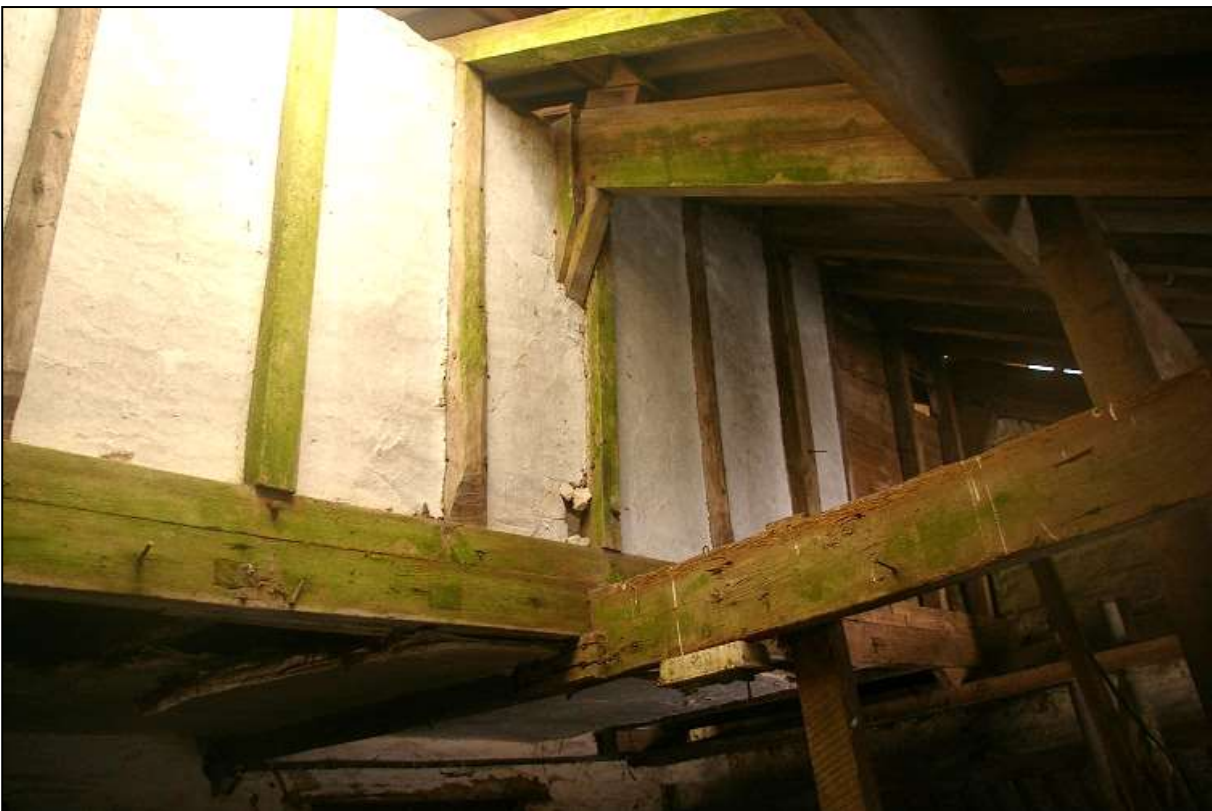
27. THE LIME PLASTERED PLANK LOFT PARTITIONS, JETTIED OVER ROOM G WHICH HAD BEEN CONVERTED TO ACCOMMODATION IN THE PAST; VIEWED FROM THE NORTH-WEST.
