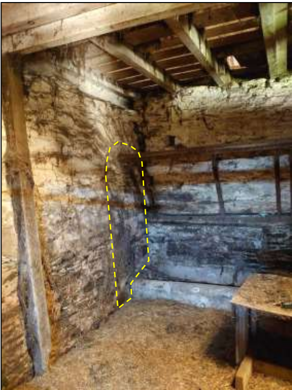
21. THE LOCATION OF THE FORMER FEED PASSAGE DOOR IN ROOM B (INDICATED), BLOCKED AND OBSCURED BY HAYRACKS AND TROUGHES; VIEWED FROM THE EAST-NORTH-EAST.
