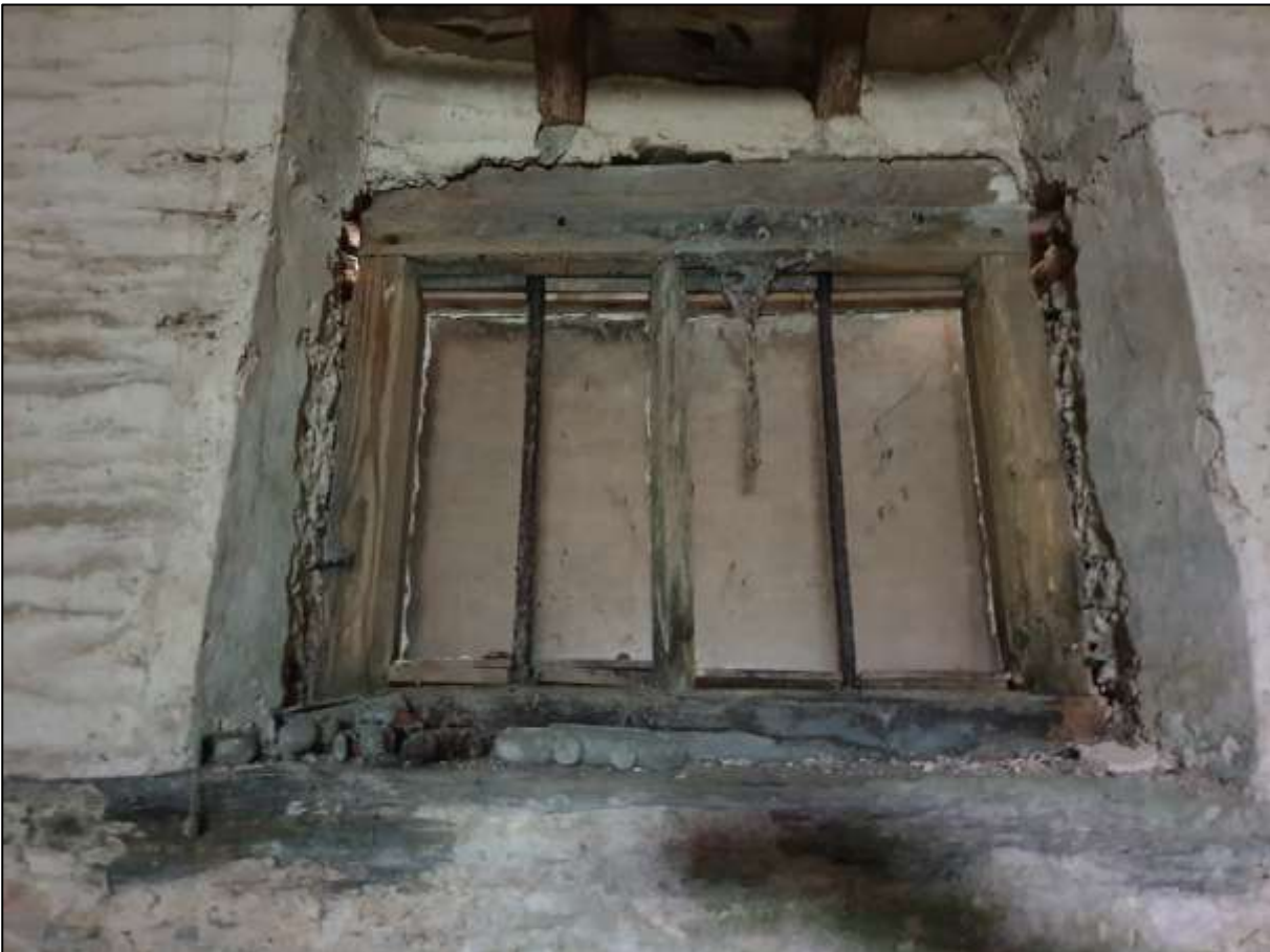
35. DETAIL OF ONE OF THE SURVIVING FIRST-FLOOR WINDOWS; VIEWED FROM THE NORTH=NORTH-EAST.
