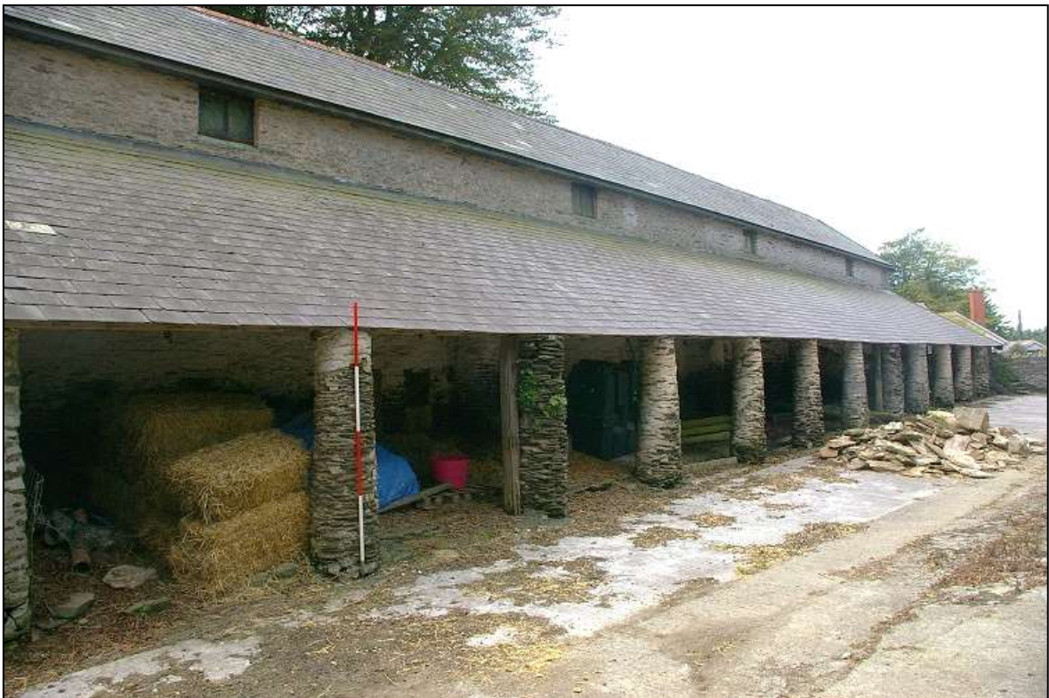
FIGURE 17: THE NORTH ELEVATION OF THE GREAT BARN AND ITS ORIGINAL AISLE (2M SCALE); VIEWED FROM THE NORTH-EAST.
