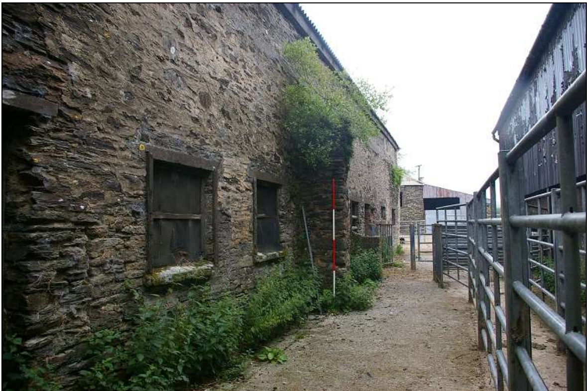
FIGURE 5: THE EAST ELEVATION OF THE GREAT BARN AT CORNHAM (2M SCALE); VIEWED FROM THE SOUTH-EAST.
