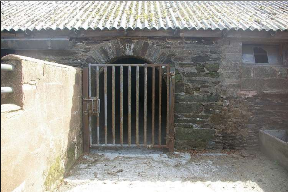
16. ONE OF THE ROUND-HEADED DOORWAYS IN THE WEST WALL, WITH FORCED AND THEN PARTLY BLOCKED WINDOW TO THE RIGHT; VIEWED FROM THE WEST.
