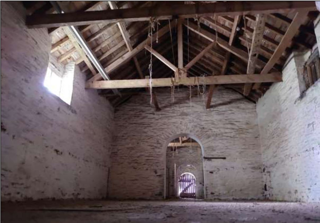
37. THE FIRST FLOOR OF HONEYMEAD GREAT BARN, WITH ROOF STRUCTURE IDENTICAL TO THAT AT CORNHAM, THE WINDOWS WITH SURVIVING FRAMES; VIEWED FROM THE WEST-NORTH-WEST.
