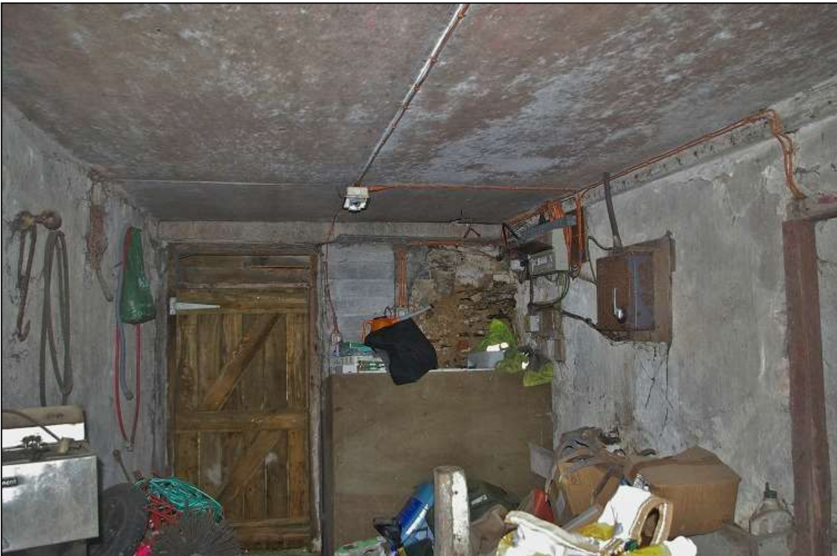
25. ROOM D AT THE NORTH END OF THE MAIN RANGE, WITH A DOOR TO THE COURTYARD NEXT TO THE FARMHOUSE; VIEWED FROM THE WEST.
