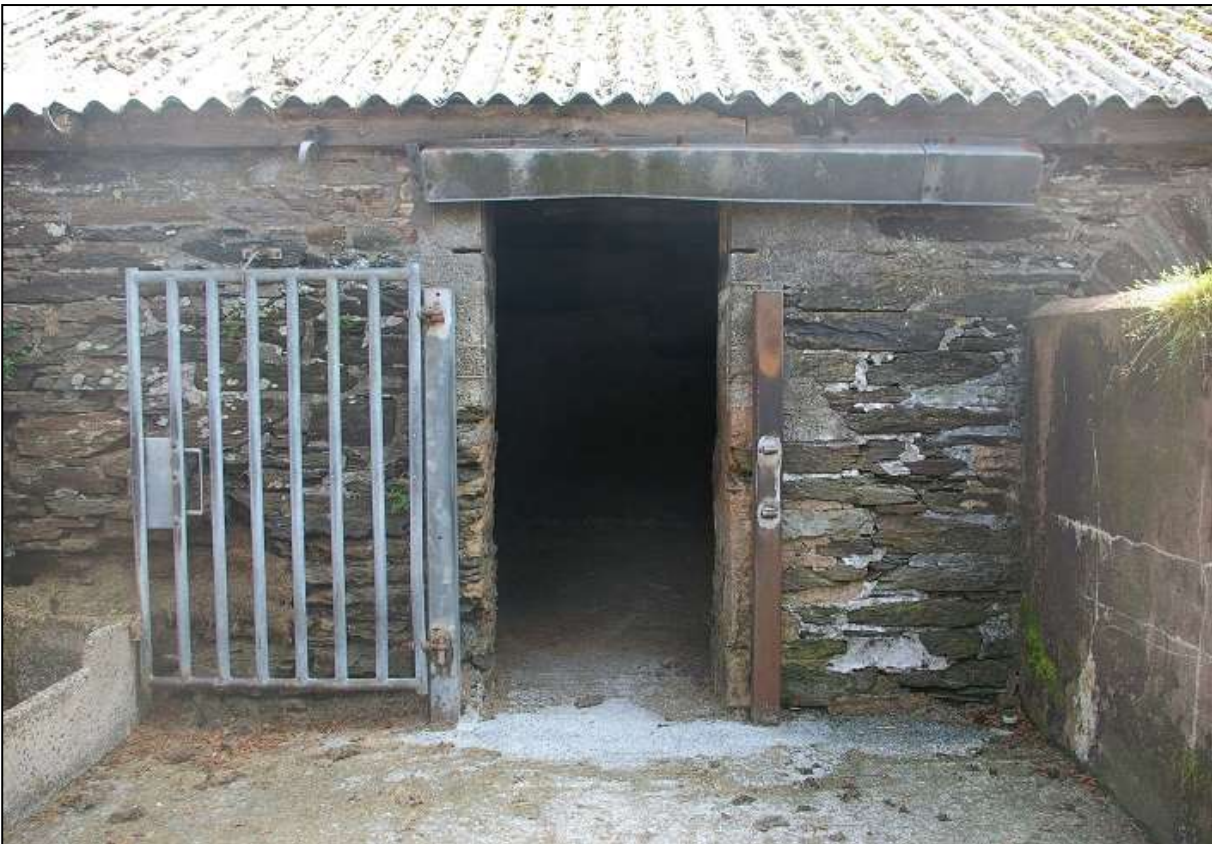
17. ONE OF THE FORCED DOORS IN THE WEST ELEVATION; VIEWED FROM THE WEST.
