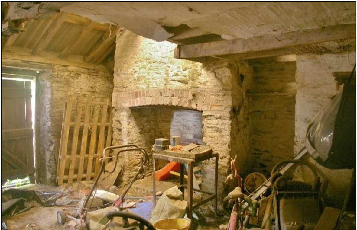
FIGURE 15: THE FIREPLACE AND PLASTER CEILING IN ROOM G; VIEWED FROM THE SOUTH-EAST.
