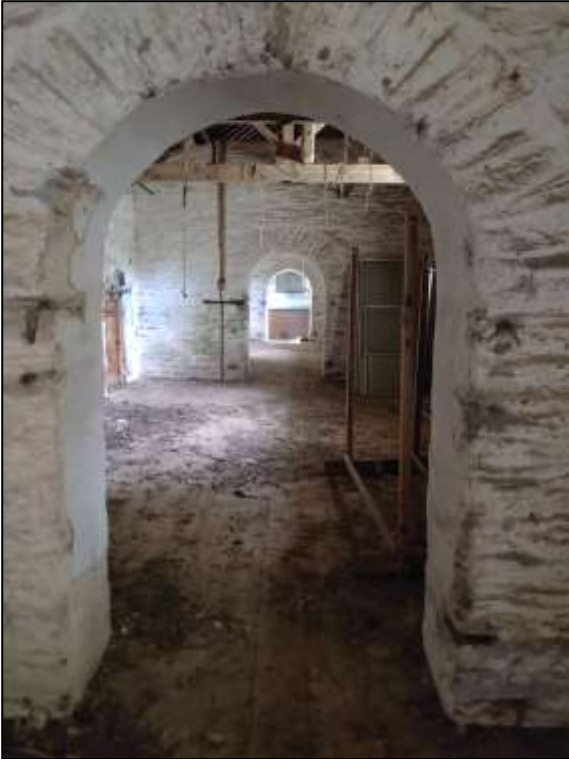
39. VIEW ALONG THE FIRST FLOOR OF HONEYMEAD GREAT BARN, LOOKING THROUGH THE ROUND-HEADED DOORWAYS; VIEWED FROM THE WEST-NORTH-WEST.
