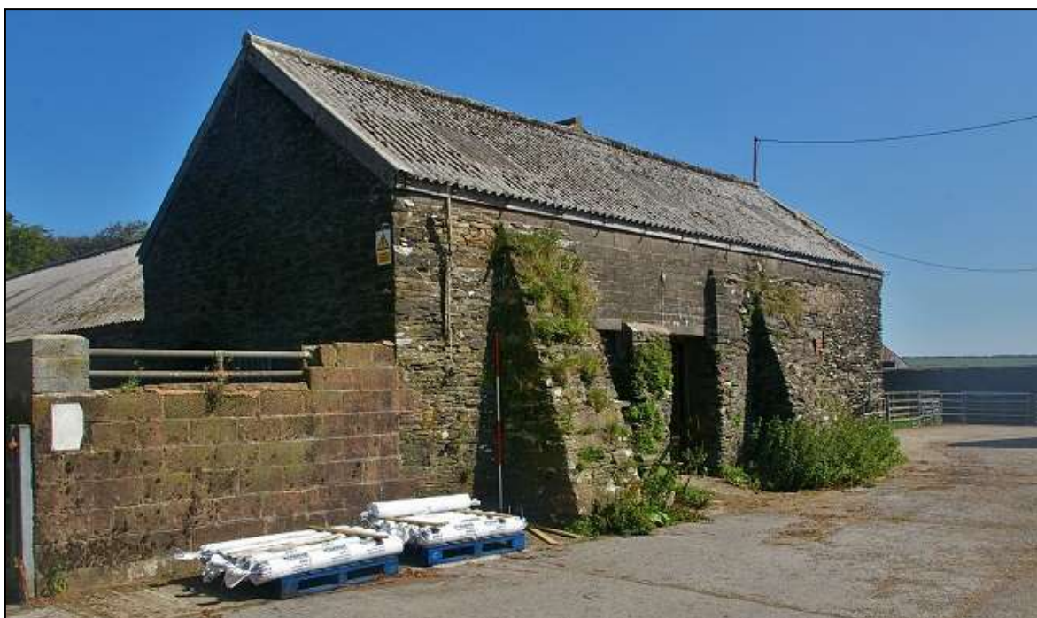
FIGURE 9: THE STABLES/BULLPEN AT CORNHAM, THE SOUTH EXTENSION (2M SCALE); VIEWED FROM THE SOUTH-WEST.
