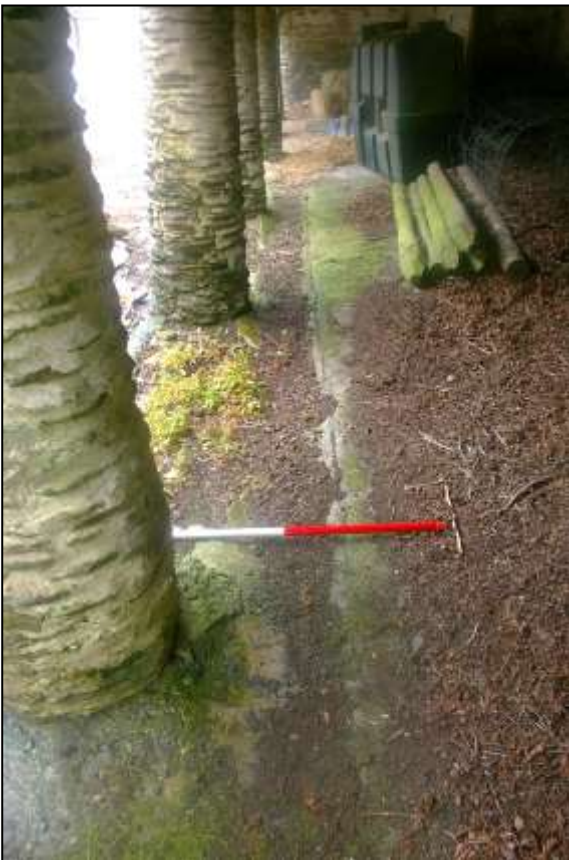
33. THE DRAIN TO THE OPEN FRONT OF THE NORTH AISLE (1M SCALE); VIEWED FROM THE WEST.
