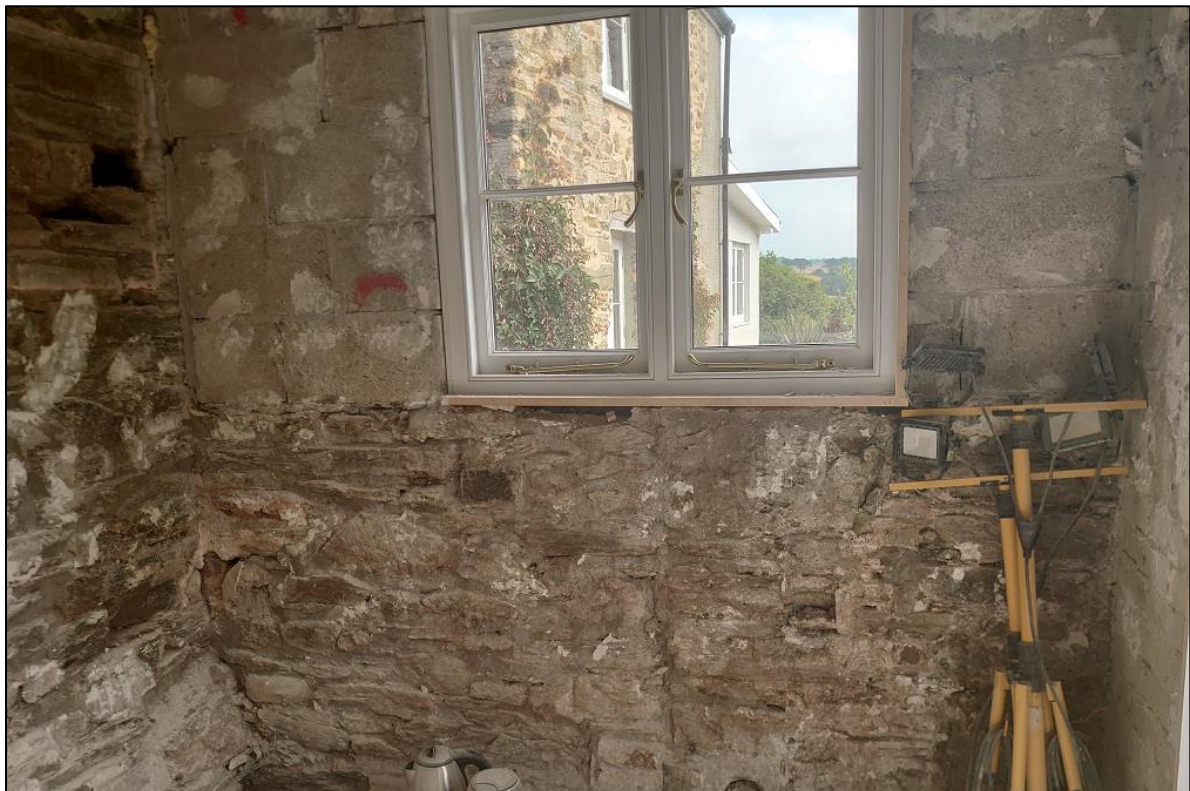
FIGURE 16: THE EAST WALL OF THE PORCH, SHOWING POST MEDIEVAL STONEMASONRY AND CONCRETE BLOCK MODERN RAISE TO THE WALL, WHICH IS PROPOSED FOR REMOVAL; FROM THE WEST.
