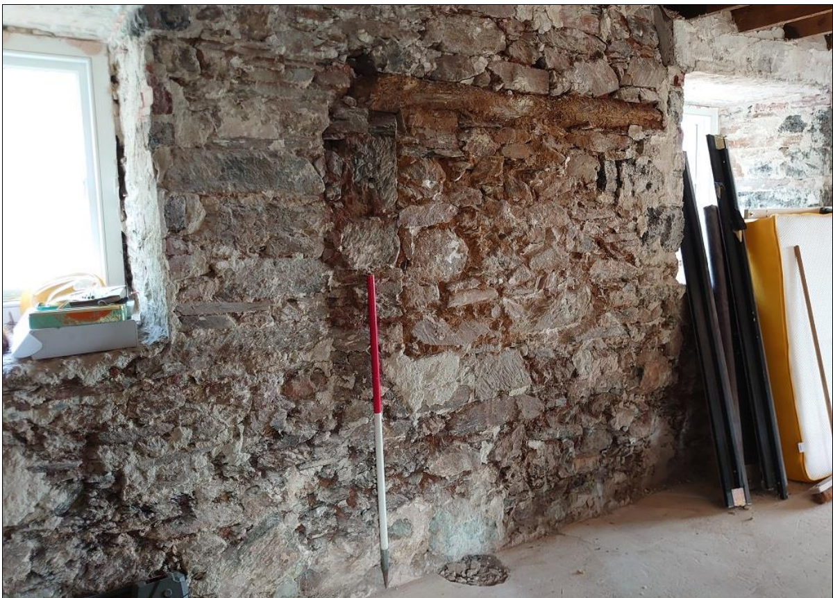
78. THE BLOCKED WINDOW IN THE NORTH WALL OF THE FARMHOUSE, WITHIN THE MEDIEVAL STONEMWORK, BLOCKED BY POST MEDIEVAL RUBBLE (1M SCALE); FROM THE SOUTH-WEST.
