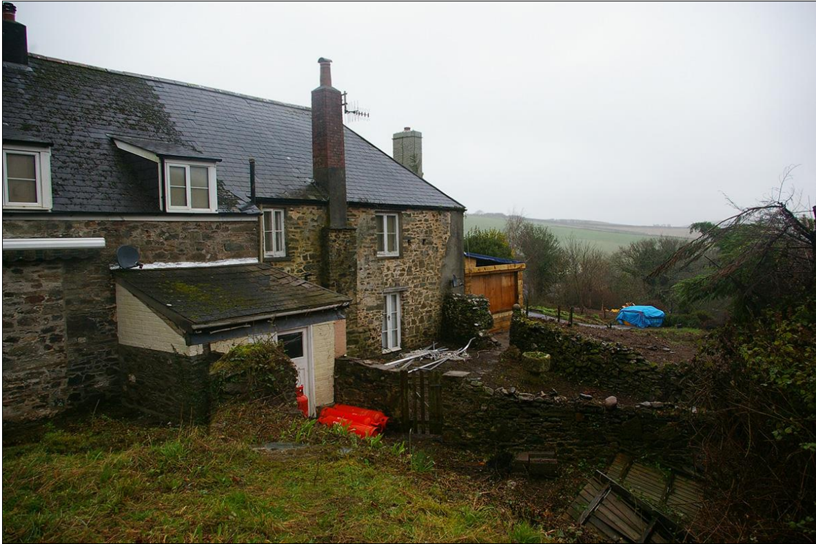
48. THE SOUTH ELEVATION OF THE FARMHOUSE, SHOWING THE PROJECTION TO THE WEST AND SMALL LATERAL STACK BUILT AGAINST THE EARLIER STONework OF THE MEDIEVAL RUIN, WHICH OCCUPIES A SECTION TO THE CENTRE OF THE WALL, FROM THE SOUTH-WEST.
