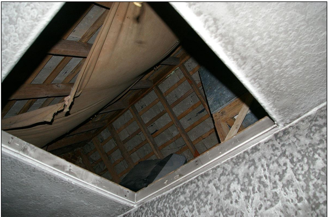
32. VIEW UP INTO THE LOFT, SHOWING THE MODERN COMMON RAFTER REPLACEMENT ROOF; FROM BELOW (NORTH-WEST).
