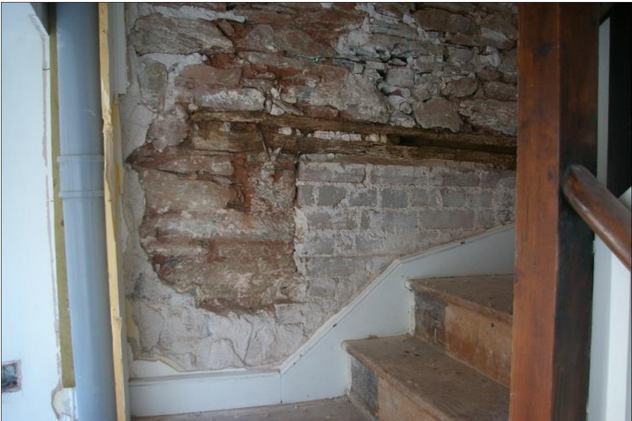
68. BLOCKED DOOR WITHIN FARMHOUSE AND COTTAGE, BLOCKED BY BRICKWORK.
