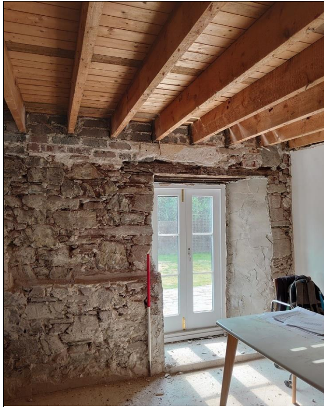
79. STEPPED MEDIEVAL FABRIC IN THE SOUTH WALL OF THE FARMHOUSE AT GROUND FLOOR LEVEL (1M SCALE); FROM THE NORTH-EAST.
