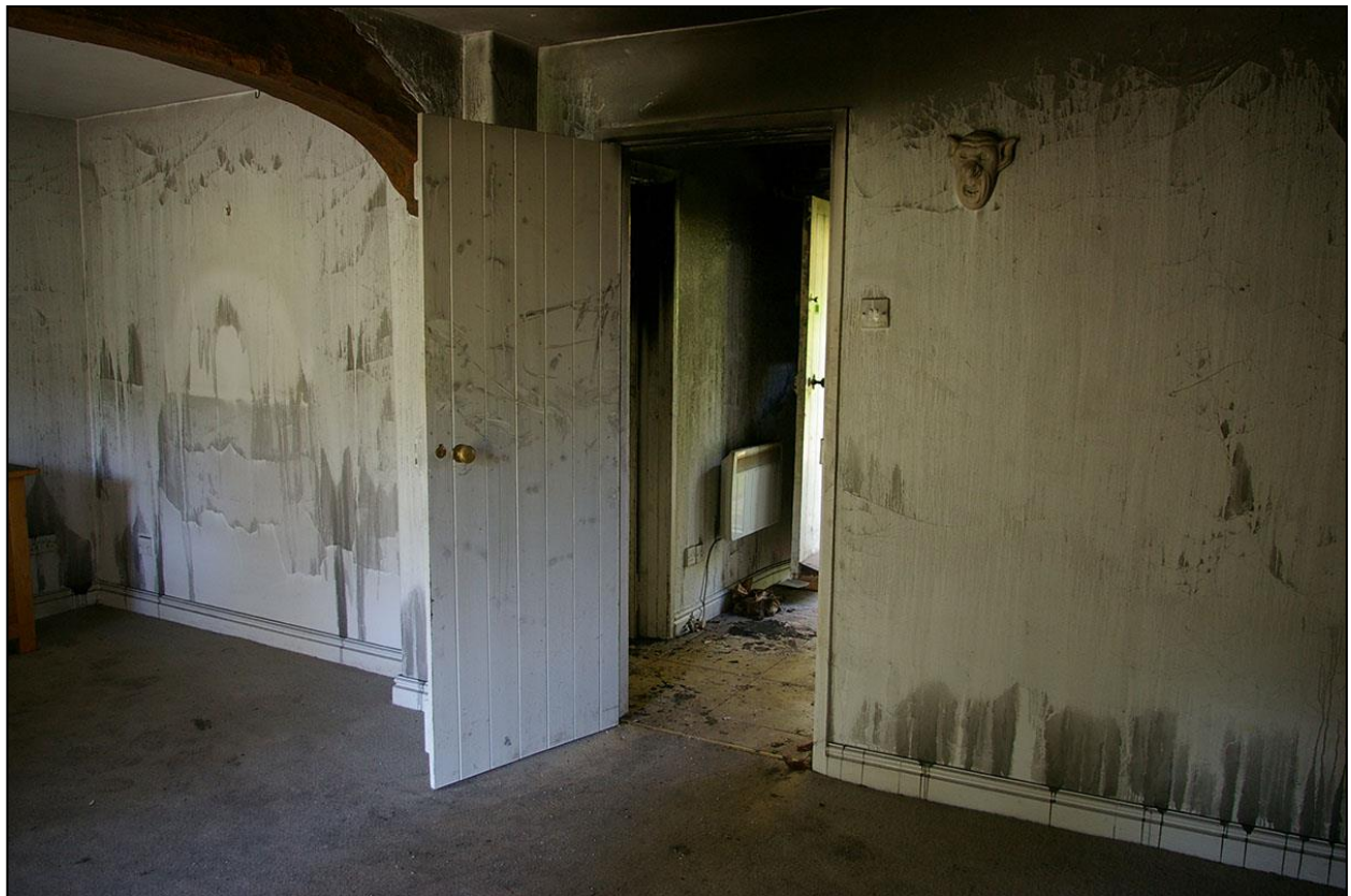
22. THE MODERN PARTITIONS, WITH A STUD OF EARLIER WALL BRACED BY A HACKED BACK BEAM IN CR3, THE SITTING ROOM, ALSO WITH DOOR BACK TO THE HALLWAY; FROM THE SOUTH-EAST.
