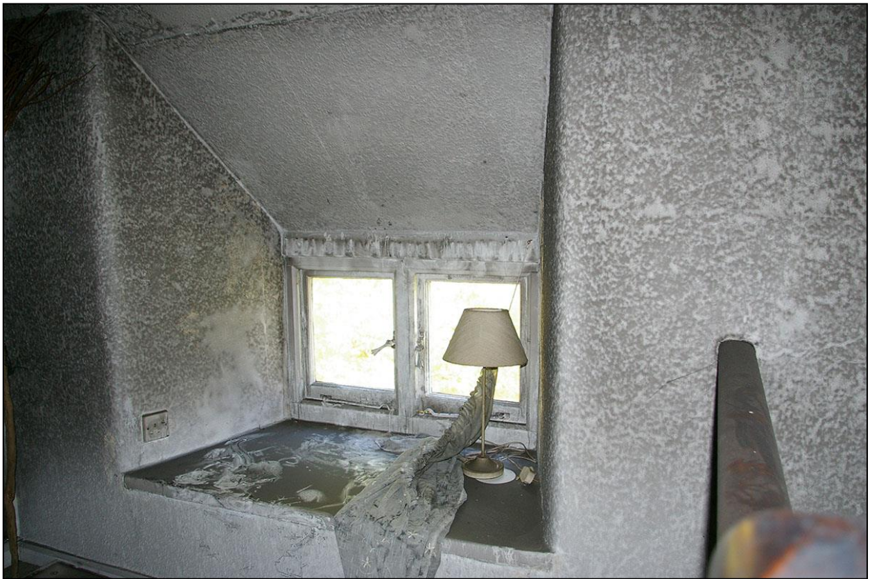
28. THE TWO LIGHT WINDOW SET INTO A BLOCKED LOADING DOOR IN THE FRONT WALL, CW4; FROM THE SOUTH-EAST.
