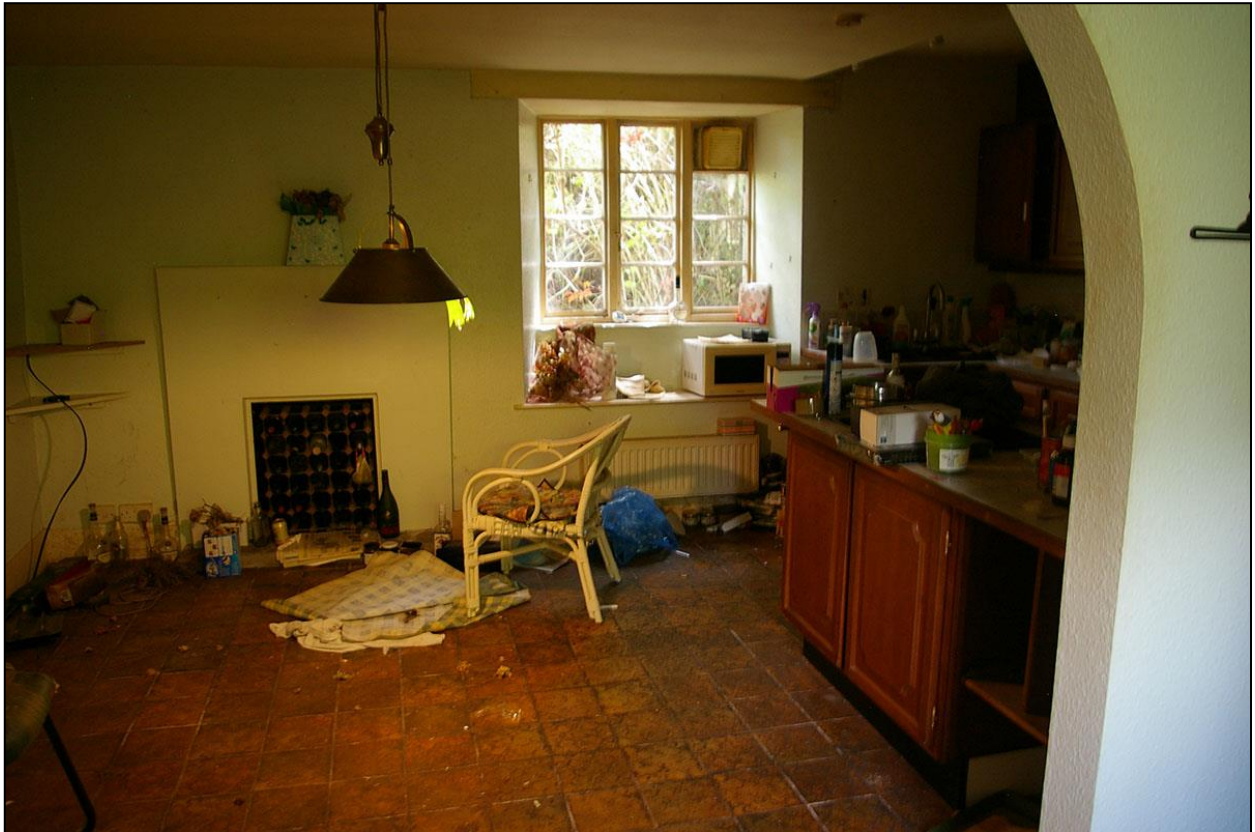
11. THE FITTED KITCHEN, WITH THE THREE LIGHT 19 TH CENTURY CASEMENT AND WINDOW SEAT, BLOCKED FIREPLACE ON THE REAR WALL, MODERN QUARRY TILED FLOOR, BOARDED OUT CEILING WHICH OBSCURES A CHANGE IN CEILING HEIGHT; FROM THE NORTH, NORTH-EAST.
