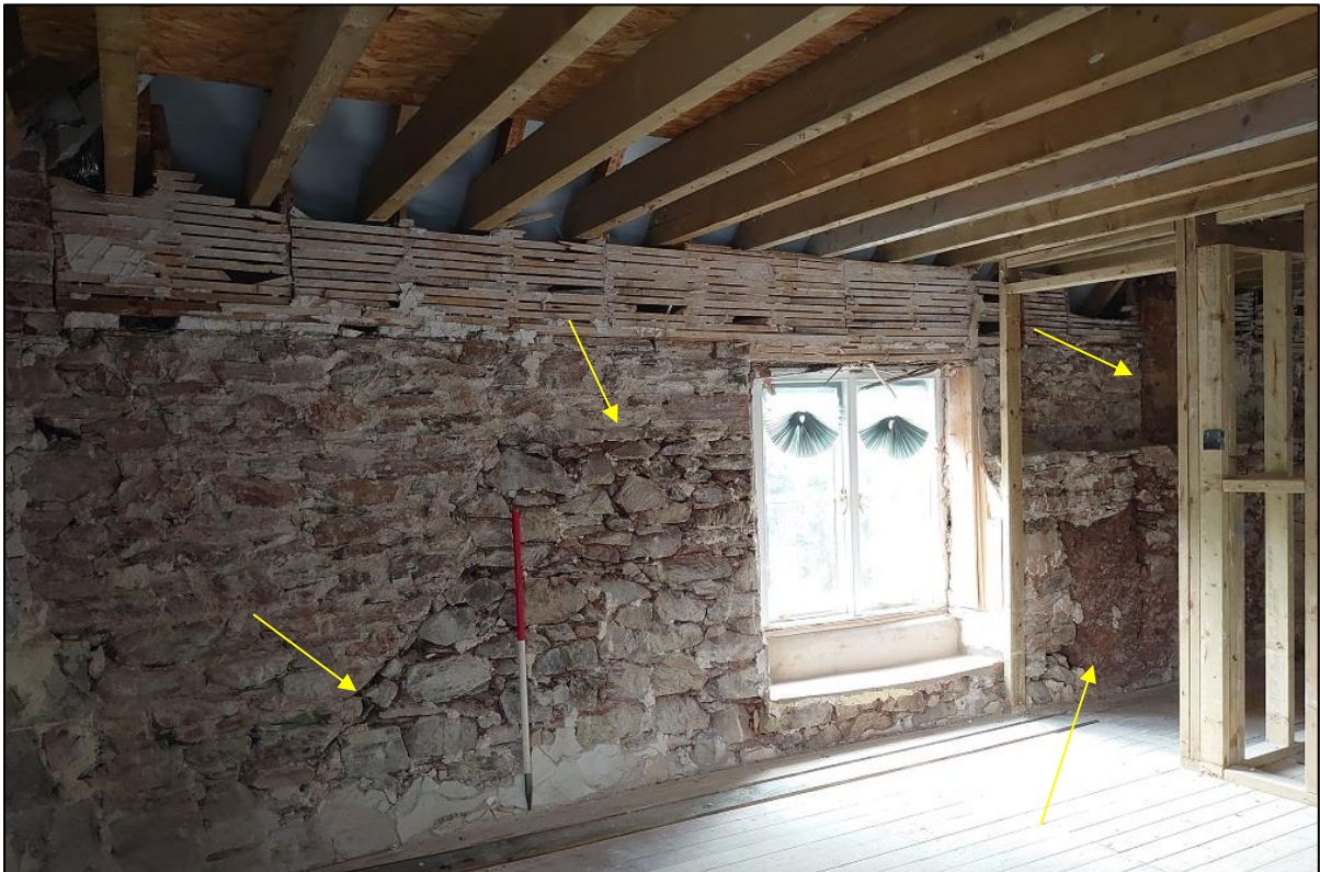
FIGURE 18: THE SOUTH WALL OF THE FARMHOUSE, AGAIN ILLUSTRATING THE COMPLEX PHASING OF THE WALLS (1M SCALE); FROM THE NORTH-EAST.
