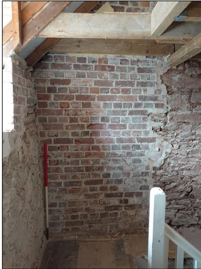
FIGURE 21: THE REBUILT BRICKWORK TO THE SOUTH OF THE CENTRAL PARTITION WALL BETWEEN THE FARMHOUSE AND COTTAGE , OF 19 TH CENTURY DATE, (1M SCALE), FROM THE EAST.
