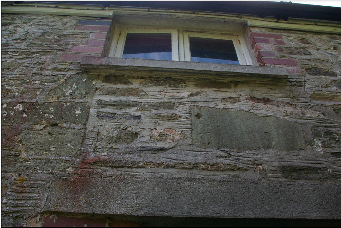
13. THE SMALL BLOCKED WINDOW WITH BRICK REVEALS SET INTO A LARGER OPENING, A LOADING DOOR ABOVE THE FORCED DOORWAY TO THE FRONT OF THE ATTACHED COTTAGE; FROM BELOW (NORTH-EAST).
