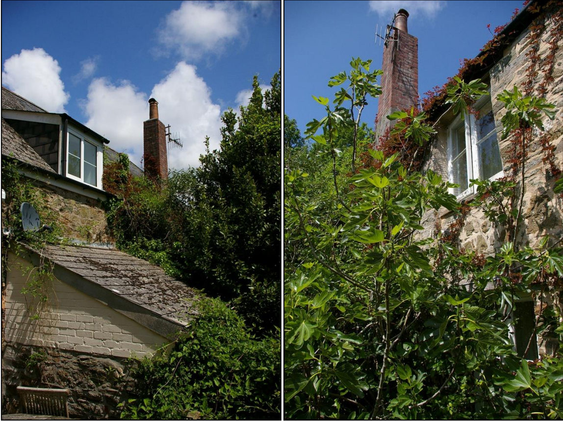
38. LEFT: VIEW BACK ALONG THE REAR OF THE FARMHOUSE, SHOWING LOOSE POST MEDIEVAL RUBBLE AT THE EAVES AND A REBUILT BRICK CHIMNEY SHAFT, AS WELL AS A DISTINCT CHANGE IN ALIGNMENT ON THE ROOF; FROM THE WEST, SOUTH-WEST.
