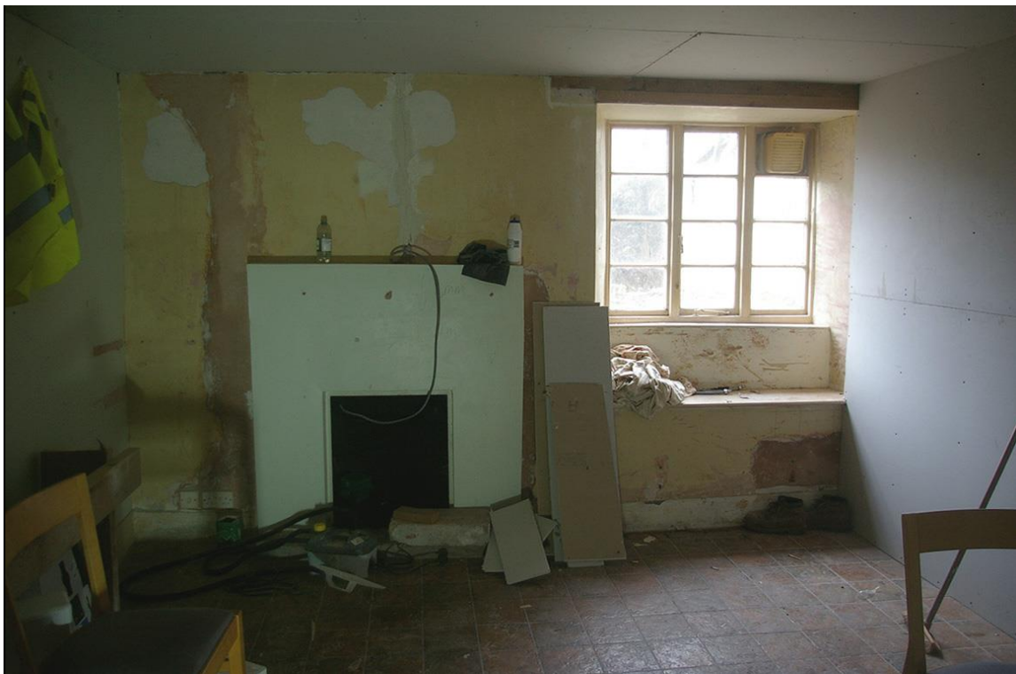
49. THE MODERNISED KITCHEN FIREPLACE AND GOOD 19 TH CENTURY WINDOW, ROOM 2B; FROM THE NORTH.
