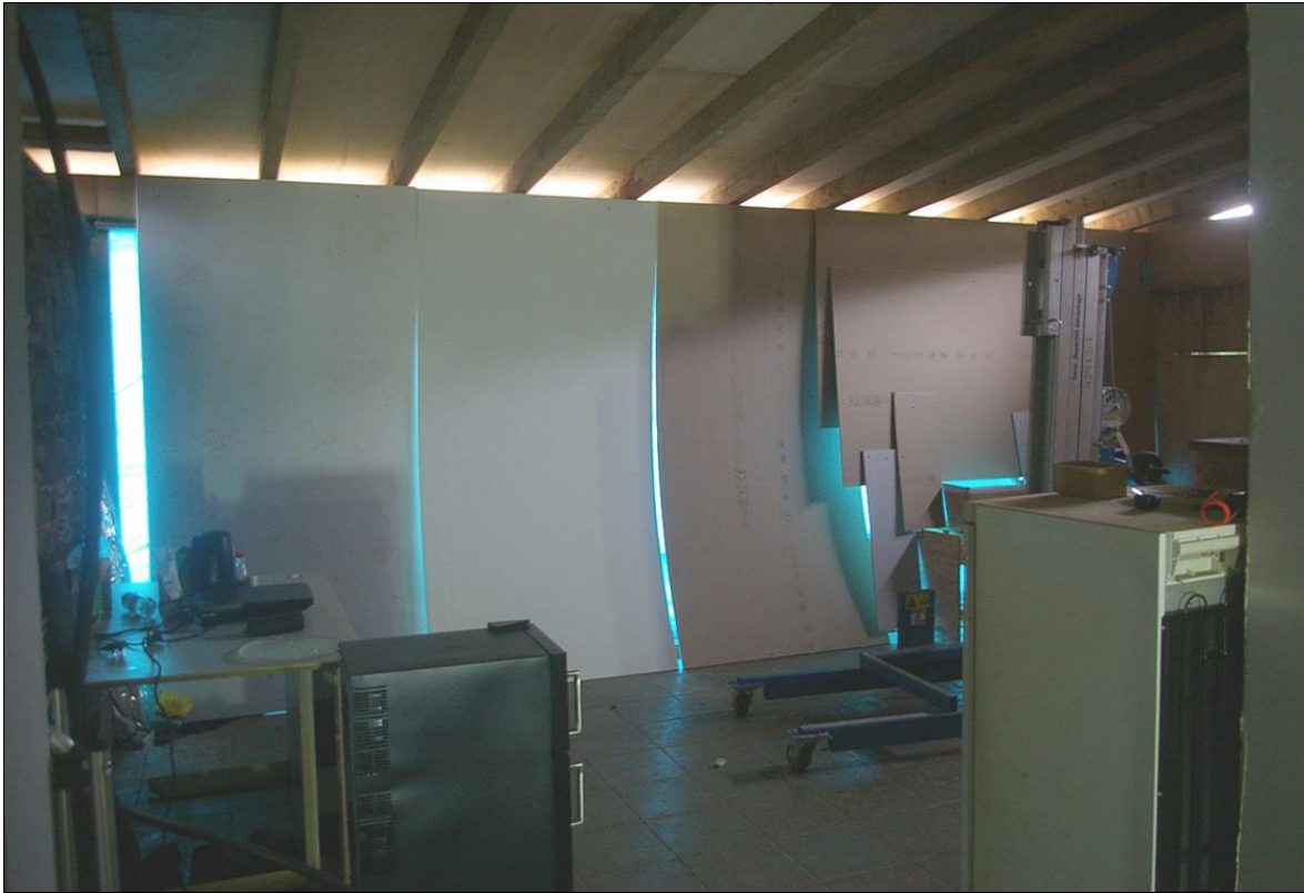
52. THE CONSERVATORY, WHICH HAS BEEN BOARDED OUT FOR SECURITY AND DUE TO PARTIAL COLLAPSE; FROM THE WEST-NORTH-WEST.
