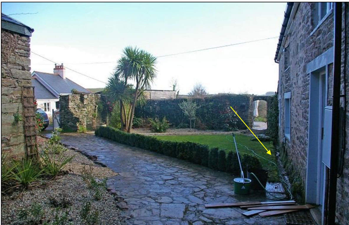
FIGURE 13: THE COURTYARD TO THE NORTH OF THE HOUSE FORMED BY THE VARIOUS MEDIEVAL RUINED WALLS, SHOWING 20 TH CENTURY CONCRETE-LINED GULLY, EXCAVATED AGAINST THE WALL OF THE HOUSE DUE TO GROUND LEVEL INCREASES, WITHIN THIS SPACE; PHOTO APRIL 2022.
