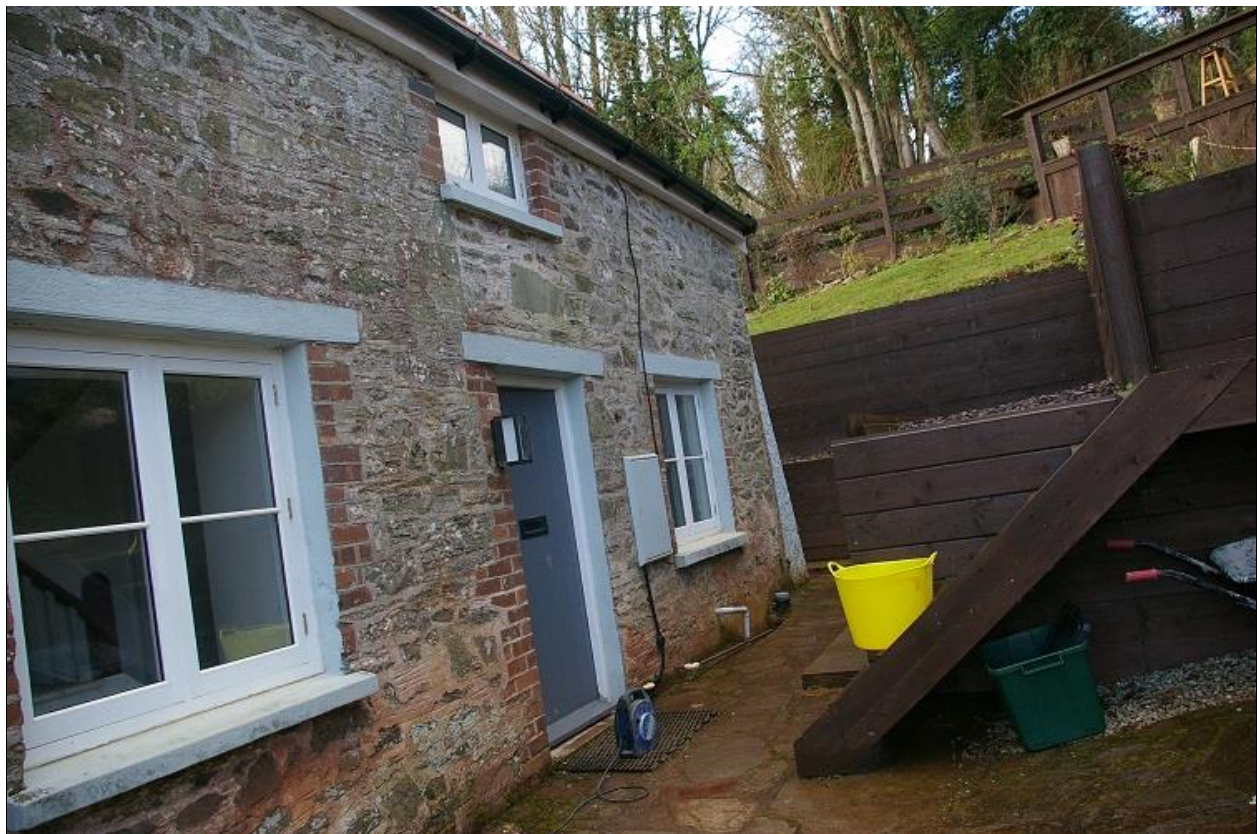
62. THE NORTH ELEVATION OF THE COTTAGE AND RETAINED WALLS OF PLANKS AND STEEL GIRDERS.
