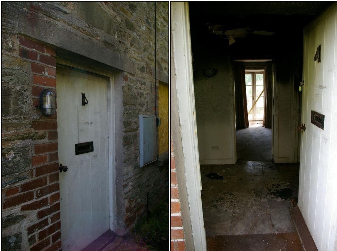
14. LEFT: THE FRONT DOOR TO THE COTTAGE, BRICK PATCHED REVEALS TO THE EAST, CONCRETE RENDER PATCHING TO THE WEST AND RENDERED LINTEL; FROM THE NORTH-EAST.
