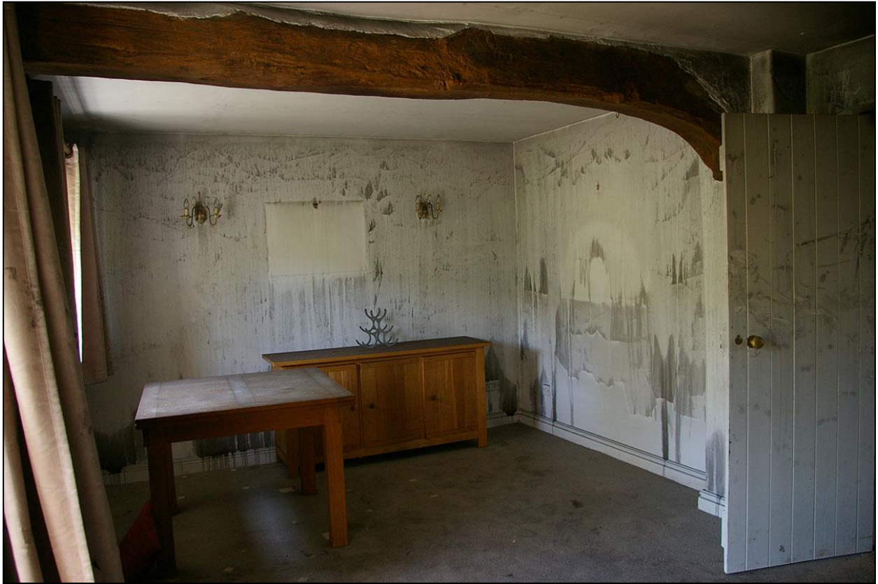
23. THE BEAM IN MORE DETAIL, BRACING A FORMER PARTITION LINE/WALL LINE; FROM THE SOUTH-EAST.
