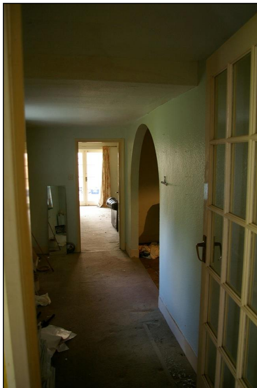
10. VIEW FROM THE HALLWAY INTO THE LOBBY/CORRIDOR CREATED BY ANOTHER MODERN PARTITION AND ARCHWAY, FORMING A FITTED KITCHEN, ALSO SHOWING FURTHER MODERN GLAZED DOORS AND MODERN FITTINGS; FROM THE WEST.
