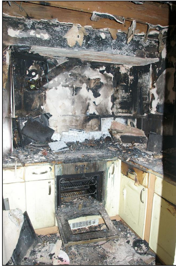
21. THE RUINED KITCHEN, CR2; FROM THE EAST.
