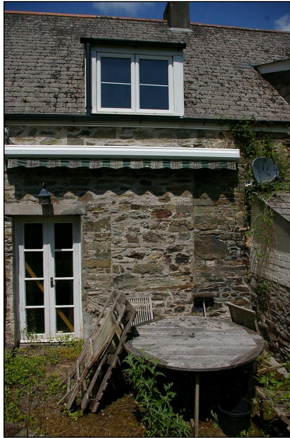
36. THE BLOCKED DOORWAY IN THE SOUTH ELEVATION OF THE COTTAGE IN THE SOUTH-EAST CORNER, SHOWING GOOD DRESSED REVEALS; FROM THE SOUTH.
