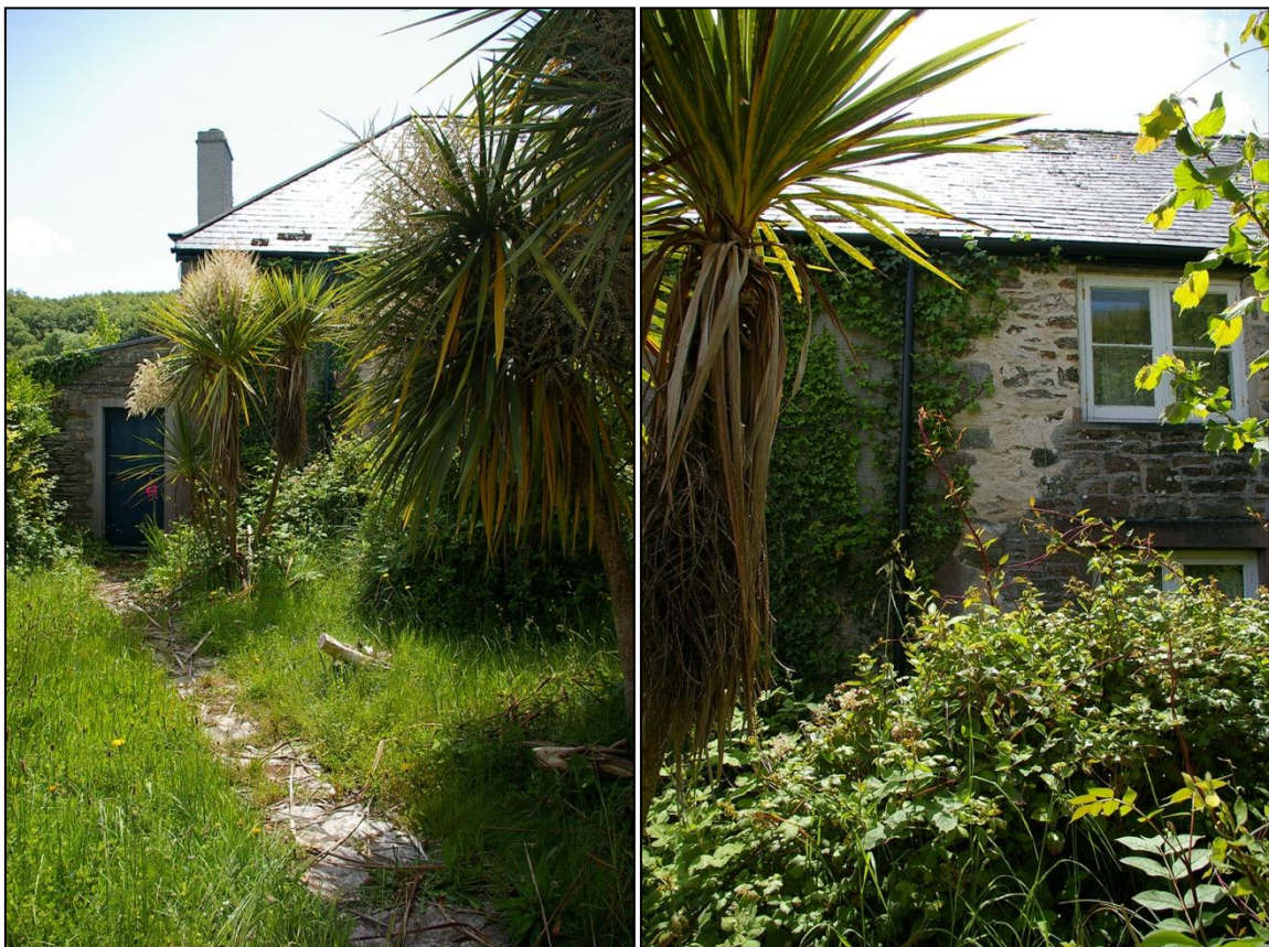
4. LEFT: THE LEAN-TO WITH AN OLD SECTION OF WALLING WHICH THE CONSERVATORY ABUTS FROM THE SOUTH SIDE; FROM THE NORTH, NORTH-WEST. RIGHT: THE RENDERED NORTH-EAST CORNER OF BATSON HALL FARM AND THE BADLY REPOINTED STONERWORK WHICH PARTLY OBSCURES A SET OF QUOINS, AT LEAST 1M INTO THE NORTH ELEVATION; FROM THE NORTH.
