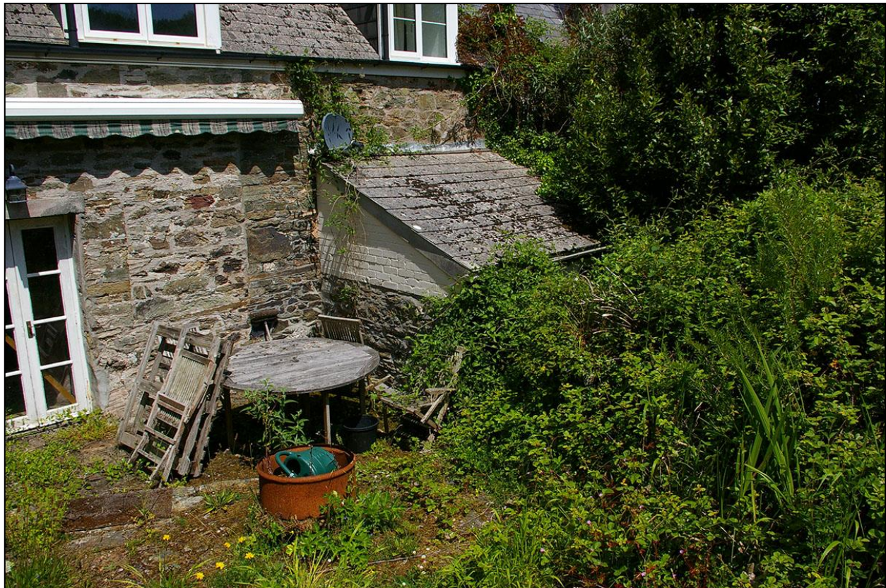
37. THE PROJECTING BLOCK, OF AN OLDER FORM OF PLATEY STONWORK, OFF THE BACK OF THE SOUTH ELEVATION ACROSS THE JOIN BETWEEN COTTAGE AND FARMHOUSE; FROM THE SOUTH-WEST.
