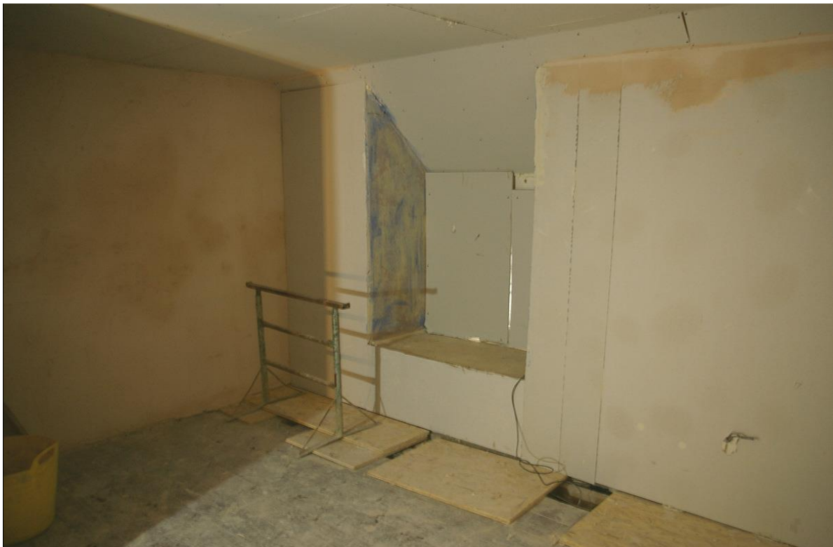
58. THE WINDOW WITHIN THE EXTENDED SECTION OF FRONT NORTH WALL, LEADING TO THE GABLE, OF THICK FULL TWO STOREY HEIGHT.
