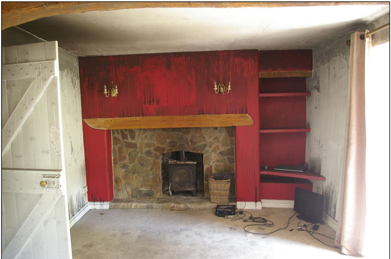
26. THE SHALLOW STACK AND BLOCKED FIREPLACE, WITH ALCOVE TO THE SOUTH, WITH TIMBER LINTEL; FROM THE WEST.
