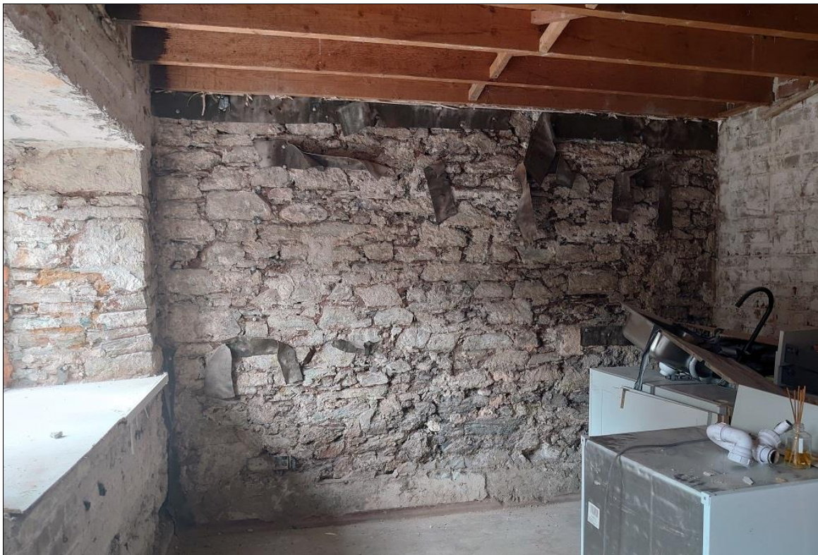
80. HEAVY MEDIEVAL WALLING TO THE WEST END GABLE OF THE COTTAGE, WITH FINE DRESSED DETAILS, ANOTHER FRAGMENT OF THE EARLIER COMPLEX; FROM THE EAST.
