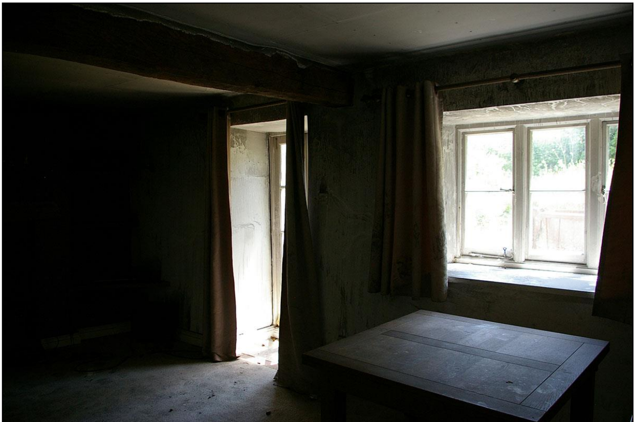
24. THE SOUTH WALL OF CR3, WITH FORCED PATIO DOORS AND 19 TH CENTURY WINDOW; FROM THE NORTH-EAST.
