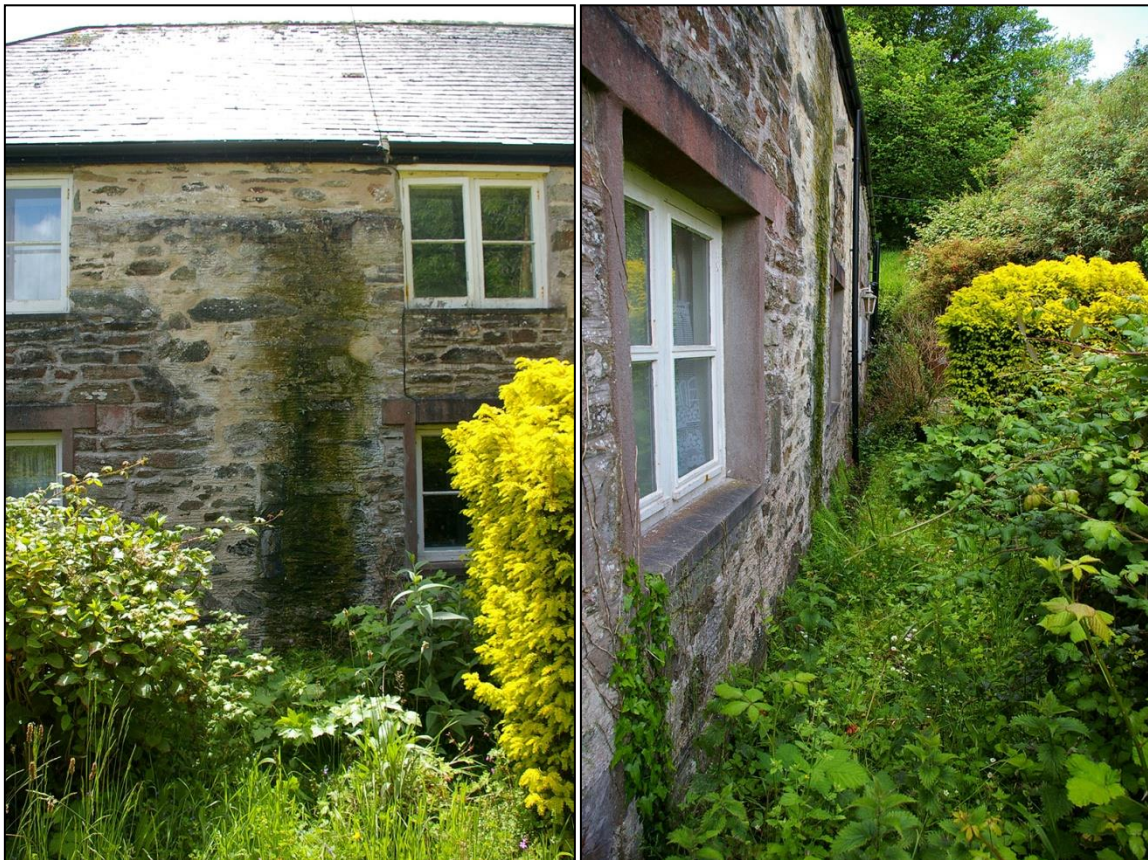
6. LEFT: DETAIL WITHIN THE RUINED WALL INCORPORATED INTO THE BUILDING SHOWING A POTENTIAL SET OF RAGGED LARGE SLAB QUOINS AND ALSO A POTENTIAL BLOCKED OPENING AT GROUND FLOOR; FROM THE NORTH. RIGHT: VIEW ALONG THE FRONT OF THE BUILDING, SHOWING HOW THE RUINED SECTION OF WALL IS ANGLING OUTWARDS QUITE CONSIDERABLY AND HOW THE ALIGNMENT OF THE RANGE CHANGES; FROM THE EAST.
