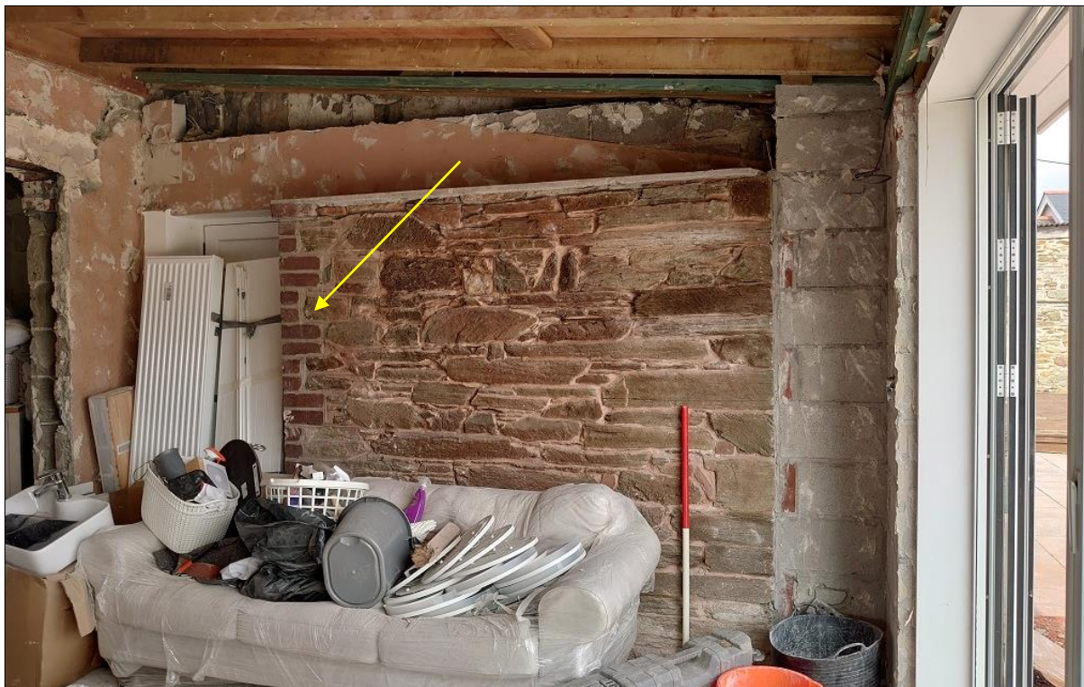
FIGURE 12: THE FRAGMENT OF MEDIEVAL WALLING WITHIN THE CONSERVATORY; 20 TH CENTURY BRICK REBUILT REVEALS TO FORCED DOORWAY ARE INDICATED (1M SCALE); FROM THE SOUTH-SOUTH-EAST.
