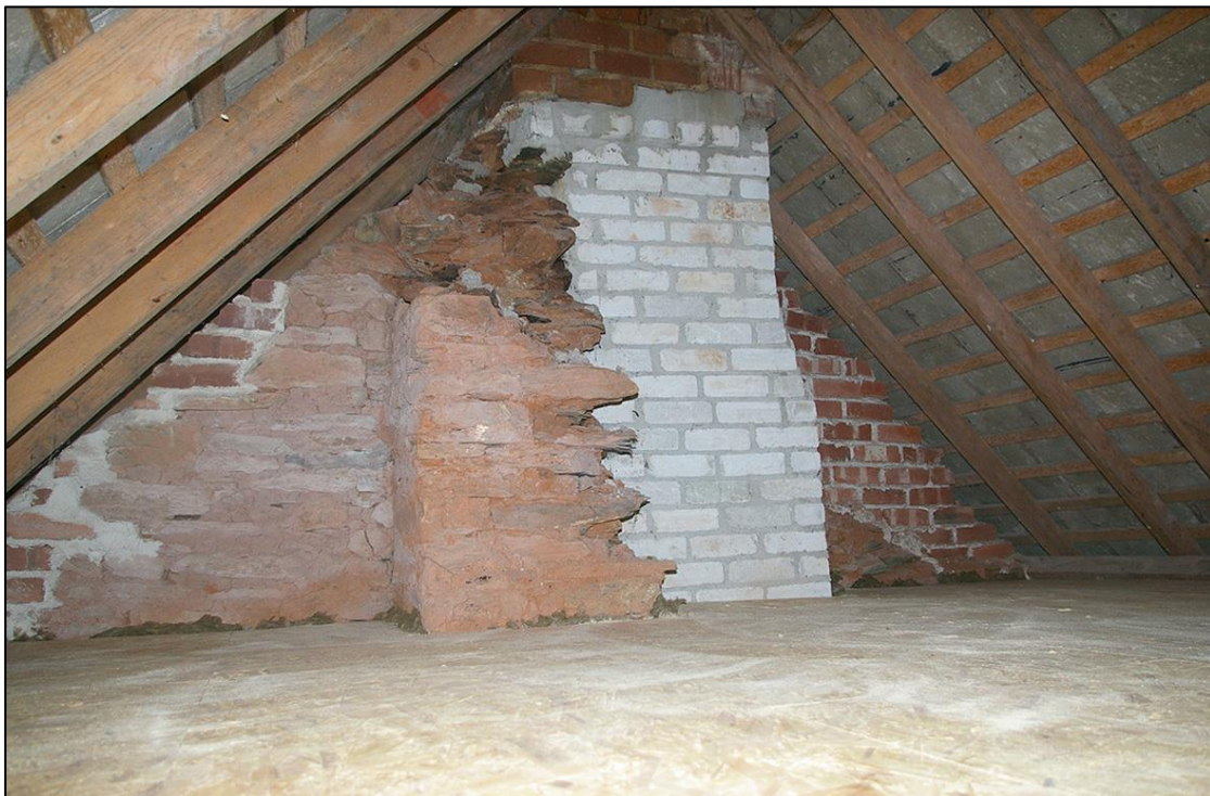
60. THE STACK TO THE WEST END OF BATSON HALL FARM; WITH FRAGMENTARY REMAINS RISING TO ONE AND A HALF STOREYS, THE STONWORK PATCHED IN BRICKWORK IN LIME MORTAR, THEN IN LATER BRICKWORK IN CEMENT AND IN CONCRETE BLOCK, INDICATING 19 TH AND SEVERAL PHASES OF 20 TH CENTURY REMODELLING.
