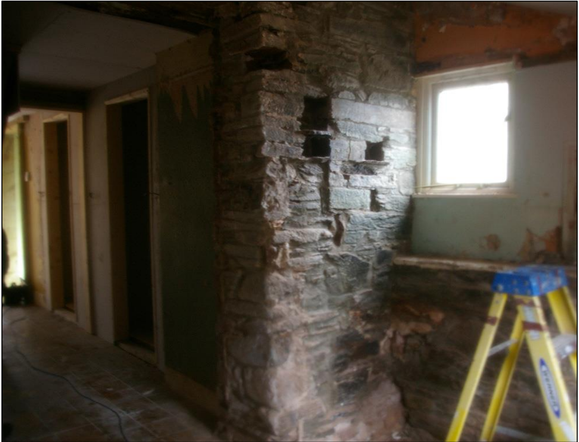
FIGURE 6: THE SHORT LENGTH OF GOOD DRESSED AND FACED MEDIEVAL STONEMWORK, WITH ABUTTING HEAVY SLATESTONE RUBBLE AROUND OPENING AND PUTLOG HOLES, REWORKED AS DOVE HOLES, WITHIN THE PROJECTION ON THE SOUTH ELEVATION OF THE FARMHOUSE, NOW ENCLOSED WITHIN THE OUTSHUT; FROM THE SOUTH-WEST.
