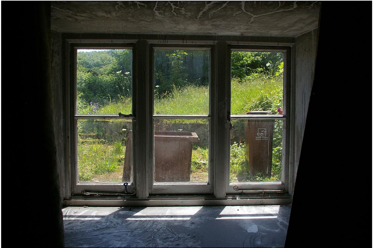
25. DETAIL OF THE GOOD 19 TH CENTURY THREE LIGHT CASEMENT WINDOW CW3; FROM THE NORTH.
