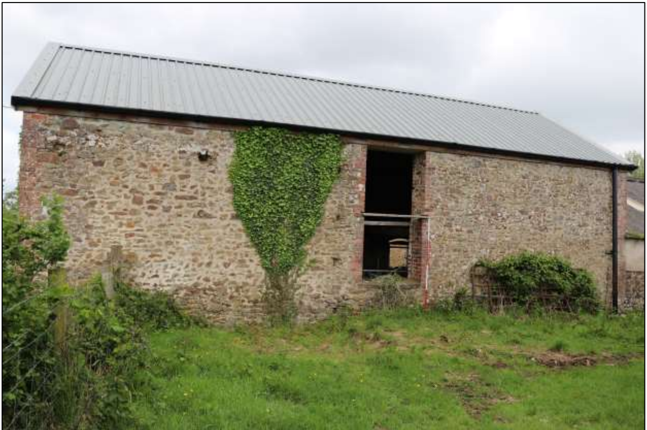
FIGURE 15: THE EAST ELEVATION OF THE BARN WITH DOUBLE-HEIGHT OPENING, AND SCARRING FOR A LOST LEAN-TO; VIEWED FROM THE ESE (SCALE 2M).
