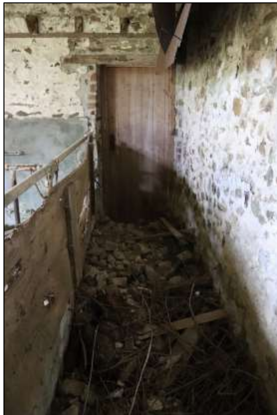
RIGHT FIGURE 22: VIEW ALONG THE FEED PASSAGE LEADING TO A PLANKED TIMBER DOOR WITH THUMB LATCH IN A PEGGED FRAME; VIEWED FROM THE SOUTH.
