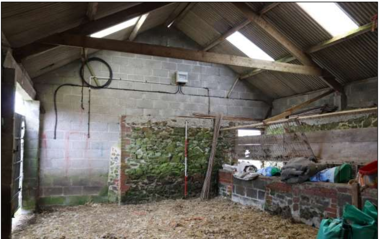
FIGURE 24: THE INTERIOR OF THE EXTENSION, SHOWING HOW IT INCORPORATES THE EARLIER WALL; VIEWED FROM THE SOUTH-WEST (SCALE 2M).
