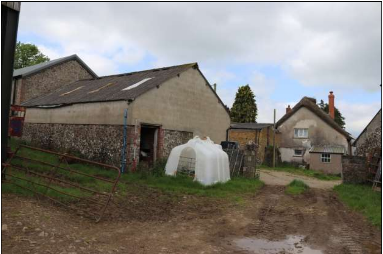
FIGURE 13: THE NORTH AND EAST ELEVATIONS OF THE EXTENSION, LOOKING BACK TOWARD HOUSE FROM THE ADJACENT FIELD; VIEWED FROM THE NNE (SCALE 2M).
