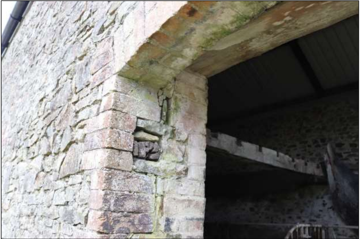
FIGURE 16: THE ORIGINAL DOORWAY TO THE BARN. BRICK DRESSINGS AND TIMBER SOCKETS FOR A DOOR FRAME THAT NO LONGER SURVIVES; VIEWED SOUTH-WEST.
