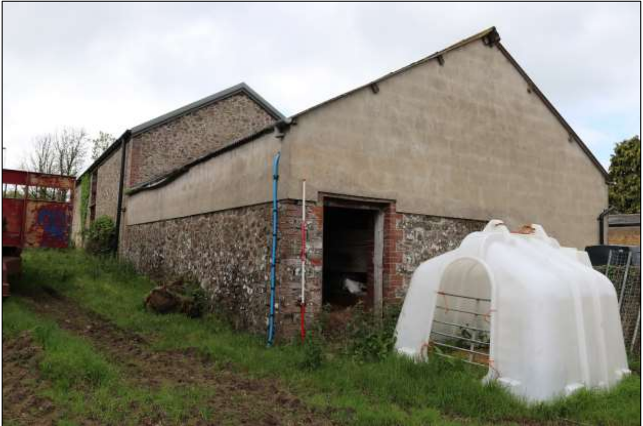
FIGURE 12: THE NORTH AND EAST ELEVATIONS OF THE EXTENSION; VIEWED FROM THE NORTH-EAST (SCALE 2M).
