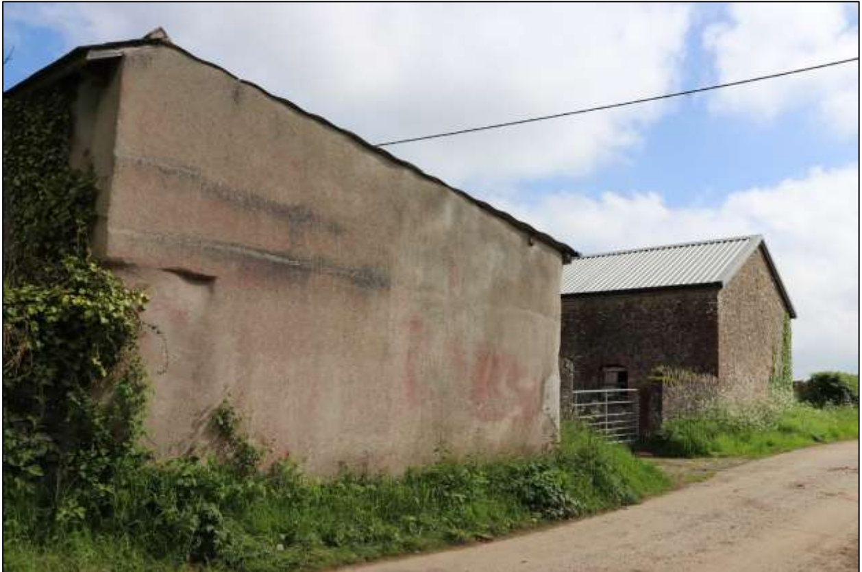
FIGURE 4: THE SOUTH ELEVATION OF THE BARN AND THE LINEAR COB RANGE TO THE WEST; VIEWED FROM THE SOUTH-WEST.
