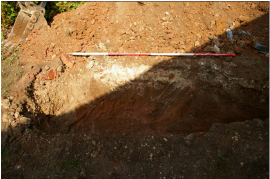
Figure 4: View of the east-facing section of the pipe trench showing context (101)(2m scale).
