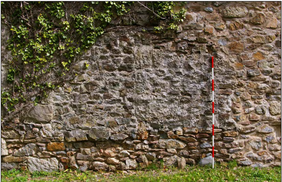
Figure 15: The north end of the west elevation showing phases of blocked openings, one with stone reveals.
