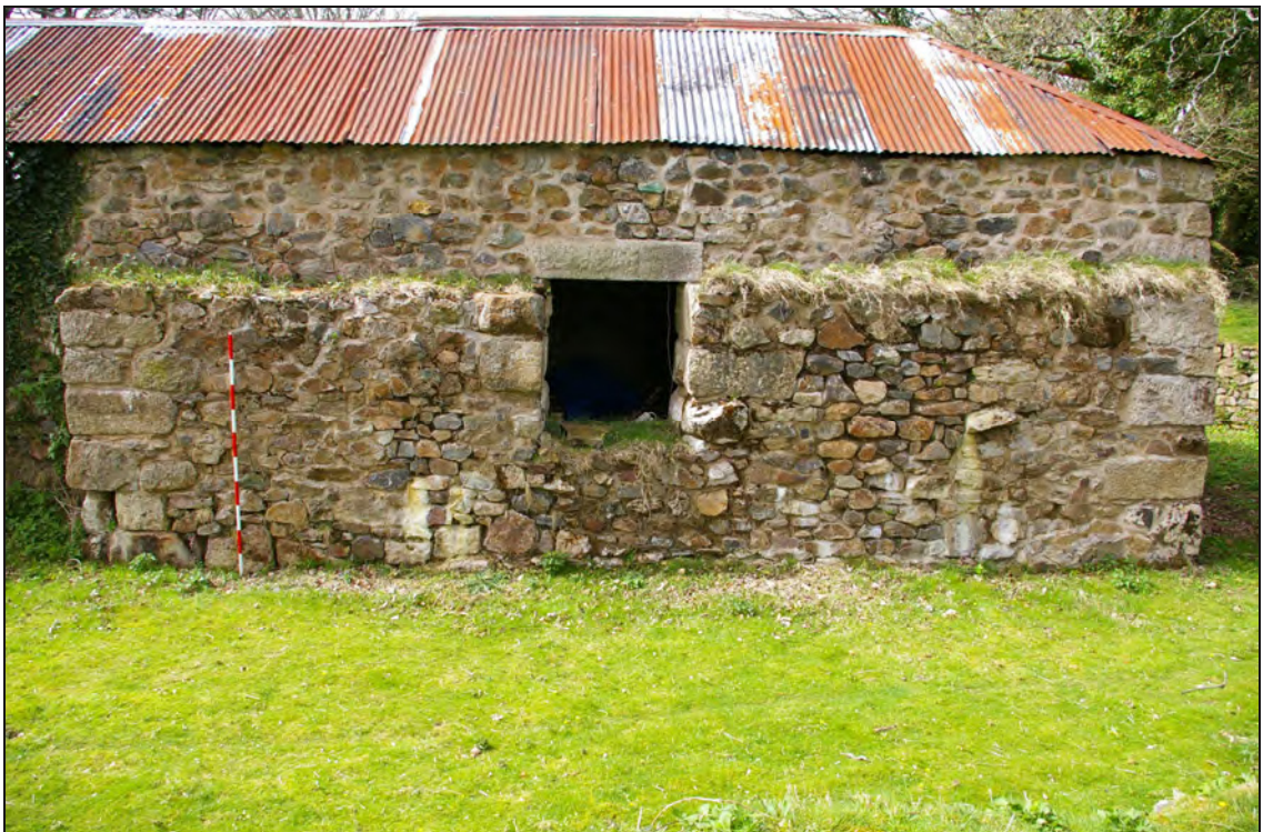
Figure 6: The northern end of the east elevation of the building, viewed from the east.
