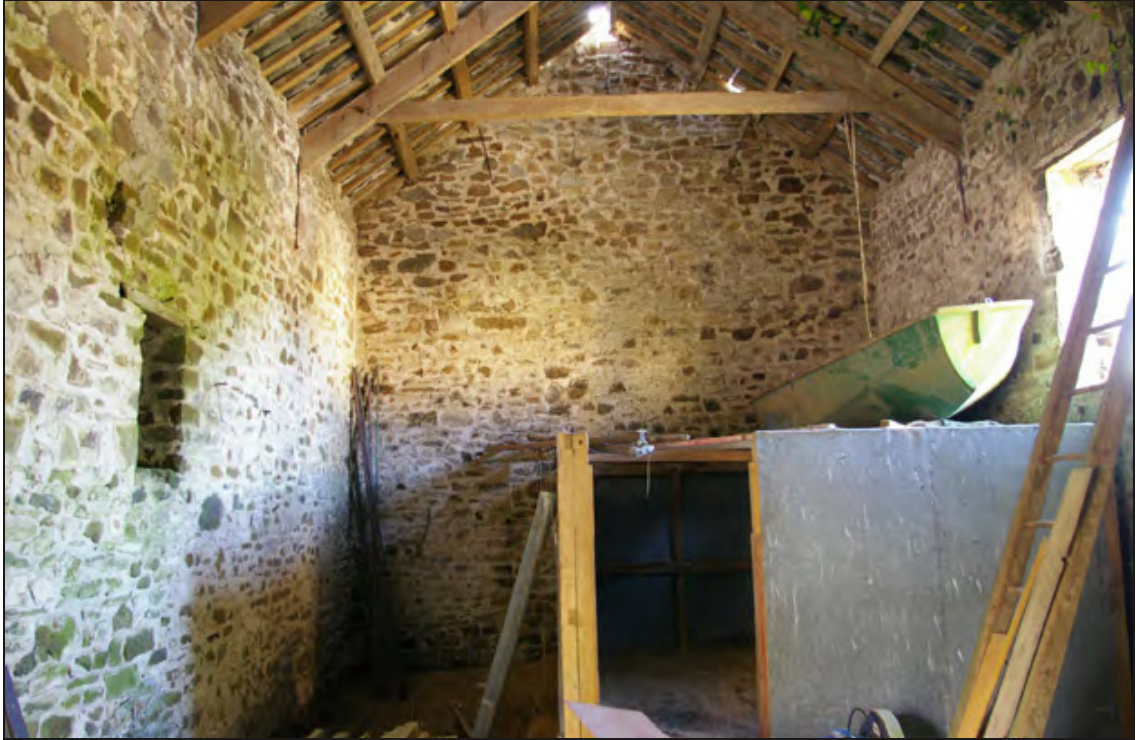
Figure 8: Interior view of the north wall of the threshing barn (B1), viewed from the south.
