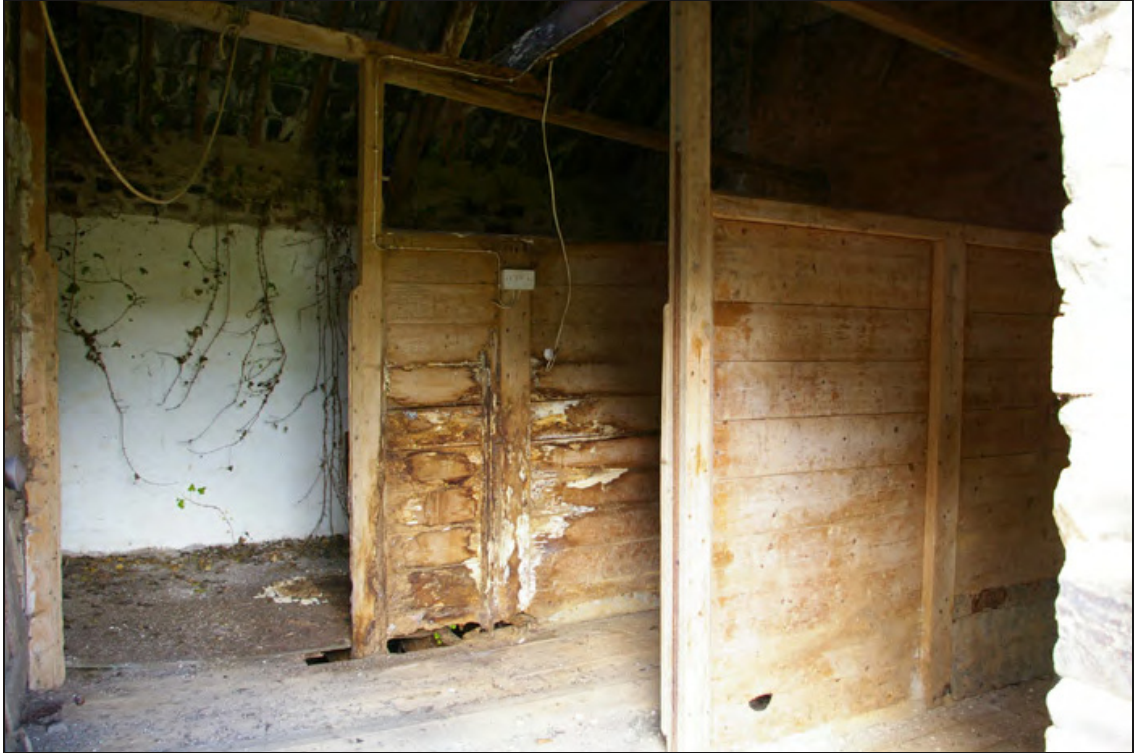
Figure 10: Interior view of the first floor of the granary (B1a), viewed from the south-east.
