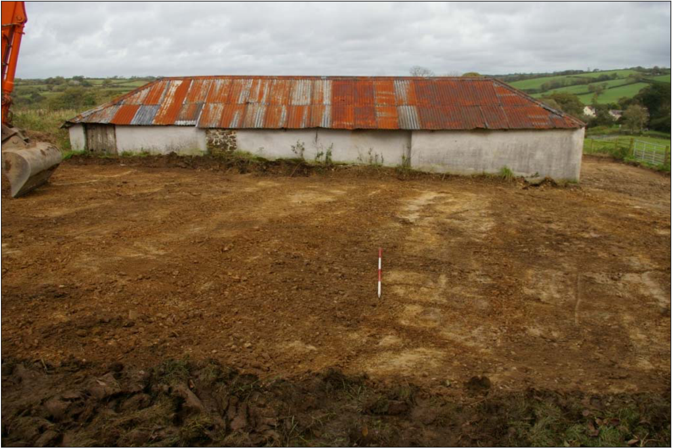
Figure 2: Area of excavation with the barns in the background, viewed from the west (scale 2m).
