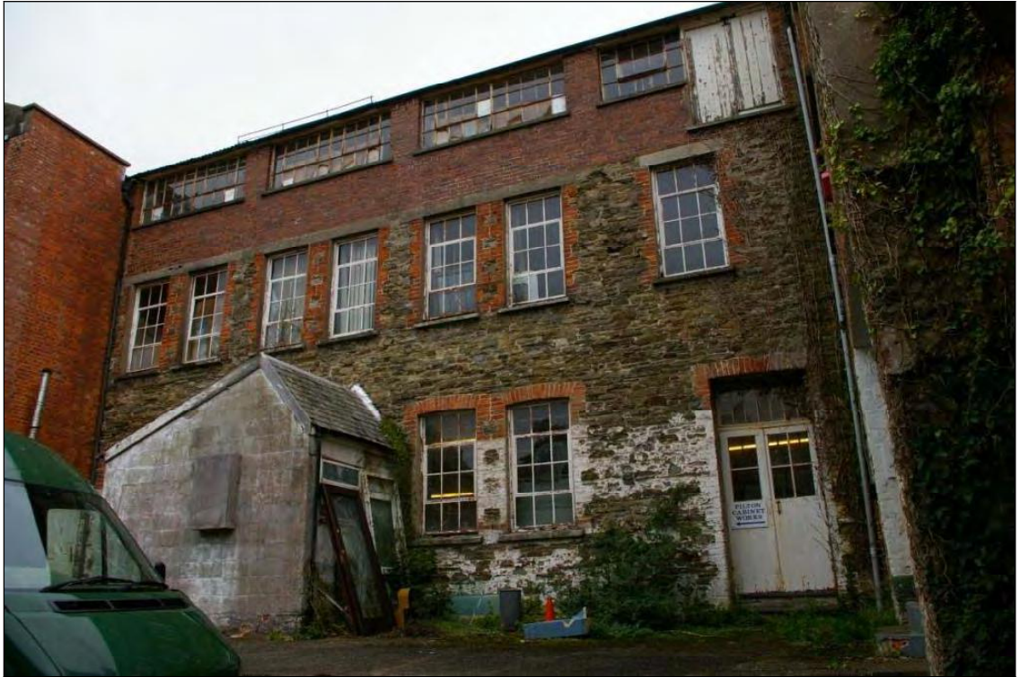
Figure 19: The west elevation of the east wing of the factory, viewed from the south-west.
