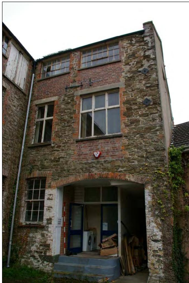
Figure 12: The north elevation of the south wing, with phases of blocked openings and the former entrance archway.
