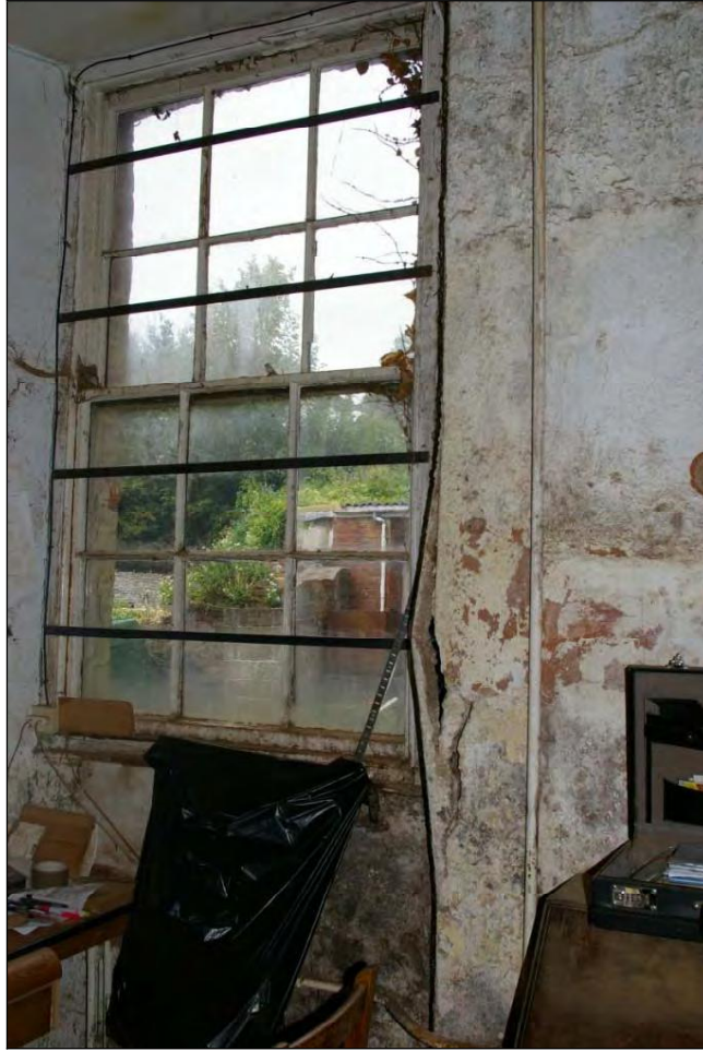
Figure 14: The hornless sash window in the north wall of the south wing, note the square top to this window, different from the others in this wing, viewed from the south-east.
