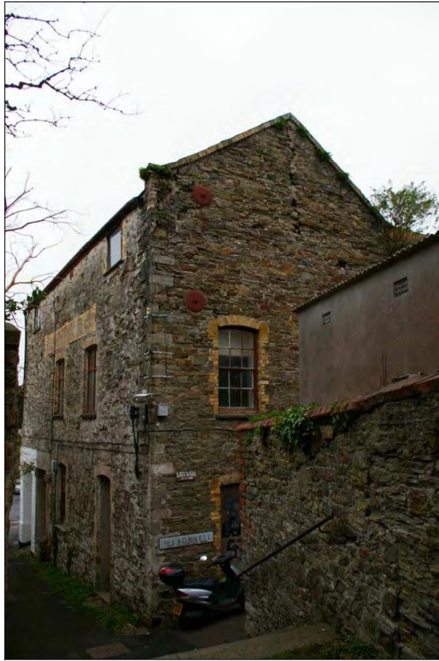
Figure 13: The south wing showing the yellow brick detailing and the raised gable, with the matching first floor hornless sash windows, viewed from the south-east.
