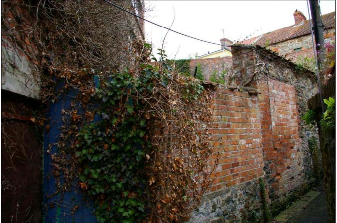
Figure 11: The stone wall of Ladywell Lane running along the length of the former north-east yards, showing the brick arches and blocked doorways into the former yards, viewed from the south-west.
