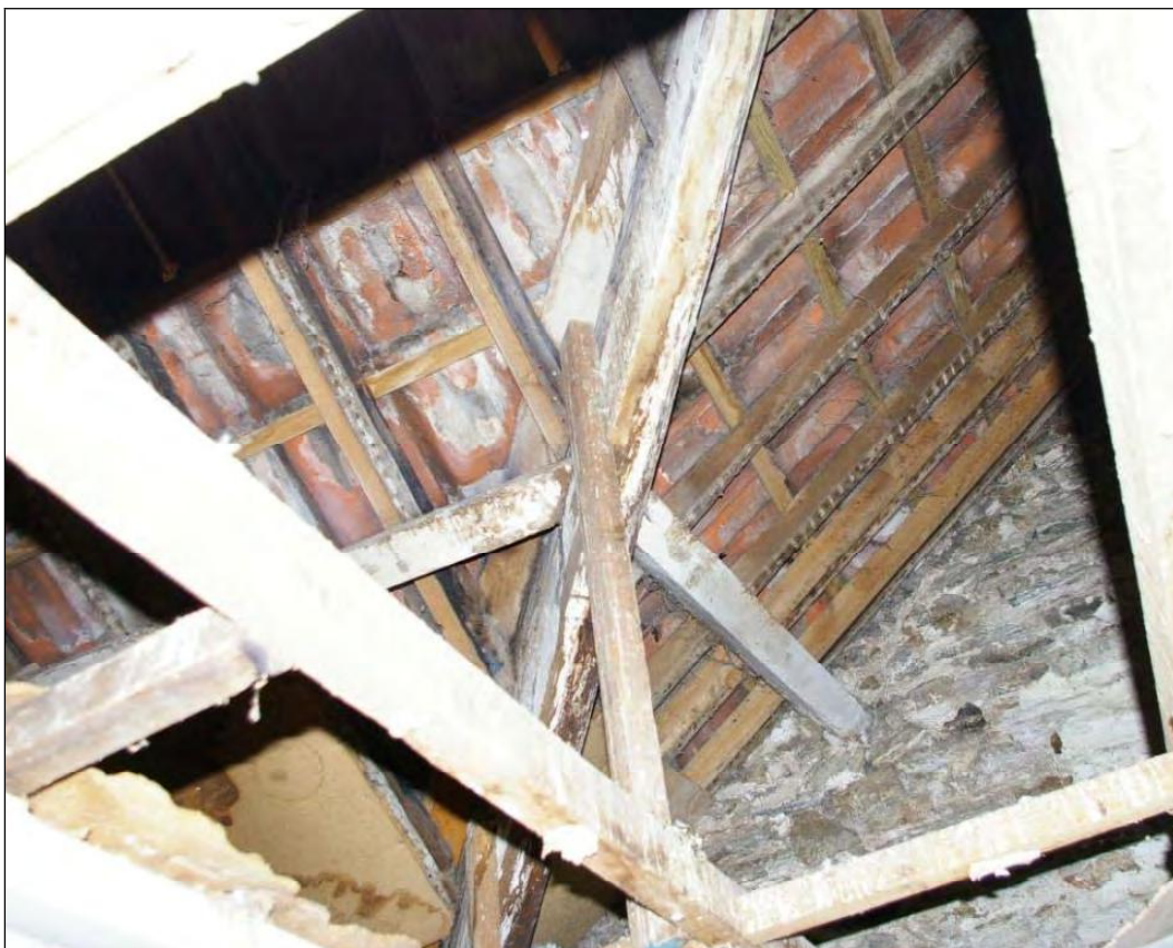
Figure 17: The roof structure over the south wing, showing the integration with the east wing roof and the marks of a former lathe and plaster ceiling to the rafters, viewed from below.
