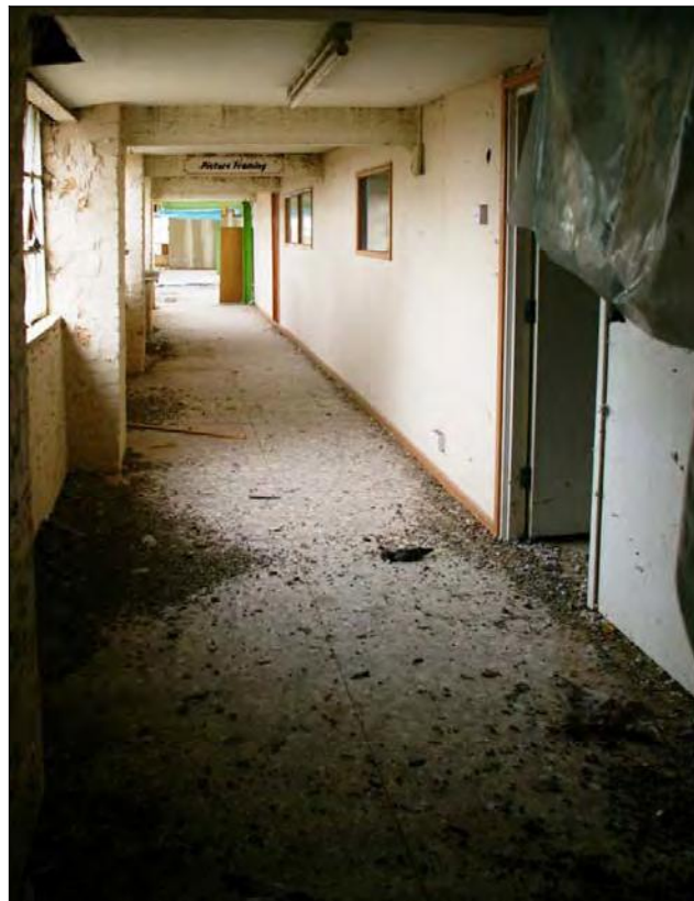
Figure 22: The second floor corridor to the west side of the east wing, viewed from the south.
