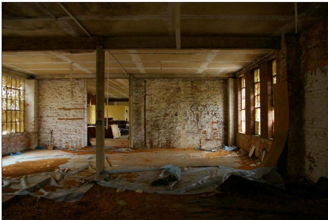
Figure 25: The former exterior north wall of the east wing, abutted to the west by the brickwork of the modern north wing, viewed from the north.
