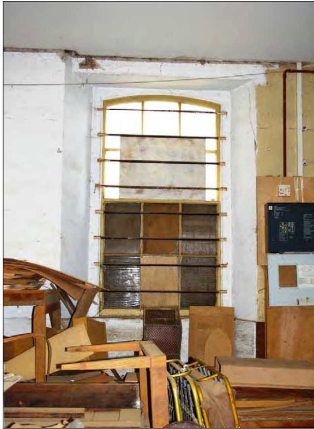
Figure 15: The sash window in the south wall of the south wing, showing the shallow arch to the top sash, viewed from the north.
