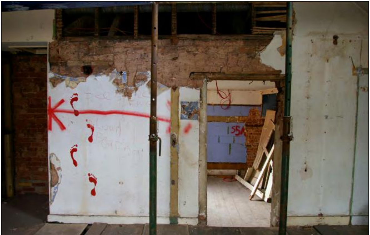
Figure 11: The south wall of Bedrooms 1 and 2, adjoining the Dressing Room, viewed from the north.
