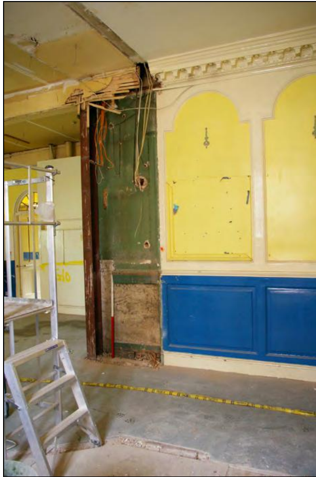
Figure 3: View of the south wall of the Entrance Hall adjacent to the stairs, viewed from the north-west.
