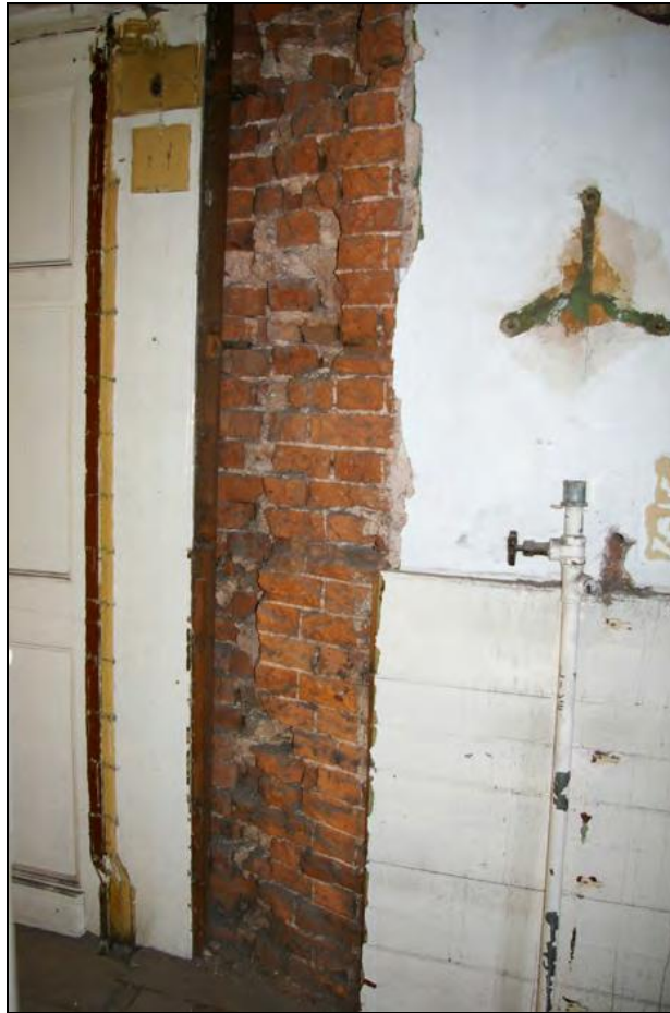
Figure 10: Brickwork exposed within the corridor from the second floor landing to the Dressing Room, north wall, viewed from the south-east.
