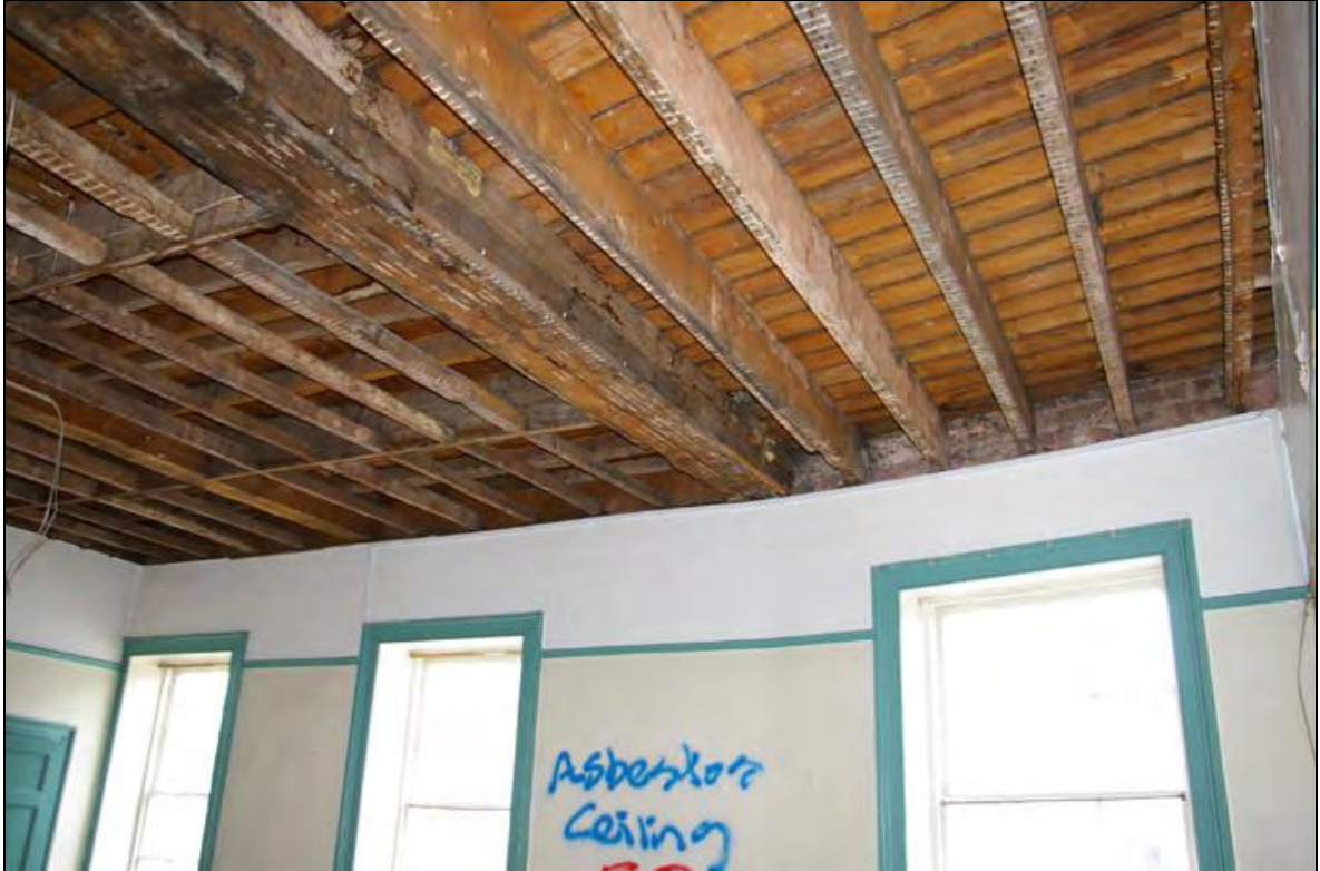
Figure 8: View of the removed ceiling of the Heavitree Room, showing exposed joists, floorboards and beams, viewed from the south-east corner of the room.
