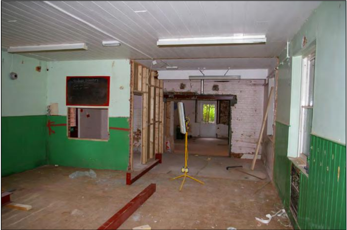
Figure 6: View to the Model Railway Room, showing the shortened Served area and the surviving 19 th century plank panelling to the north wall, viewed from the north-east.
