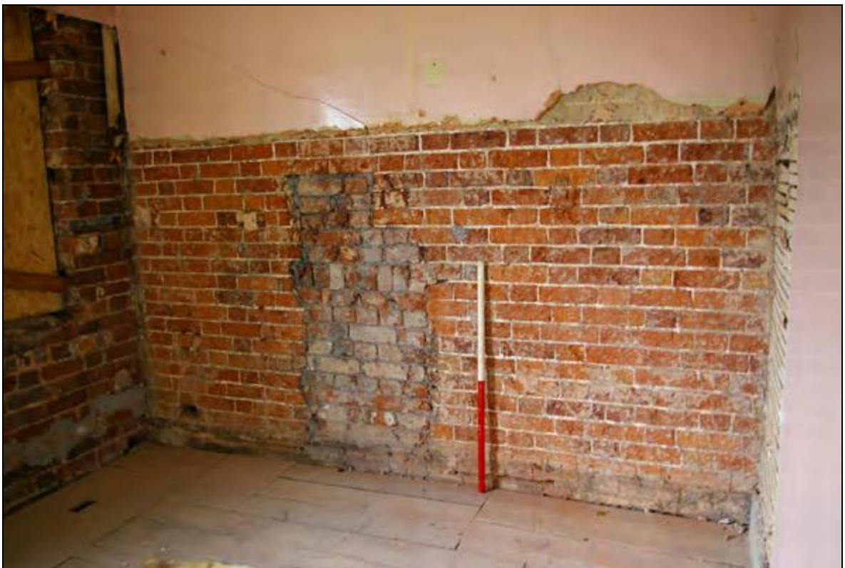
Figure 12: The north wall of the Bathroom, showing the position of the removed chimney stack from the blocked fireplace in the Dressing Room, viewed from the south.
