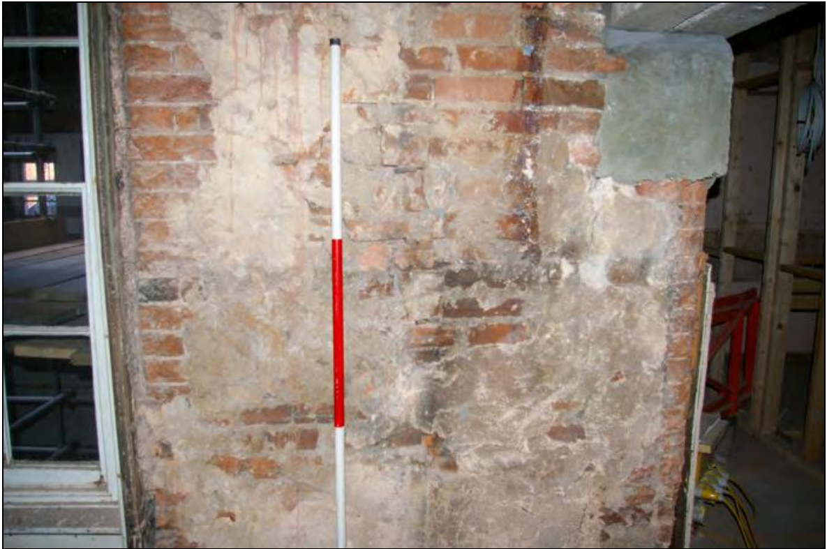
Figure 9: South wall of the first floor Hallway to the Pennsylvania Room, showing the join between the 1790-1820 phase and the sub-phase of 1760-1790, with some modern repairs, viewed from the north.
