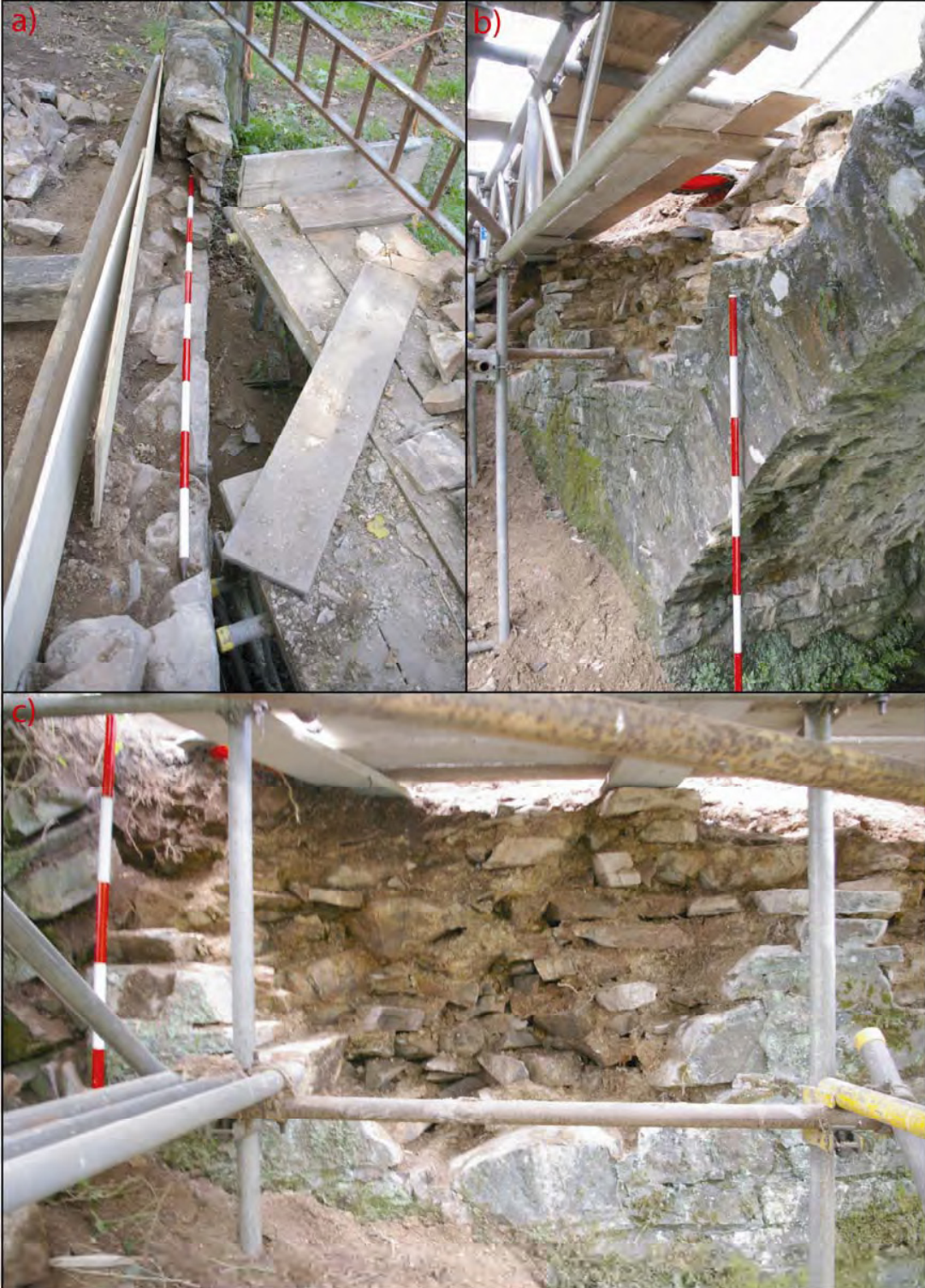
Figure 3: (a) The northern part of repairs to the eastern parapet, viewed from the south (2m scale). (b) The repairs to the southeast spandrel panel, viewed from the northeast (2m scale). (c) The southern end of repairs to the southeast spandrel panel, viewed from the east (2m scale).
