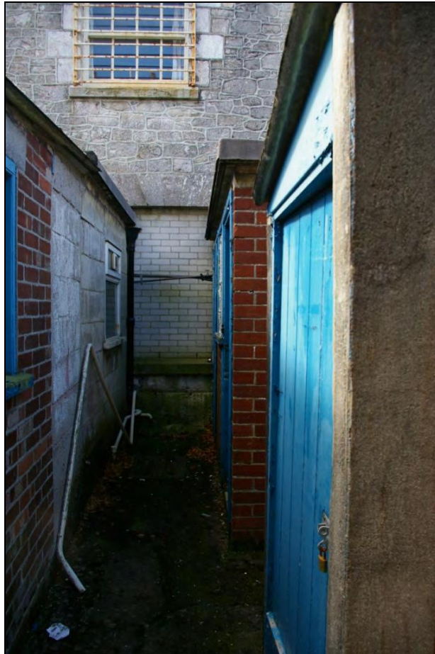
Figure 20: The east elevation of the West Pavilion, showing the blocked window opening overlooking the courtyard, viewed from the east.
