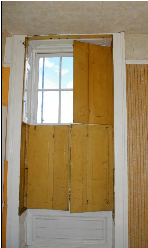
Figure 26: The south window in the east elevation of the East Pavilion, viewed from the west.
