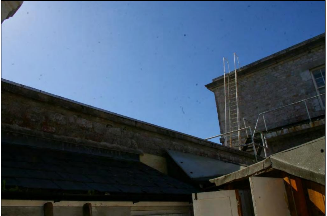
Figure 24: The Courtyard between the East Pavilion and Admiralty House, showing the south curtain wall and the passageway built up against it, viewed from the north-east.
