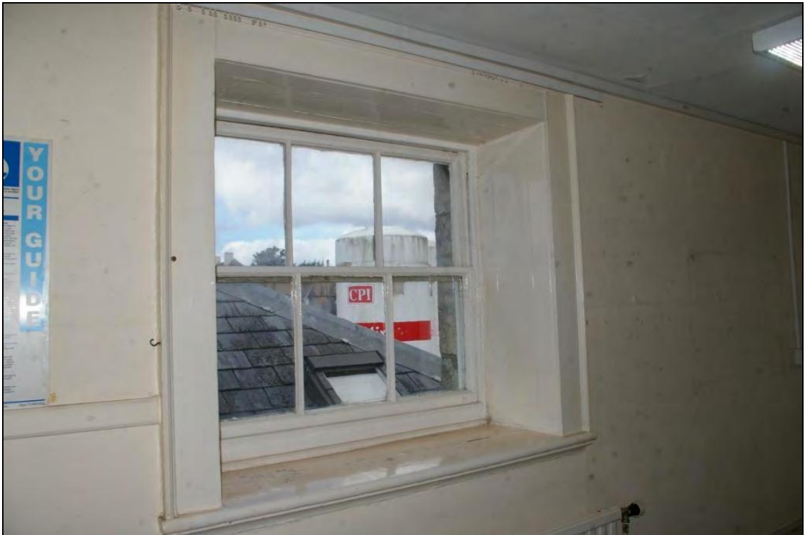
Figure 19: The large hornless sash window in the west wall of the West Pavilion, at first floor height, in a deep moulded architrave with painted shutters to either side, viewed from the south-east.
