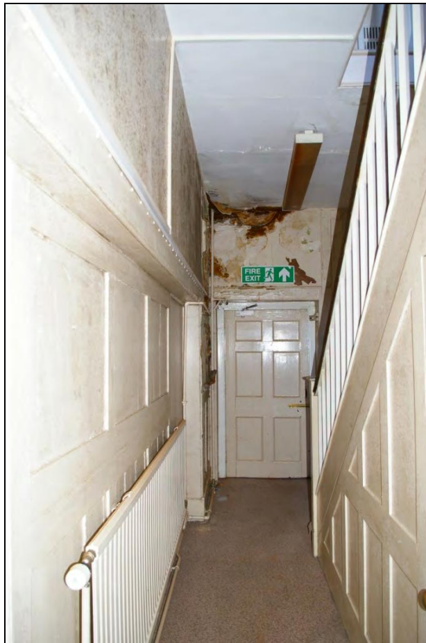
Figure 18: The stair hall in the centre of the West Pavilion, viewed from the west.
