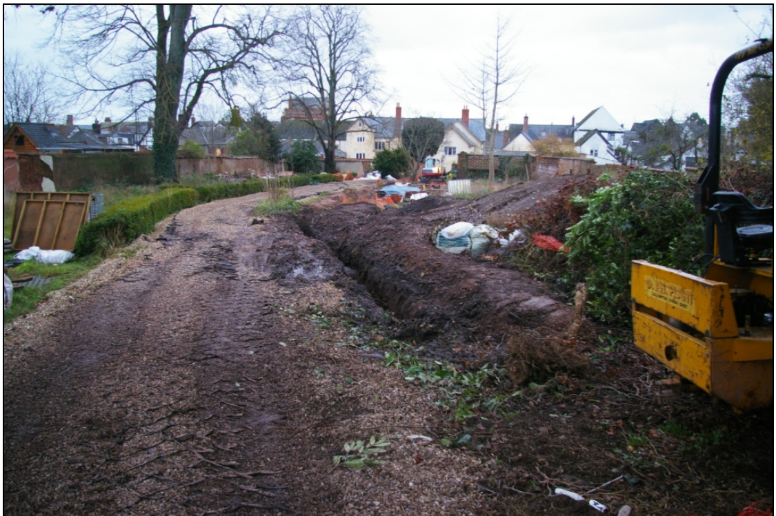
Figure 7: Service trench during excavation within the ‘Big Garden’, viewed from west (no scale).
