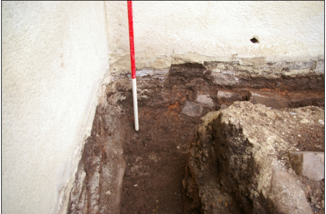
Figure 14: The footings of the Main Hall (to the right) and projecting Main Stair (to the left), viewed from west (2m scale).
