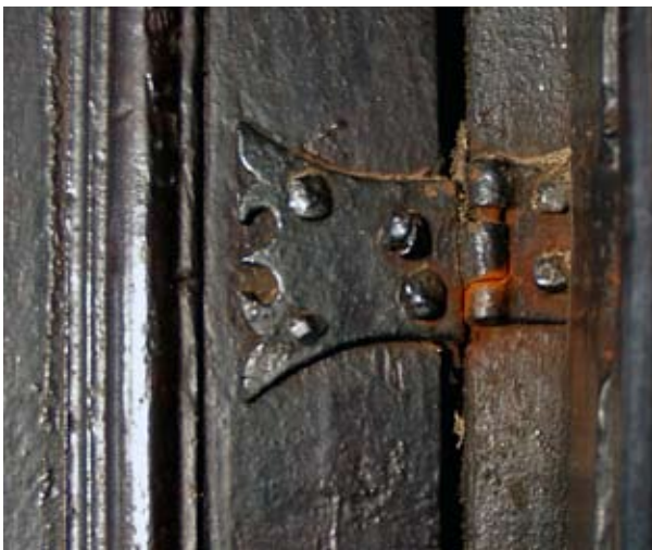
The upper hinge on the doorway from the parlour to the corridor; 09.06.2009.
