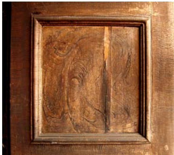
The grained walnut decoration shows through the Victorian varnish on one of the panels on the northern window shutter to the inserted east window, 01.07.2007.
