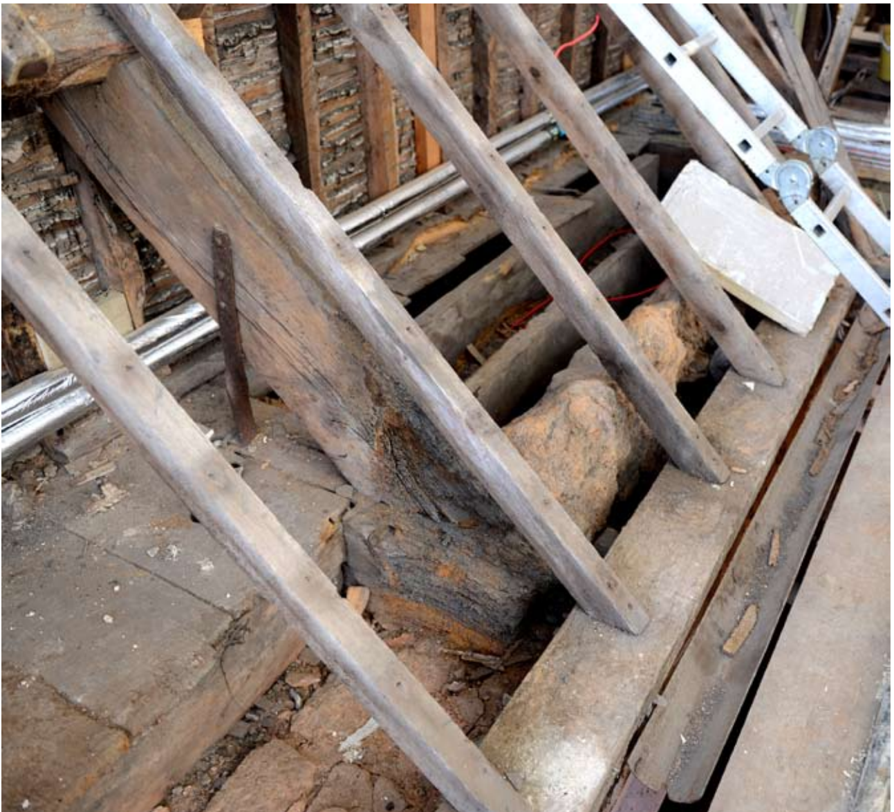
Detail of the north pitch of the south wing roof looking west at the base of the western truss. The common rafters and eaves plate date from 1890-1. Beyond the truss original cobbing up survives, 30.01.2013.
