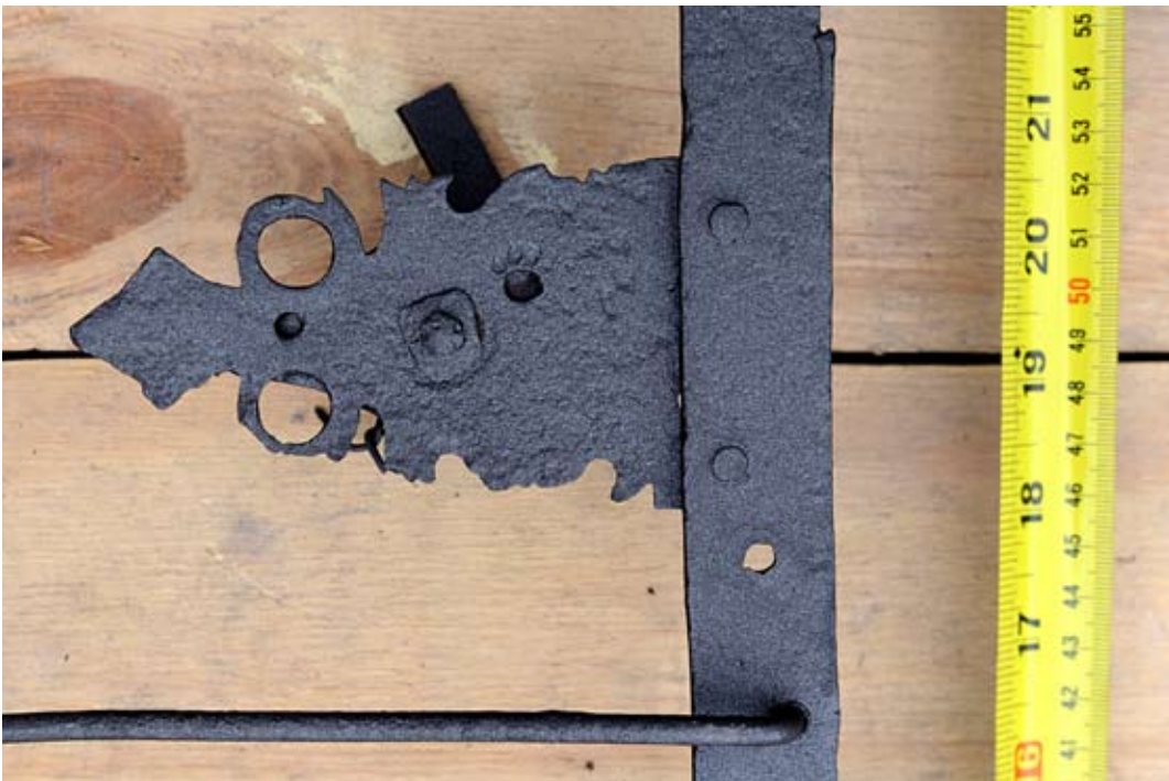
Inside and outside views of the c1605 wrought-iron catch in the east window casement (W.F. 04). The turnbuckle looks like an 1890-1 Burrow replacement. One can see the scar left from the removal of the original spring latch system. Photographed during repairs at the Brockwier Glass workshop, 20.05.2013.
