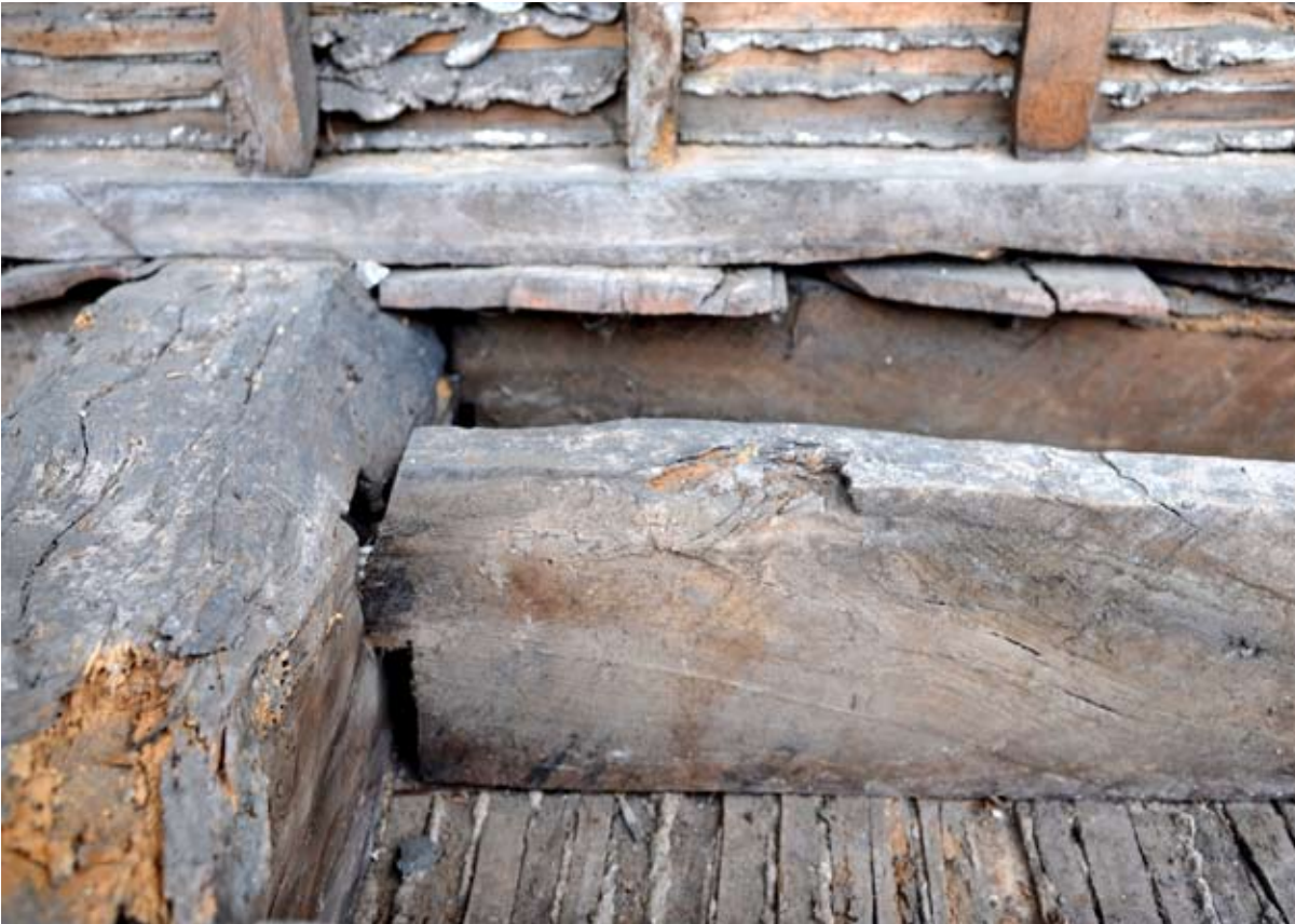
Detail of the arrangement of the joists and floorboards in the east bay on the south side, 16.11.2012.
