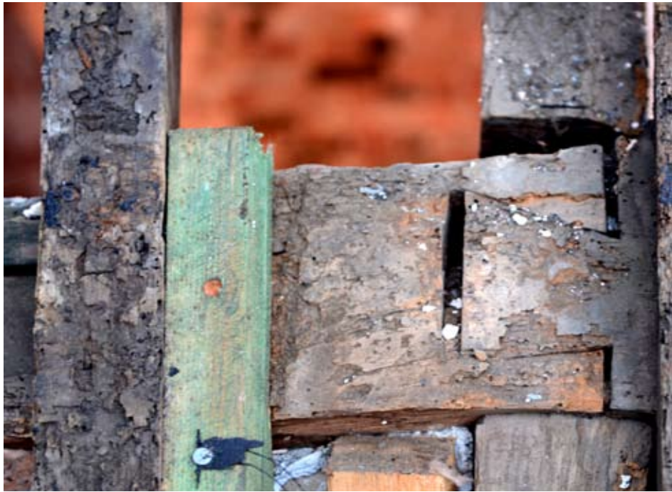
The joint between the two lengths of purlin on the back of the western truss on the north side, 16.11.2012.
