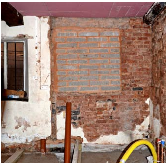
The south wall of the kitchen is faced up with reused 1890-1 brick. In 2012-13 window W.G. 20 was taken out and the opening blocked up, 30.01.2013.
