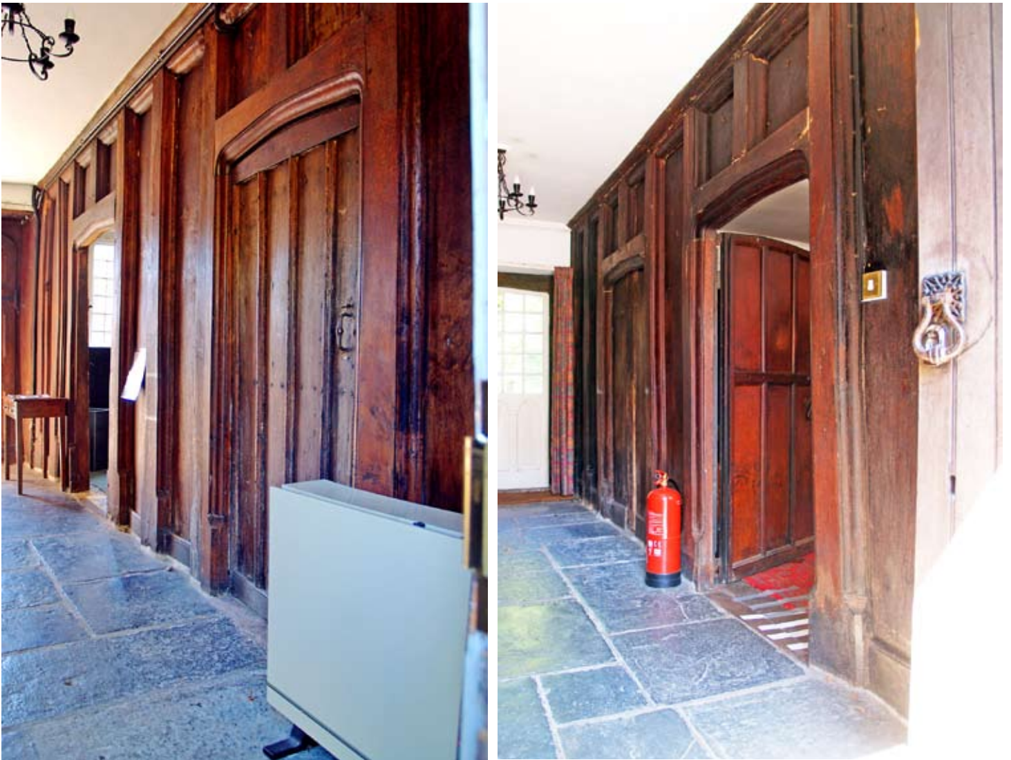
The oak screens lining the cross passage. The southern screen (to left) is on the service side with doorways off to the Justice Room and Kitchen Lobby. The northern screen (to right) had two doorways into the Hall, both 02.06.2009.
