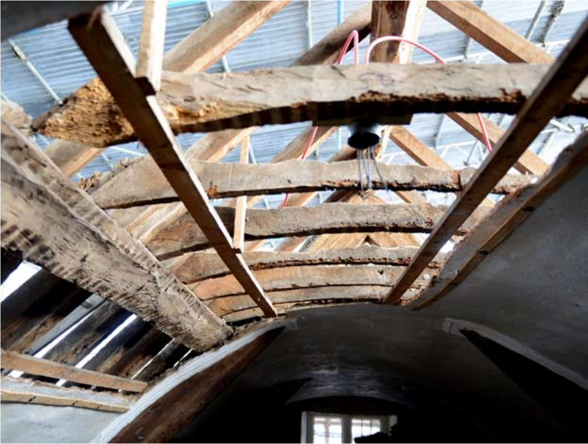
Plaster repairs showing the construction of the coved ceiling in the south wing, 30.01.2013.
