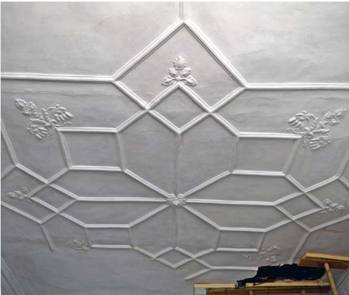
The ornamental plaster ceiling awaiting repair, 17.10.2012.
