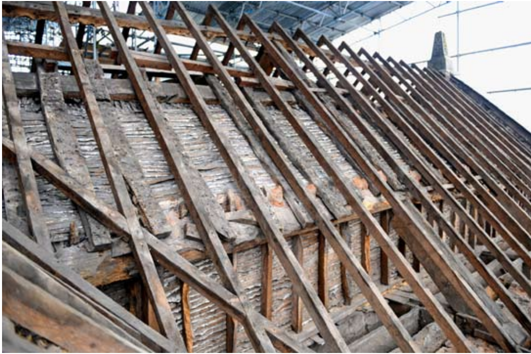
The southern pitch of the south wing roof looking east. The working common rafters are replacements from 1890-1 but the original were preserved between the purlins since the laths of the c1605 ceiling are nailed to them, 16.11.2012.
