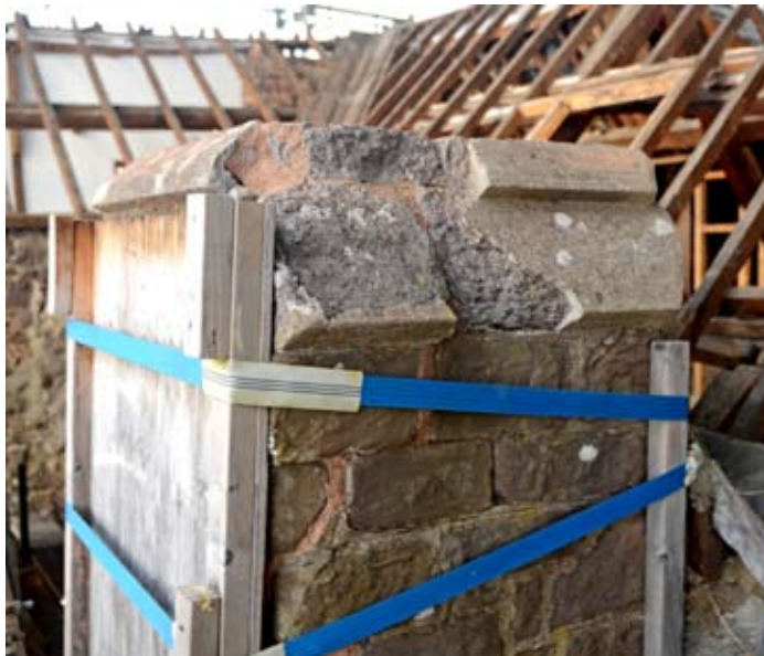
Detail of the top of the hall chimneystack and base of the shaft before repairs, 29.10.2012.
