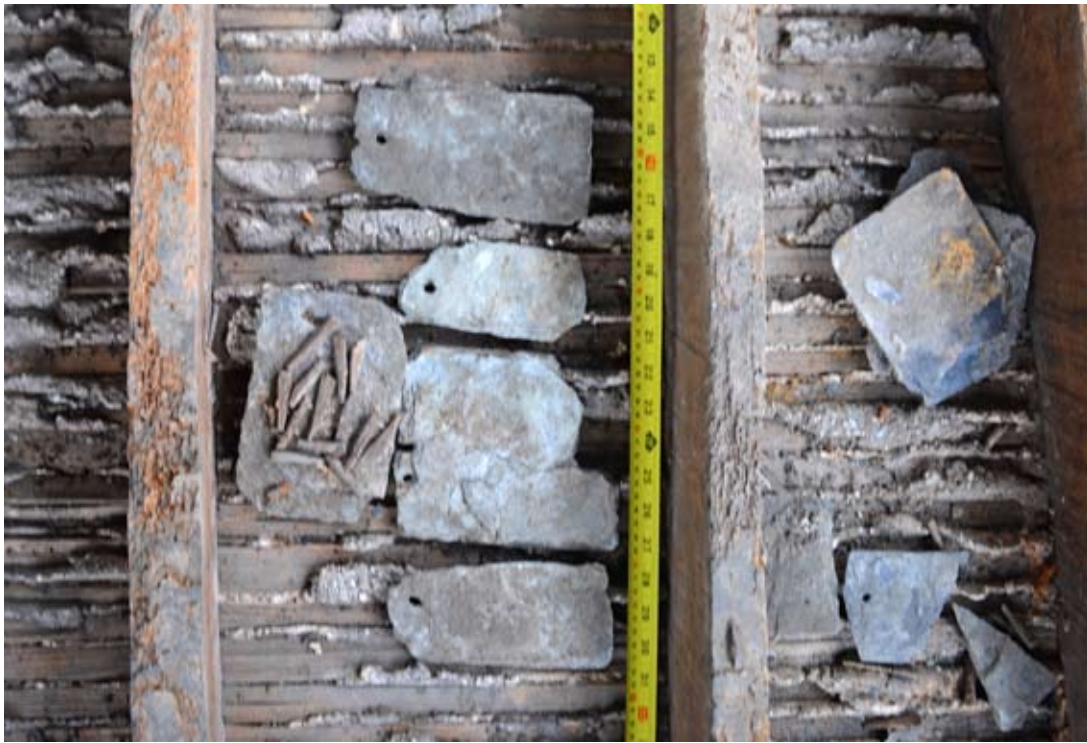
Some of the slates and pins in the roofspace of the south wing, 16.11.2012.
