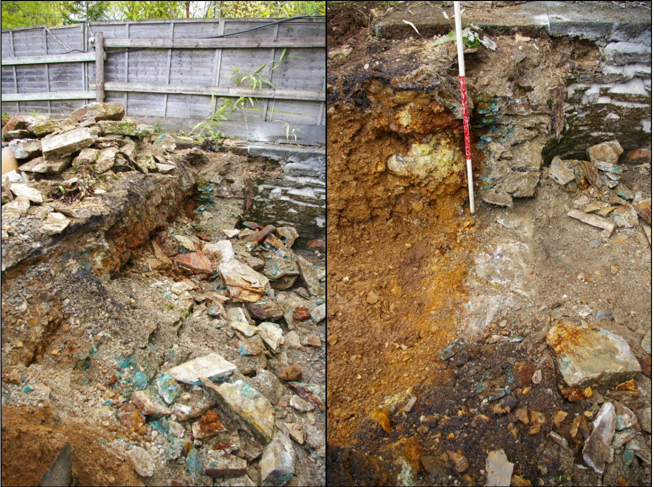
Figure 2: Left - is a shot during the demolition of the eastern portion of the retaining wall (note the copper staining), viewed from the south-west. Right - is the same area post-excavation, viewed from the south-west (2m scale).
