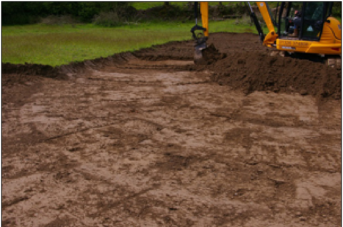
Figure 10: Working shot during topsoil strip in Field C, viewed from north (no scale).
