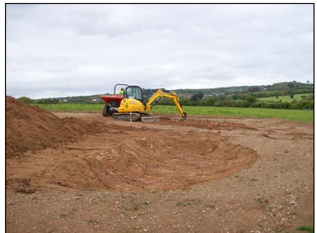
Figure 6: Field A post excavation of bunkers; viewed from the south-east (2m scale).
