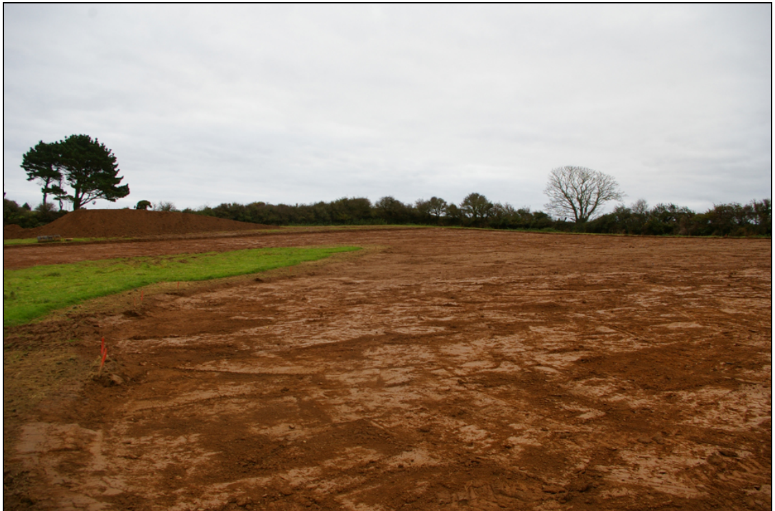
Figure 4: Area in Field A after the initial topsoil strip, viewed from the north-west (no scale).
