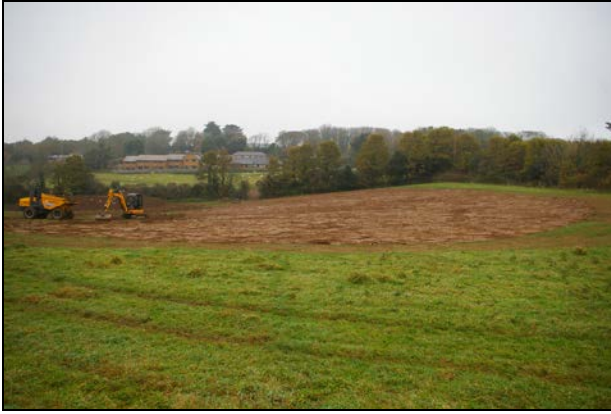
Figure 8: Area in Field B post topsoil strip, viewed from the south-west (no scale).
