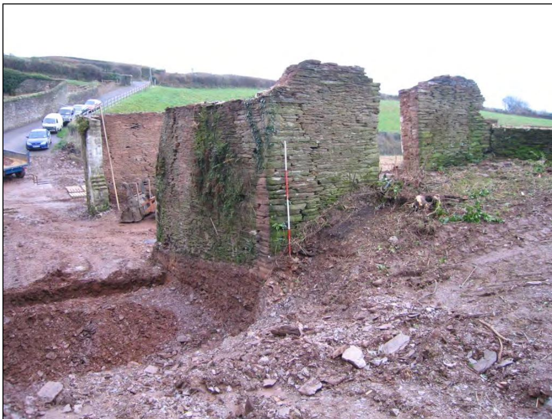
Figure 6: General view of Building A during works, viewed from the north-west (2m scale).
