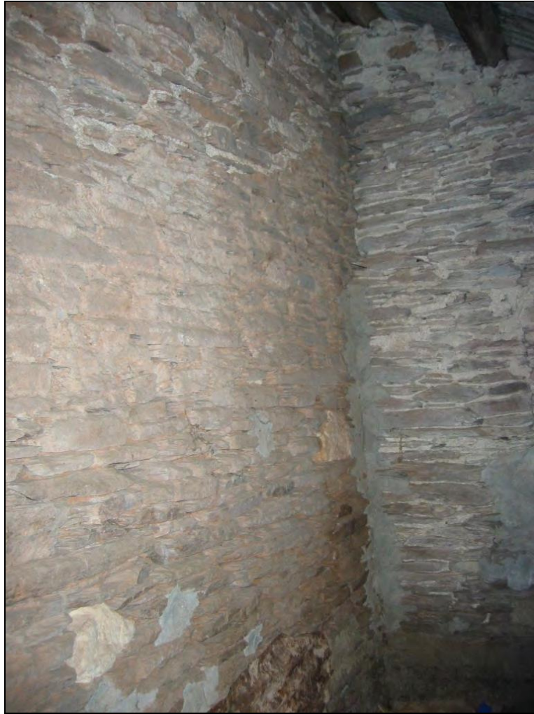
Figure 12: Shot of the south-west corner of Building F, with fragments of Beer stone mullion and centre-head visible in the southern elevation {227}.
