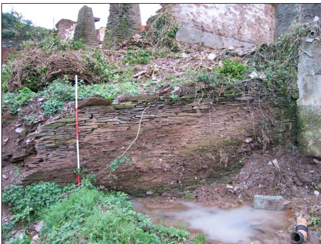
Figure 7: East facing pond wall {203} with Building 1 behind (buttresses {199} and {200} visible), viewed from the east (2m scale).
