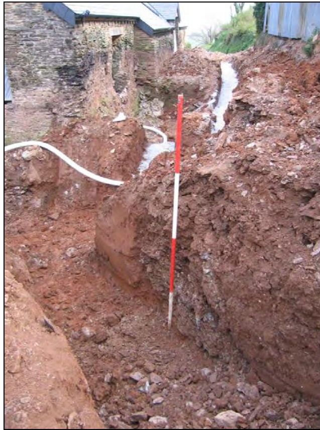
Figure 16: Shot of the lower end of Pipe Trench 7 and Pit [224], viewed from the north (2m scale).
